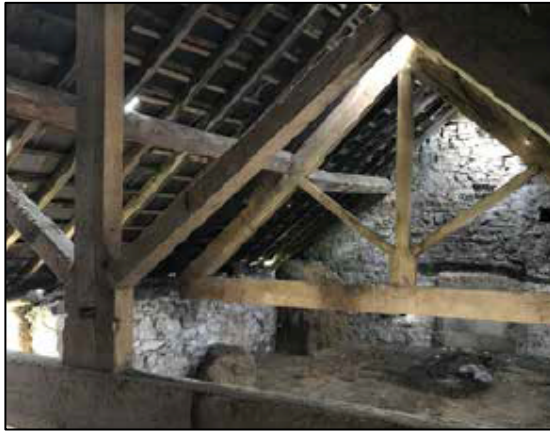
Plate 11. Detail of the hayloft with blocked in fireplace in the end wall and king-post roof construction.
