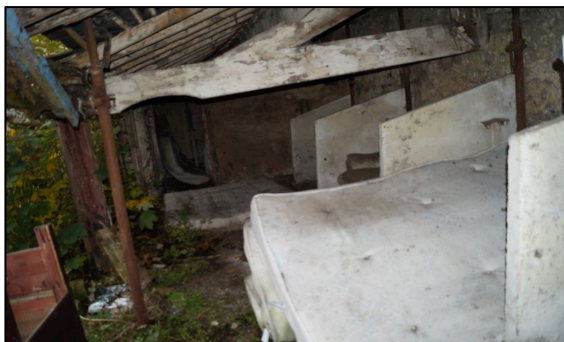
Plate 13. Interior of the ‘cart shed’ looking west showing concrete stalls, acrow props and reused ceiling timber.
