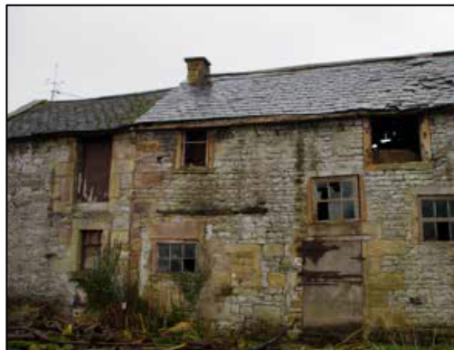
Plate 7. Front elevation of barn/cowhouse eastern half. The widened doorway for cows has a plywood stable door.
