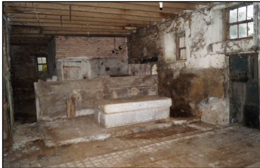
Plate 10. View across the cowhouse towards the brick built milking parlour. Tiled drainage channels are shown at the bottom of the photograph. Old mattresses have been discarded behind the stall divider.
