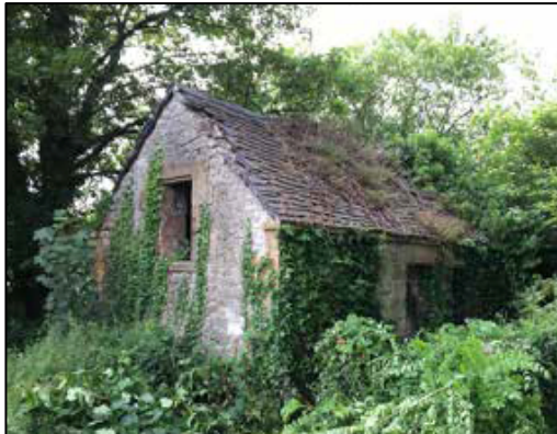
Plate 15. General view of the front and side elevations of the piggery showing opening to poultry loft and entrance to loose boxes.
