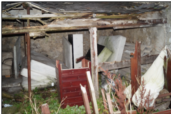
Plate 12. The front of the ‘cart shed’ showing two phases of construction and general condition of disrepair.
