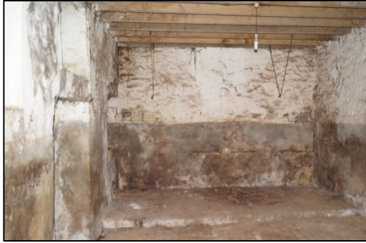
Plate 8. Interior of the barn showing location of Stalls and metal hangers for a suspended water pipe. The outline of water feeders can be traced on the far wall along with the truncated remains of metal stalls.
