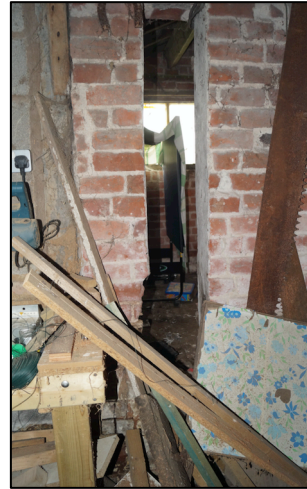
Plate 11. Slot in internal wall.
