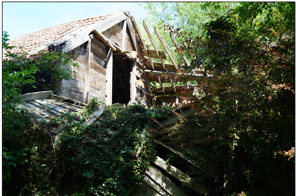
Plate 2. Collapsed end of former workshop.
