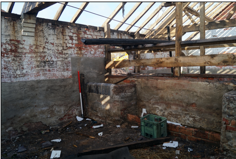
Plate 8. Interior of one of the cells with feeding troughs and tying up posts.
