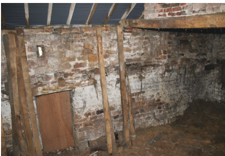
Oak posts (former joists) set aside. The sockets for the joists can still be seen in the masonry
