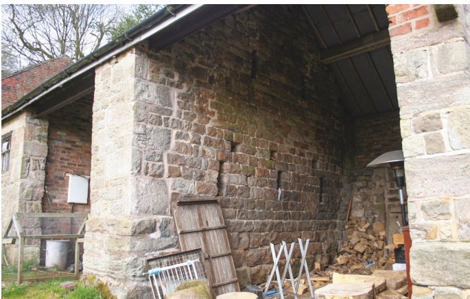
The former end wall of a late 17th century barn survives within the dividing wall of the 19th century cart bays
