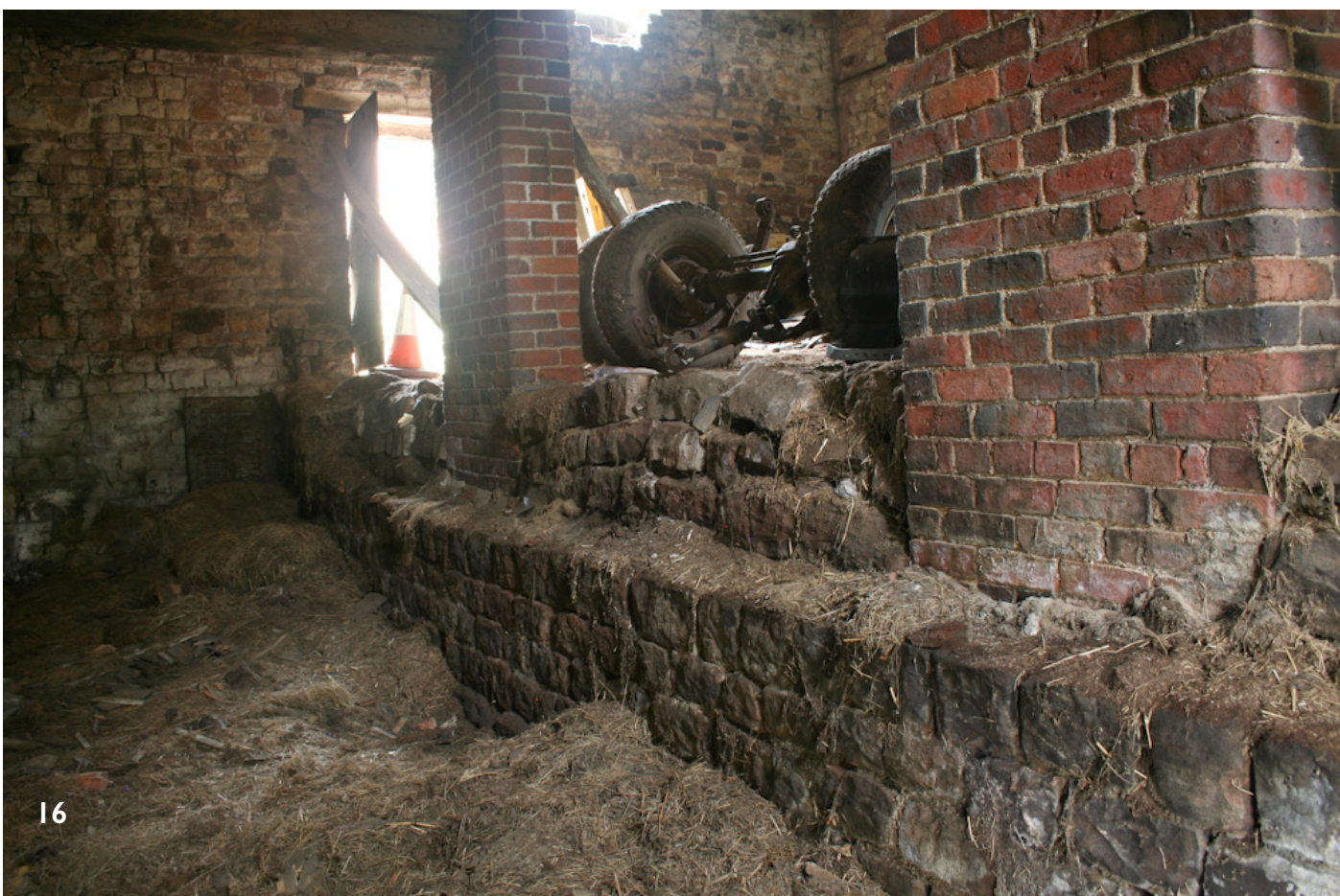
16 - Cowhouse looking south up into the large barn; the coursed stone plinth at the lower level supported the timber framework and the brick piers were inserted in the 19th century. Rubble stone infilled the gaps and the floor may have been re-laid.
