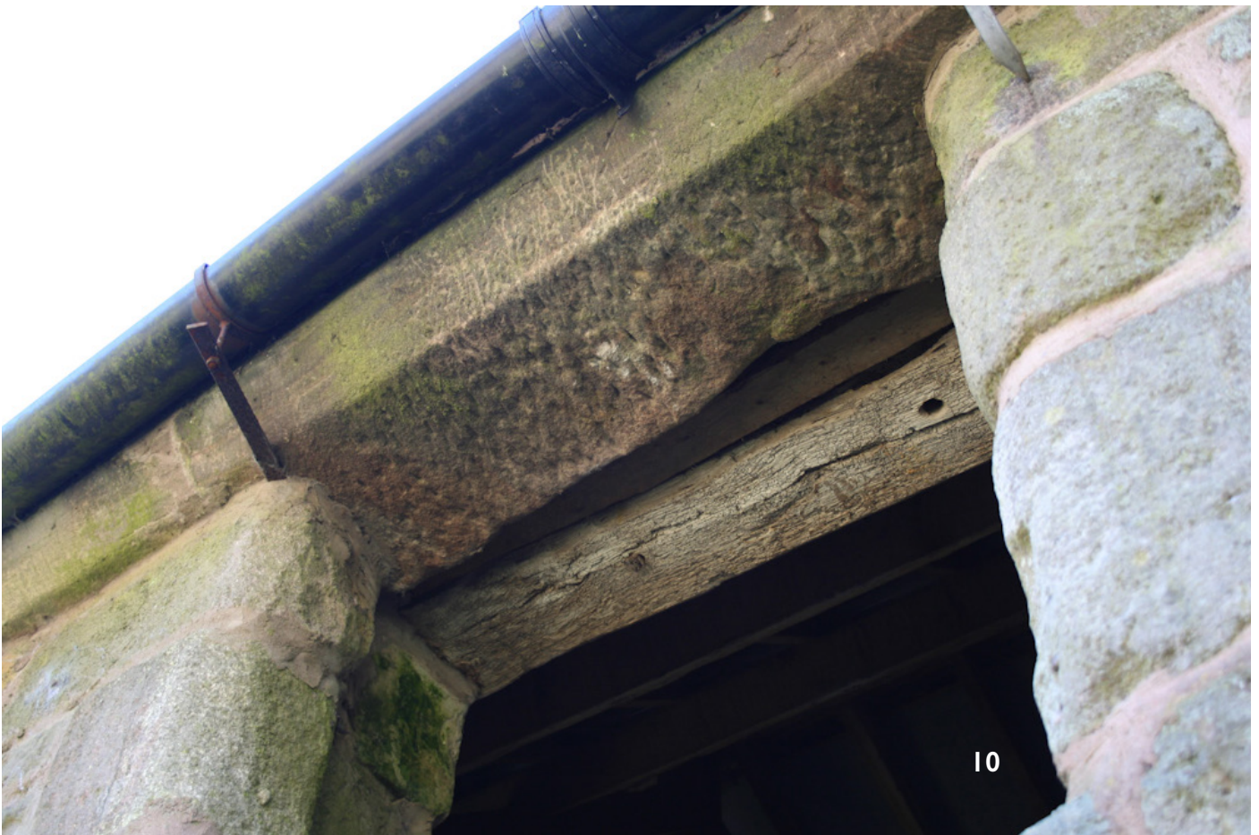
10 - stone eaves to threshing barn with weathered surround to pitching eye and oak lintel to inner wall
