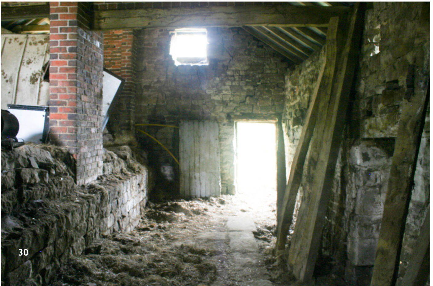
30 - view looking north through the cowhouse; manuring passage door and former mullioned window, and stone plinth, brick piers inserted to replace timber posts.
