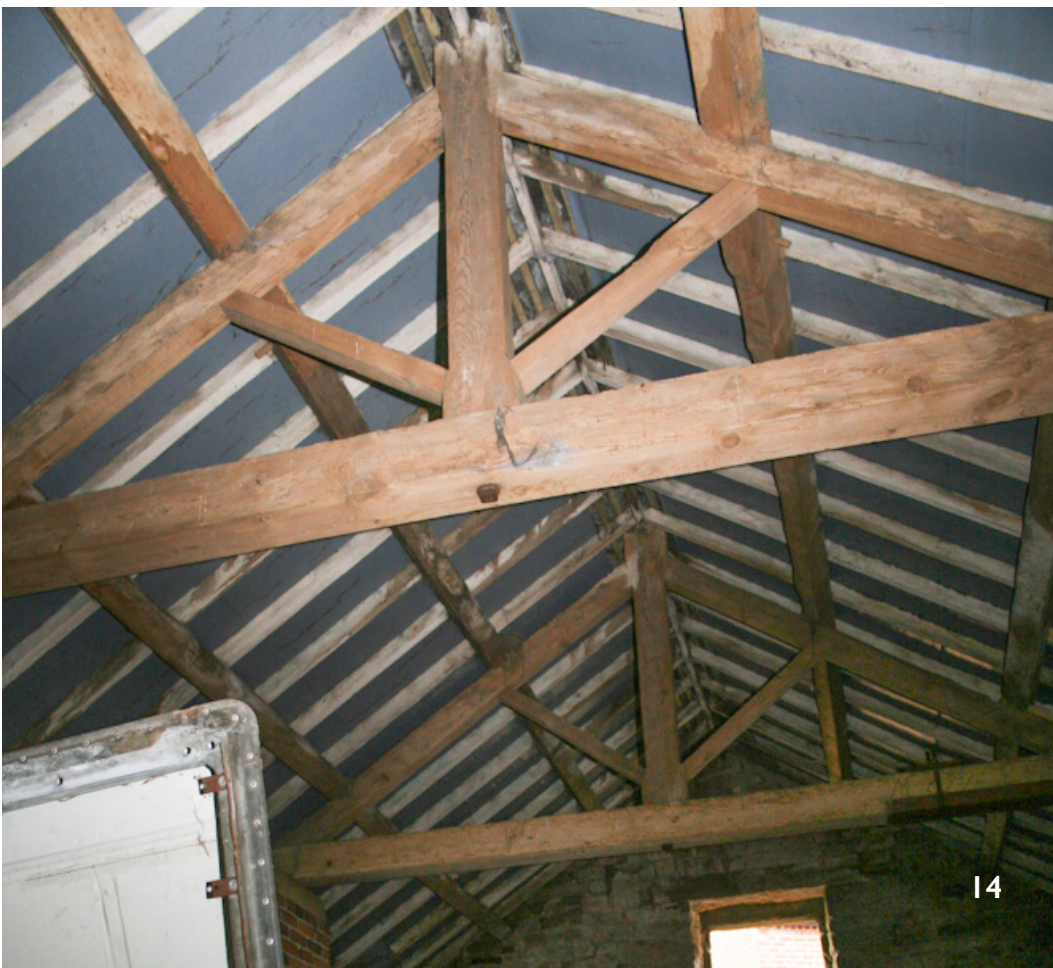
14 - king post trusses to the southern half of the Bank Barn, with double purlin roof construction, coach bolts through the tie beams and king posts and struts. All of the inserted roof is Scots pine.
