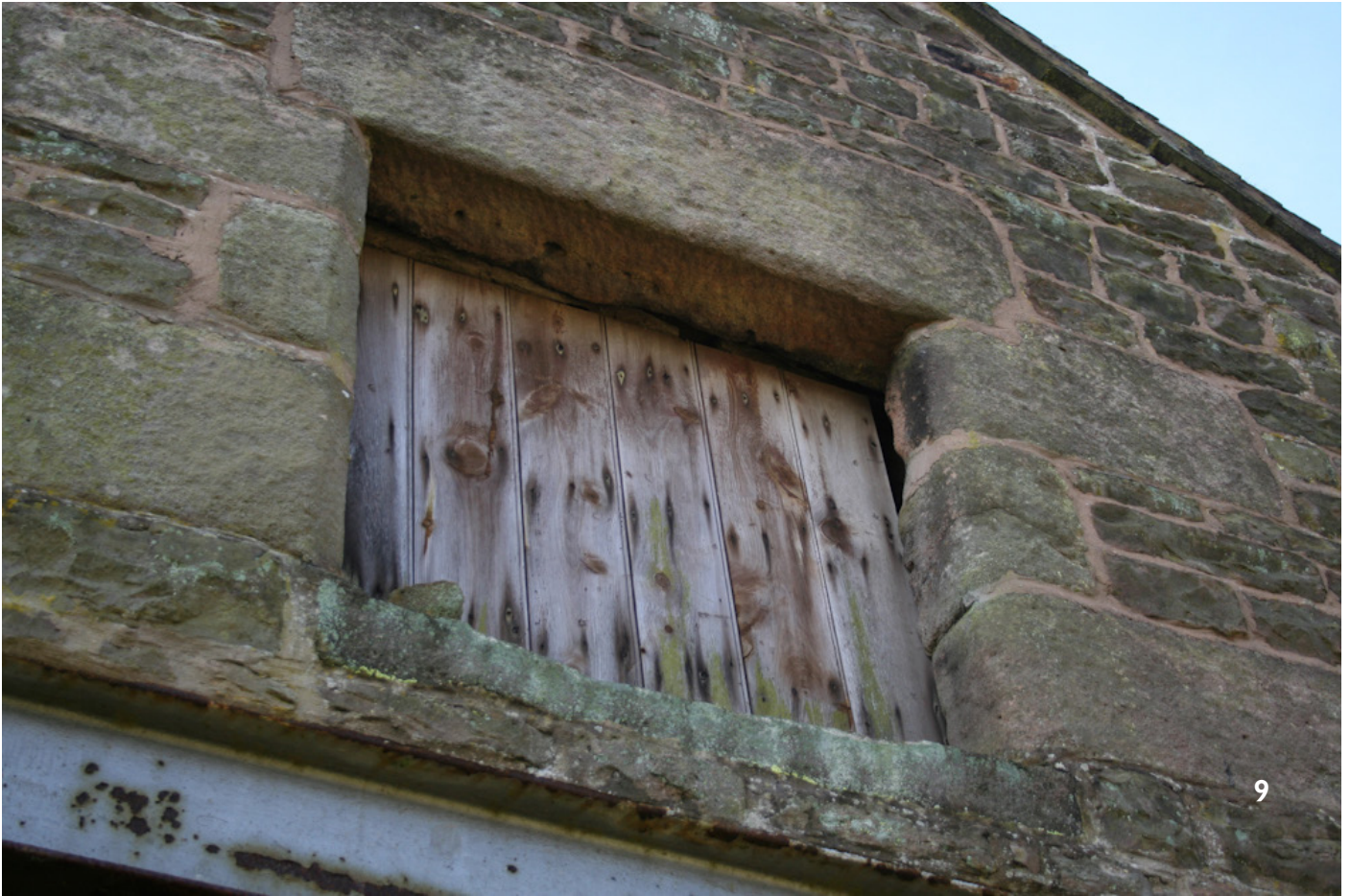
9 - Pitching eye to northern gable end, with chamfered surround, rebated stone masonry and shallow chamfered lintel, and heavily worn cill
