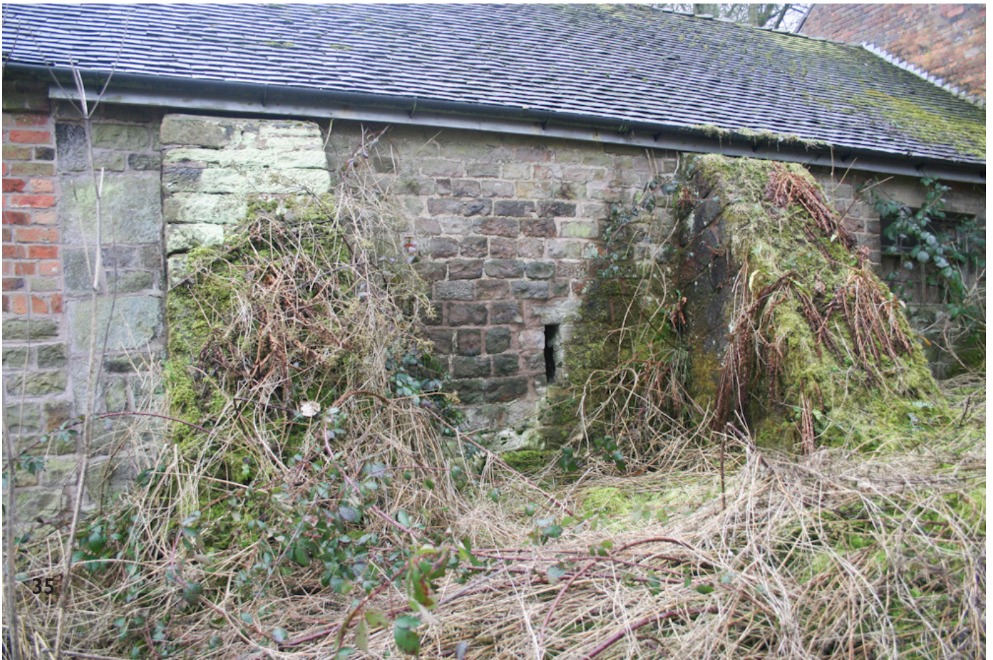
35 - North (rear) wall of barn to Stable Range. Ventilation slits, coursed sandstone with large irregular quoins, and later stone buttresses
