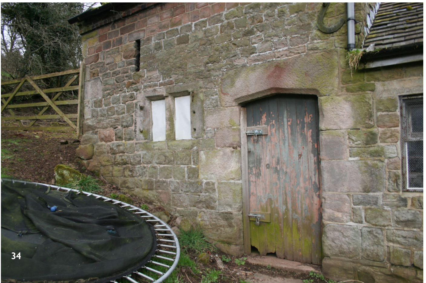
34 - Stable door with Tudor-arched doorway and small chamfered mullioned window. External shutters removed. The eaves were raised in three courses of pink coloured sandstone, with a corbelled brick eaves.
