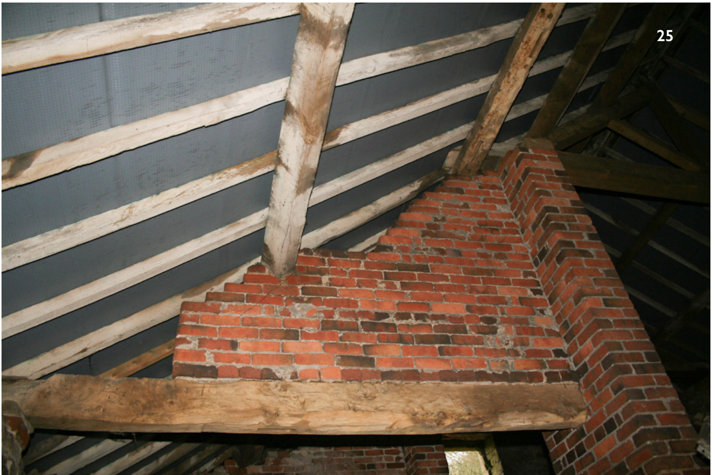
25 - re-used oak beam to the cowhouse, with inserted brickwork supporting the purlins, a 19th century alteration 26 - second re-used oak beam to the cowhouse, inserted 19th century brickwork
