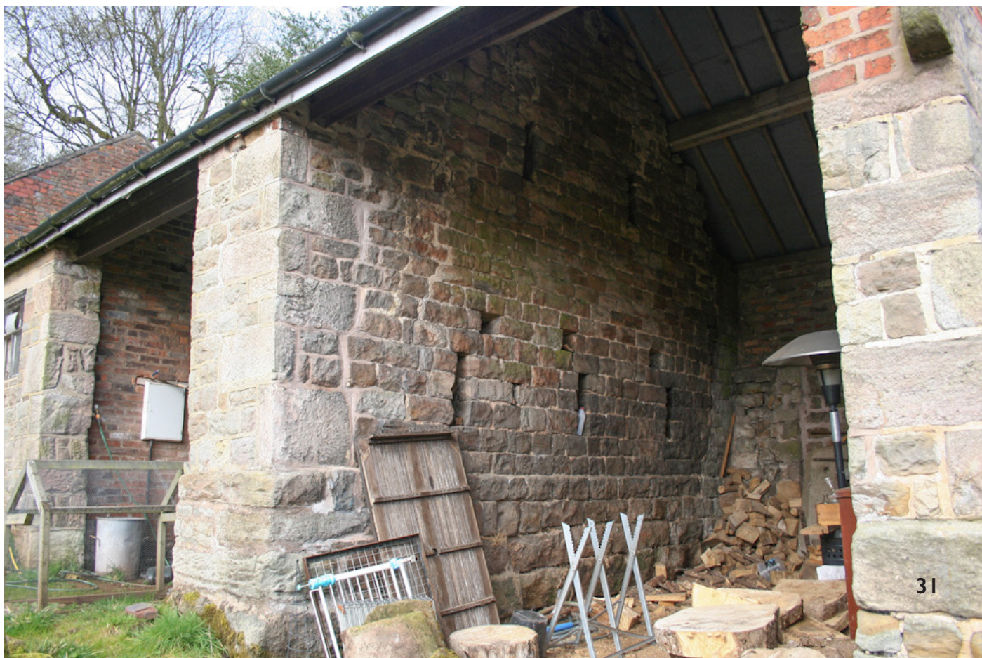
31 - Stable Range. View through cart entrance to former gable end of stone hay barn, with tiered ventilation slits, large masonry plinth, massive stone quoins.
