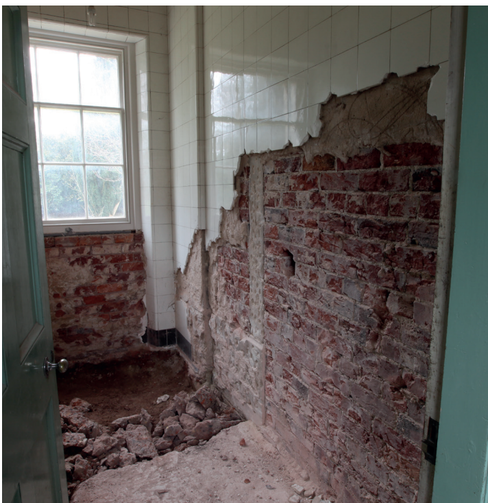
Removal of tiles within the 1851 service wing in 2021 have revealed the masonry of the original tripartite window to the west elevation, as recorded in the 1844 Buckler drawing (photo MM - 19.3.21). The windows were removed and the openings bricked-up flush in 1851.
