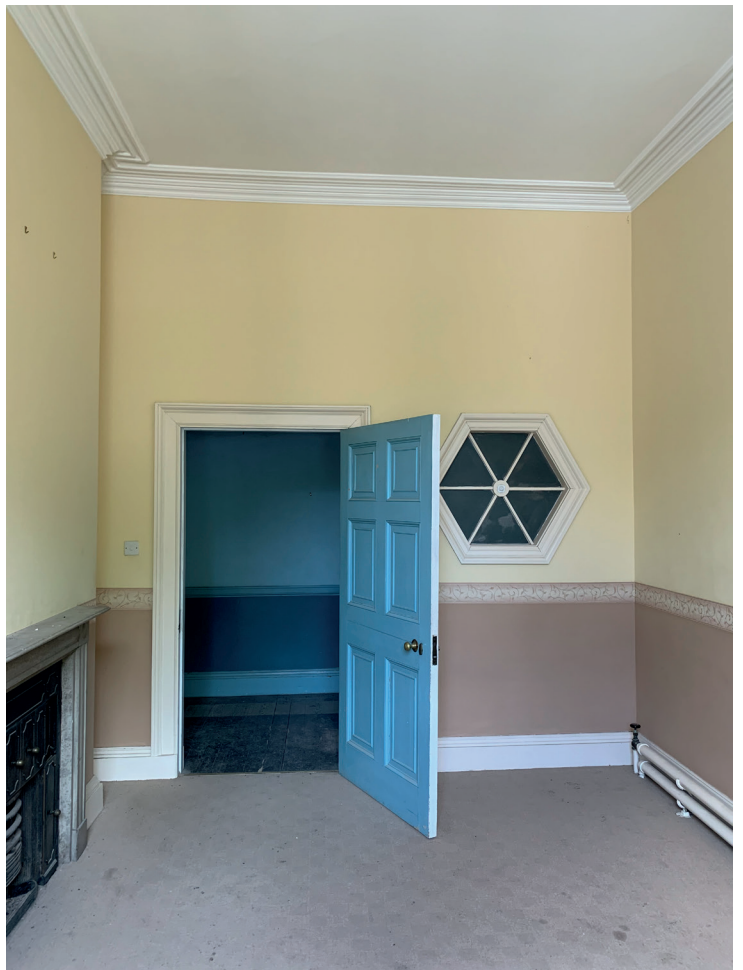
f12_002_14.05.20 Bedroom with small internal window and new partition, probably added in 1851 to light the corridor
