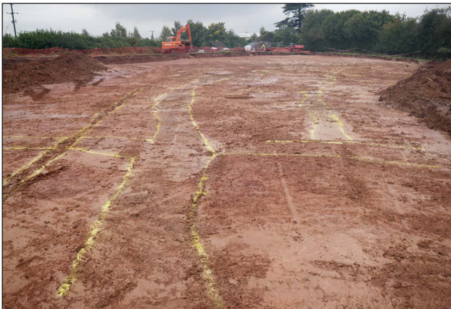
Plate 2: Pre-excavation shot of enclosure and field systems in Area A; view from east.
