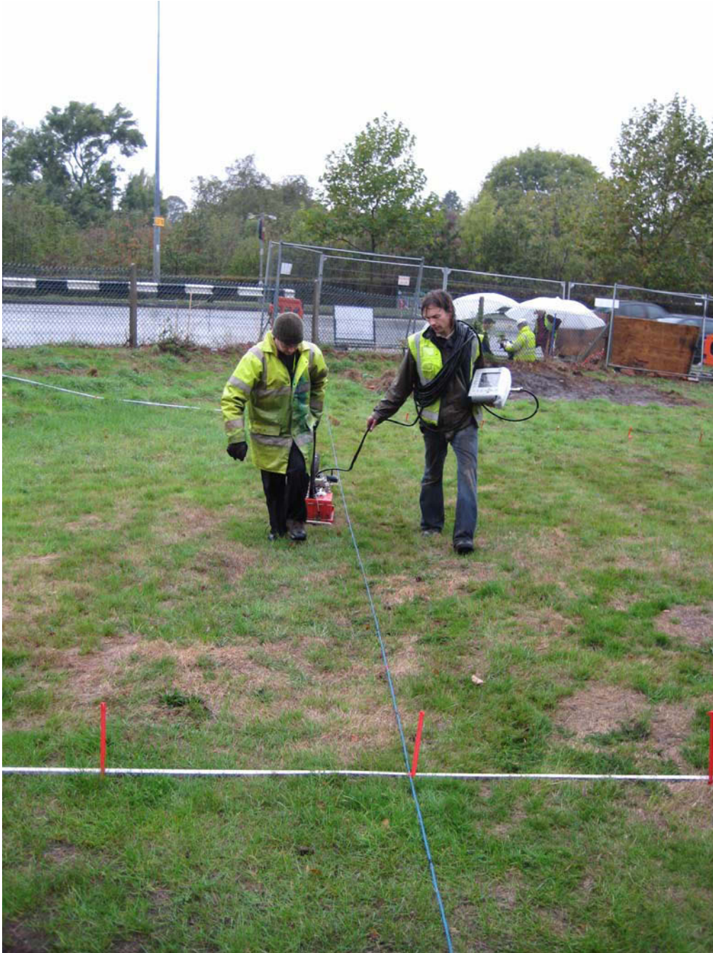
Fig 9 GPR survey in progress at the south end of the site (looking W towards Priory Crescent)
