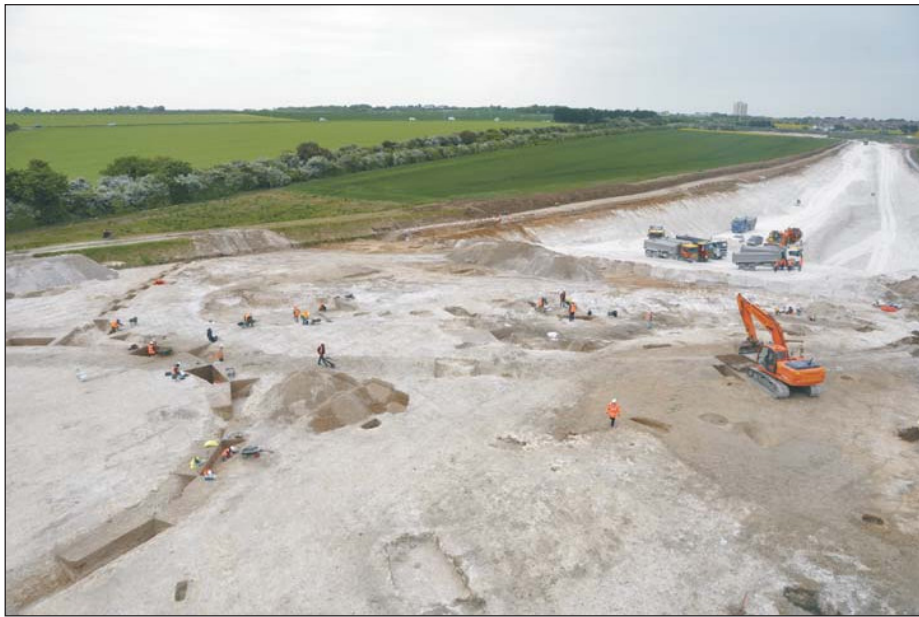
Plate 7: Zone 13: Excavation of Bronze Age and Iron Age features immediately ahead of construction works
