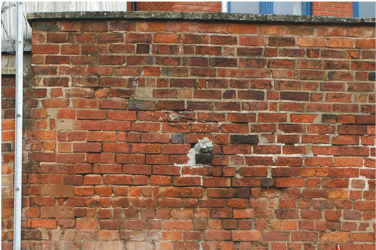
Plate 59: Building scar from roof of demolished structure Netherton Lane
