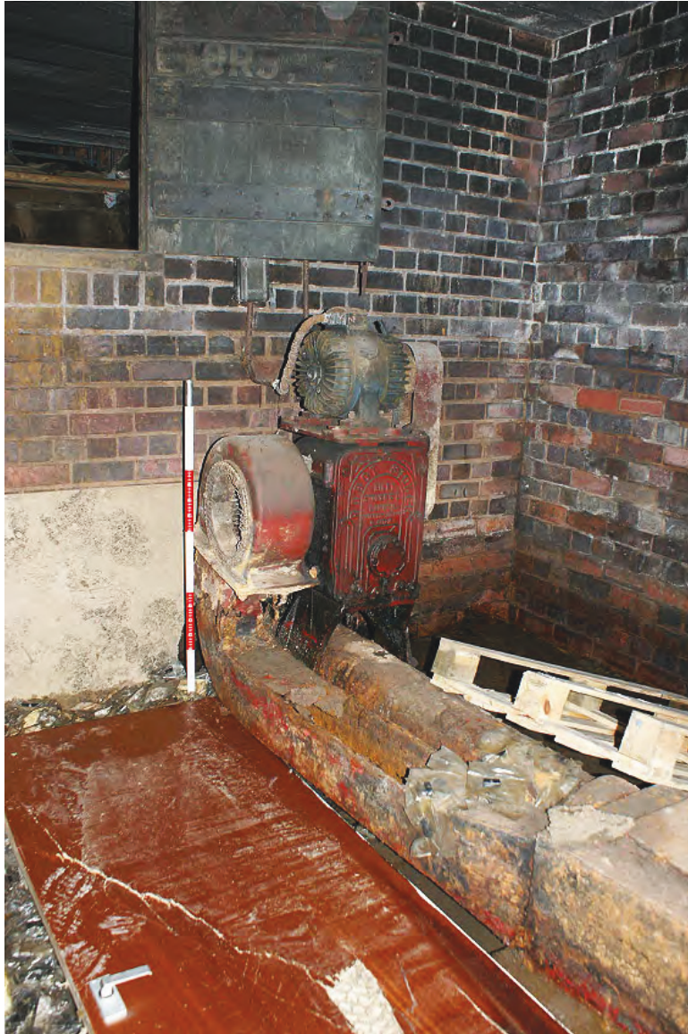
Plate 18 'Robot Stoker' and coal cellar hatch from the south
