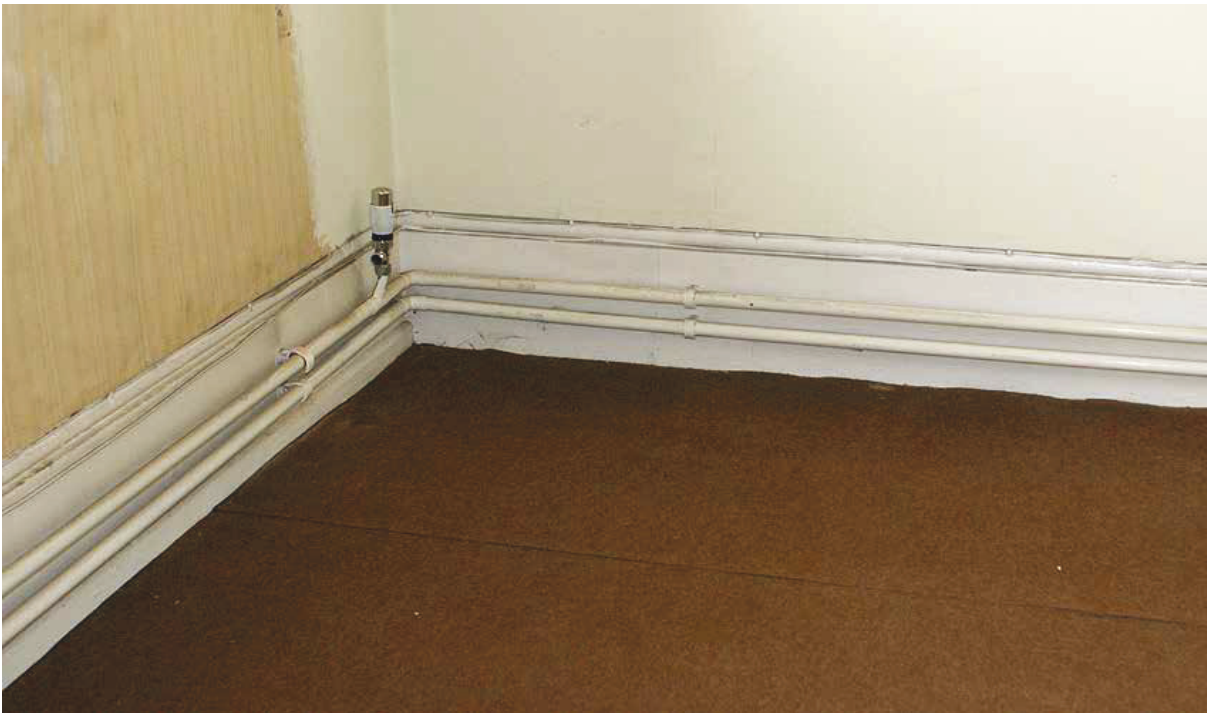
Plate 123: Example of roll beaded skirting, Room F1
