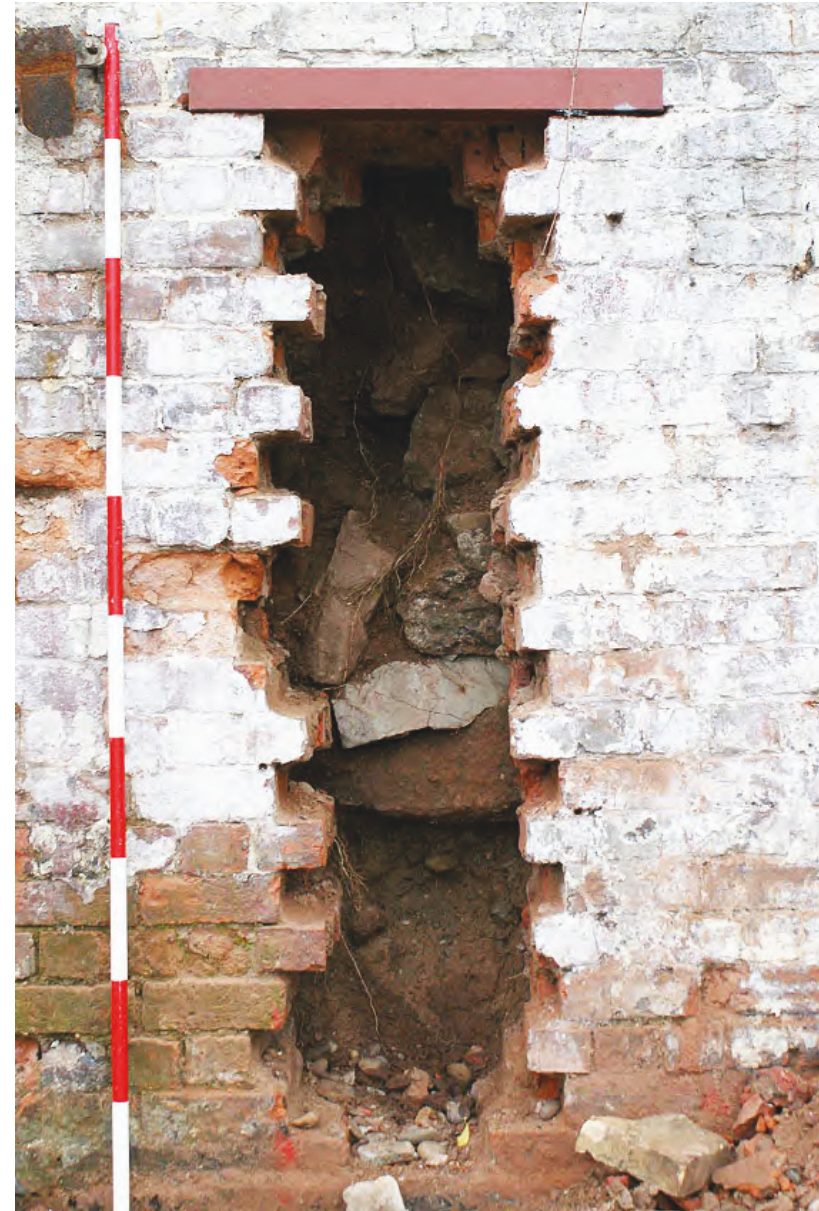
Plate 37 East side hole cut into city wall
