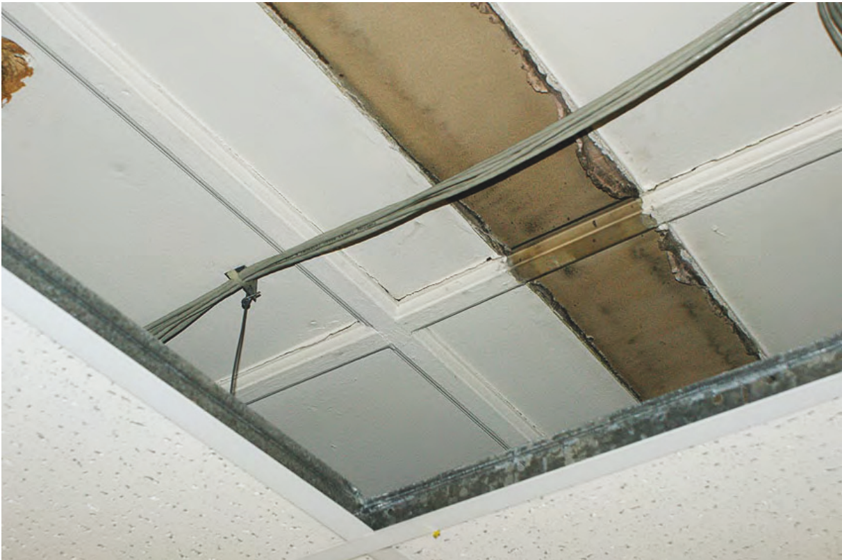
Plate 130: Ovolo moulded wood creating panelled ceiling, above later suspended ceiling, Room F10
