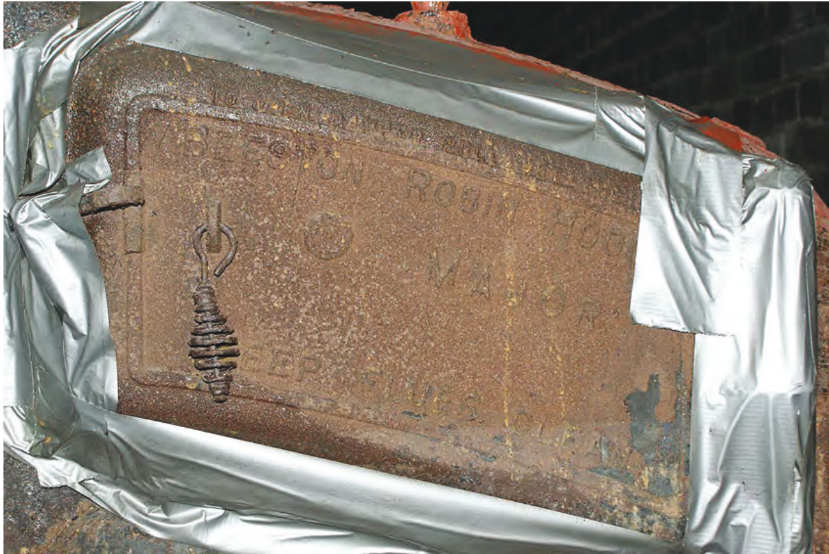
Plate 15: Beeston 'Robin Hood Major' boiler
