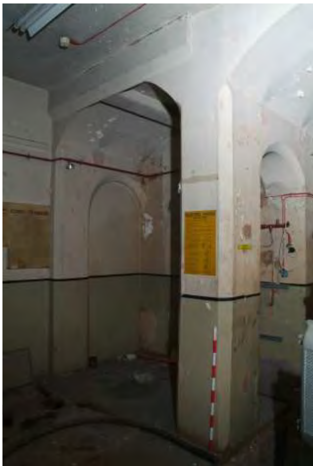
Plate 22.71: Building 22 (LGF): interior of the transformer room, view to the southeast
