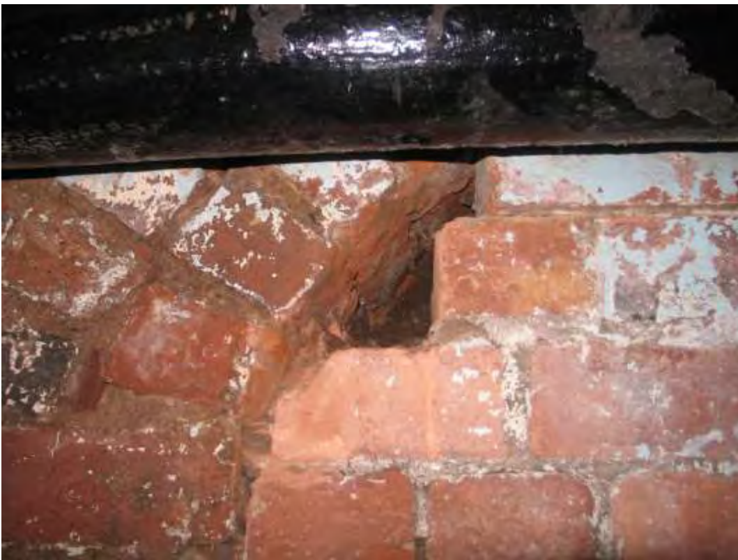
Plate 48.12: Building 48: basement – detail of brickwork following partial removal of blocking, view to the north
