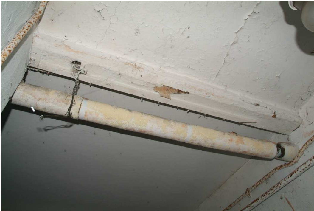
Plate 30.29: Building 30 (LGF): westernmost part of original basement showing remnants of service bell arrangement, view to the north
