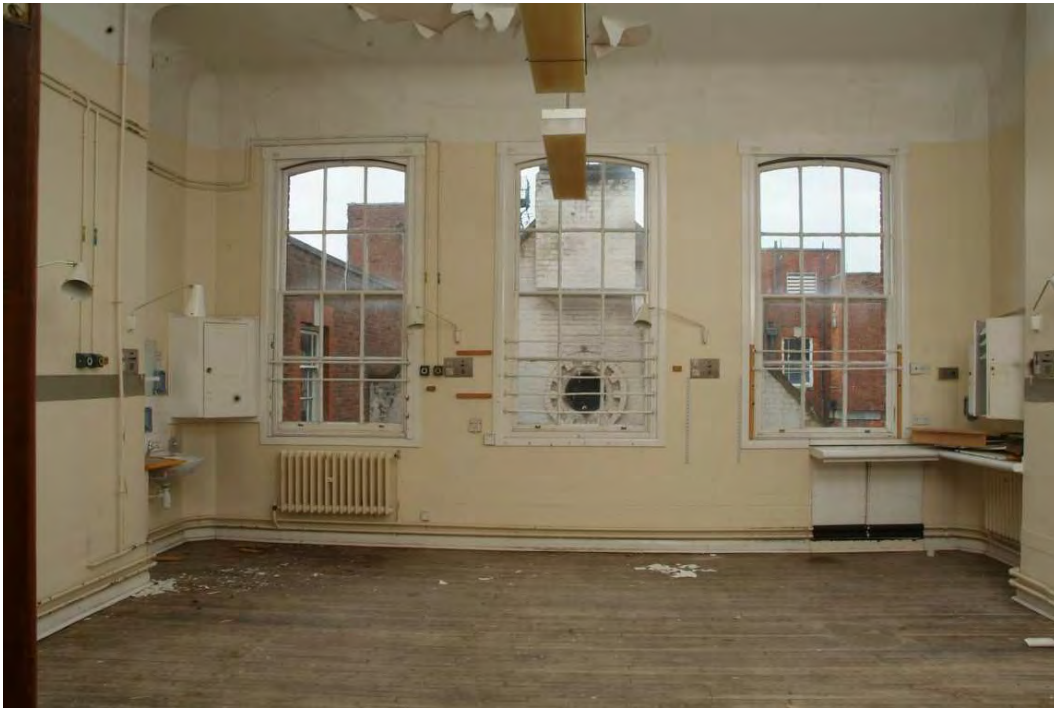
Plate 24.159: Building 24 (FF): ward [Room 2.22] over board room showing original windows in canted bay, view to the west
