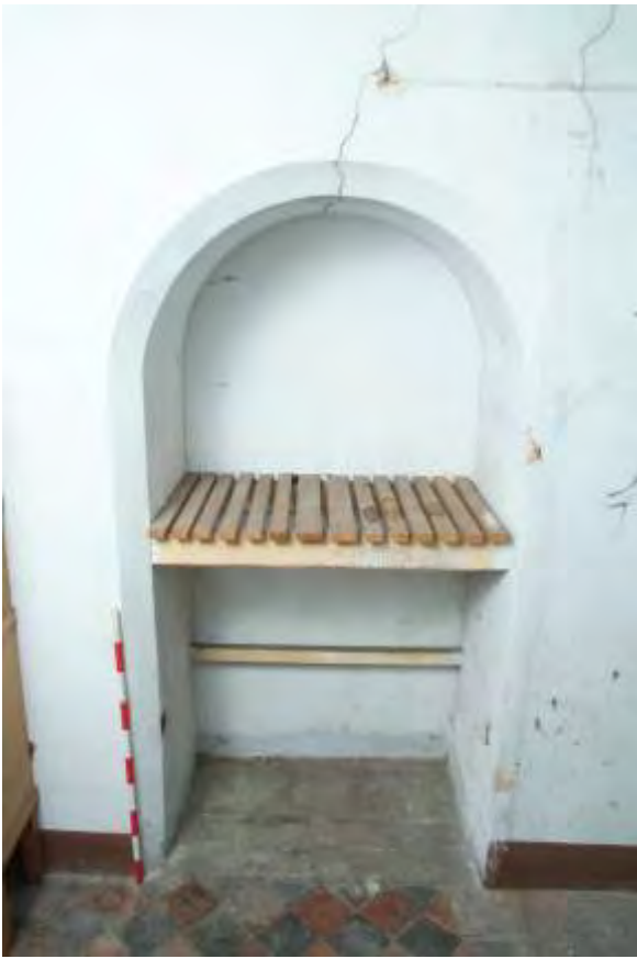
Plate 22.79: Building 22 (LGF): interior of apse showing former doorway from central aisle, view to the south
