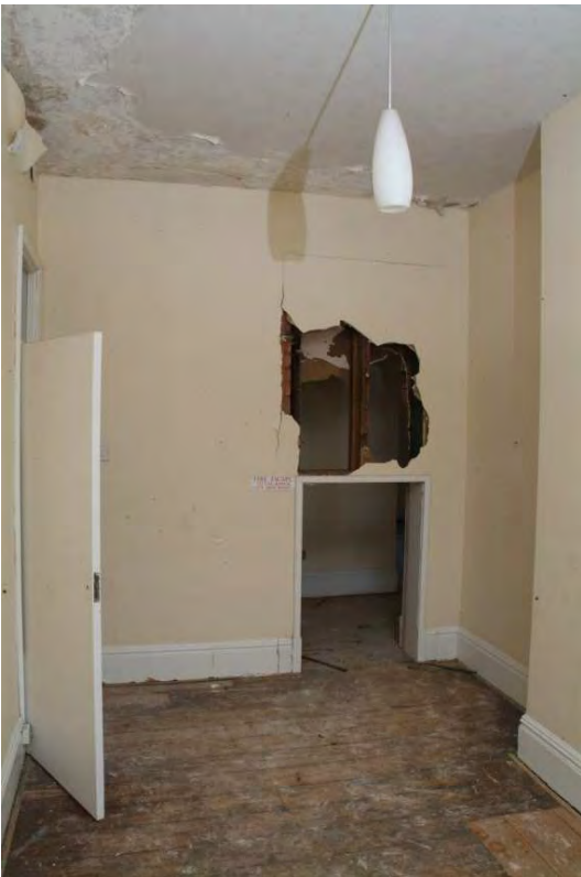
Plate 43.57: Building 43 - first floor: southernmost bedroom in central range showing fire escape in lower part of the original doorway, view to the east
