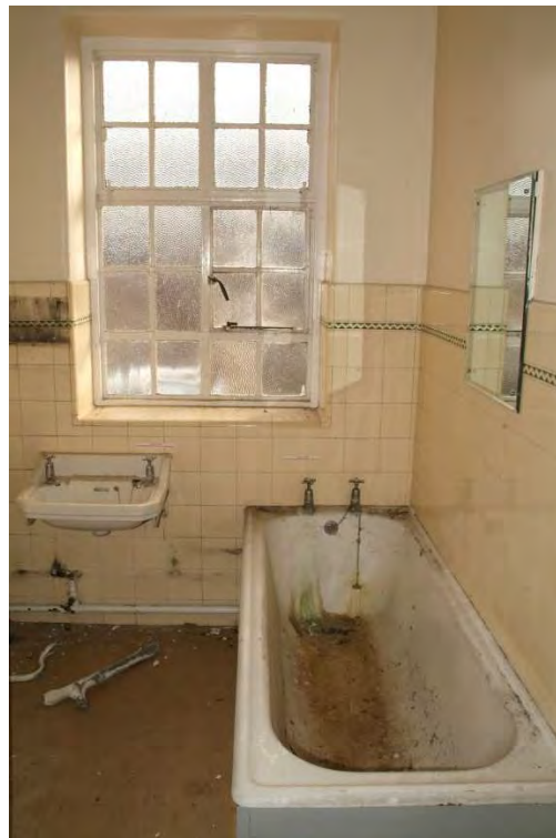
Plate 27.58: Building 27b – ground floor: original bathroom suite and tiling, view to the south
