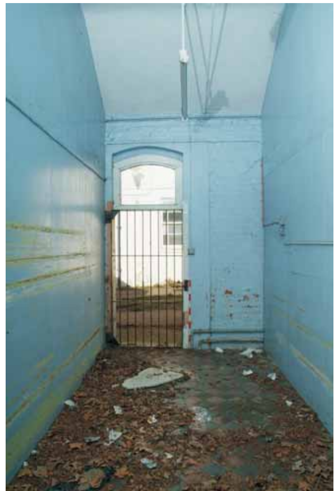
Plate 14.20: Building 14 – interior of room in east wing showing tiled floor, view to the north
