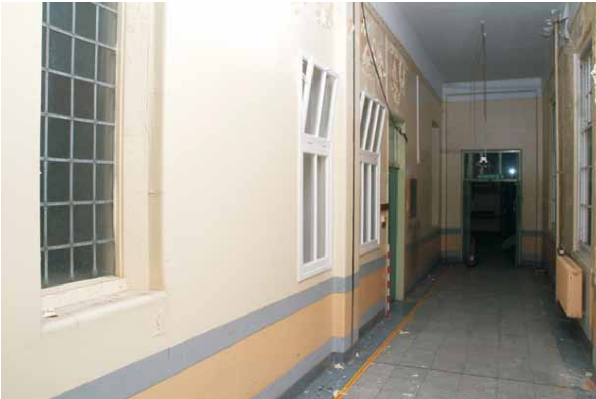
Plate 22.5: Building 22 – upper ground floor: later openings in former external southern elevation, view to the northeast
