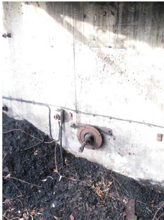
Plate 25.8: Buildings 25: apertures in lower part of boiler house southern elevation, view to the northwest
