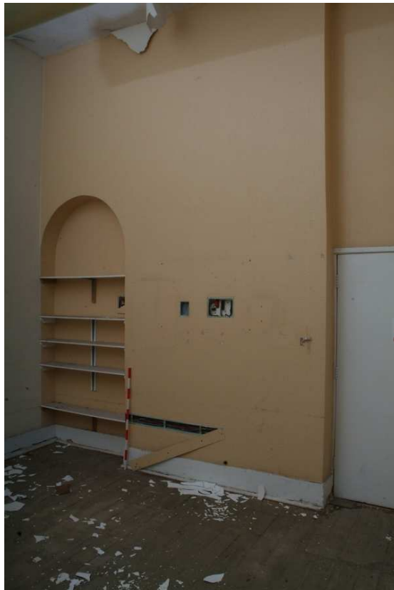
Plate 24.170: Building 24 (FF): interior of 'Relatives Room' showing blocked fireplace, view to the northwest
