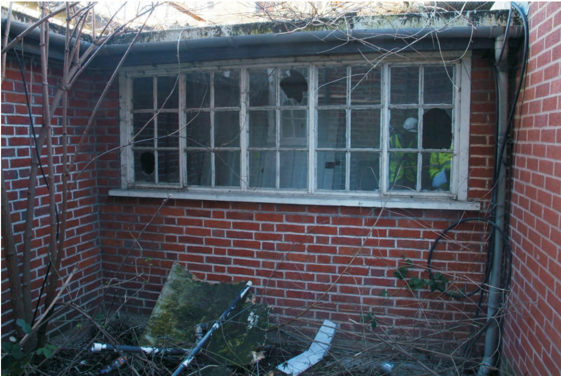
Plate 23.3: Building 23 - exposed southern elevation of the E - W corridor at the western end of the structure, view to the north
