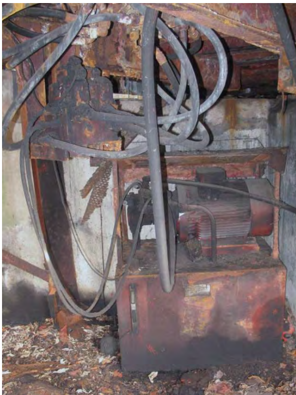
Plate 25.5: Building 25: hydraulic reservoir and pump beneath the conveyor, view to the east
