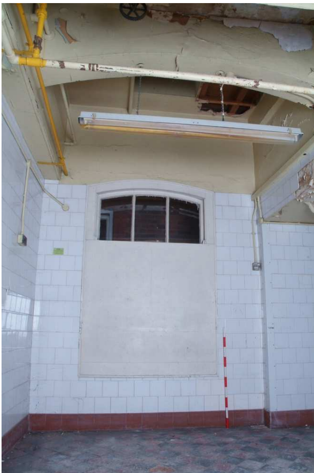
Plate 24.114: Building 24 (LGF): former side entrance to kitchens showing supporting arch for the closet wing, view to the north
