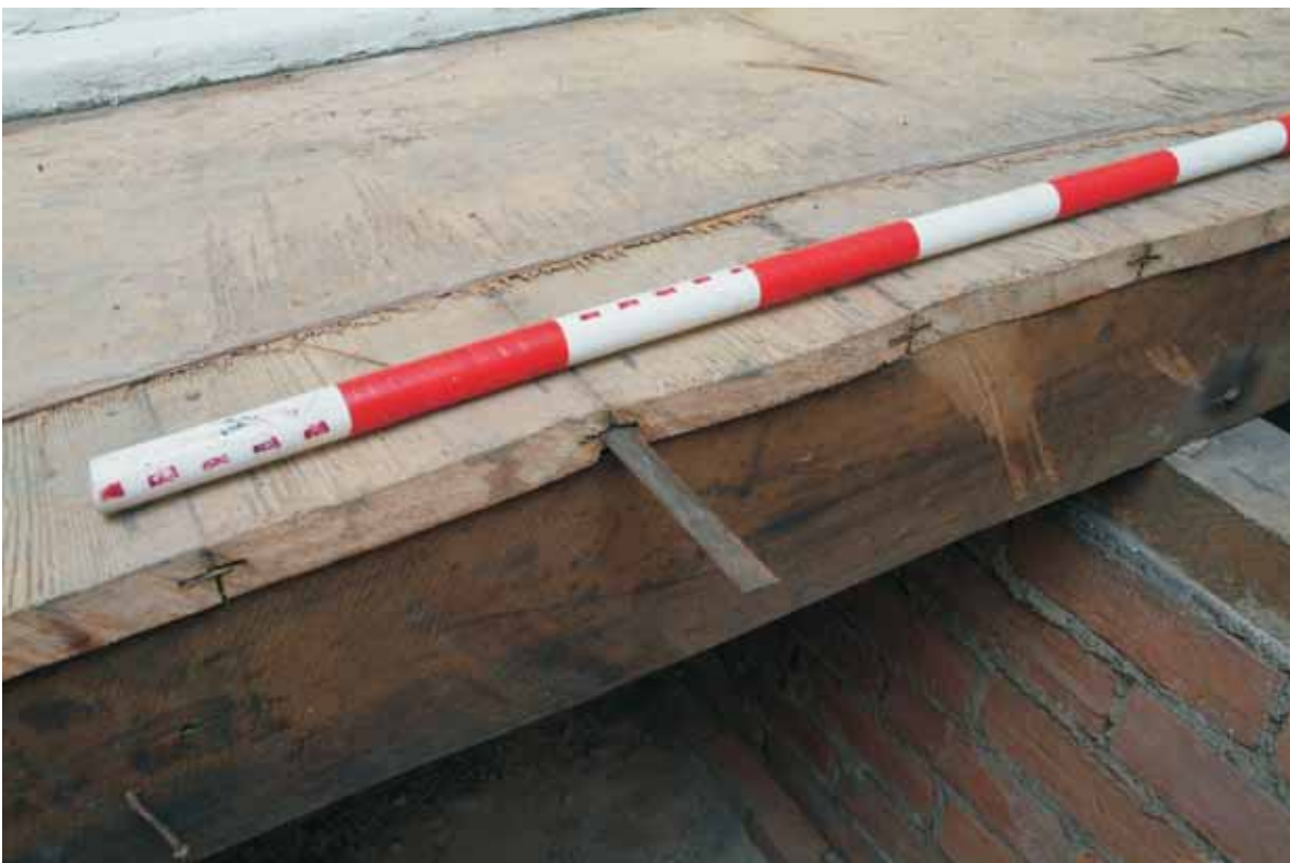
Plate 18.30: Building 18 – ground floor: detail of double grooved floorboards and metal fillet, view to the southeast
