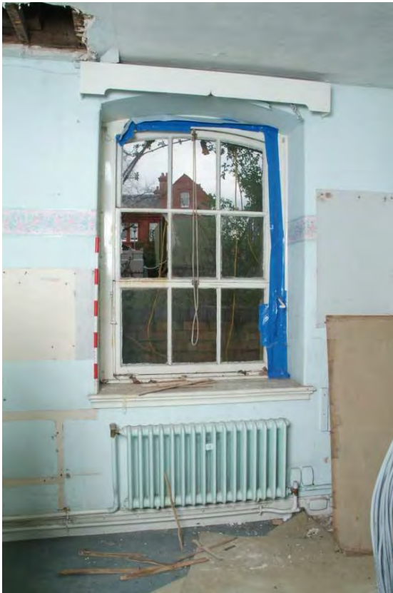
Plate 24.137: Building 24 (LGF): interior of office [Room 88] showing modified original window, view to the west
