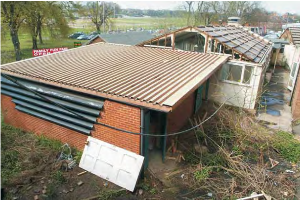
Plate 19.1: Building 19 – general view from first floor of building 18, view to the northwest
