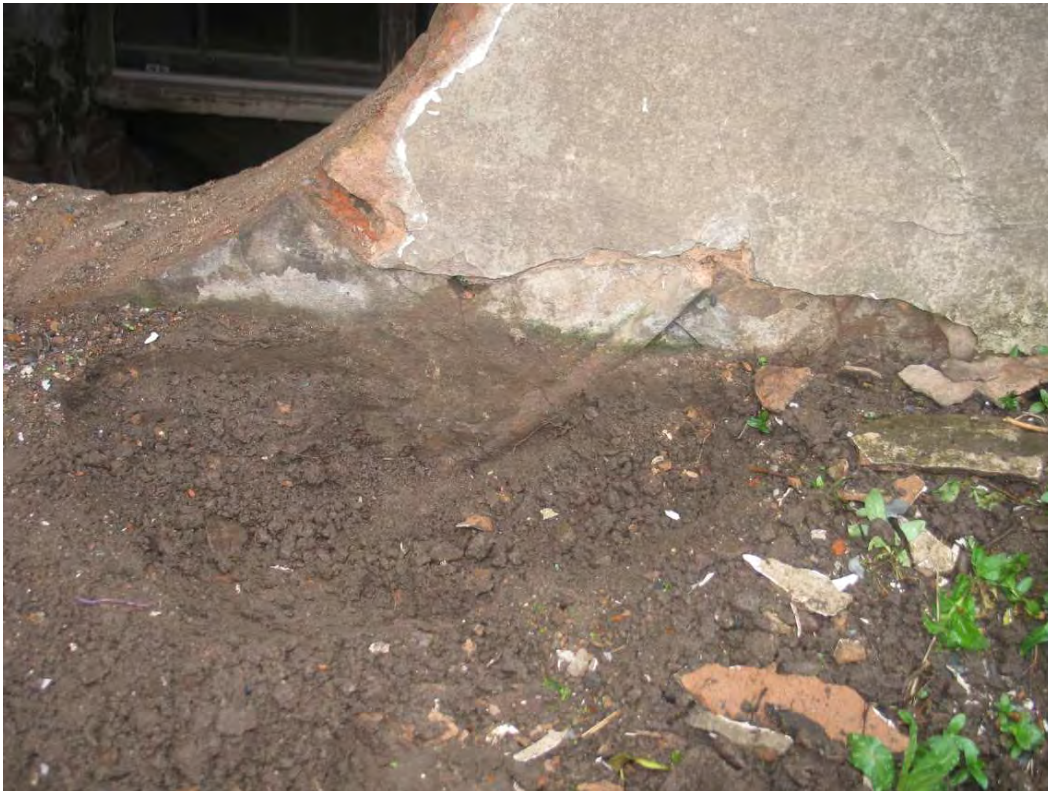
Plate 24.11: Building 24: detail showing surviving bead moulding around base of oculus, view to the southwest
