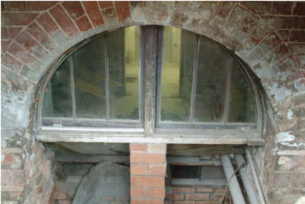
Plate 24.13: Building 24: enlarged opening through the infirmary wall beneath the central platform, view to the west
