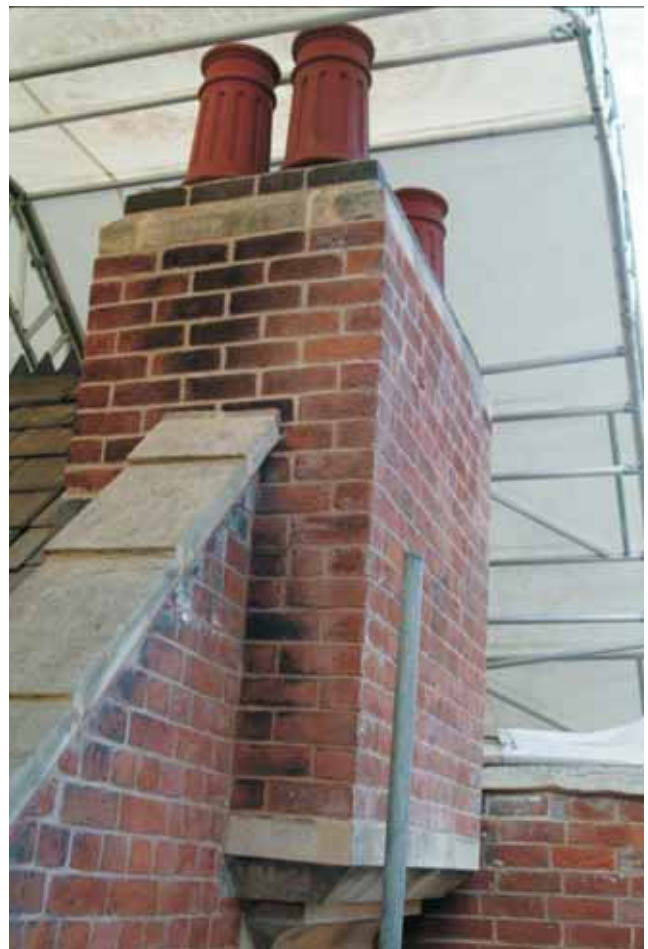
Plate 22.16: Building 22 – chimney stack at apex of east elevation, view to the northwest
