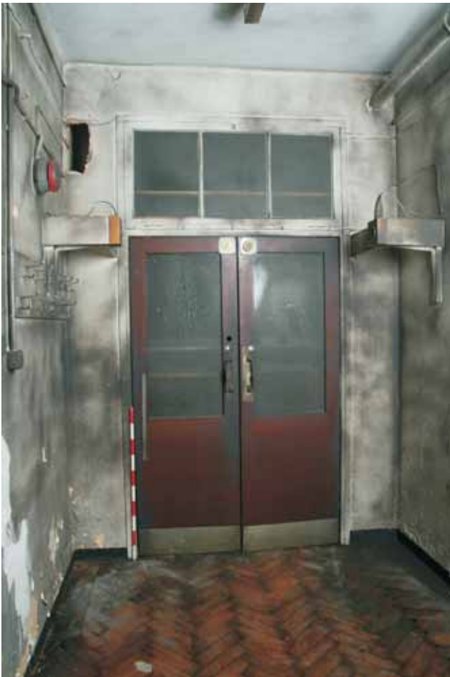
Plate 17.17: Building 17a – basement: 1938 swing doors within the central corridor, view to the south
