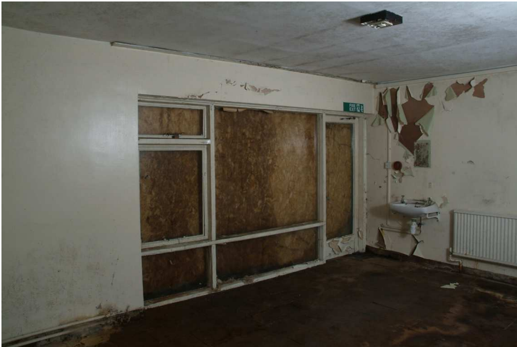
Plate 30.35: Building 30 (LGF): rear entrance to late 20th century extension, view to the southwest
