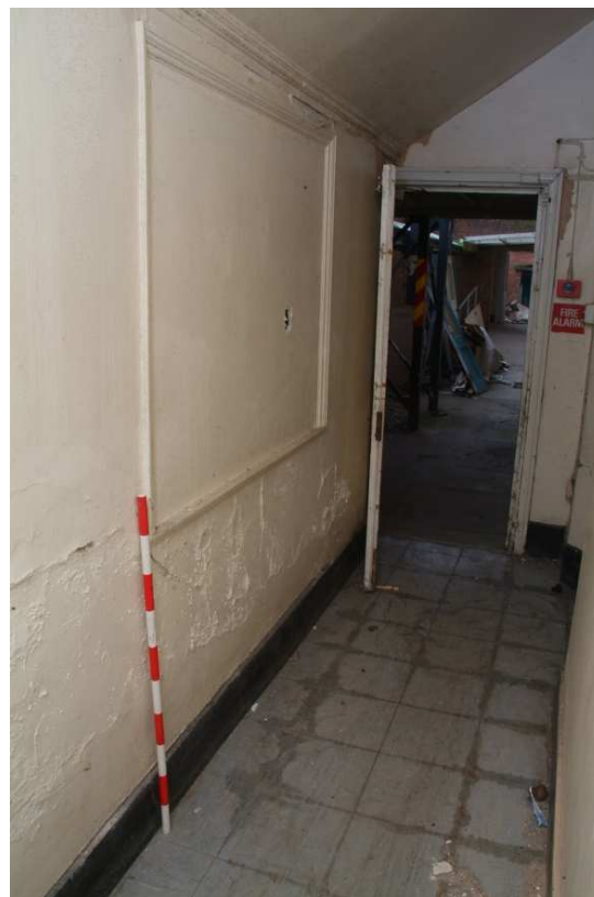
Plate 24.108: Building 24 (LGF): later lean-to corridor against southern elevation of Building 24f, view to the west
