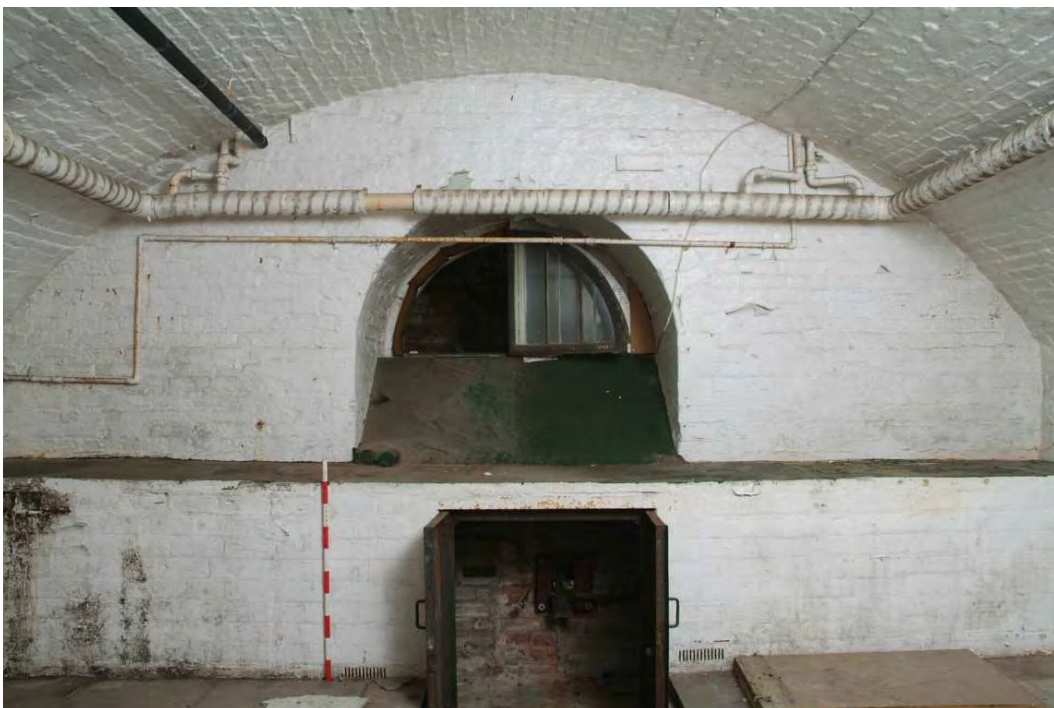
Plate 24.130: Building 24 (LGF): Room 89 showing inner conduit, view to the east
