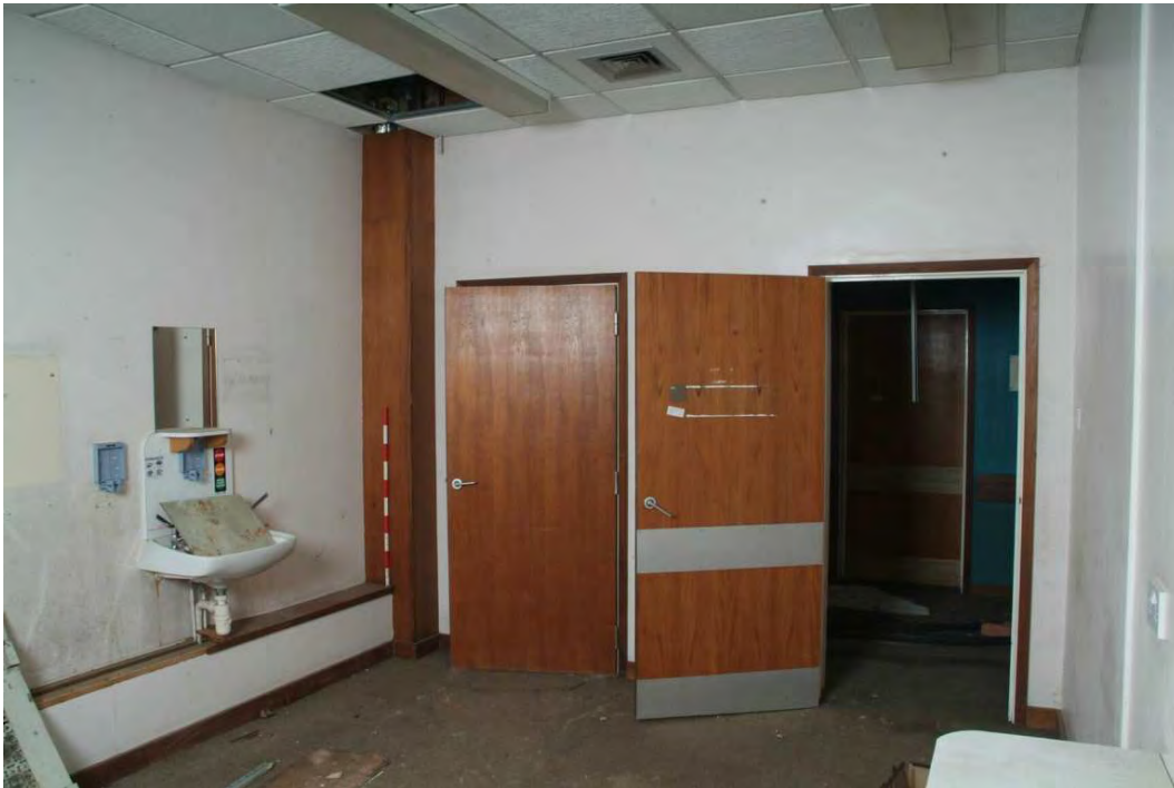
Plate 40.13: Building 40 (LGF): typical fittings [Room 0.24], view to the north
