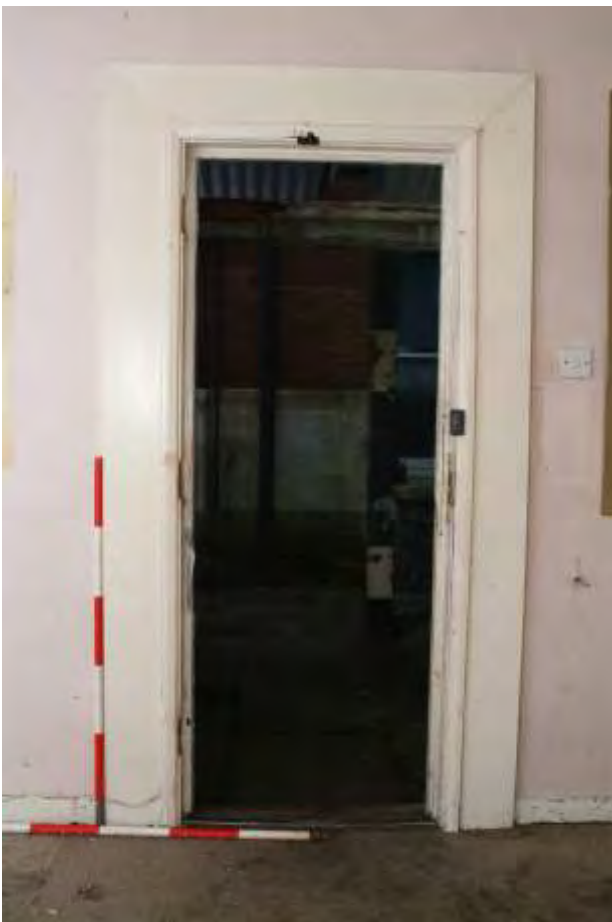
Plate 35.8: Building 35 – interior of eastern part showing architrave to entrance, view to the north
