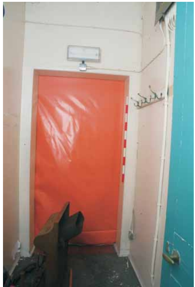
Plate 22.42: Building 22 – connecting range: north – south corridor on upper ground floor, view to the north
