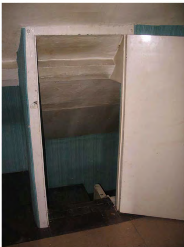
Plate 30.48: Building 30 (attic floor): early 20th century stair enclosure, view to the northeast
