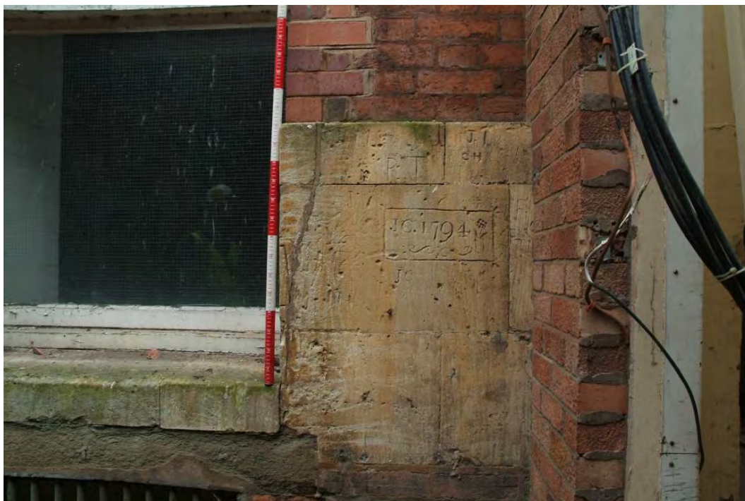
Plate 24.32: Building 24: southern elevation showing detail of graffiti on lower ground floor of original building (Building 24a)
