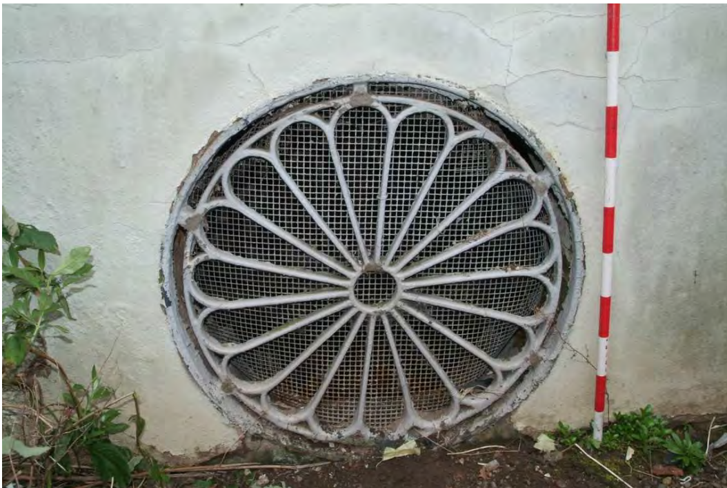
Plate 24.10: Building 24: detail of decorative grill across central oculus, view to the west
