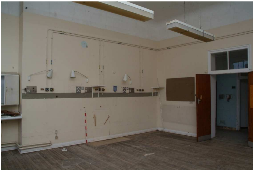
Plate 24.160: Building 24 (FF): north wall of ward [Room 2.22] showing blocked fireplace and typical remodelled doorway, view to the northeast
