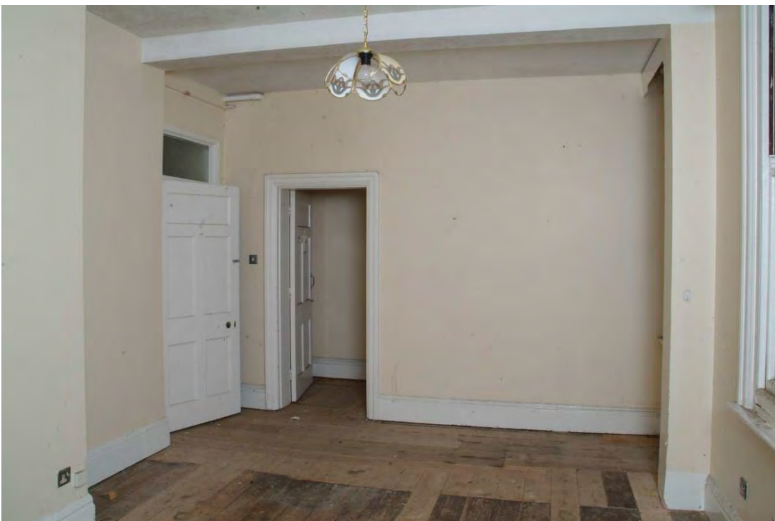
Plate 43.72: Building 43 - second floor: eastern room of southern range showing identical alterations to room below, view to the northwest
