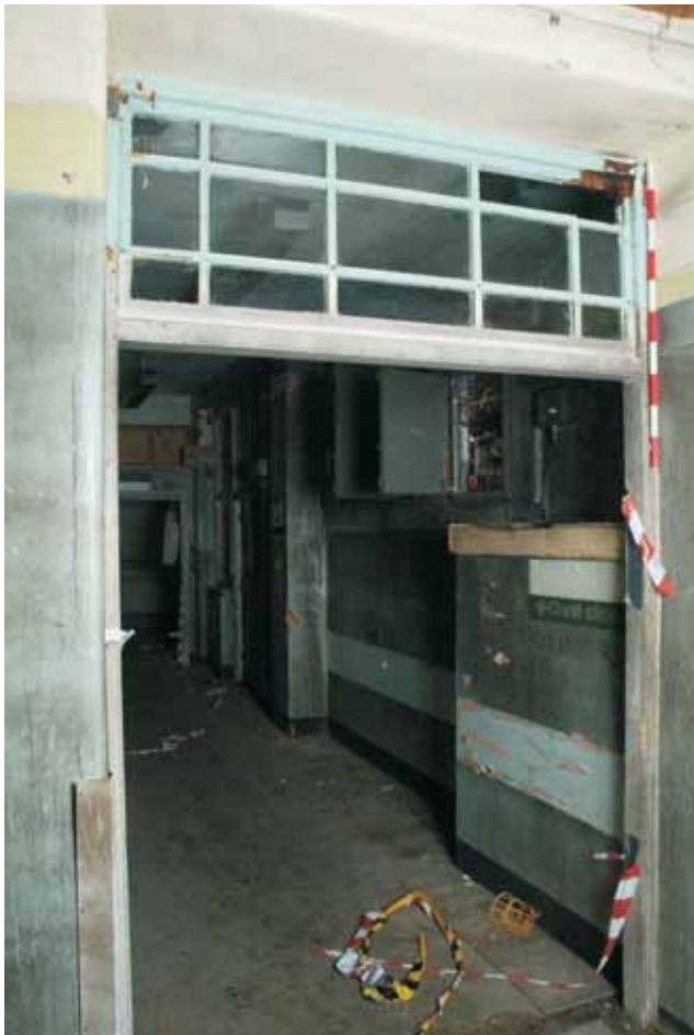
Plate 17.15: Building 17a – basement: 1938 doorcase and overhead at entrance to N-S link corridor, view to the northeast
