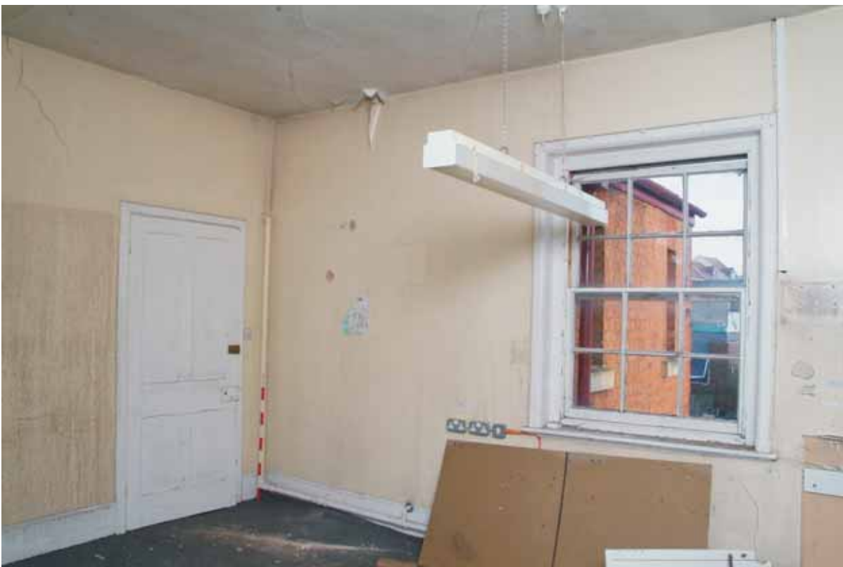
Plate 18.18: Building 18 – first floor: southeast corner of west ward showing location of former openings, view to the southeast
