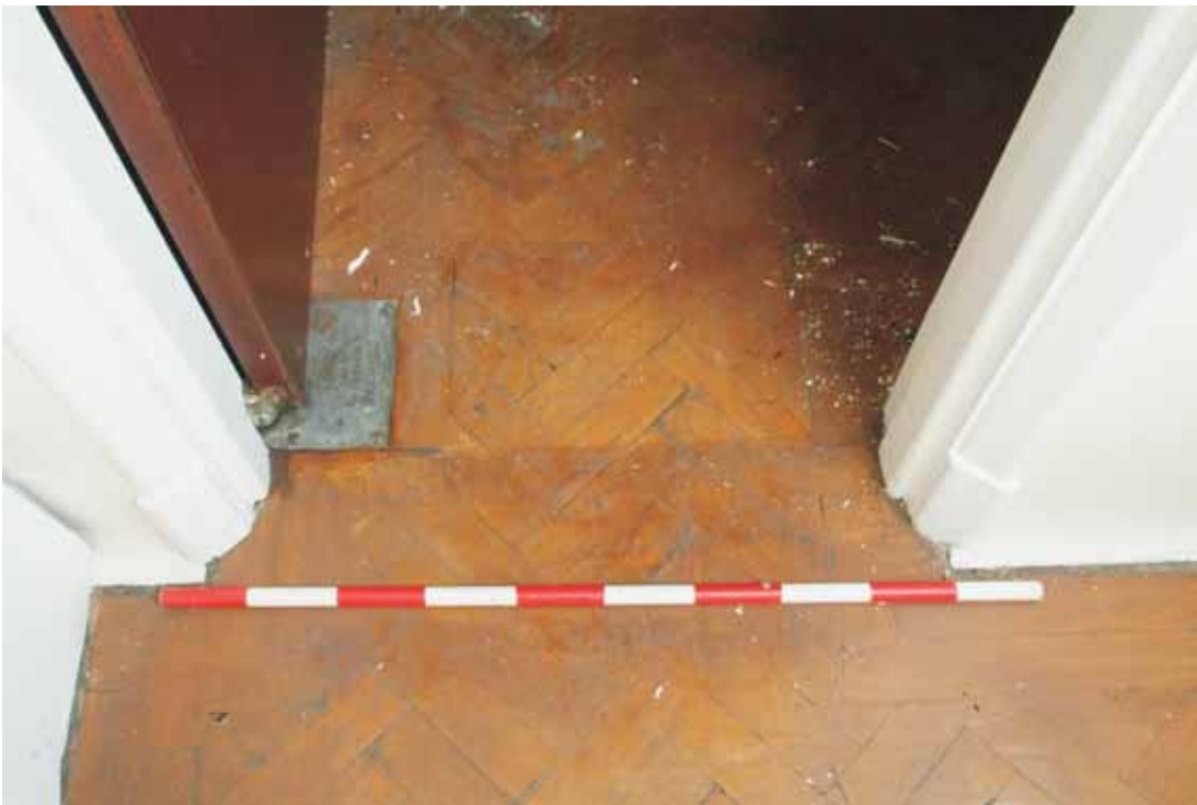
Plate 17.40: Building 17b – ground floor: floor and skirting detail at entrance to office within 1938 extension to 17b, view to the south
