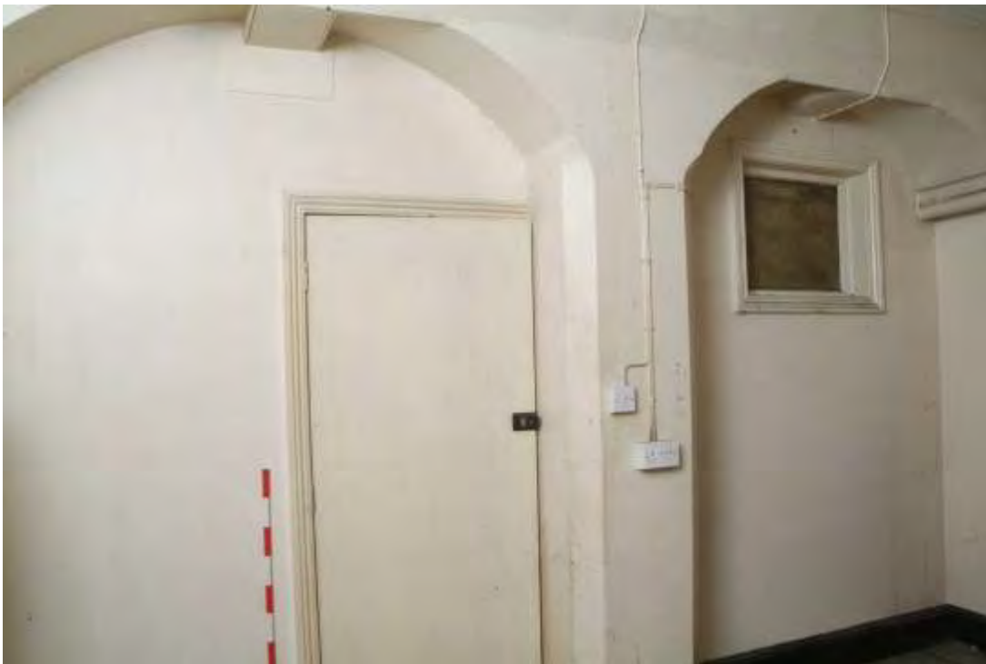
Plate 22.57: Building 22 (LGF): interior of 'Porter's Rest Room' showing piers and high level window, view to the northeast
