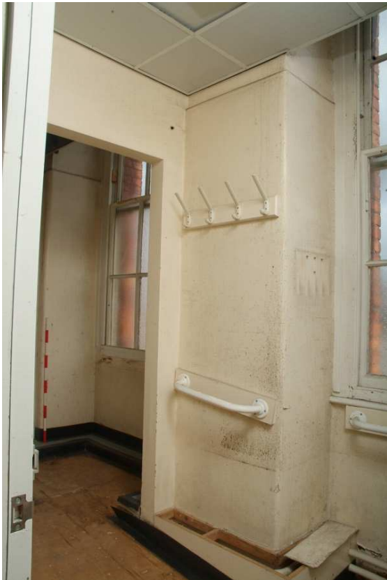
Plate 24.171: Building 24 (FF): interior of shower room showing later partitions, view to the northeast
