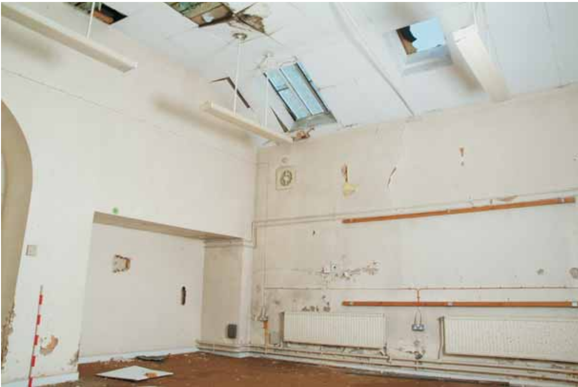
Plate 14.25: Building 14 – detail demonstrating difference between original and later roof lights, view to the southeast
