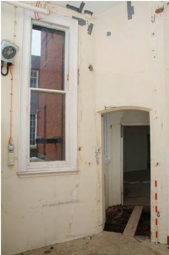
Plate 24.85: Building 24: Wheeley Lea Ward [Room 1.35] showing interior of corner tower (Building 24g), view to the west
