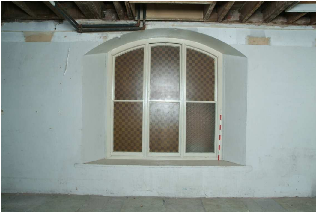
Plate 24.135: Building 24 (LGF): detail of southern original window and blocking of Building 17 link corridor [Room 91], view to the south
