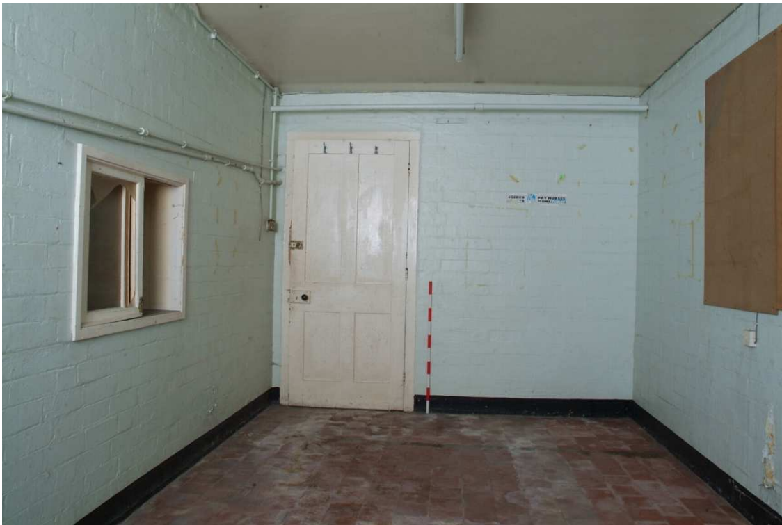
Plate 43.45: Building 43 – basement: porters room to the west of the basement entrance hall showing tally window, view to the south
