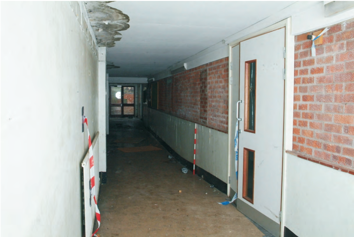
Plate 23.9: Building 23 - internal southern elevation of the E - W corridor showing inserted doorway to Building 32, view to the southeast
