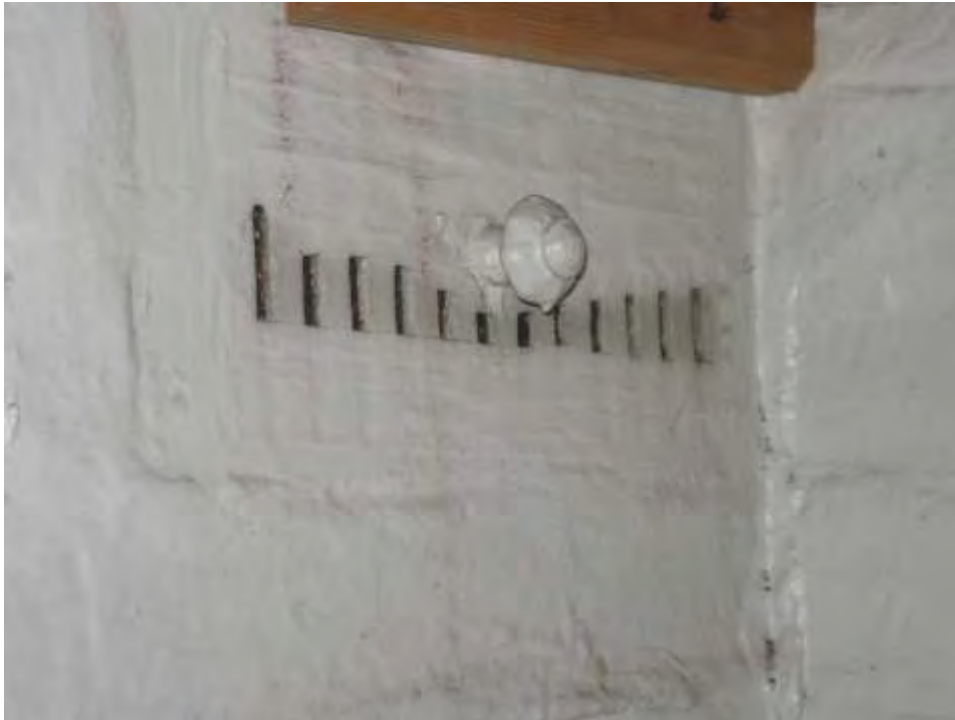
Plate 36.11: Building 36 – detail of closable vent in east side, view to the southeast
