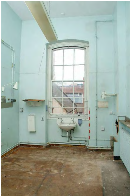
Plate 24.161: Building 24 (FF): interior of ward [Room 2.18] showing original window, view to the west
