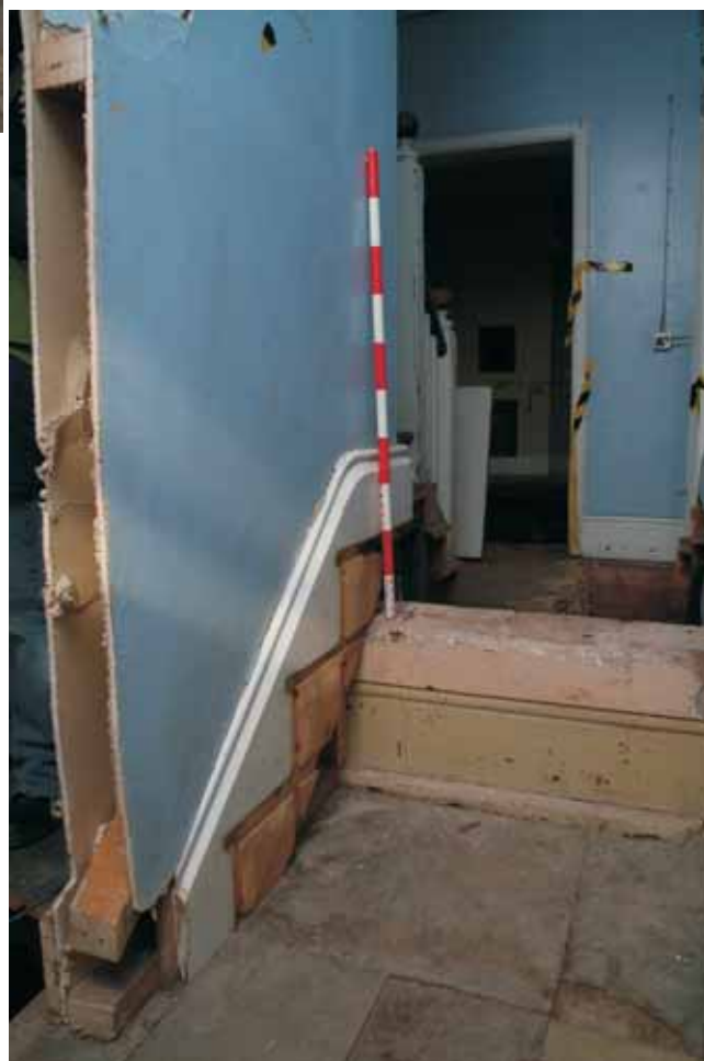
Plate 18.16: Building 18 – ground floor: detail showing original west ward skirting beneath inserted steps, view to the northeast
