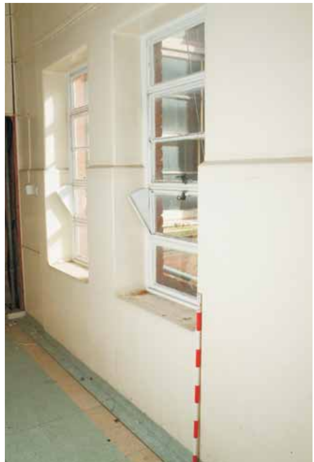
Plate 17.38: Building 17b – ground floor: hopper-light windows on the south side of link corridor between 17a and 1938 extension to 17b, view to the southeast
