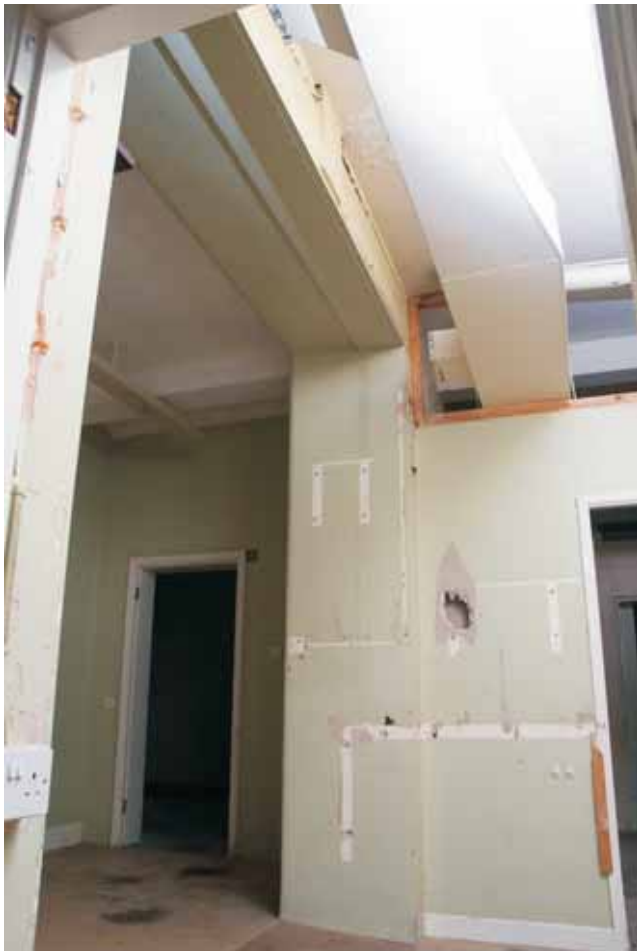
Plate 17.37: Building 17b – basement: former window opening on south side of VD Clinic enlarged to access 1938 extension, view to the northeast
