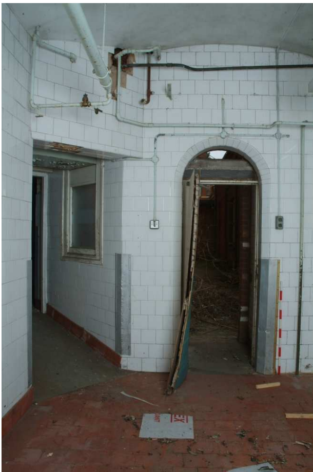
Plate 24.118: Building 24 (LGF): interior of southwest corner tower showing original external doorway, view to the east
