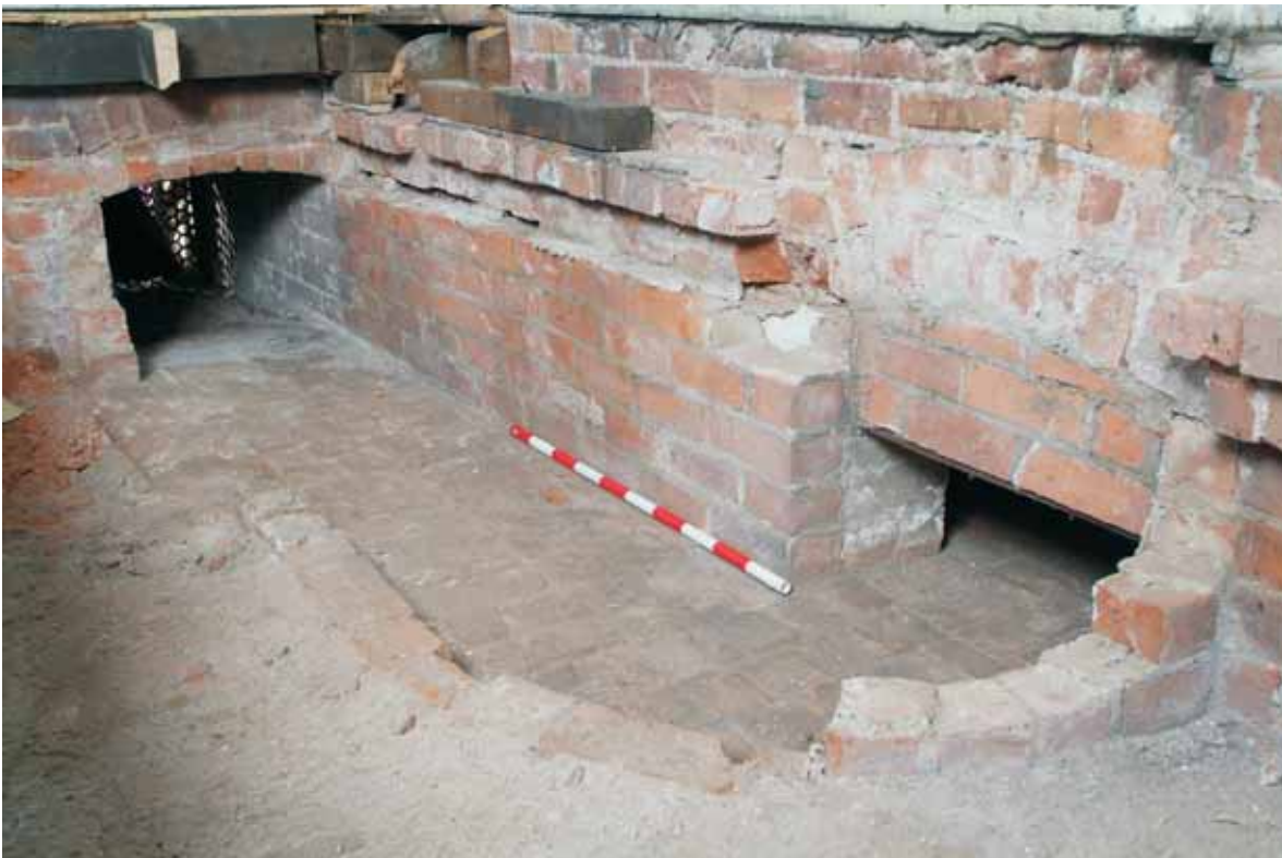
Plate 18.27: Building 18 – ground floor: main air inlet duct beneath duty room floor, view to the northwest
