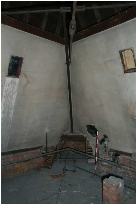
Plate 24.211: Building 24 (SF): lathe and plaster lining to roof of the southeast corner tower, view to the northwest
