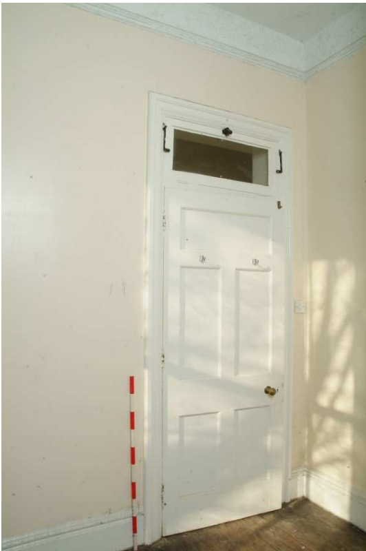
Plate 43.29: Building 43 – ground floor: typical original door and overlight to bedrooms in north and south ranges
