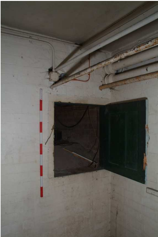
Plate 43.43: Building 43 – basement: hatch over below floor service duct, view to the southwest
