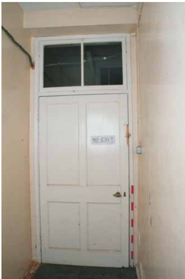
Plate 22.9: Building 22 – upper ground floor: interior of modified original door in formerly external southern elevation, view to the south
