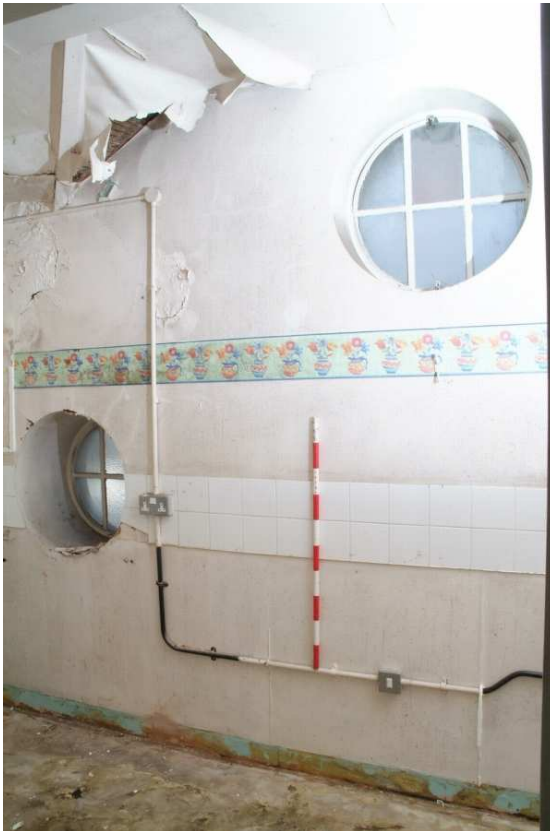
Plate 40.23: Building 40 (UGF): splint room [Room 1.8] showing oculus windows, view to the northwest
