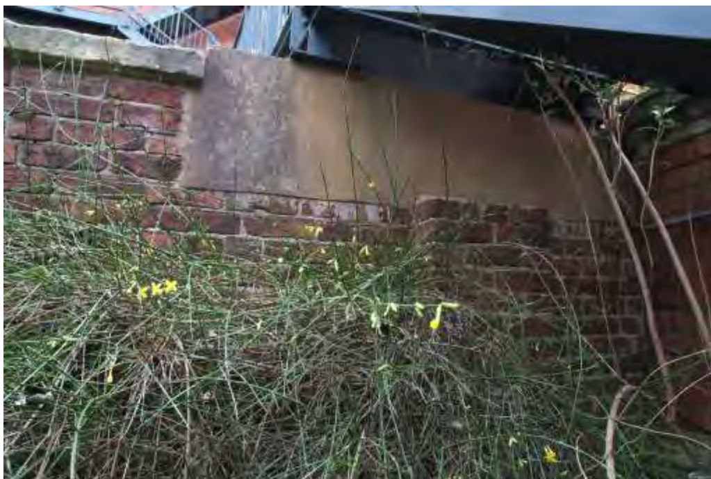
Plate 36.7: Building 36 – southern elevation showing 20 th century insertion of concrete foundation for fire escape, view to the northeast
