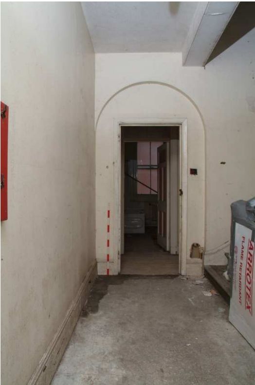
Plate 43.51: Building 43 - first floor: part blocked opening to northern range, view to the north
