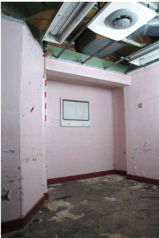
Plate 24.145 Building 24 (LGF): former original entrance to Building 24b now blocked in Room 72, view to the southwest
