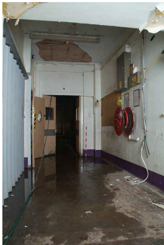
Plate 24.92: Building 24 (LGF): southern lift and entrance to Building 17 link corridor, view to the west
