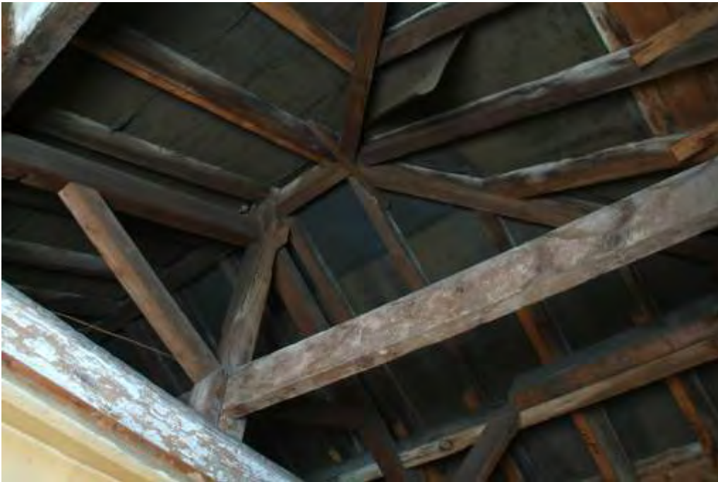
Plate 35.11: Building 35 – detail of roof structure in eastern part, view to the northeast
