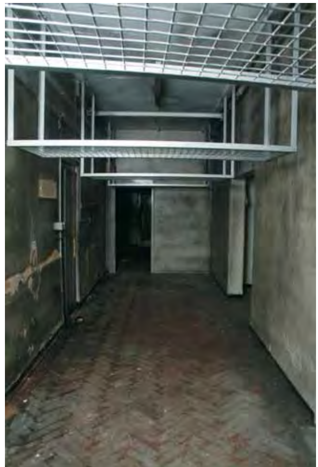
Plate 17.16: Building 17a – basement: 1938 parquet flooring of N-S link corridor, view to the north
