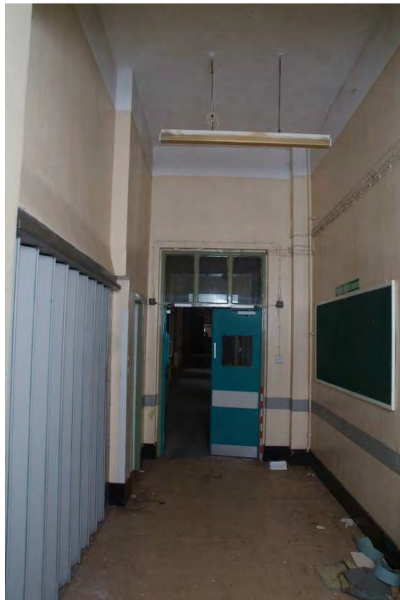
Plate 24.76: Building 24: corridor and southern lift looking toward the Building 17 link corridor, view to the west
