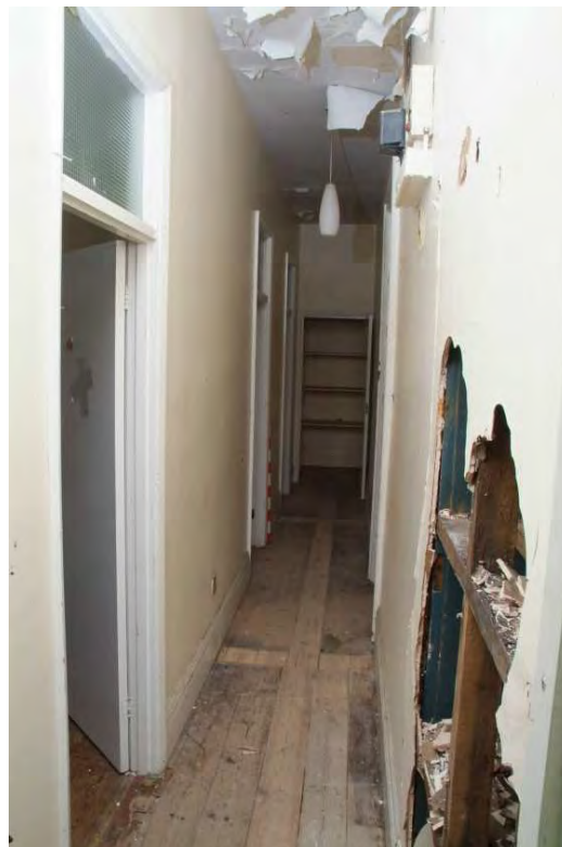
Plate 43.54: Building 43 - first floor: inserted corridor to the west of the central corridor wall showing blocked original openings, view to the north
