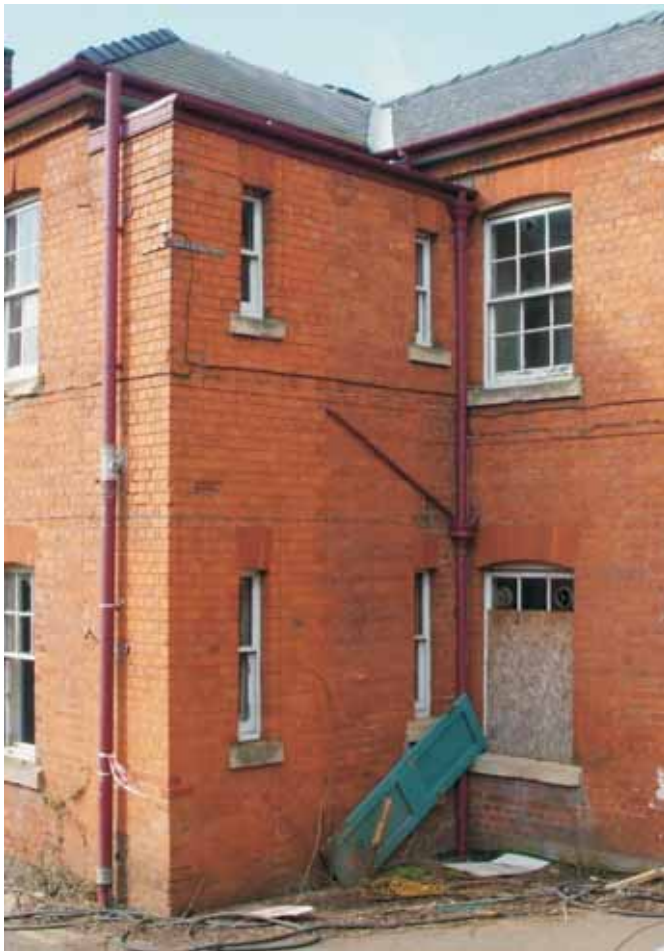
Plate 18.7: Building 18 – detail of eastern closet wing showing vertical joints in brickwork, view to the northwest
