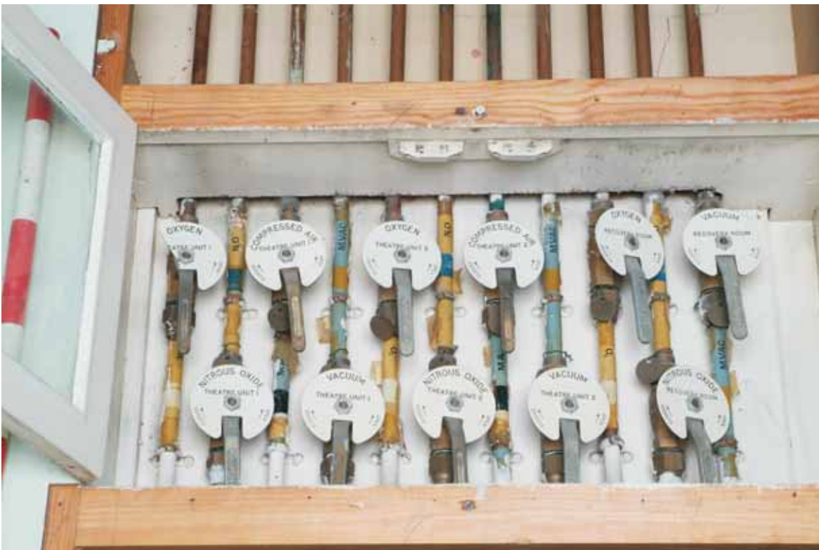
Plate 17.32: Building 17a – second floor: detail of gas supply controls to operating theatres
