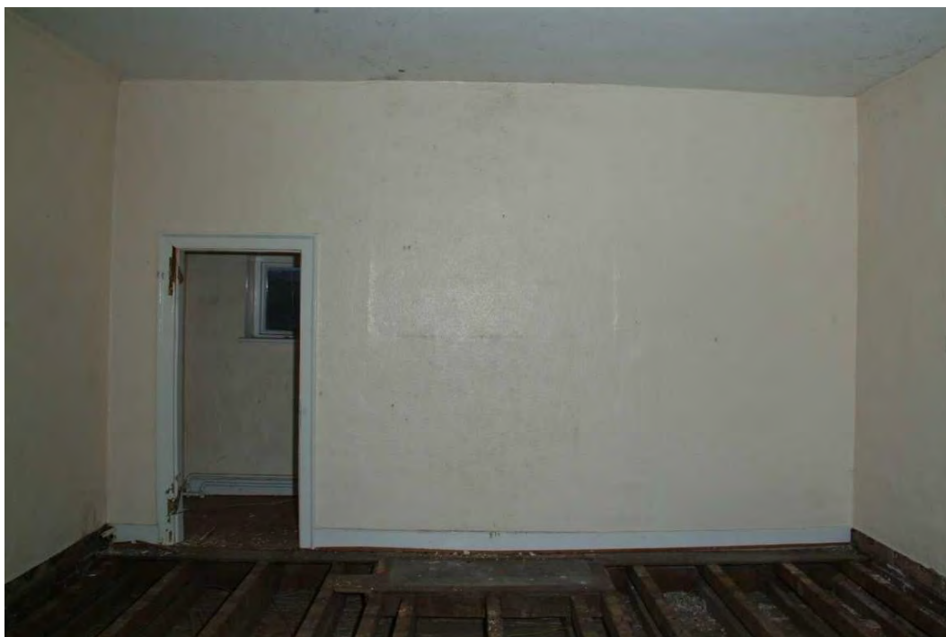
Plate 30.43: Building 30 (FF): northeast principal room showing doorway to wardrobe, view to the south
