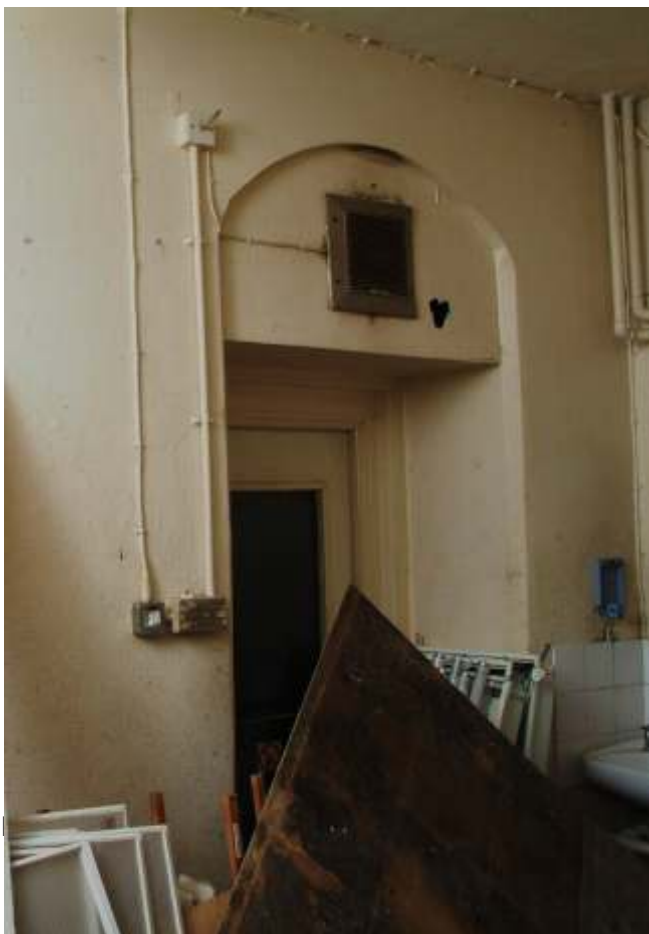
Plate 22.65: Building 22 (LGF): interior of 'Porter's Rest Room' showing detail of inserted doorway in north wall, view to the northwest
