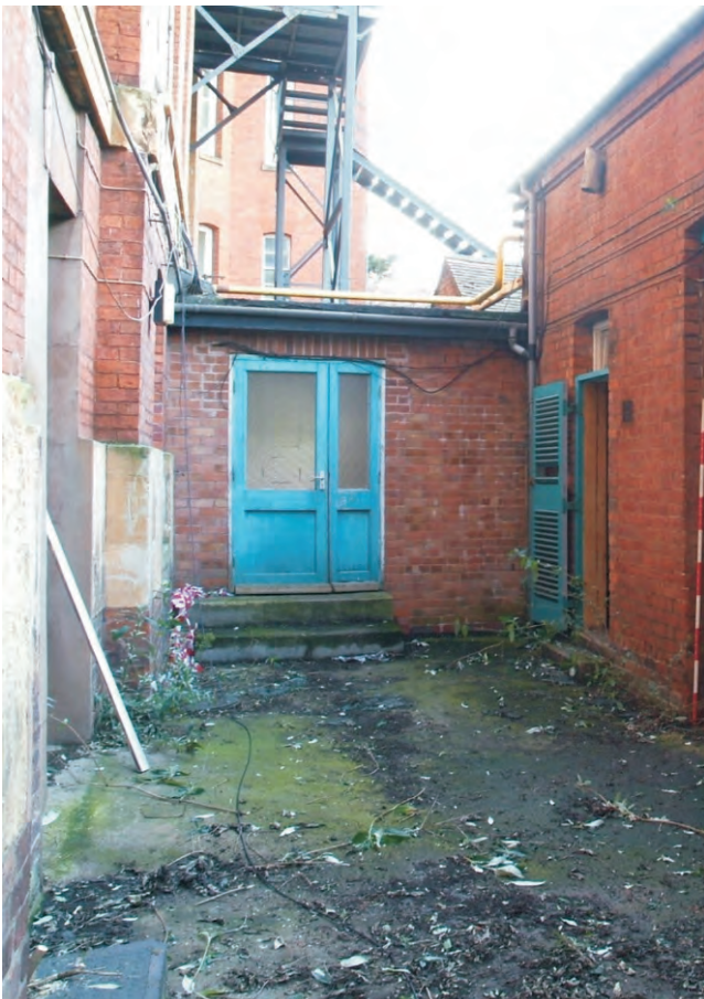
Plate 23.4: Building 23 - exposed western elevation of short N - S corridor at the eastern end of the structure, view to the east
