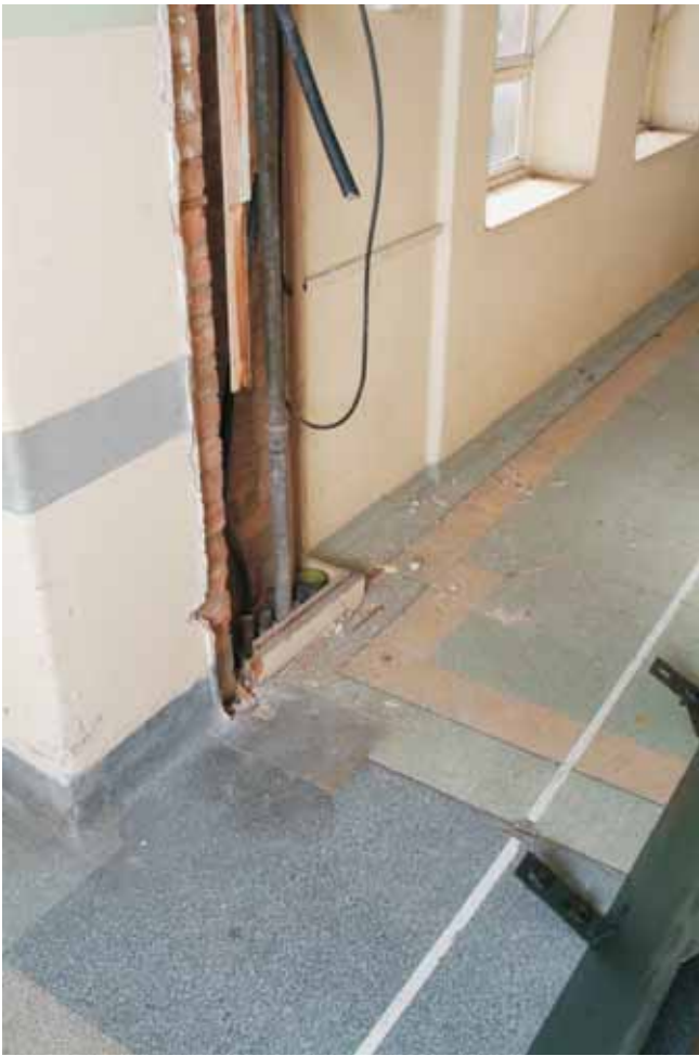
Plate 17.39: Building 17b – ground floor: floor and skirting detail at entrance to link corridor between 17a and 1938 extension to 17b, view to the southwest
