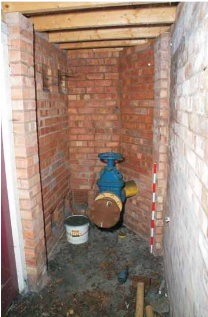
Plate 9.2: Building 9 – interior showing mains riser, view to the west
