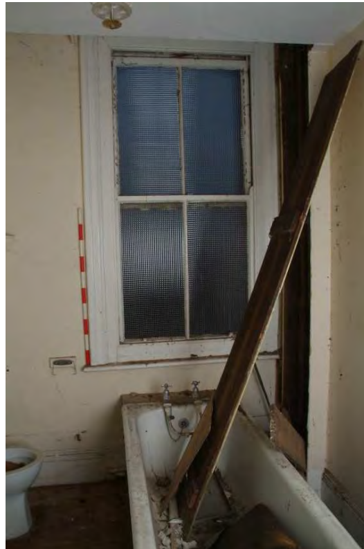
Plate 43.70: Building 43 - second floor: bathroom in central range showing original vertical pipe box, view to the east
