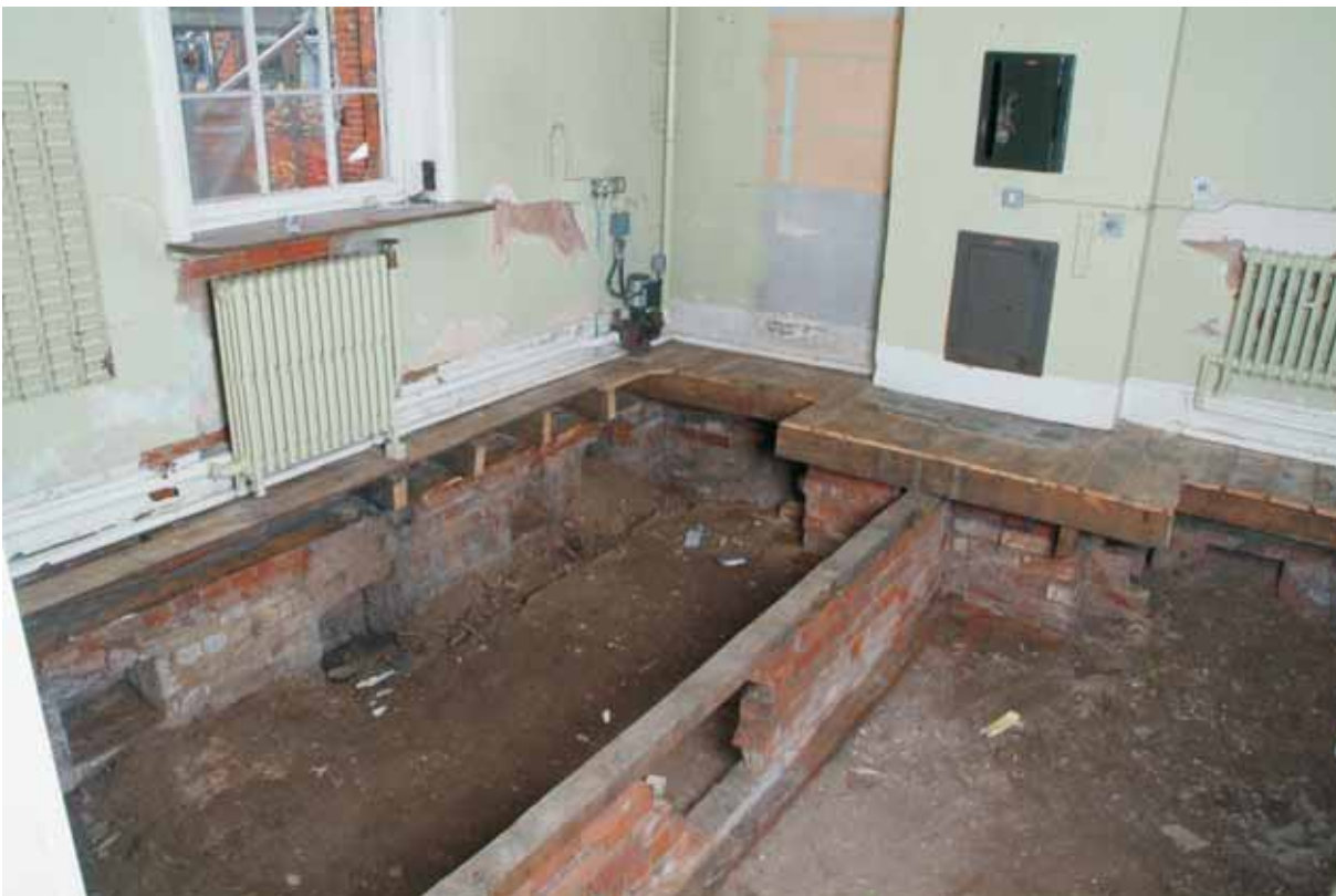
Plate 18.22: Building 18 – ground floor: east ward following removal of the floor showing traces of brick ducting, view to the northeast
