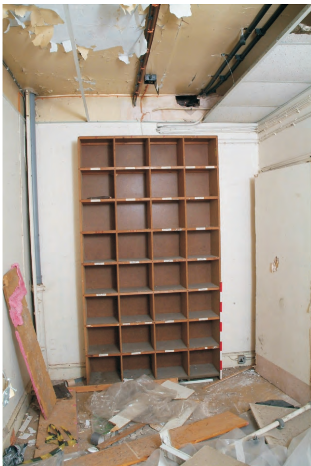
Plate 22.49: Building 22 – connecting range (LGF): interior of the 'Contingency Store', view to the west
