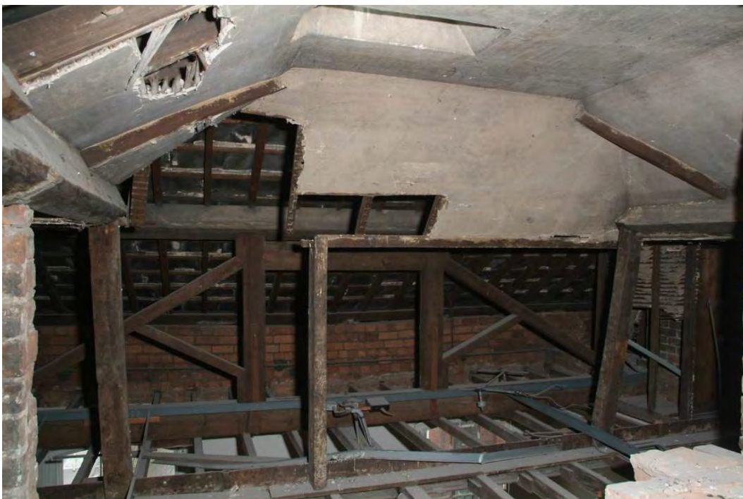
Plate 24.216: Building 24 (Roof Structure): lathe and plaster chamber in roof west of centre
