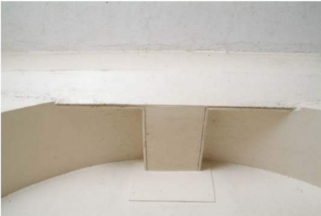
Plate 22.61: Building 22 (LGF): interior of 'Porter's Rest Room' showing high level ducts, view to the north
