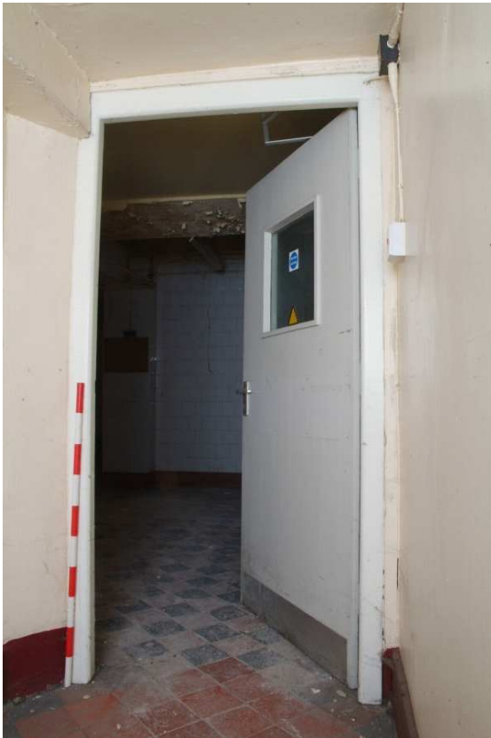
Plate 24.111: Building 24 (LGF): doorway from central corridor through to main kitchens [Room 110], view to the west
