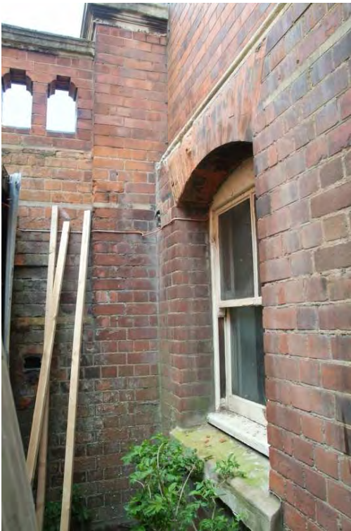
Plate 43.11: Building 43 – basement window to the east of the porch, view to the southeast
