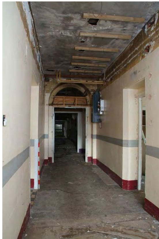
Plate 24.90: Building 24 (LGF): central corridor [Room 90] from the south, view to the north
