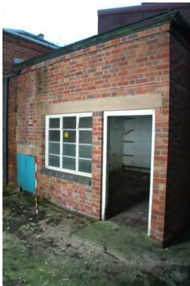
Plate 33.4: Building 33 – northern elevation showing blocked entrance in western part, view to the southwest
