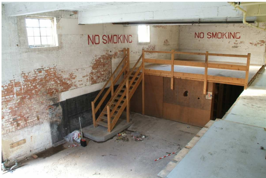
Plate 27.62: Building 27b – lower ground floor: loading bay and mezzanine at western end, view to the northwest
