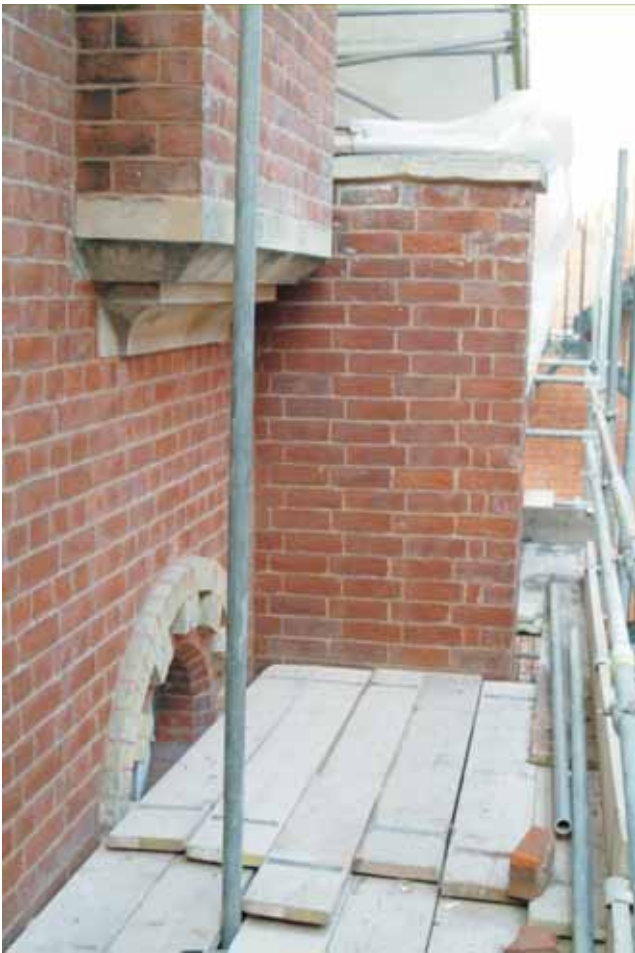
Plate 22.15: Building 22 – oculus in eastern elevation (partly obscured by scaffolding), view to the northwest
