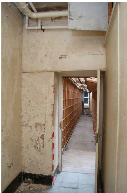
Plate 24.110: Building 24 (LGF): interior of southeast corner tower looking through inserted opening into Building 8, view to the south
