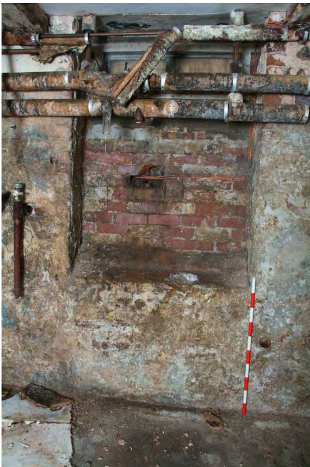
Plate 30.32: Building 30 (LGF): easternmost part of original basement showing part blocked window, view to east
