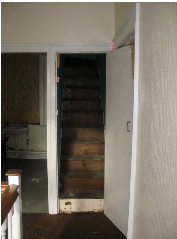
Plate 30.38: Building 30 (FF): landing showing original doorways to the bathroom and attic stairs
