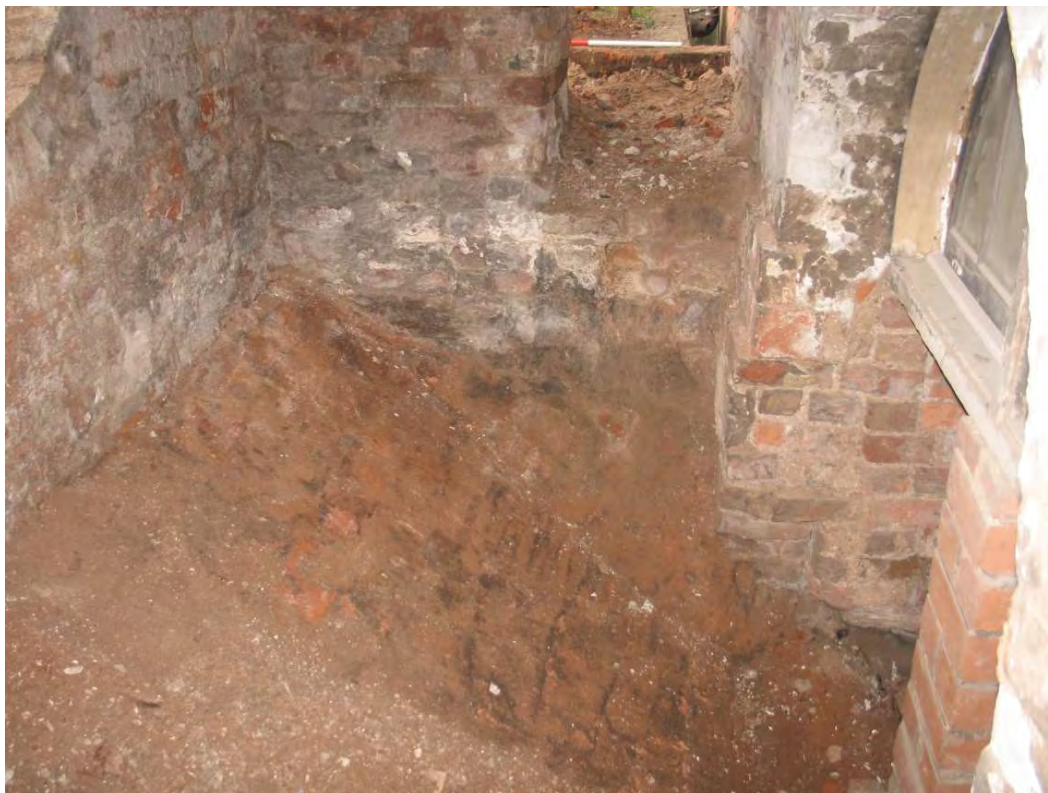
Plate 24.12: Building 24: sloping floor inside barrel vault of central platform, view to the south
