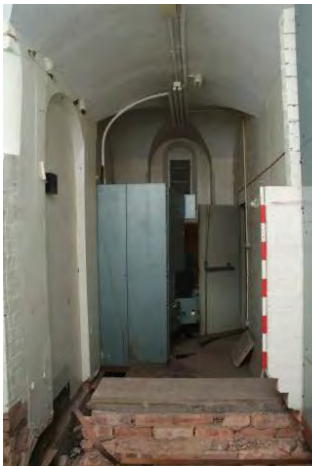
Plate 22.69: Building 22 (LDF): interior of western part of the electricity switch room, view to the north
