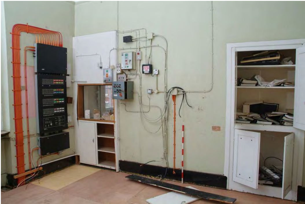
Plate 24.55: Building 24: comms room [Room 1.19], view to the northwest
