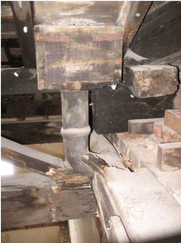
Plate 24.219: Building 24 (Roof Structure): internal lead rainwater hopper and pipe, view to the west
