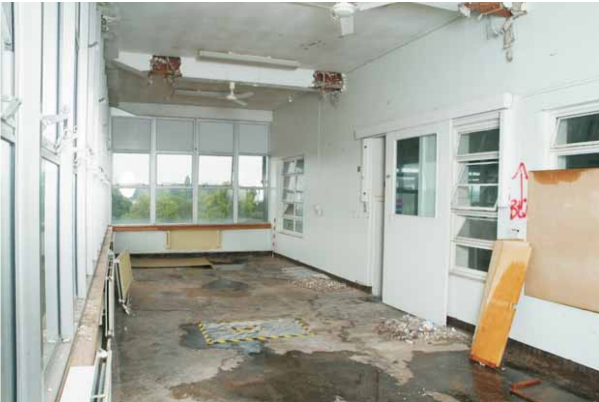
Plate 17.45: Building 17b – second floor: interior of 1960s extension on south side of main block, view to the west
