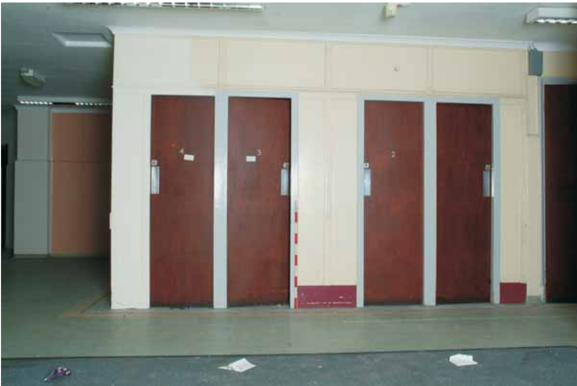
Plate 17.42: Building 17b – ground floor: original doors to changing rooms, view to the north
