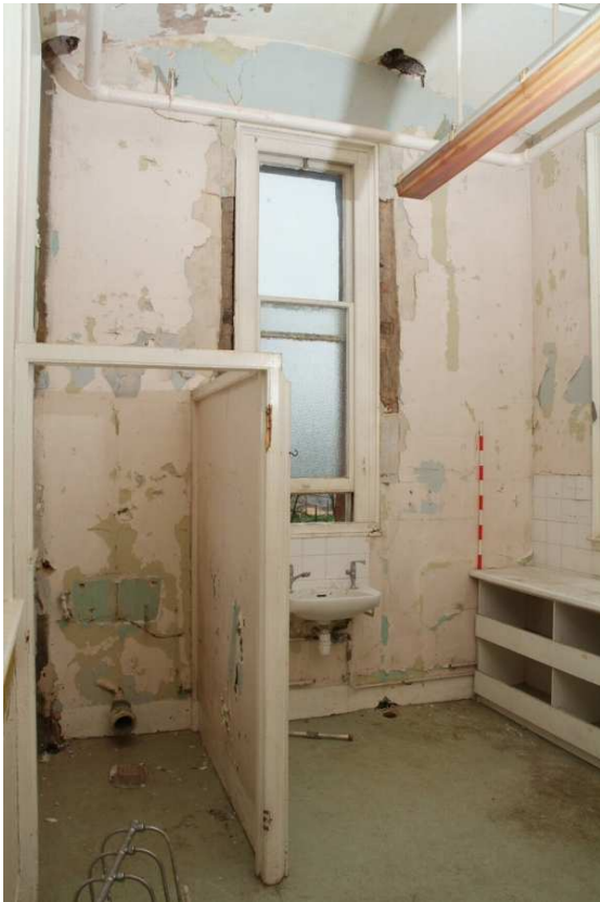
Plate 24.65: Building 24: Rushout Ward [Room 1.12 and 13] showing interior of corner tower, view to the northwest
