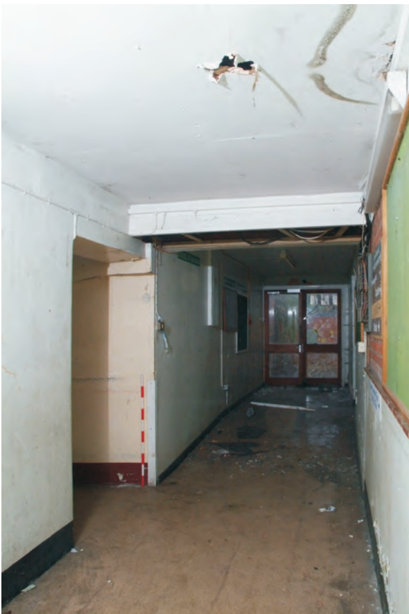
Plate 23.10: Building 23 - inserted opening to staff restaurant at east end of the E - W corridor, view to the northeast
