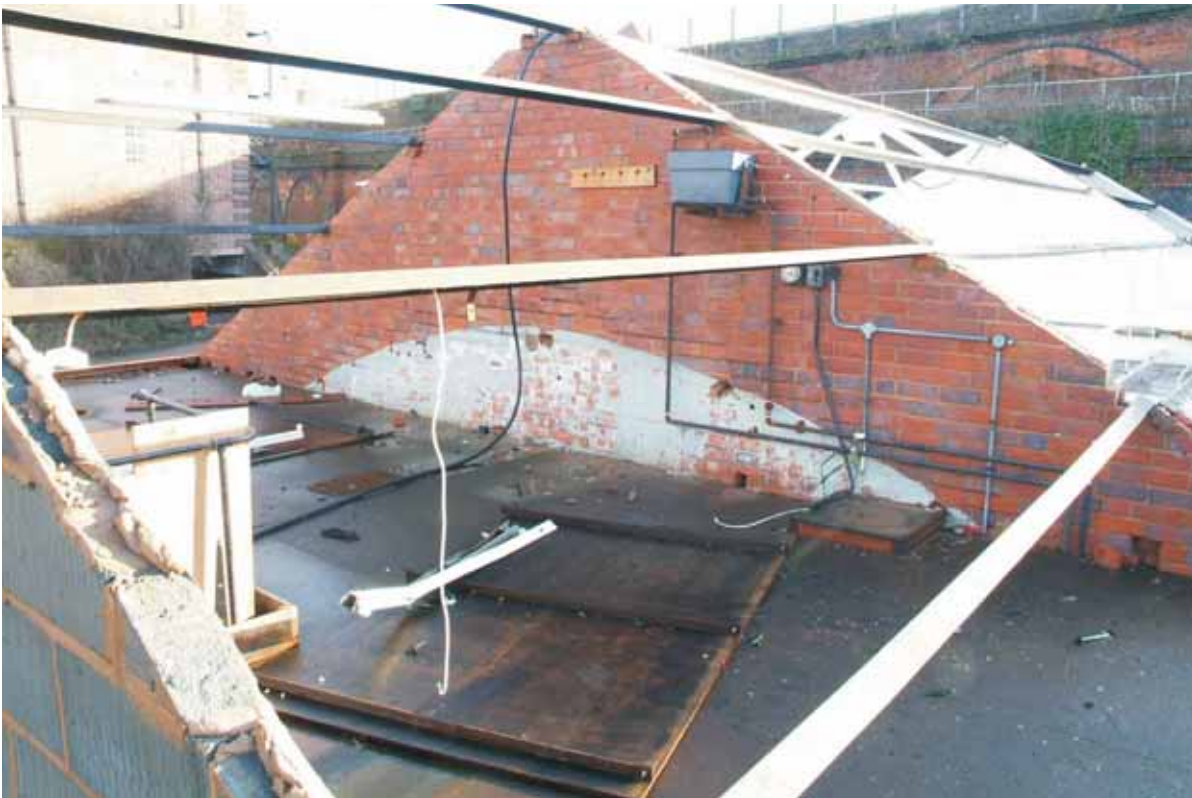
Plate 6.19: Building 6 – detail of wall between former southern workshop and remainder of building showing former bowed roof, view to the southeast
