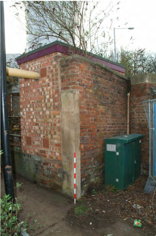
Plate 45.1: Building 45 – southern extremity of pre 1897 boundary wall backed by building 9, view to the southwest
