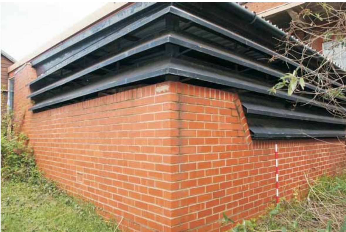
Plate 19.2: Building 19 – southern and western elevation showing detail of louvers, view to the northeast
