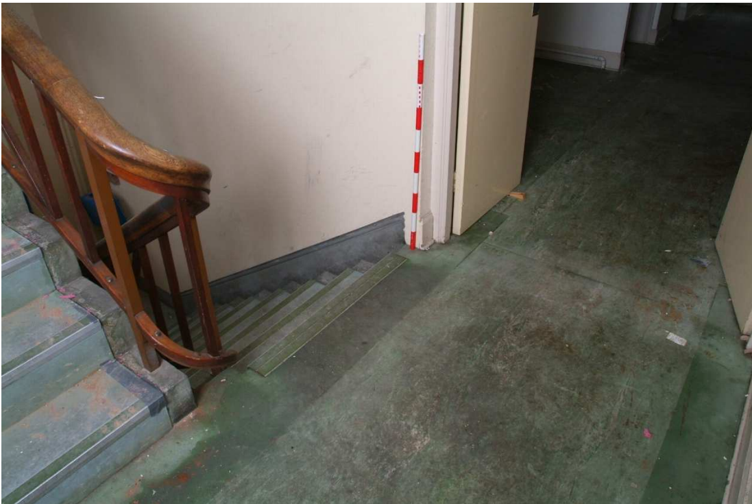
Plate 27.40: Building 27a - second floor: detail of original linoleum, view to the northwest
