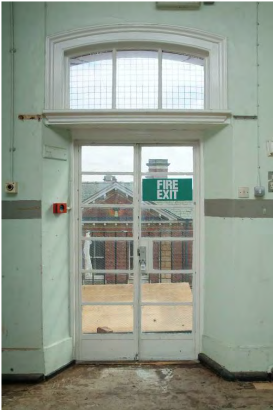
Plate 24.209: Building 24 (SF): inserted fire escape doors in south wall of Bonaker Ward, view to the south
