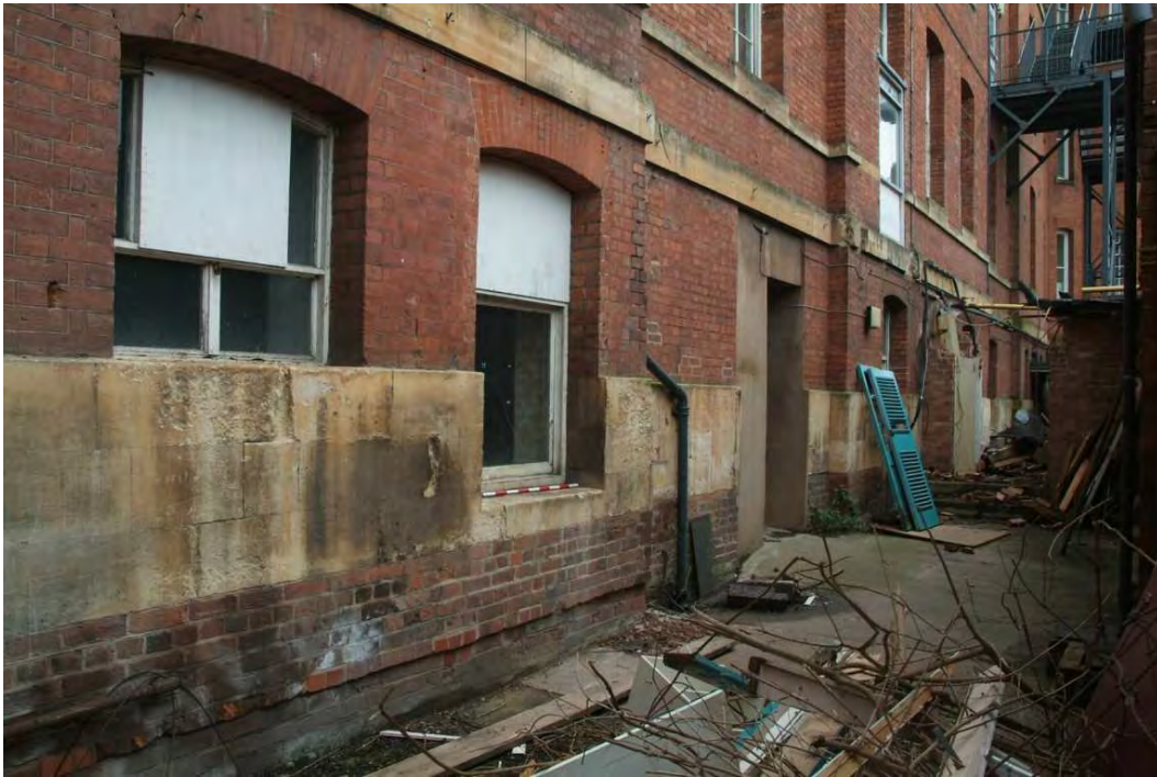
Plate 24.27: Building 24: southern elevation showing detail of left hand part of lower ground floor, view to the northeast
