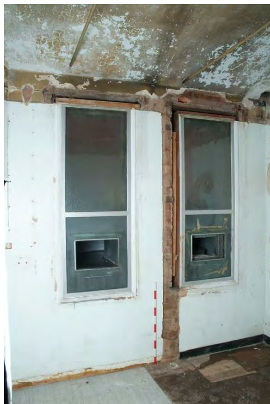
Plate 24.148: Building 24 (LGF): air ducts in modified original window openings, view to the southwest
