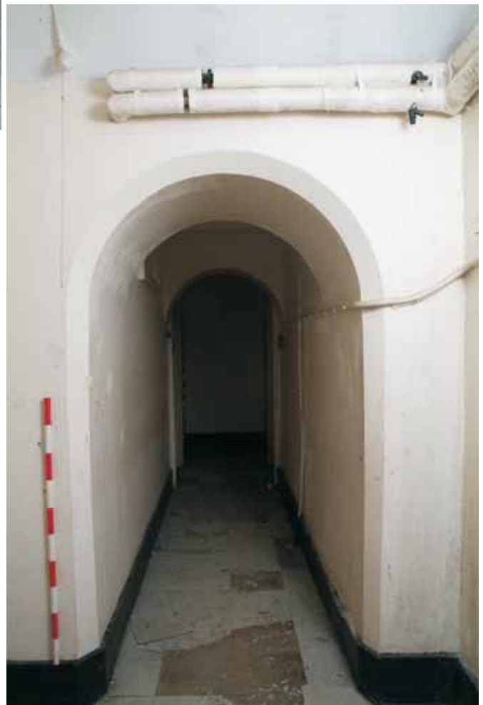
Plate 22.44: Building 22 – connecting range: central corridor on lower ground floor looking into central corridor beneath the nave, view to the west
