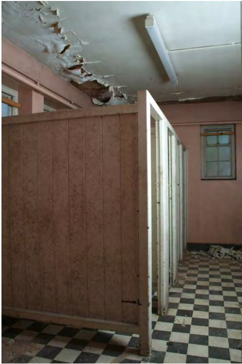
Plate 27.19: Building 27a – ground floor: interior of toilet block to the north of the principal entrance, view to the east
