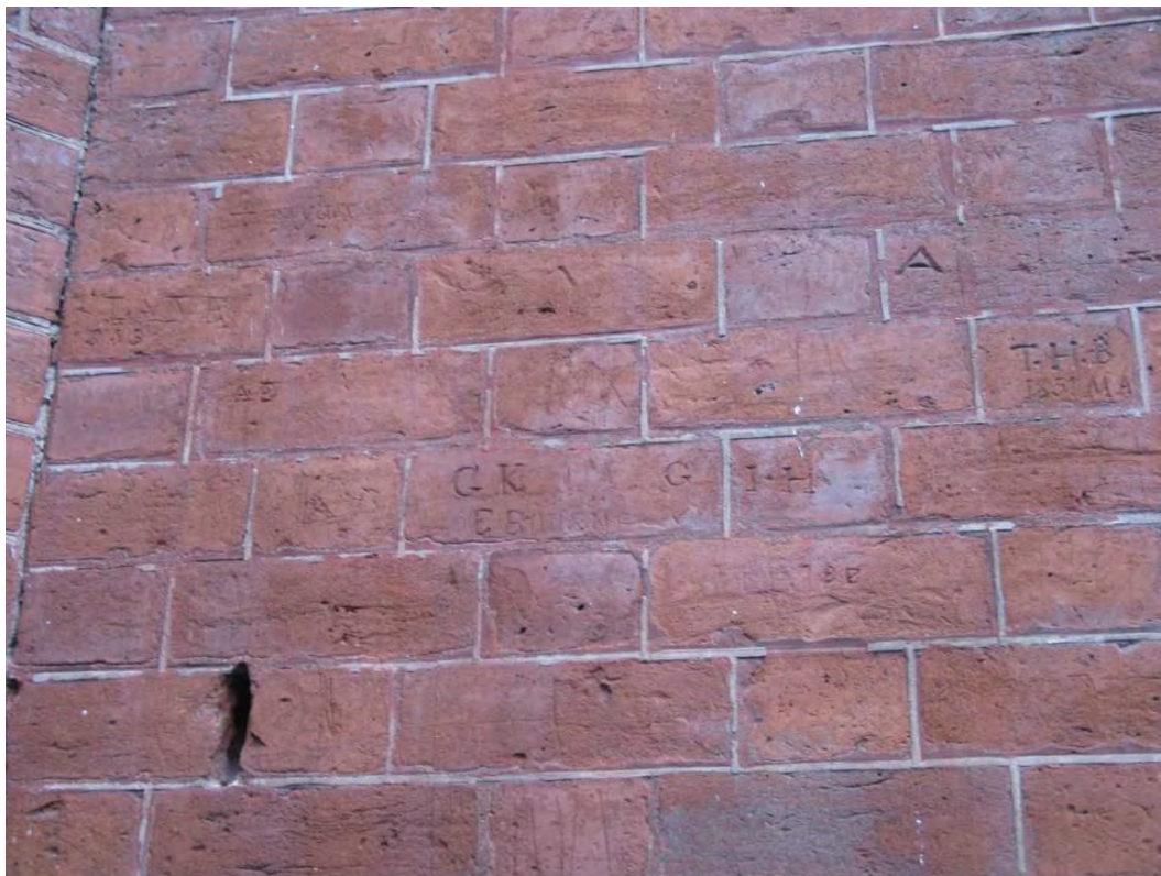
Plate 24.31: Building 24: southern elevation showing detail of graffiti on lower ground floor of western extension (Building 24d), view to the north
