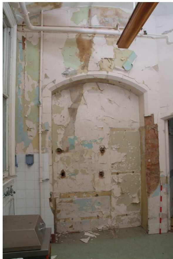
Plate 24.66: Building 24: Rushout Ward [Room 1.12] showing interior of corner tower, view to the east
