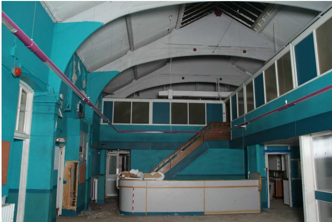
Plate 41.5: Building 41: general view of the interior showing inserted mezzanine, view to the west
