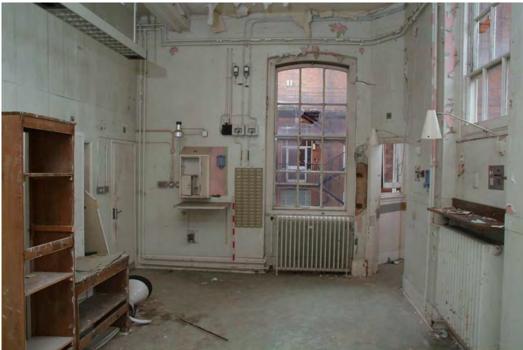
Plate 24.60: Building 24: Rushout Ward [Room 1.11], west end (Building 24b), view to the west
