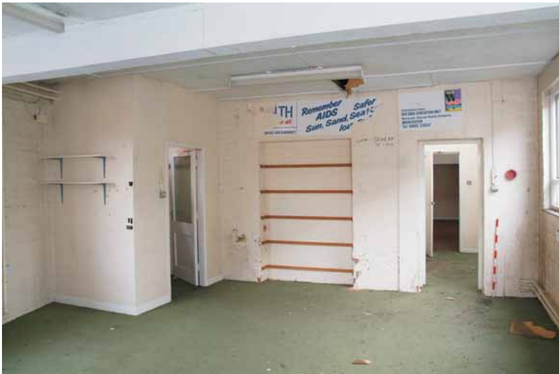
Plate 13.9: Building 13 – Interior of ground floor showing connecting door to Building 14, view to the east
