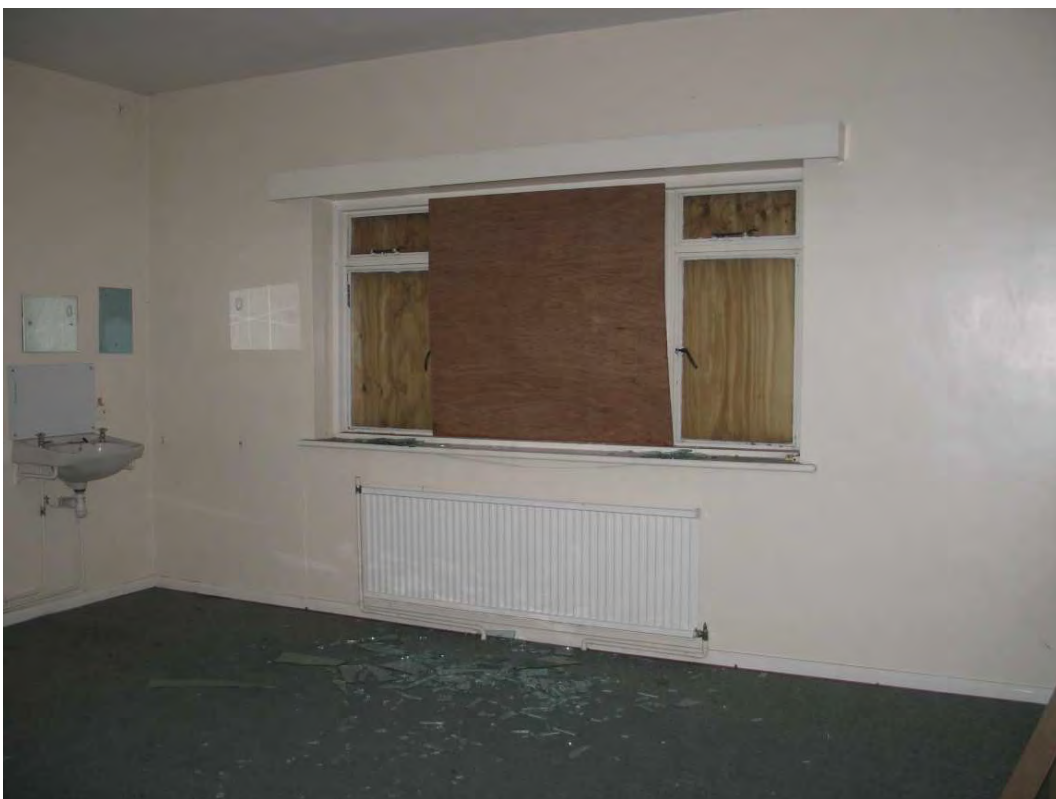
Plate 30.36: Building 30 (LGF): interior of south eastern room in the late 20th century extension, view to the southeast
