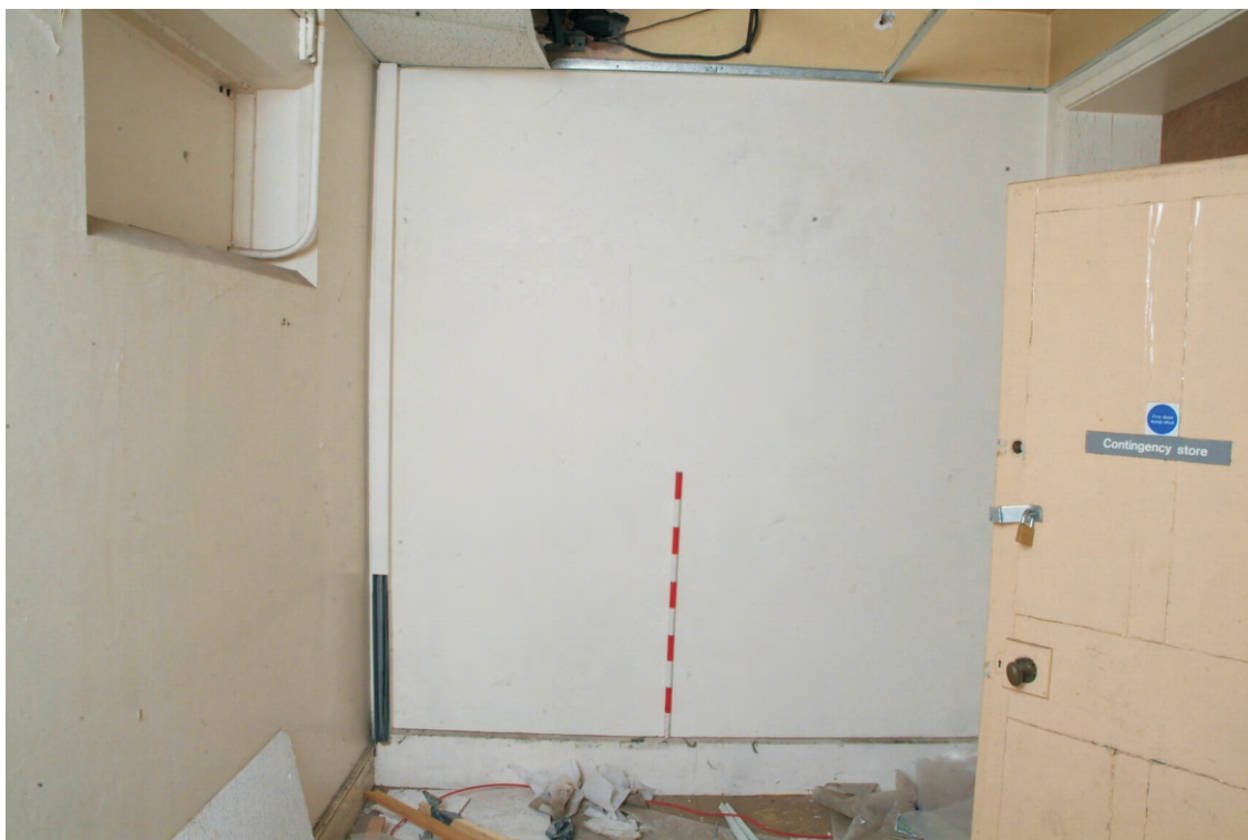
Plate 22.50: Building 22 – connecting range (LGF): interior of the 'Contingency Store' showing high level blocked window (left), view to the east
