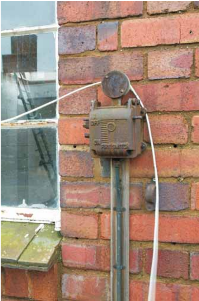
Plate 6.7: Building 6 – detail of emergency electricity isolation switch
