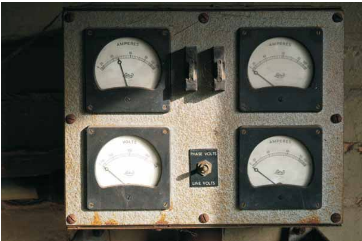
Plate 7.9: Building 7 – detail of amp metre in generator room
