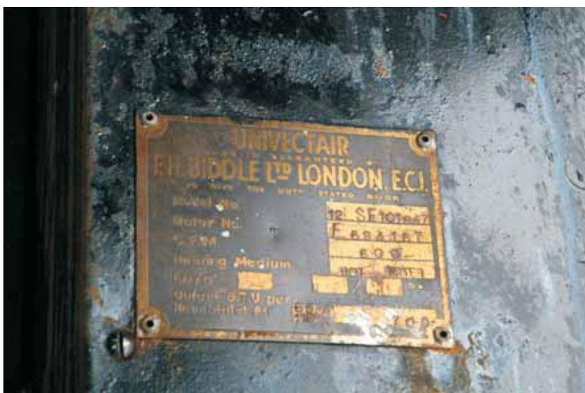
Plate 6.16: Building 6 – detail of makers plate on heater unit, northern workshop
