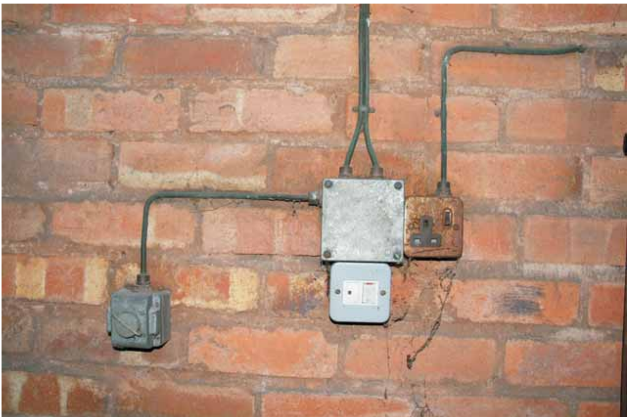
Plate 1.7: Building 1 – detail of switches
