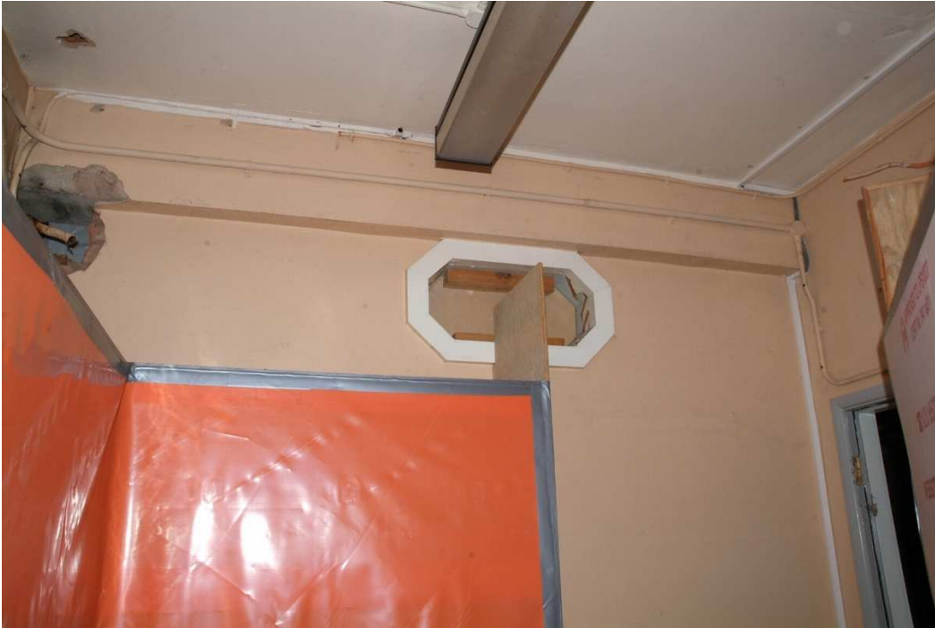
Plate 27.61: Building 27b – lower ground floor: interior of projector room, view to the west
