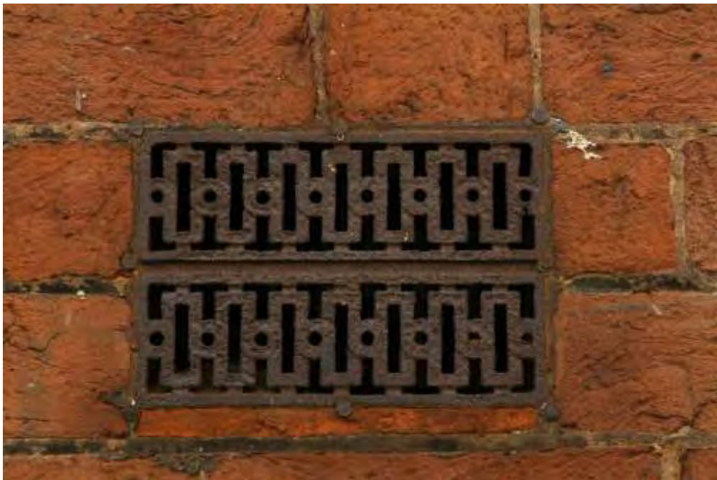
Plate 34.6: Building 34 – detail of air brick in the western part, view to the south
