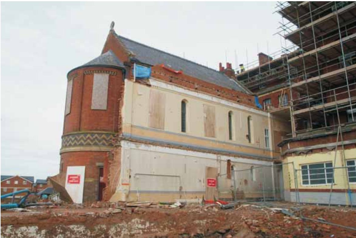
Plate 22.3: Building 22 – southern elevation following the demolition of the link corridor to Building 17a, view to the northeast
