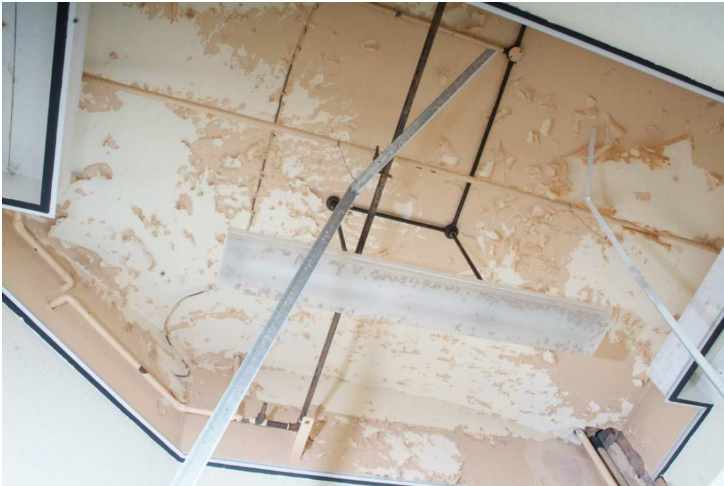
Plate 24.183: Building 24 (FF): exposed original ceiling of the southwest corner tower, view up
