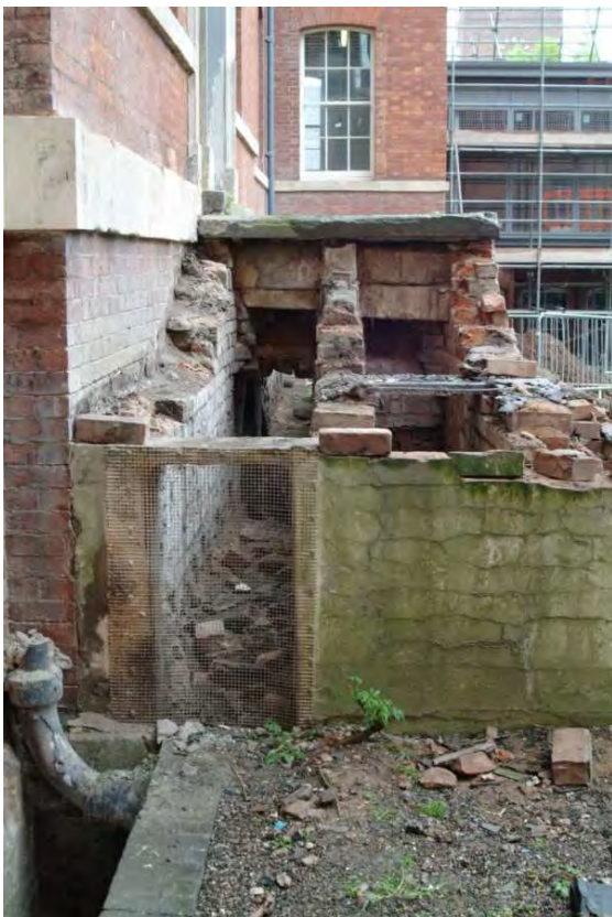
Plate 24.15: Building 24: modern grille across the mouth of the vent, view to the north
