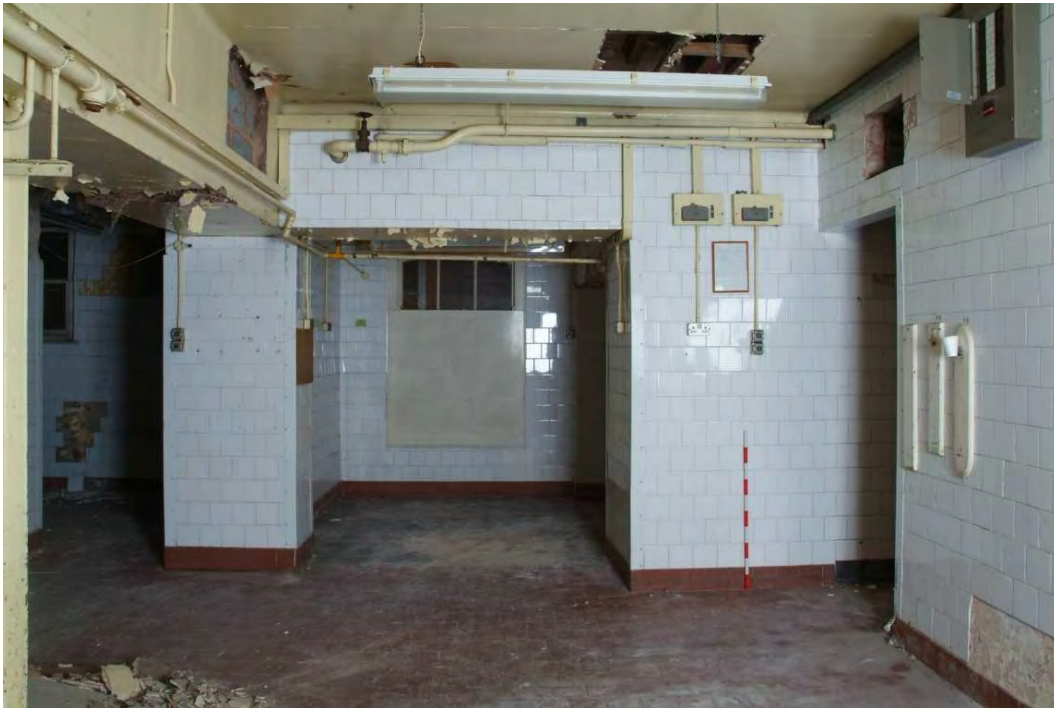
Plate 24.113: Building 24 (LGF): central part of main kitchens looking towards side entrance, view to the north
