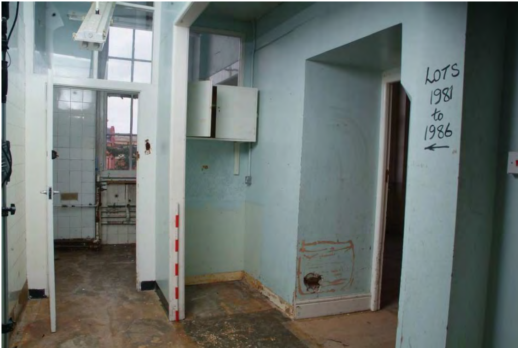
Plate 24.173: Building 24 (FF): interior of Room 2.24 showing inserted partitions and openings (right), view to the east
