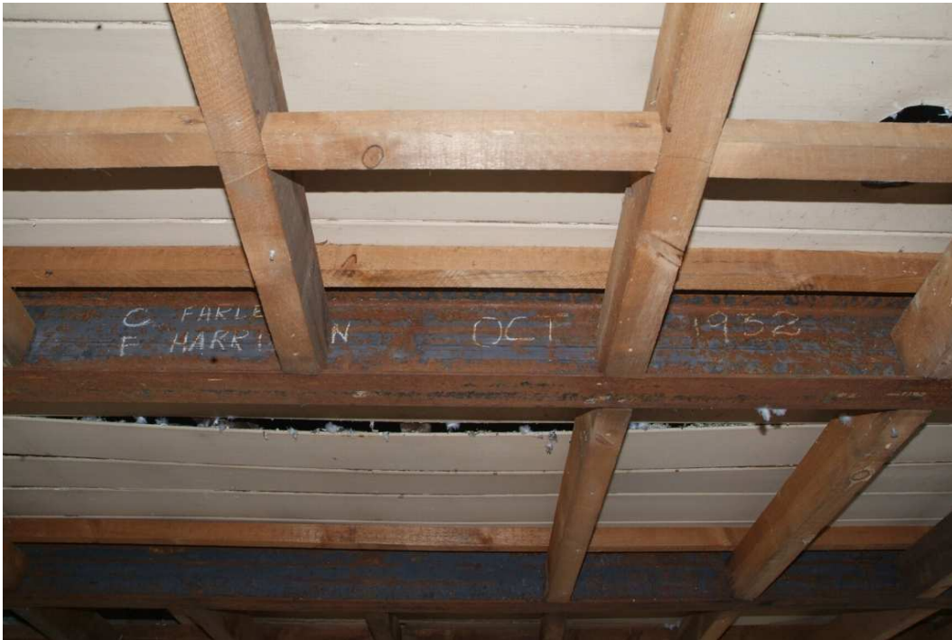
Plate 24.203: Building 24 (SF): detail of chalked inscription on steel joists, view to the south
