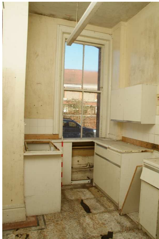
Plate 43.34: Building 43 – ground floor: kitchen area formerly bathroom, adjacent to the entrance hall, view to the east
