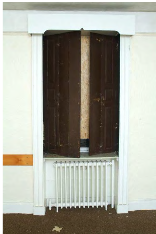
Plate 30.18: Building 30 (GF): northwest principal room showing detail of 1820s shutters, view to west
