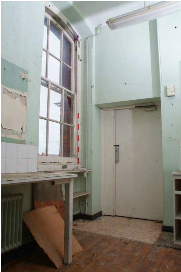
Plate 24.168: Building 24 (FF): interior of utility store room, showing inserted door to relatives room, view to the southeast
