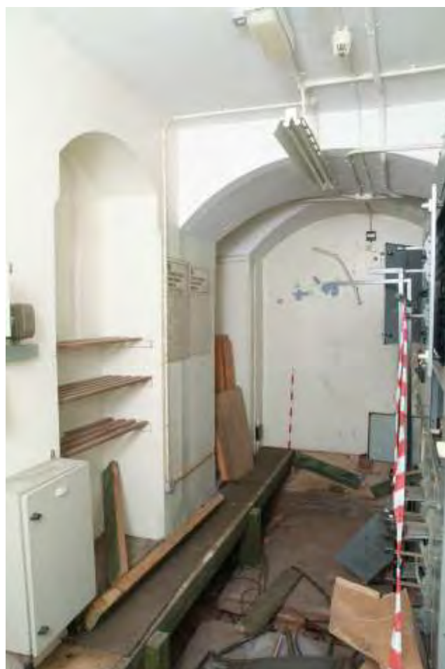
Plate 22.70: Building 22 (LGF): interior of southern part of the electricity switch room, view to the west
