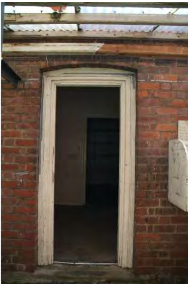
Plate 35.6: Building 35 – southern hip to the roof of the eastern part, view to the west
