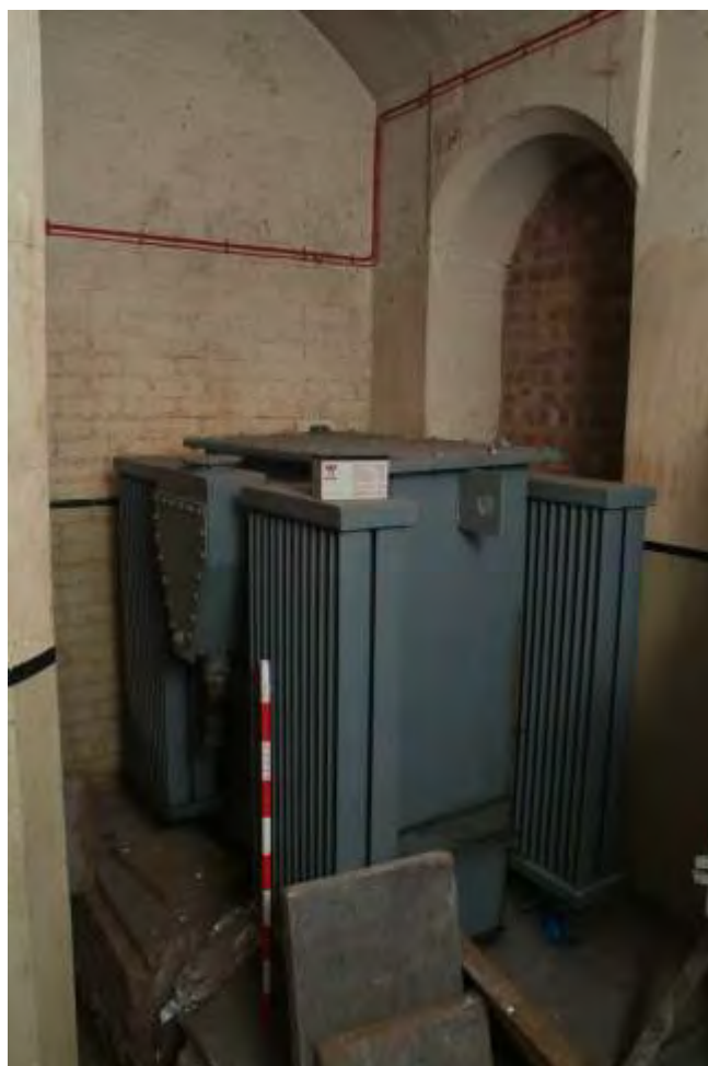
Plate 22.72: Building 22 (LGF): interior of the transformer room showing surviving transformer and brick lined sub floor ducting, view to the southwest
