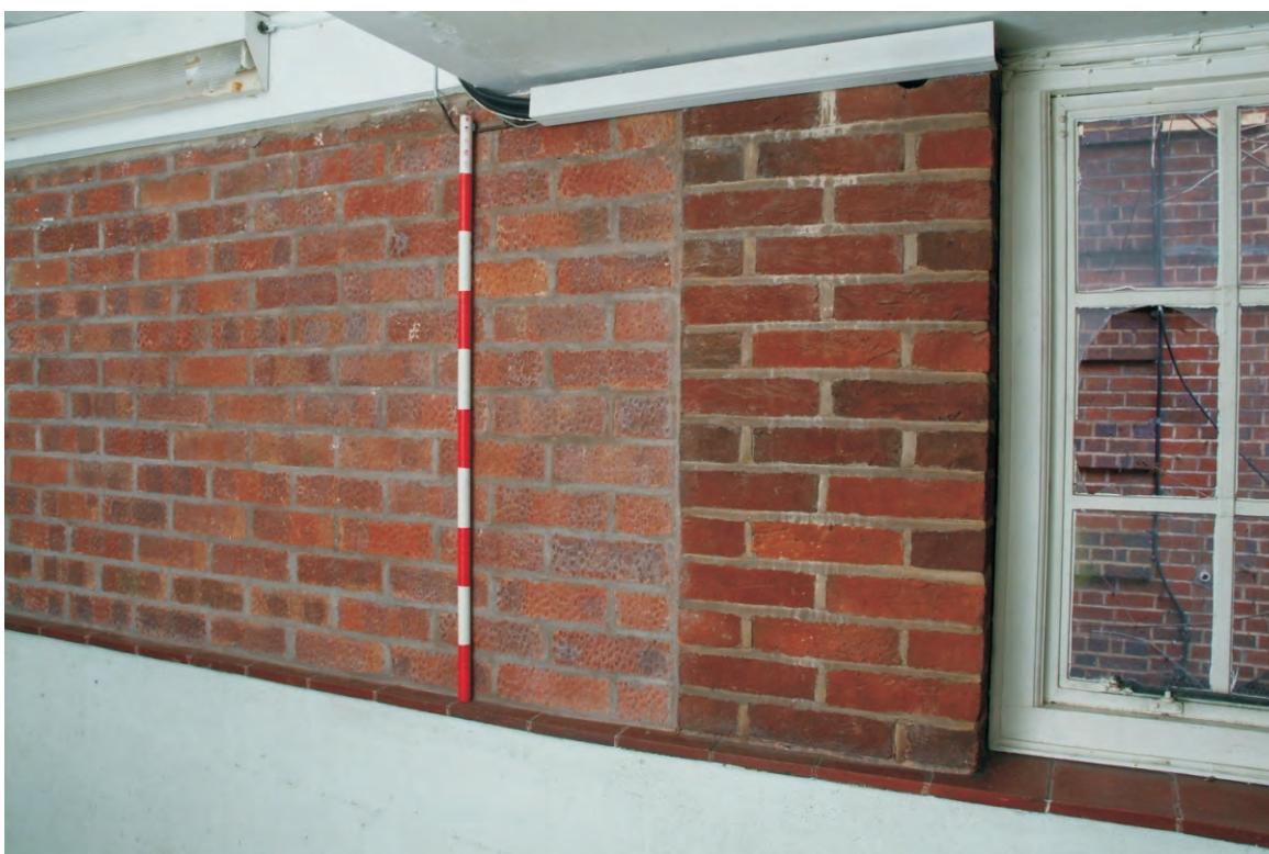
Plate 23.8: Building 23 - internal southern elevation of the E - W corridor at the western end of the structure showing pier and blocked opening, view to the southeast
