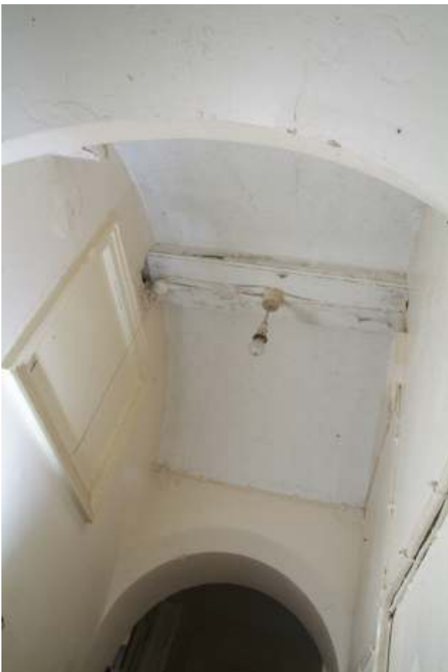
Plate 22.62: Building 22 (LGF): detail of connecting conduit crossing central corridor and high level window from the 'Porter's Rest Room' view to the west
