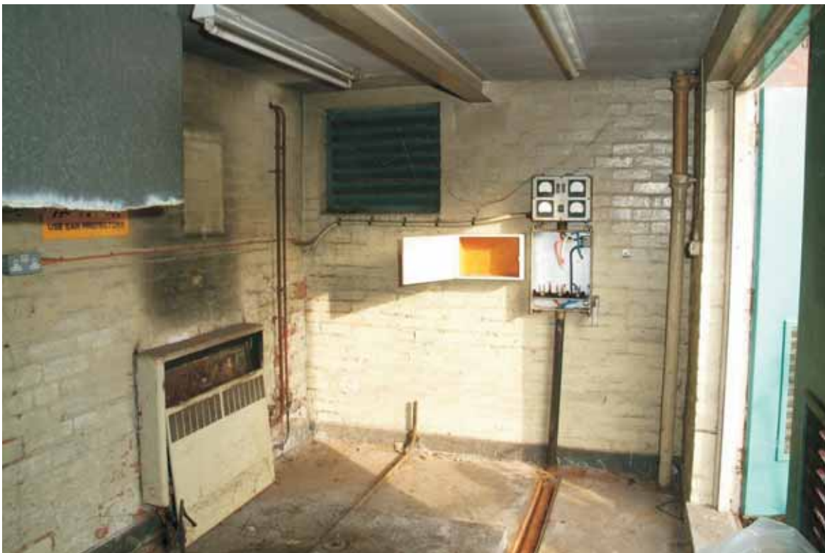
Plate 7.8: Building 7 – interior of generator room, view to the northeast
