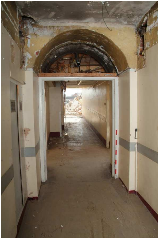
Plate 24.89: Building 24 (LGF): central corridor [Room 90] looking through the southern entrance, view to the south
