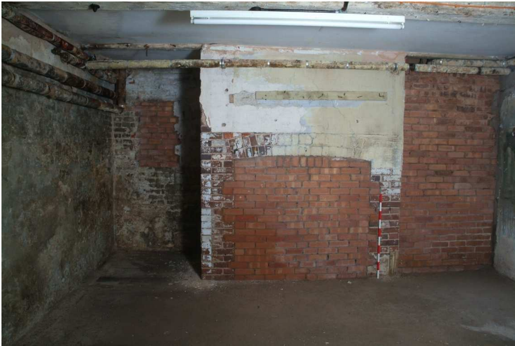
Plate 30.31: Building 30 (LGF): easternmost part of original basement showing blocked fireplace and window, view to the south
