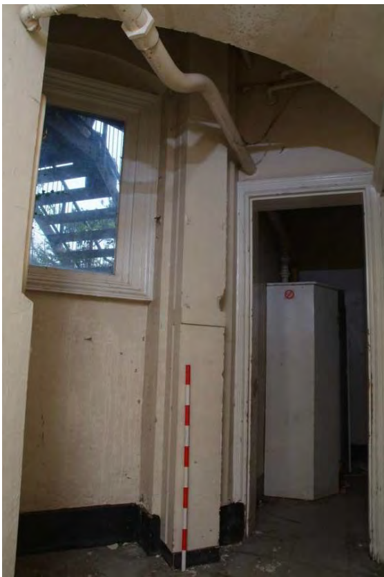
Plate 24.109: Building 24 (LGF): original opening in base of southeast corner tower, view to the northeast
