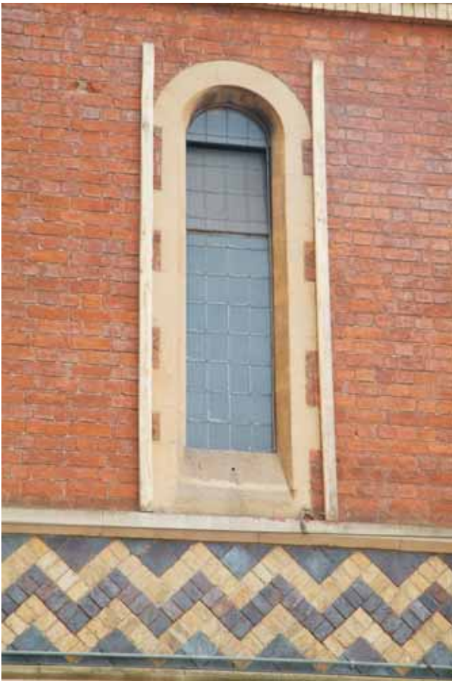
Plate 22.11: Building 22 – detail of nave lancet on northern elevation, view to the southwest
