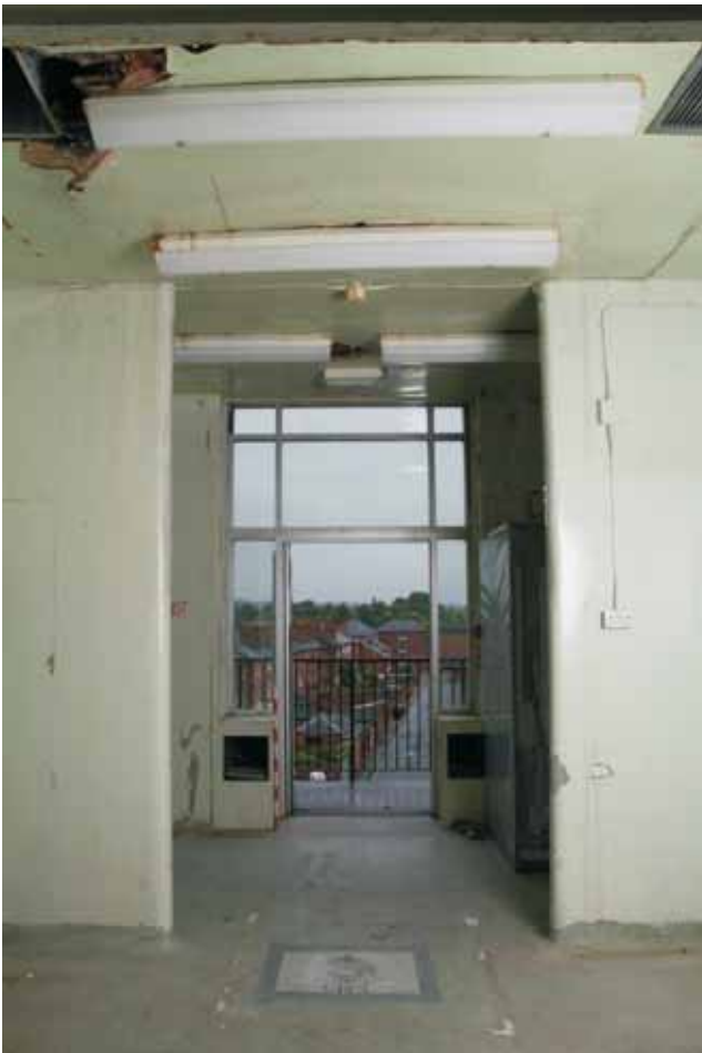
Plate 17.31: Building 17a – second floor: central corridor looking through to the preparation/ sterilizing room, view to the north
