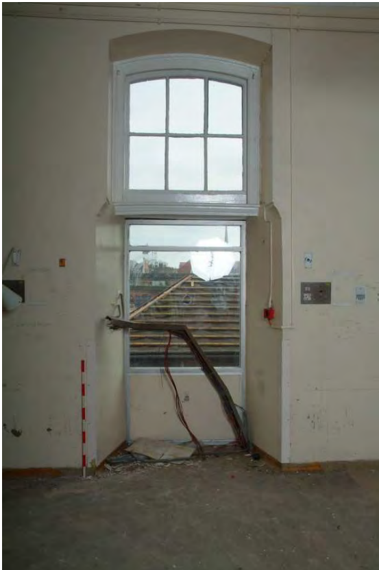
Plate 24.83: Building 24: Wheeley Lea Ward [Room 1.35] showing redundant fire exit, view to the south
