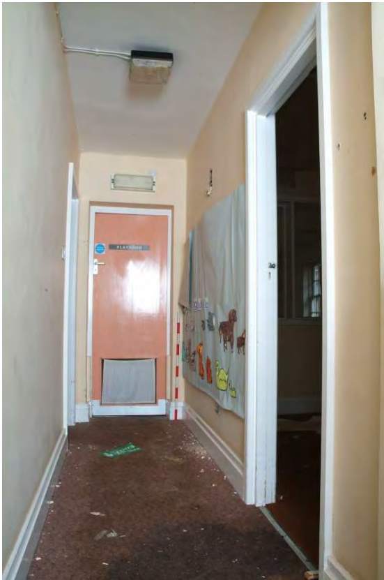
Plate 31.15: Building 31 (GF): inserted corridor between dining and sitting room leading to southern extension, view to the south
