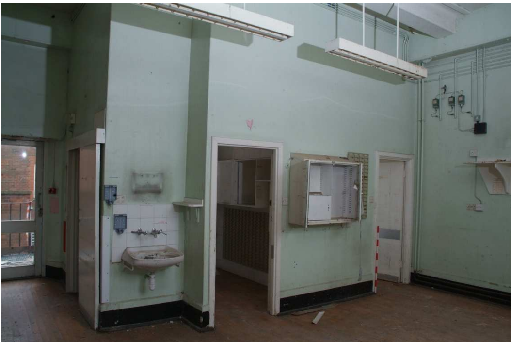
Plate 24.164: Building 24 (FF): inserted 1940s partitions at west of Garlick Ward, view to the southwest
