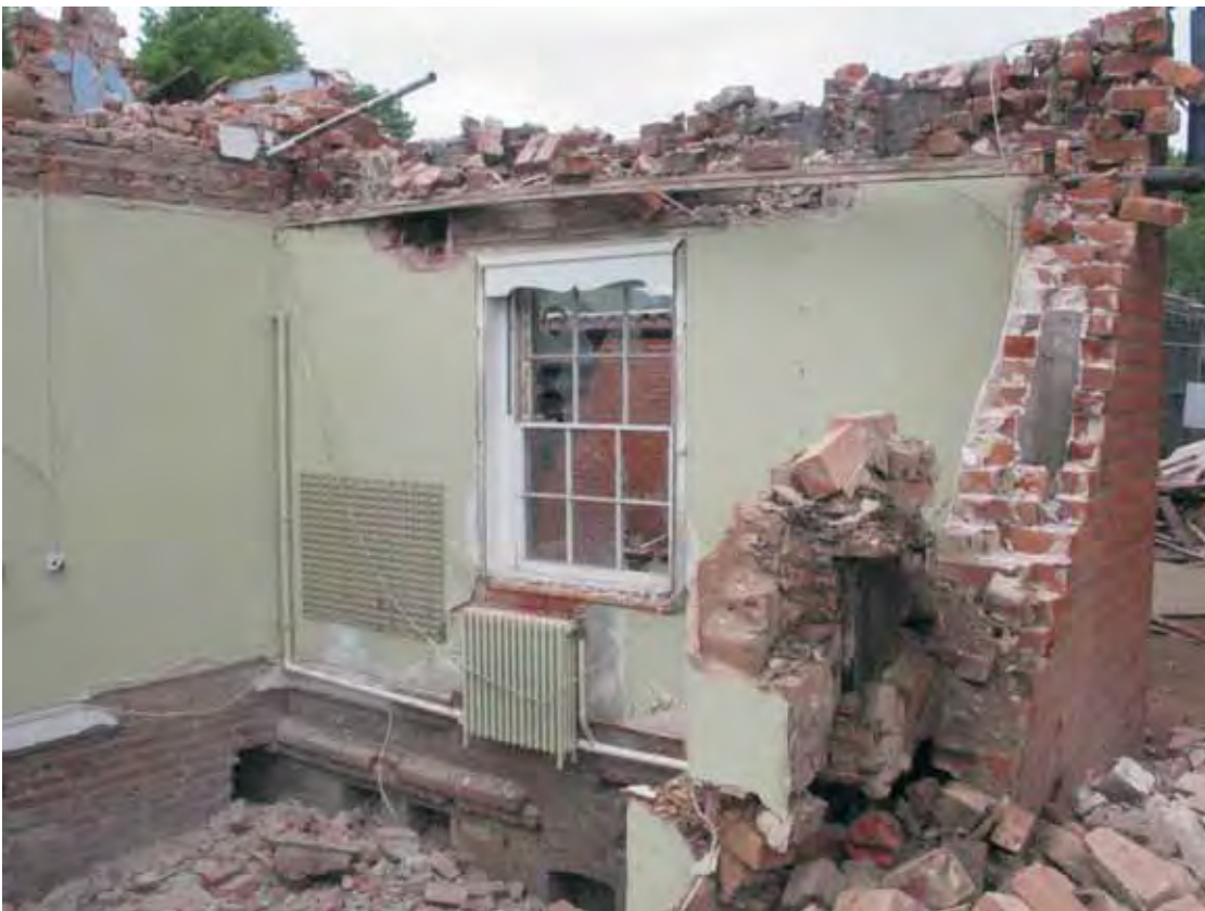
Plate 18.26: Building 18 – demolition of lower storey showing plaster lined shafts within the north and east walls, view to the northwest
