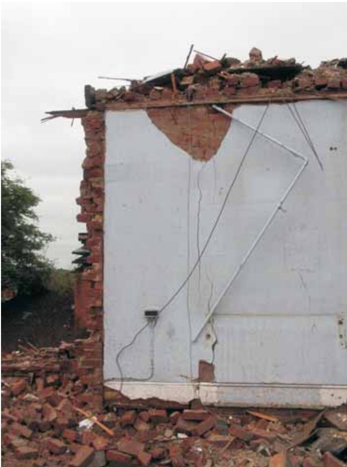
Plate 18.17: Building 18 – ground floor: exposed vousoir of the former opening between the west wing and the duty room, view to the north
