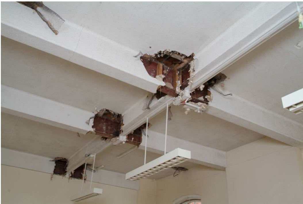
Plate 24.86: Building 24: Wheeley Lea Ward [Room 1.35], showing first floor structure in eastern extension (Building 24f), view to the northeast
