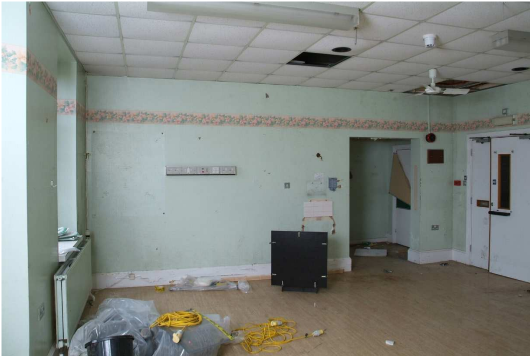
Plate 27.25: Building 27a – ground floor: typical room to the north of the entrance hall, view to the north
