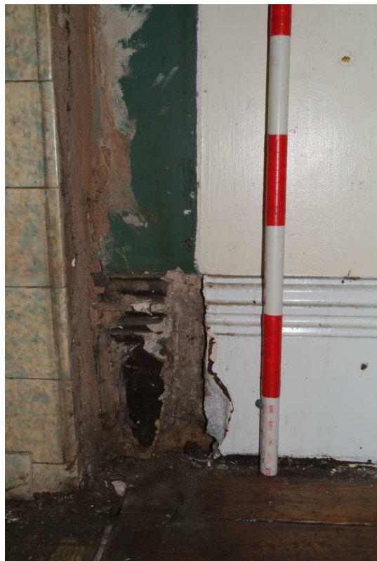
Plate 43.38: Building 43 – ground floor: detail of historic paintwork and skirting preserved beneath later fire surround, view to the east
