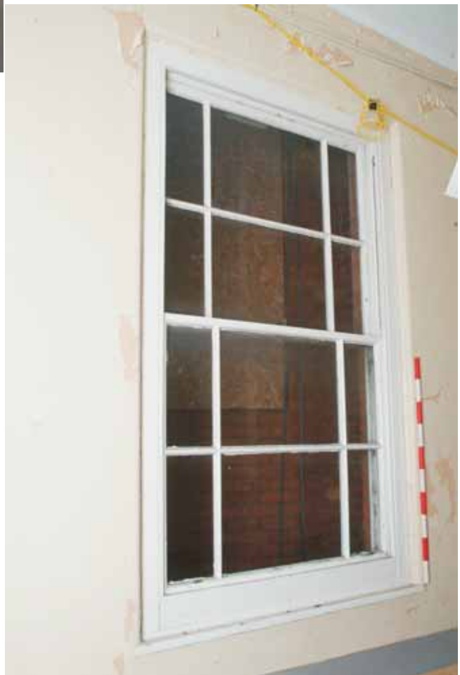
Plate 17.24: Building 17a – ground floor: detail of typical original corridor window, view to the northeast
