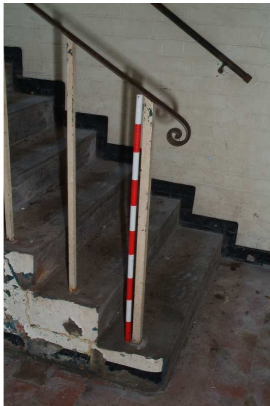
Plate 43.44: Building 43 – basement: detail of balustrade at foot of basement steps, view to the southeast
