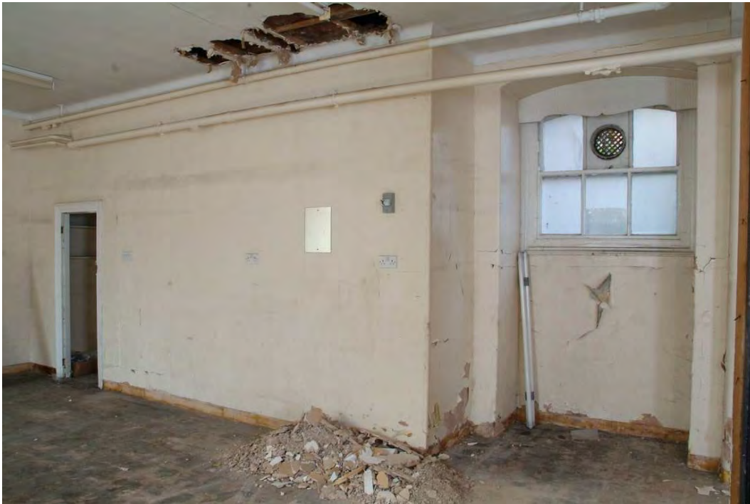
Plate 24.101: Building 24 (LGF): nursing staff changing area [Room 109] showing blocked cooking range, view to the northwest
