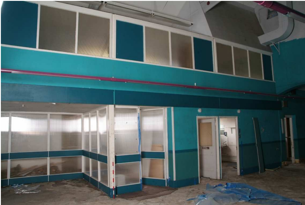
Plate 41.7: Building 41: former street entrance enclosure and inserted offices below mezzanine, view to the northeast
