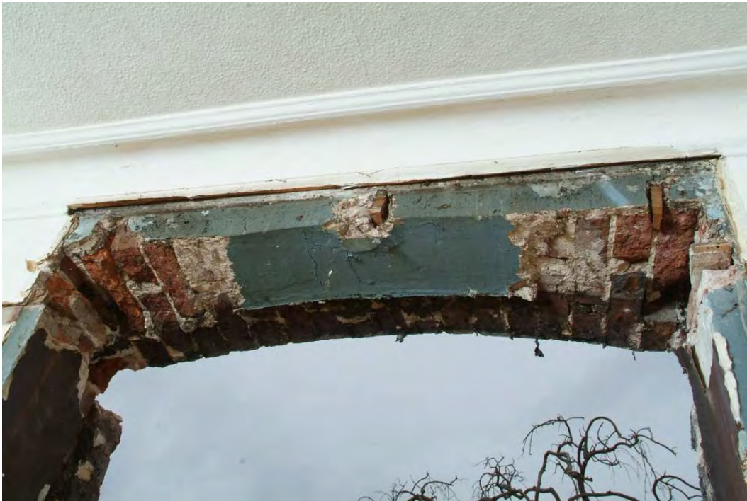
Plate 30.57: Building 30 (GF): reshaped window opening and earlier paint decoration in northwest room, view to the northeast
