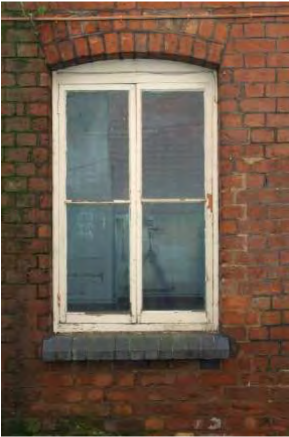
Plate 34.4: Building 34 – detail of window in the western part, view to the south
