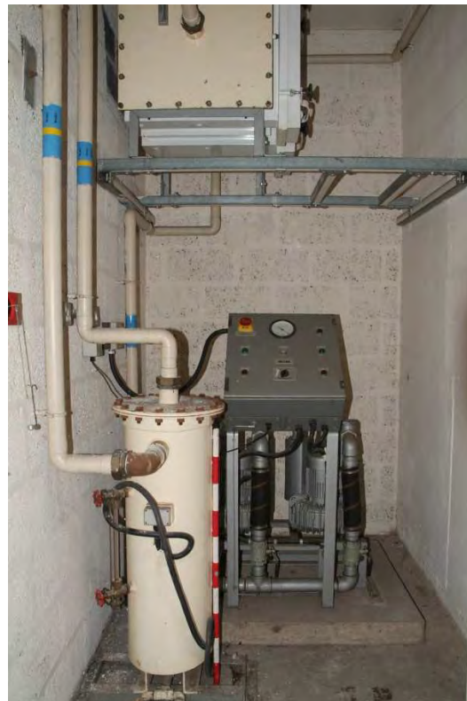
Plate 39.16: Building 39 - lower ground floor plant room, view to the east
