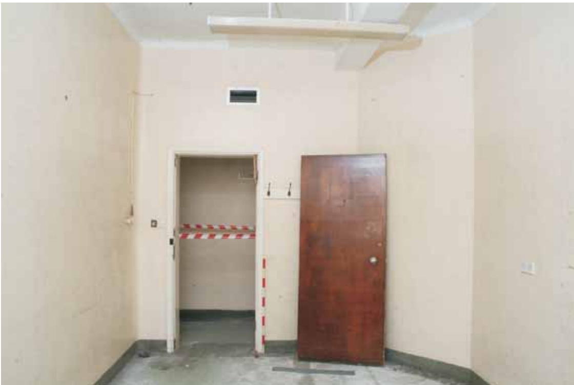
Plate 17.34: Building 17b – basement: interior of original consulting room within the VD clinic showing original door, view to the north
