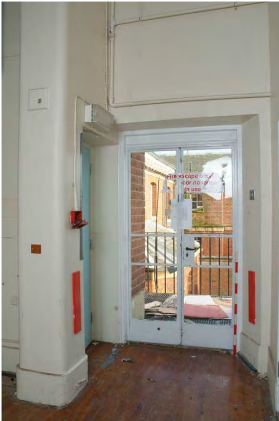
Plate 24.197: Building 24 (SF): inserted fire escape doors in west of Maddox Ward, view to the south
