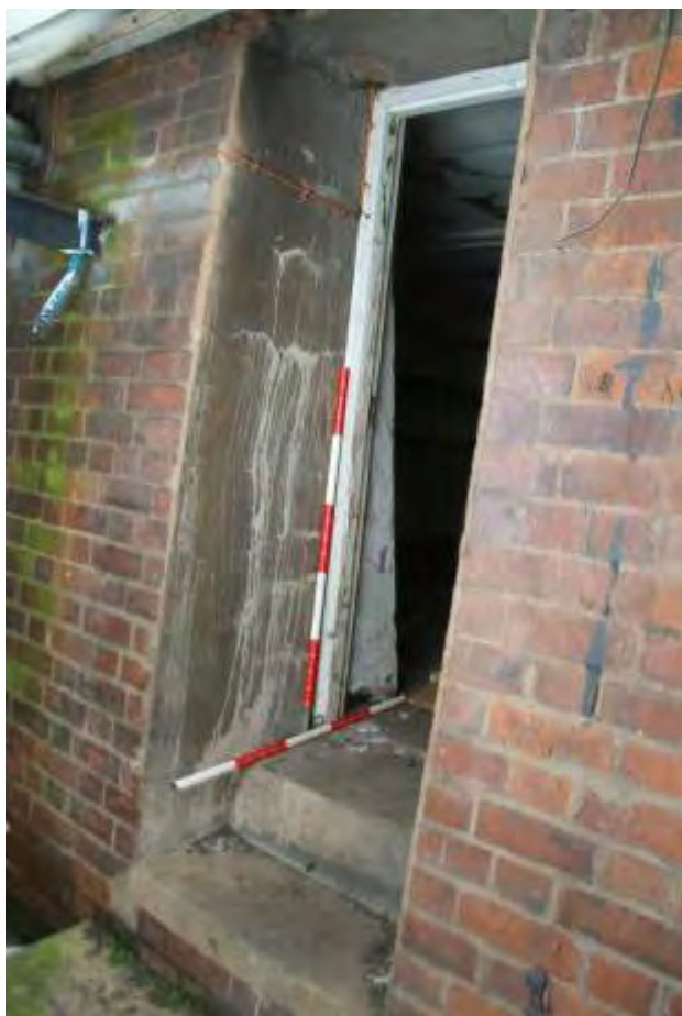
Plate 36.8: Building 36 – entrance in northern elevation showing steps to elevated floor level, view to the southeast
