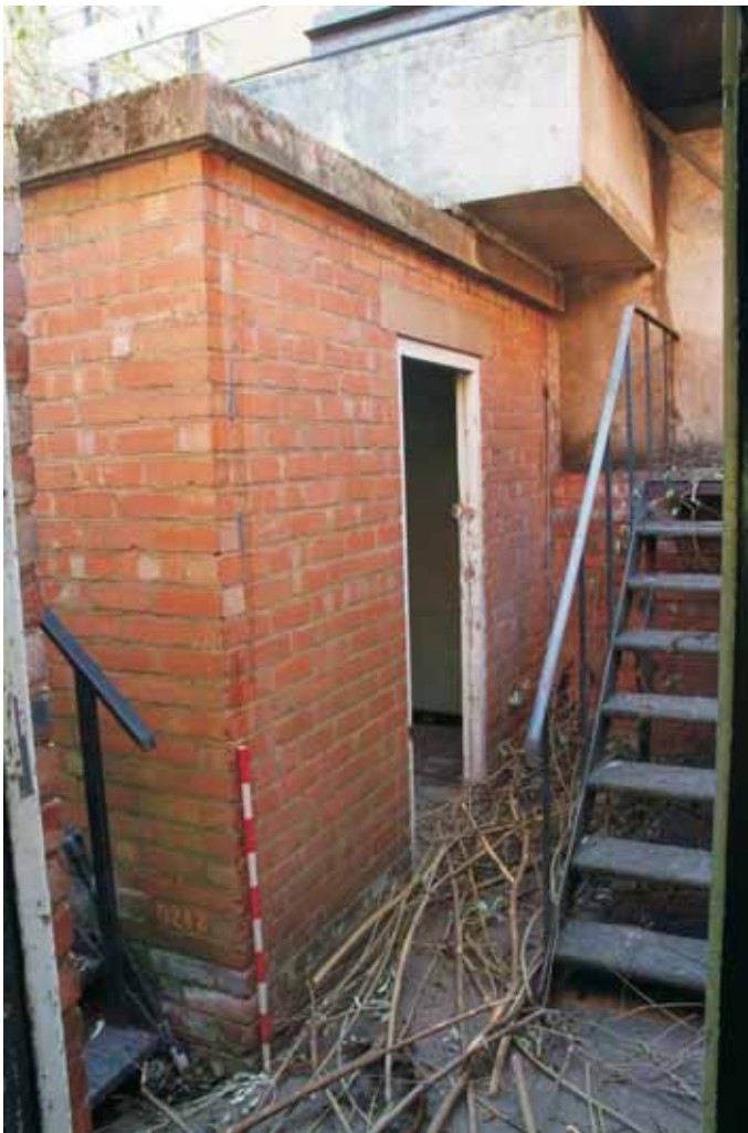
Plate 10.12: Building 10 – ancillary store and steps to elevated water tank to the south east of main building, view to the southeast
