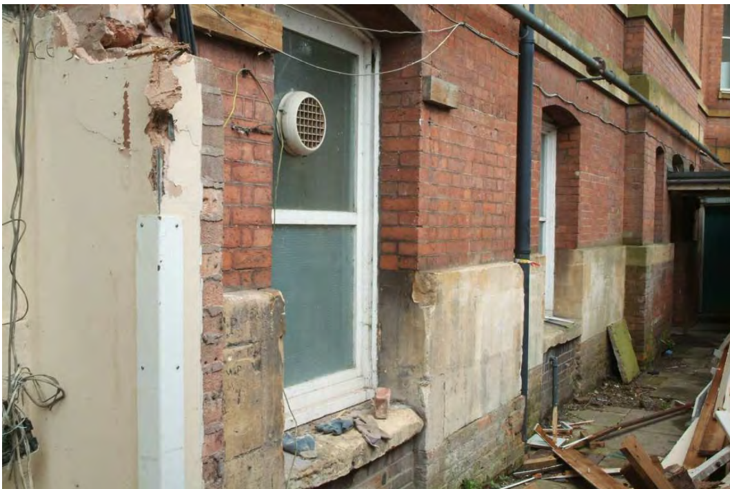
Plate 24.28: Building 24: southern elevation showing detail of right hand part of lower ground floor, view to the northeast
