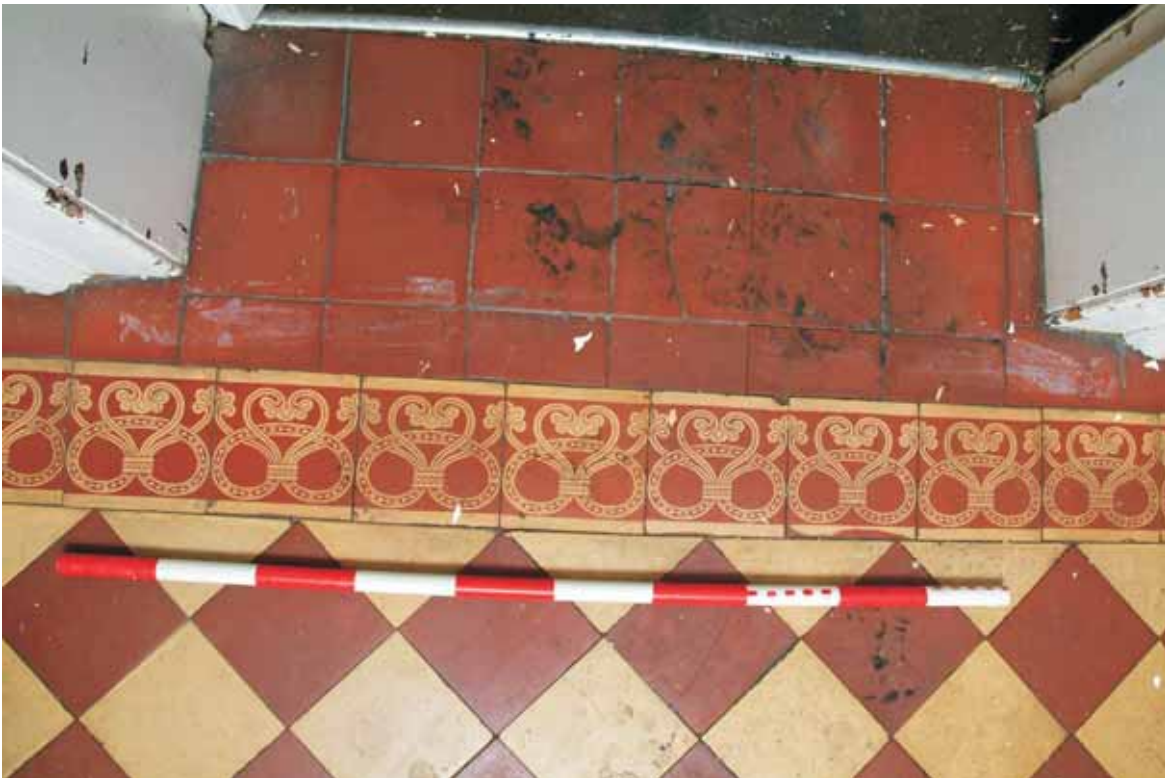
Plate 22.37: Building 22 – connecting range: central corridor on upper ground floor showing detail of floor tiles, view to the north
