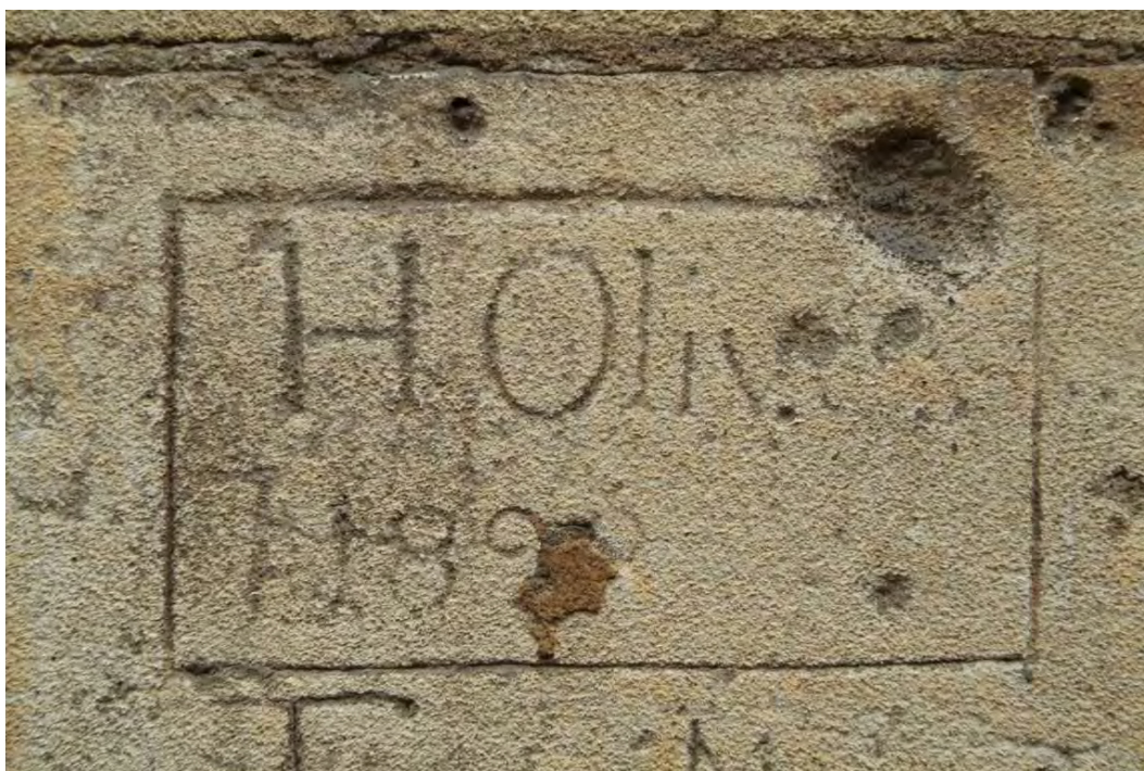
Plate 24.34: Building 24: southern elevation showing detail of graffiti on lower ground floor of original building (Building 24a)
