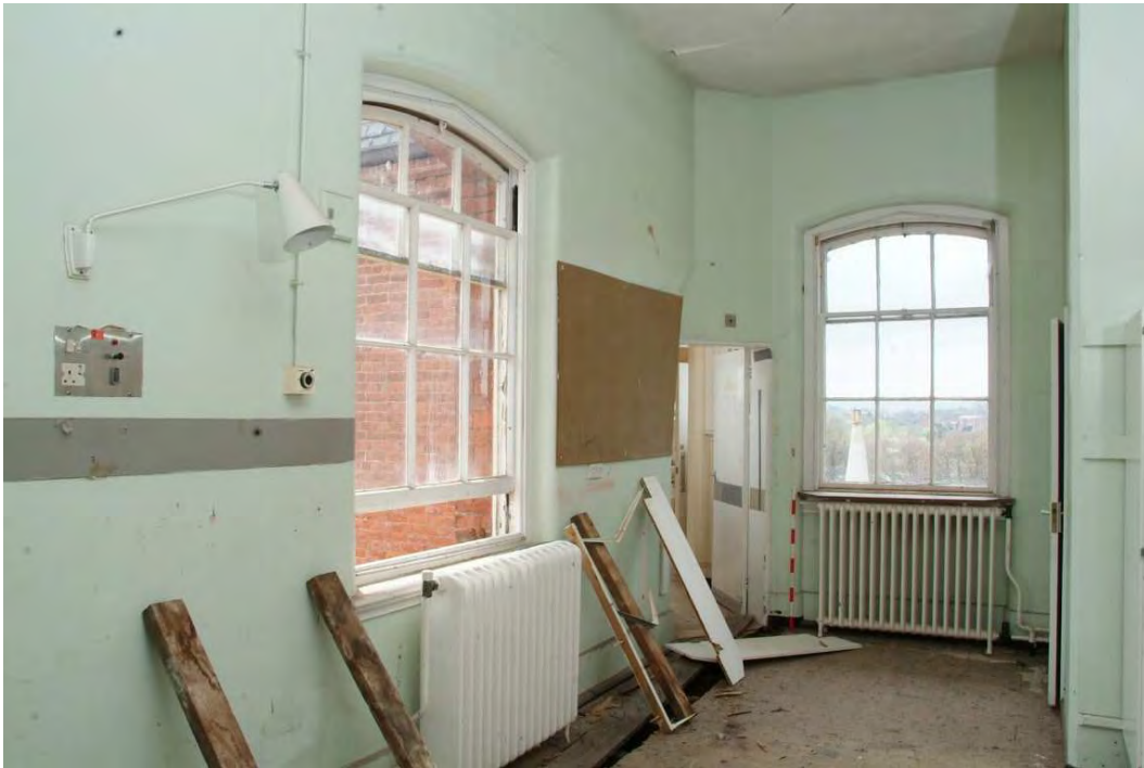
Plate 24.213: Building 24 (SF): western part of Bonaker Ward showing subdivision and entrance to the southwest corner tower, view to the southwest
