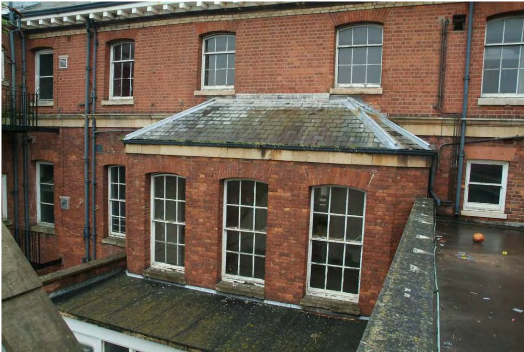
Plate 24.21: Building 24: detail of central part of western elevation showing canted bay, view to the northeast
