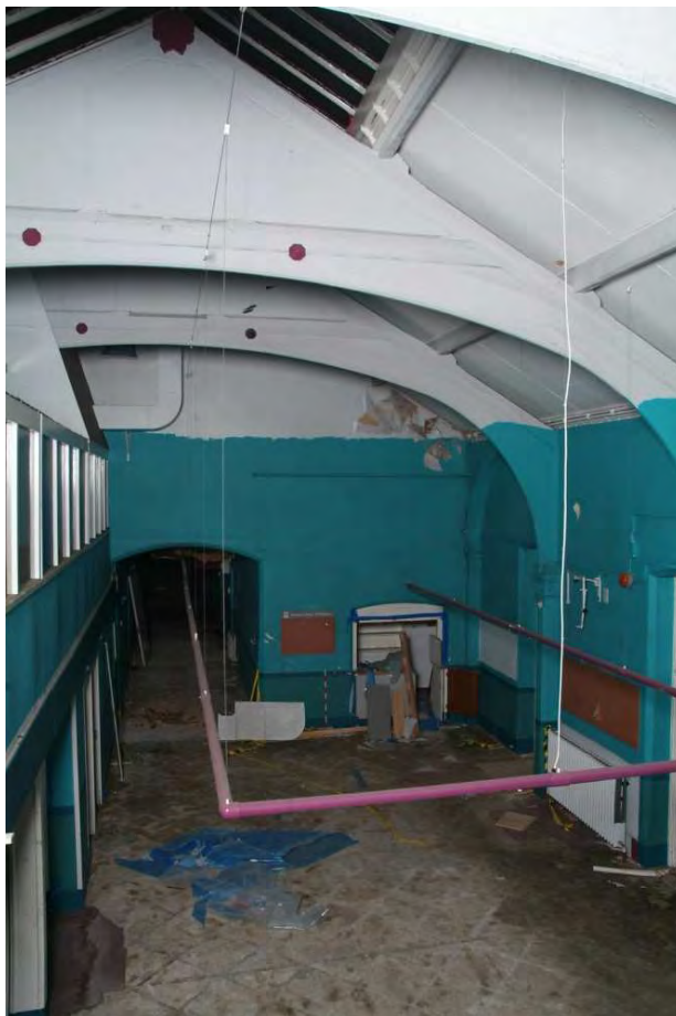
Plate 41.6: Building 41: general view of the interior from mezzanine, view to the east
