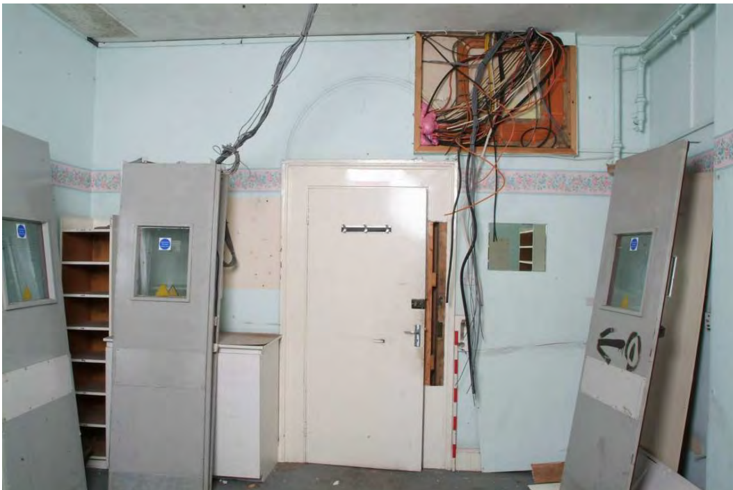
Plate 24.136: Building 24 (LGF): interior of office [Room 88] showing blocked head, view to the west
