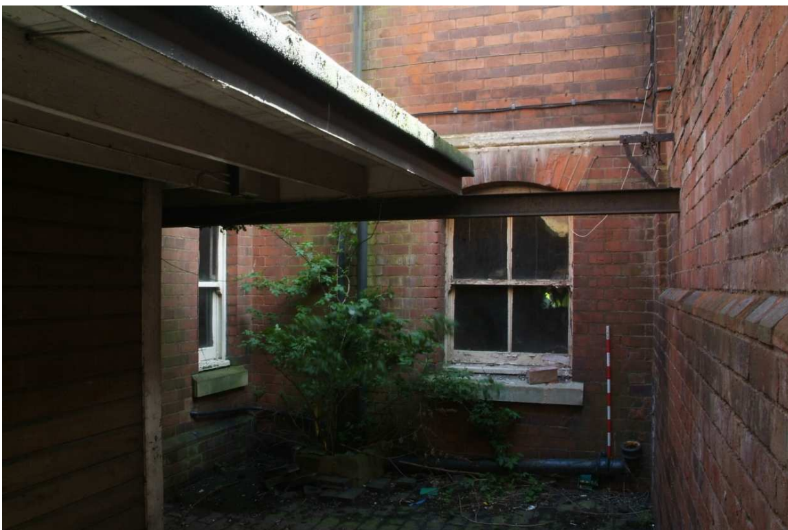
Plate 43.12: Building 43 - basement window to the west of the porch, view to the south
