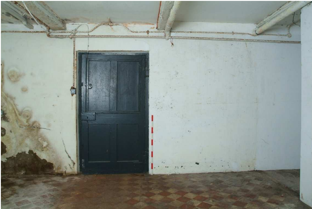
Plate 30.27: Building 30 (LGF): westernmost part of original basement showing original door to central room, view to the east
