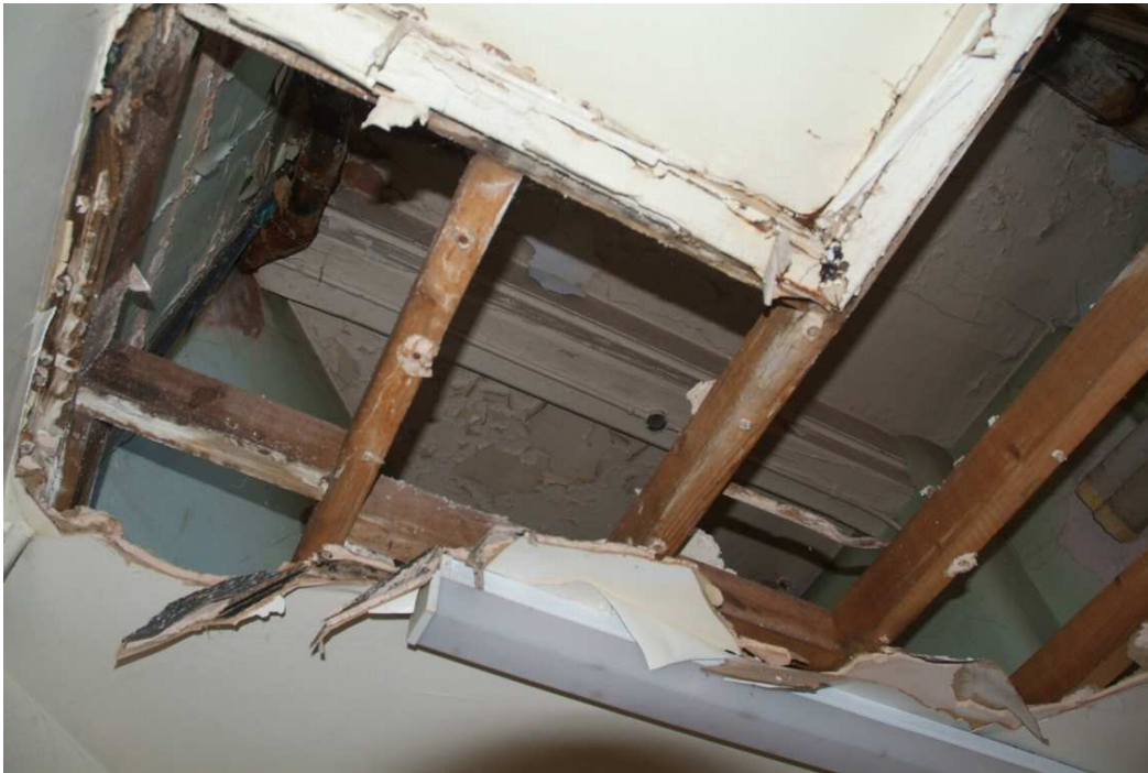
Plate 24.181: Building 24 (FF): exposed joist carrying 3rd floor over closet wing opening, view to the southwest
