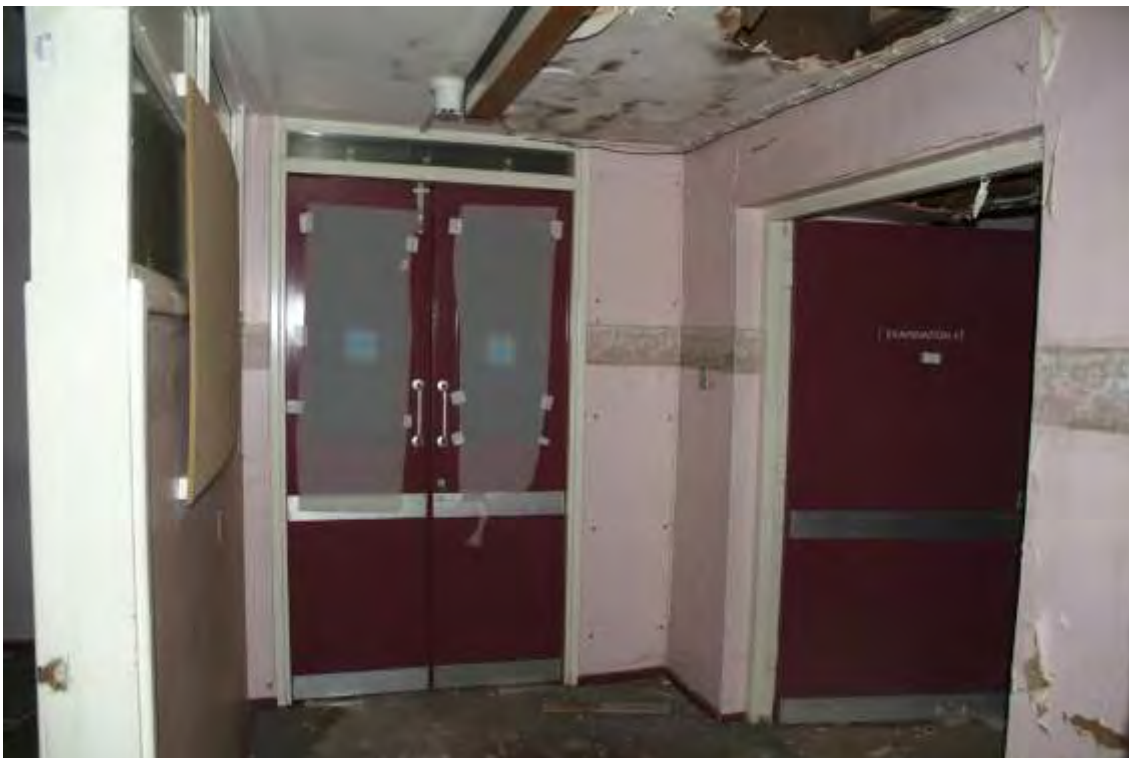
Plate 41.23: Building 41 – ground floor - corridor along south showing opening through original infirmary wall to Room 61, view to the southeast
