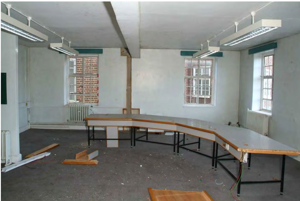
Plate 27.68: Building 27b – first floor: converted and refurbished bedrooms, view to the northeast
