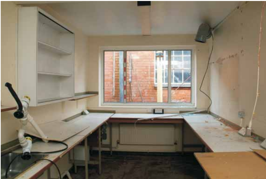
Plate 7.6: Building 7 – interior of typical room showing plastic ducting, view to the east
