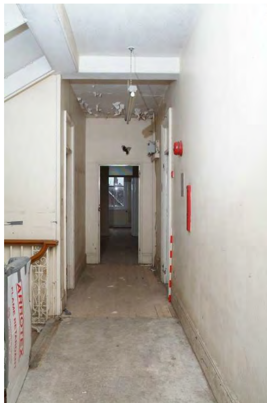
Plate 43.52: Building 43 - first floor: original opening to southern range, view to the south
