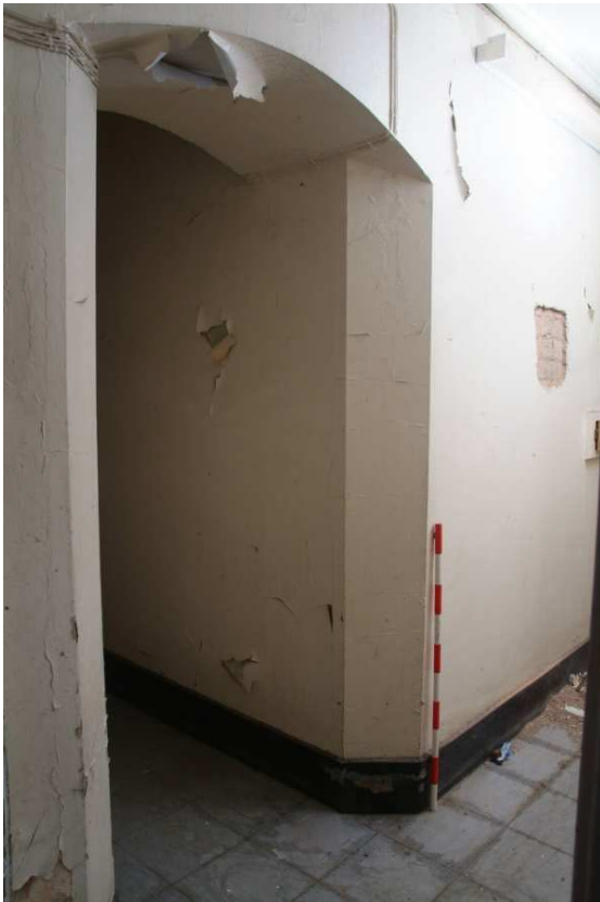
Plate 24.107: Building 24(LGF): original opening in southern elevation of Building 24f, view to the northeast
