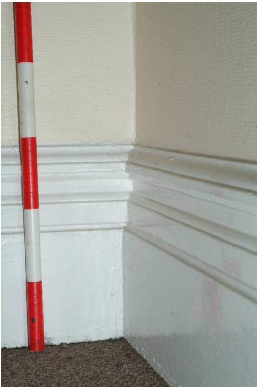
Plate 43.25: Building 43 – ground floor: detail of skirting in lounge, living room and sitting
