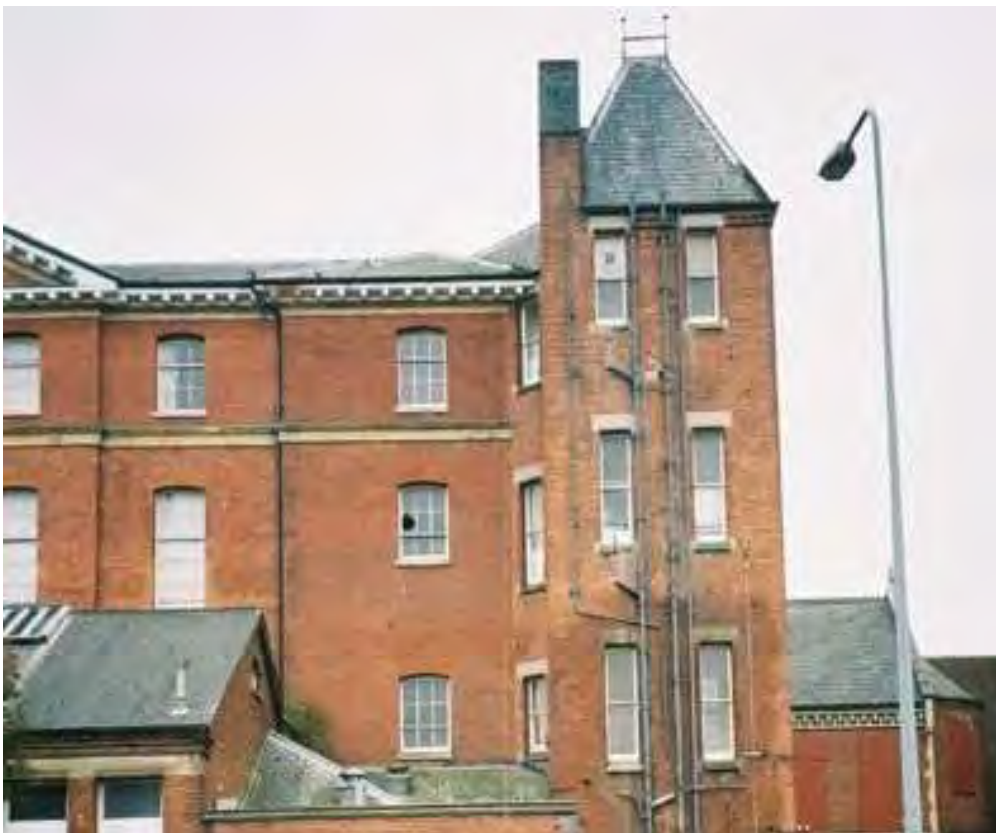
Plate 24.18: Building 24: detail of north western extension (Buildings 24b and 24g) showing vertical and horizontal changes in brickwork
