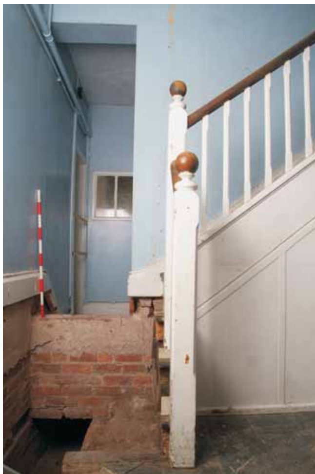
Plate 18.15: Building 18 – ground floor: inserted opening in western wall of the stair well, view to the west
