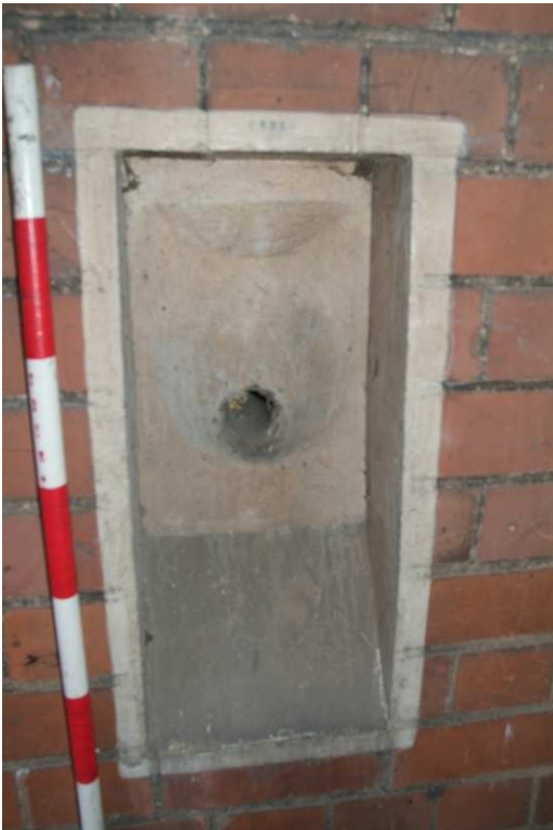
Plate 43.13: Building 43 – detail of former bell pull rebate to west of basement door, view to the southeast
