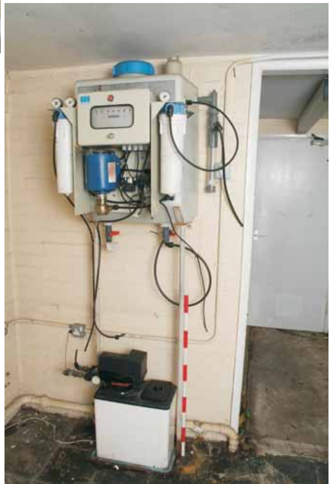
Plate 20.6: Building 20 – detail of effluent scrubber in northern hut, view to the northeast
