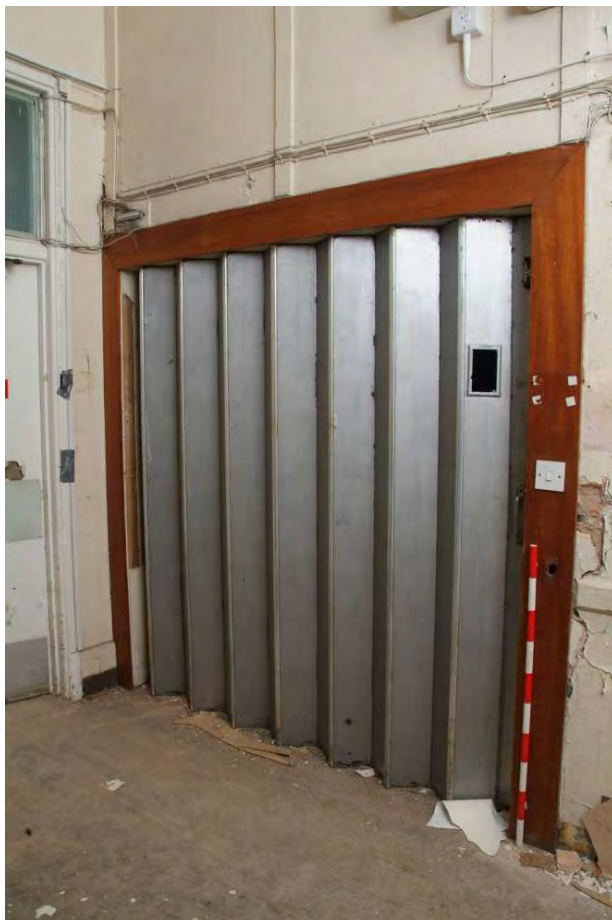
Plate 24.154: Building 24 (FF): detail of northern lift and surround, view to the northeast
