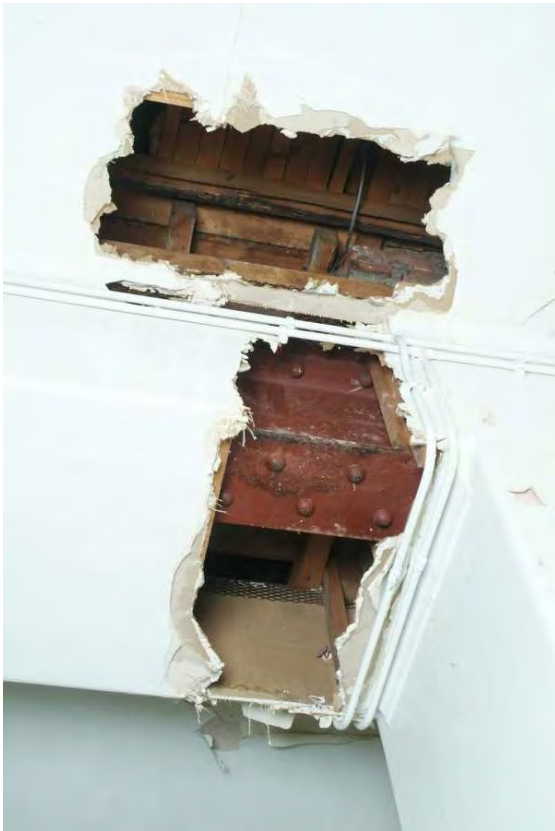
Plate 24.63: Building 24: Rushout Ward [Room 1.11] showing detail of riveted beam, view up and to the northwest
