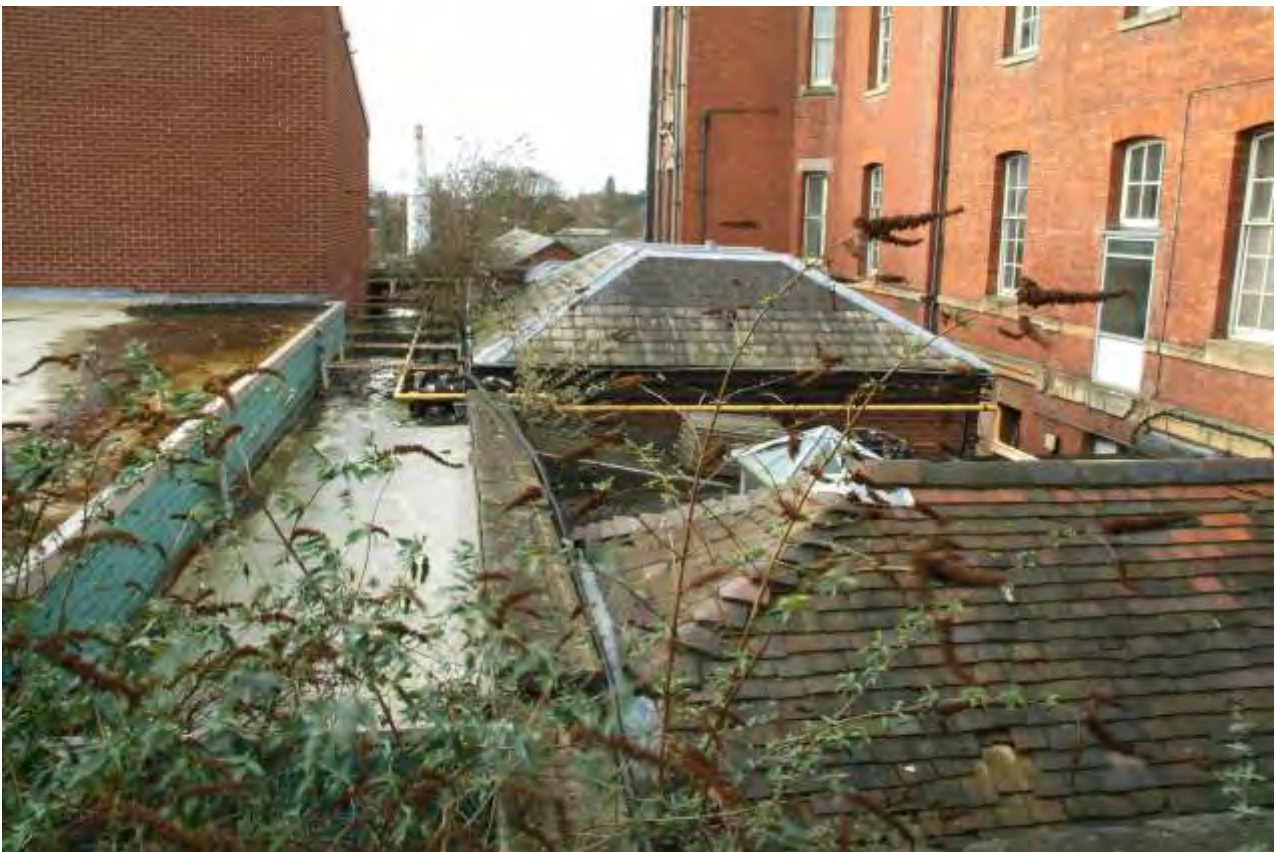
Plate 46.5: Building 46 - capping of wall between Buildings 49 (left) and 35/ 23, view to the east
