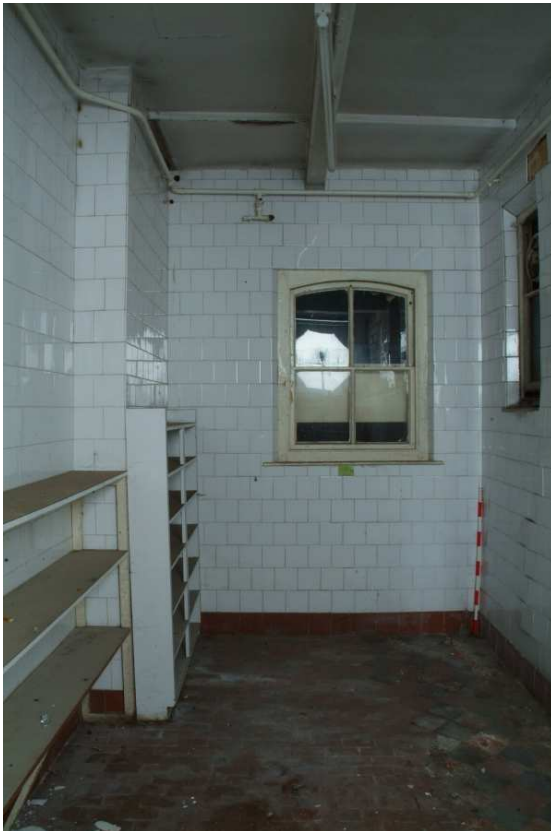
Plate 24.121: Building 24 (LGF): interior of northern annex to kitchens [Rom 105], view to the west
