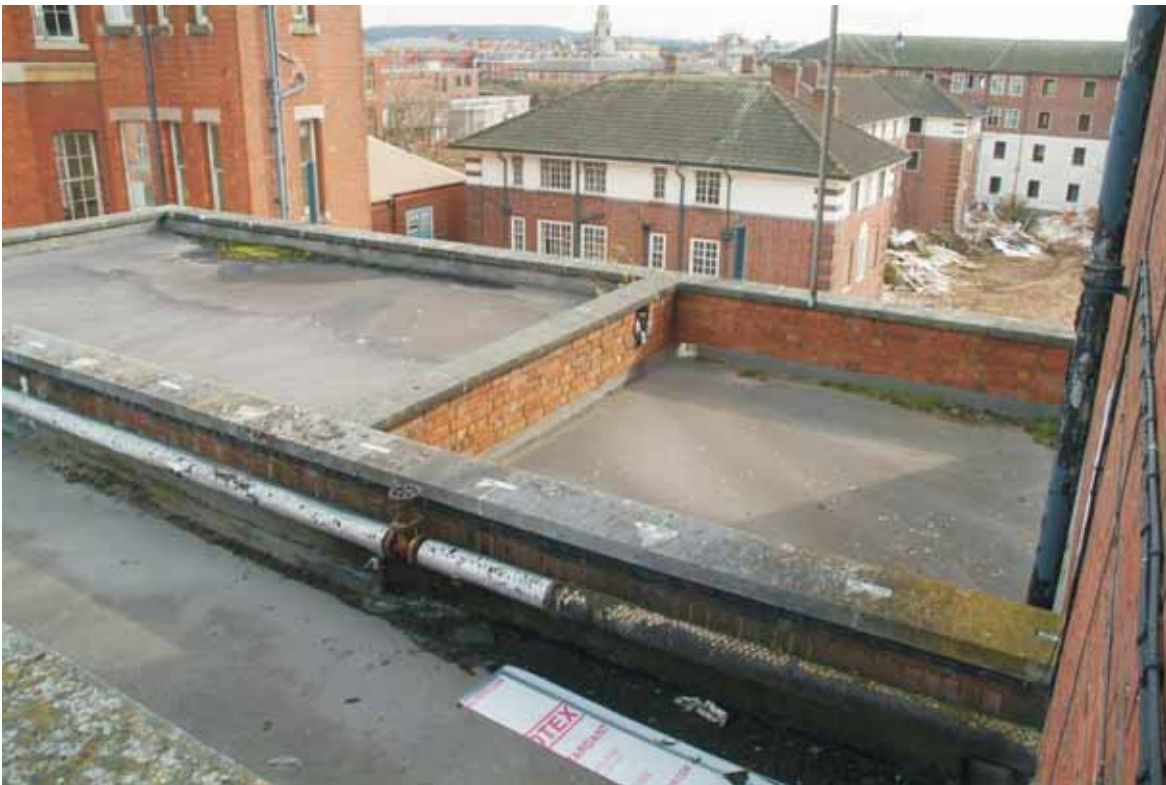
Plate 16.4: Building 16 – roof showing later extension to the left, view to the southeast
