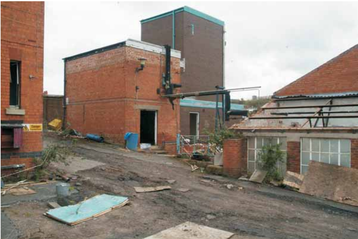
Plate 11.1: Building 11 and 12 – view to the southeast showing structures in relation to Building 18 (far left), Building 26 (behind) and Building 10 (far right)
