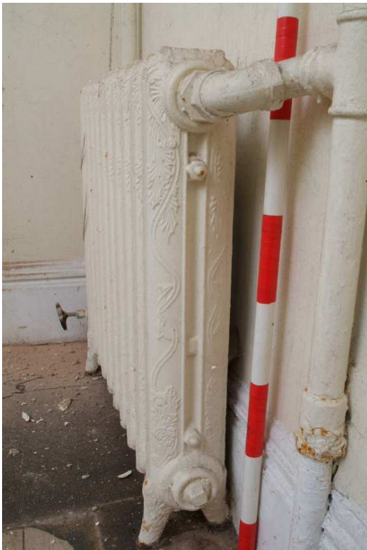
Plate 43.59: Building 43 - first floor: detail of historic, possibly original radiator in bathroom of the central range, view to the south
