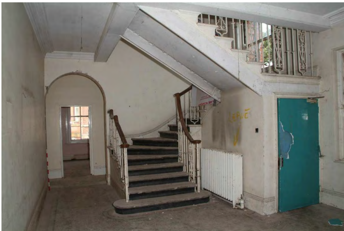
Plate 43.18: Building 43 – ground floor: entrance hall showing formerly blocked opening to the north range and entrance basement, view to the north
