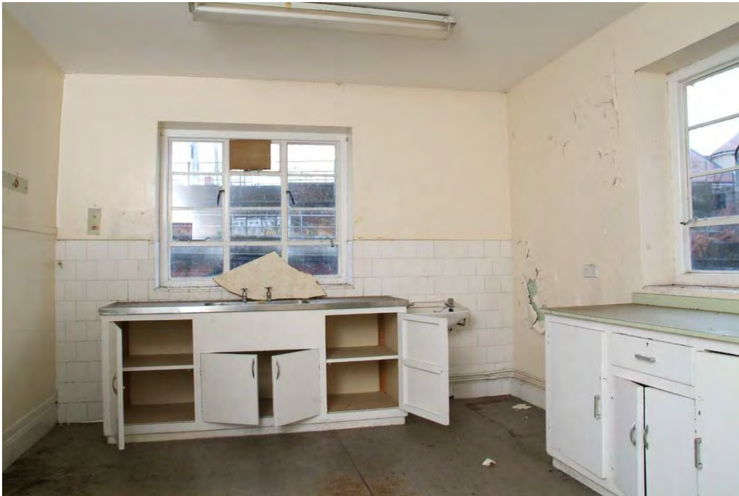
Plate 30.23: Building 30 (GF): kitchen in mid 19th century extension to southwest wing, view to the south
