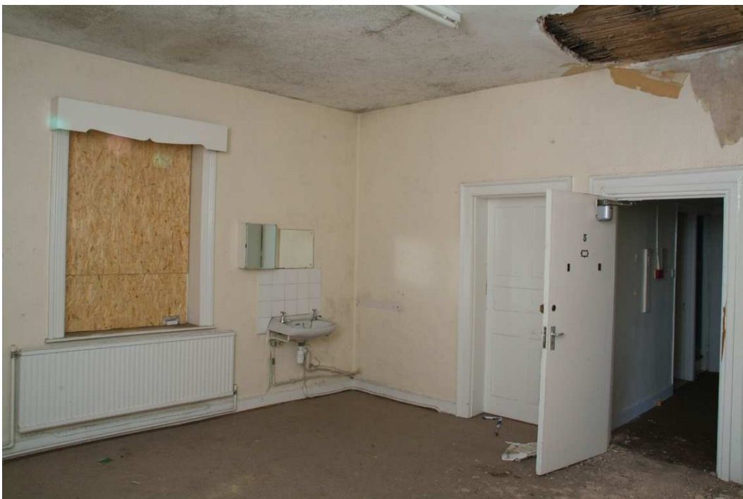
Plate 30.40: Building 30 (FF): northwest principal room showing blocked connecting door to bathroom, view to the northeast
