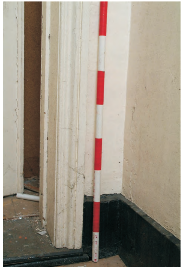
Plate 22.46: Building 22 – connecting range (LGF): detail of skirting within the central corridor and architrave to the contingency store, view to the southwest
