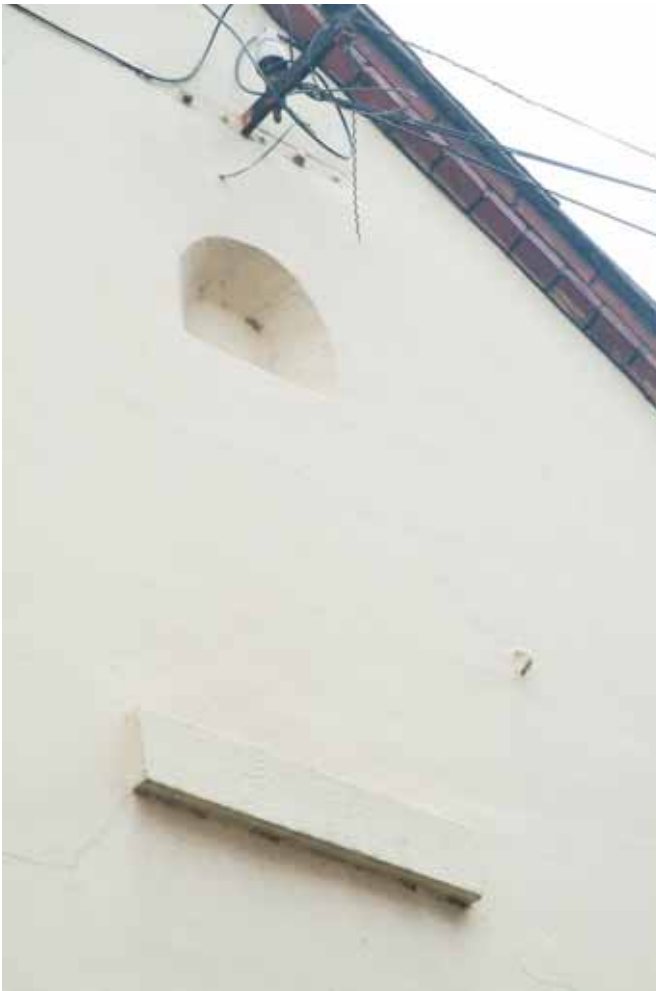
Plate 14.5: Building 14 – detail of rebate and drip moulding in central gable, view to the southwest
