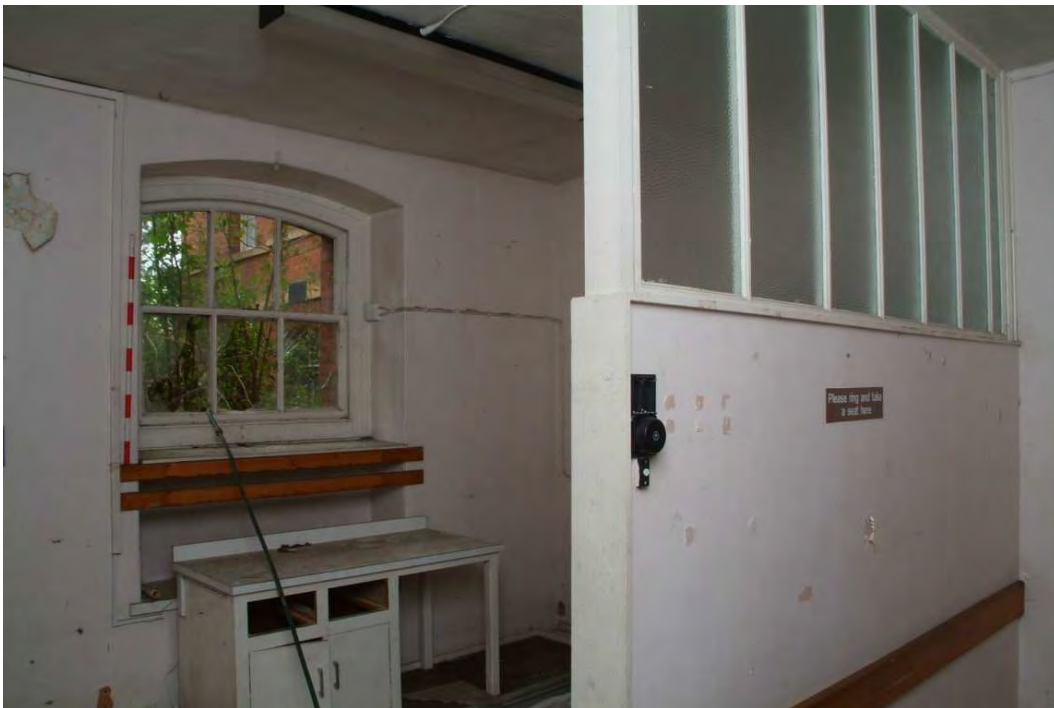
Plate 24.128: Building 24 (LGF): interior of 'Blood Sampling' [Room 102] showing inserted glazed partition, view to the southwest
