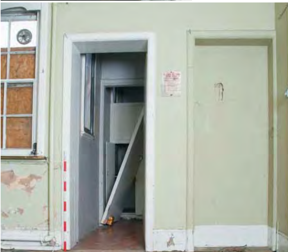
Plate 18.20: Building 18 – ground floor: southwest corner of eastern ward showing door to eastern closet and former entrance to duty room, view to the south
