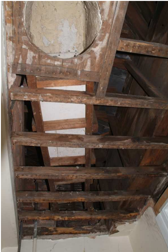
Plate 24.199: Building 24 (SF): ceramic conduit in roof above closet wing, view to the east
