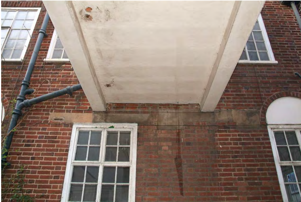
Plate 27.8: Building 27a – detail showing underside of the elevated corridor, view to the north
