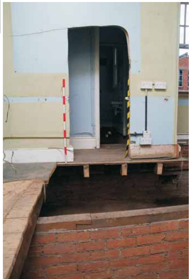
Plate 18.14: Building 18 – corridor inserted into the southeast corner of the west ward, view to the south
