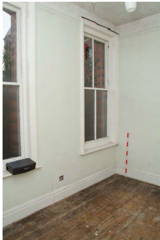
Plate 43.28: Building 43 – ground floor: typical details of former bedrooms in northern range, view to the northwest
