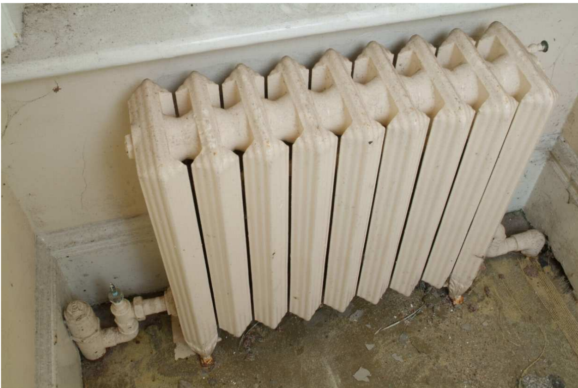
Plate 43.36: Building 43 – ground floor: detail of early 20 th century ideal radiator at west end of corridor, view to the south
