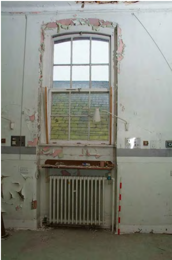
Plate 24.19: Building 24: detail of upper ground floor window in the northern elevation showing hopper light, view to the northwest
