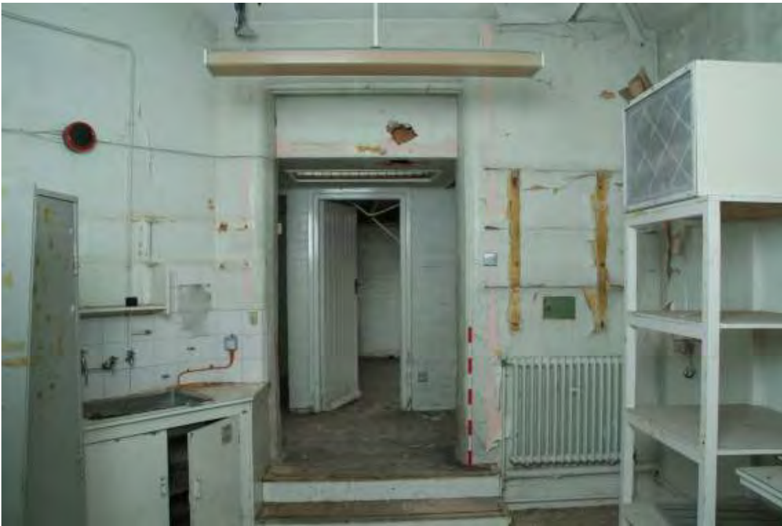
Plate 41.22: Building 41 – ground floor - office store looking through to Building 48, view to the west
