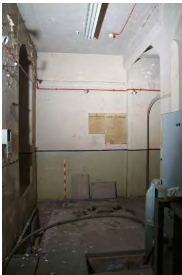
Plate 22.74: Building 22 (LGF): interior of northern side of the transformer room showing historic signage, view to the east
