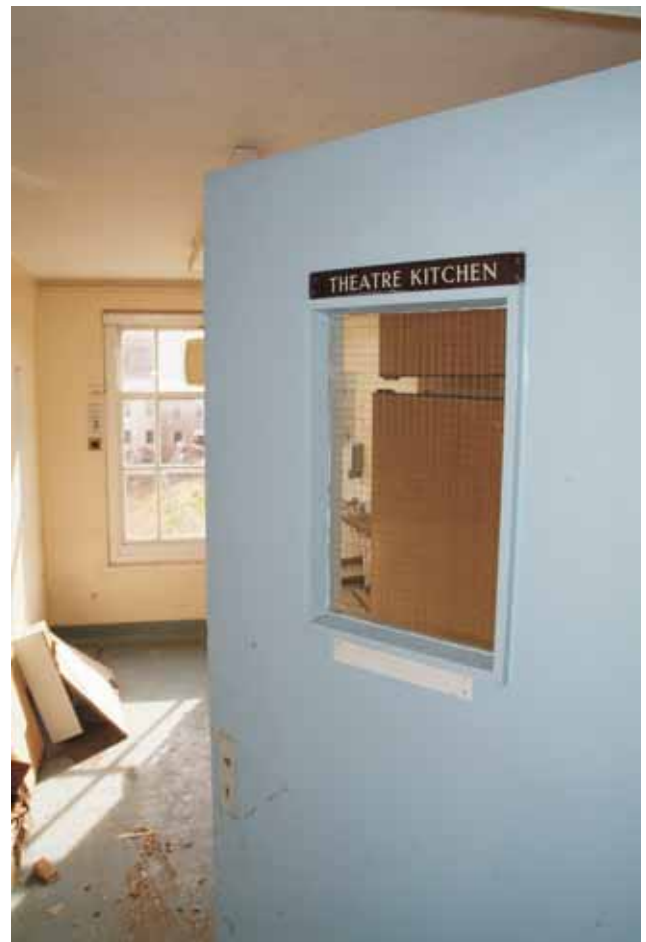
Plate 16.9: Building 16 – detail of original door with viewing panel and Bakelite signage, view to the south
