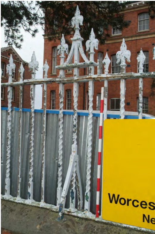
Plate 42.9: Building 42 – detail of railings to south of gates, view to the southwest
