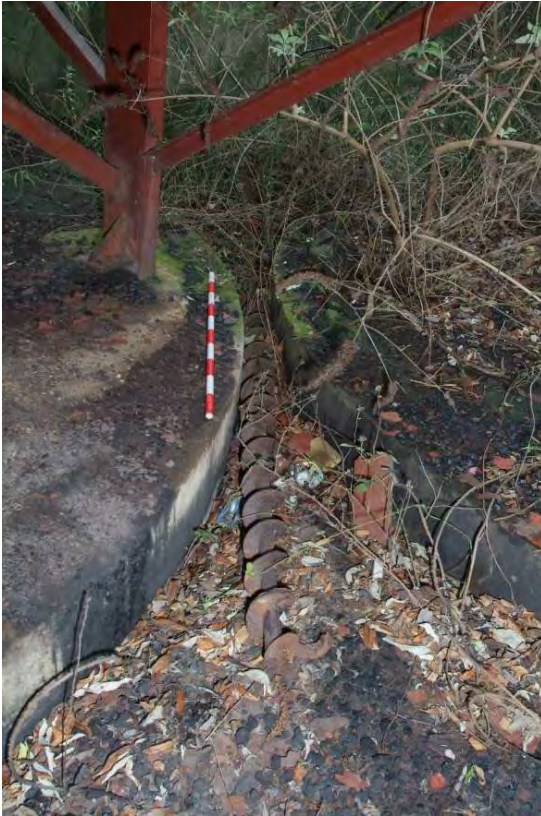
Plate 25.7: Building 25: foundation slabs for former oil storage tanks showing discarded screw, view to the south
