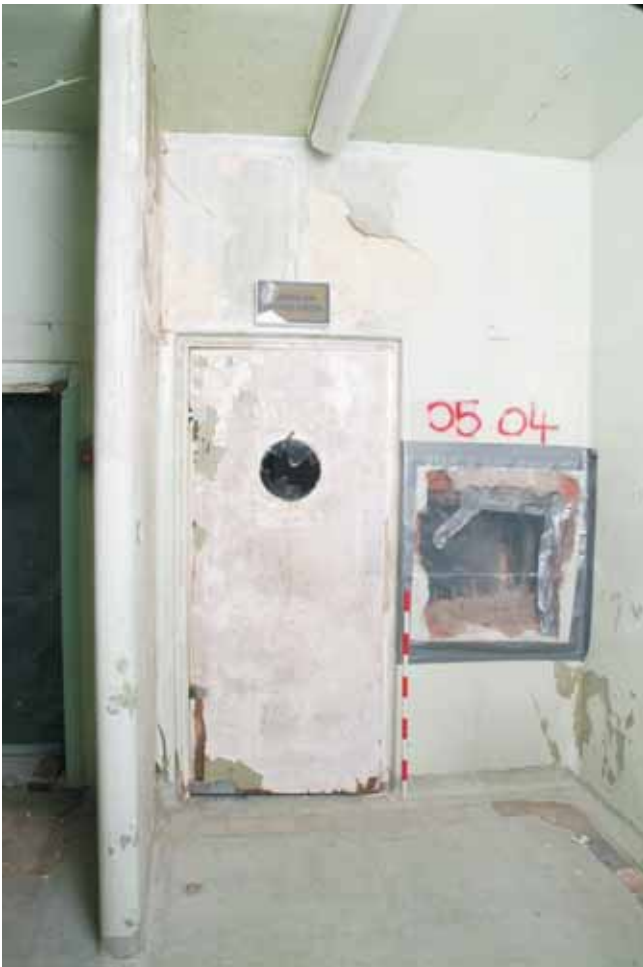
Plate 17.33: Building 17a – second floor: door from the sterilizing room to Theatre 1 with laser warning sign above, view to the west
