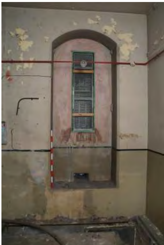
Plate 22.73: Building 22 (LGF): interior of transformer room showing modified window, view to the north
