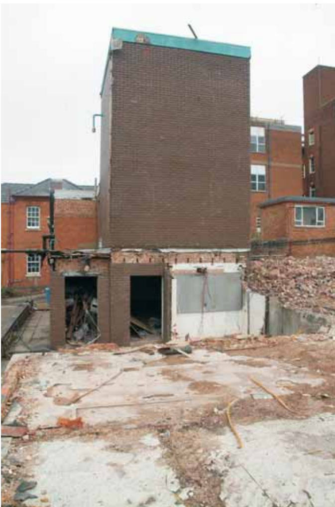
Plate 12.1: Building 12 – south elevation following the partial demolition of the single storey range
