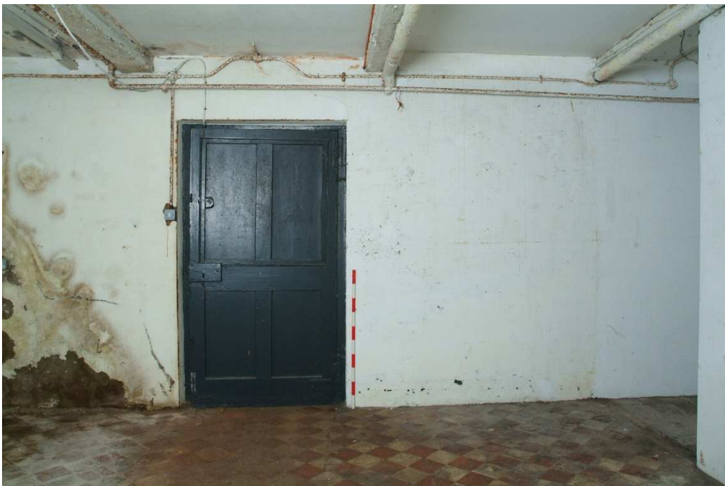
Plate 30.26: Building 30 (LGF): westernmost part of original basement showing inserted door and blocked fireplace, view to the south
