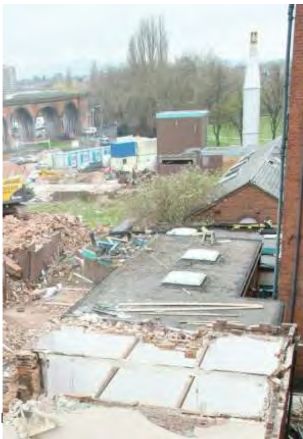
Plate 33.1: Building 33 – roof showing plan form and relationship to the southwest corner tower of the main infirmary, view to the west
