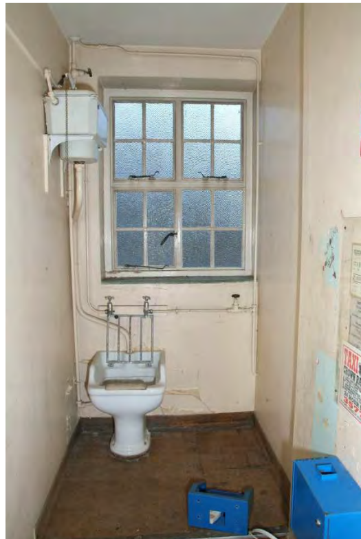
Plate 27.66: Building 27b – first floor: original sluice room and fittings, view to the south
