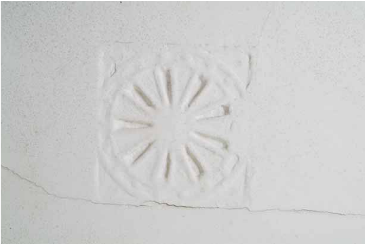
Plate 18.29: Building 18 – first floor: over-papered vent in ceiling of ward, view up
