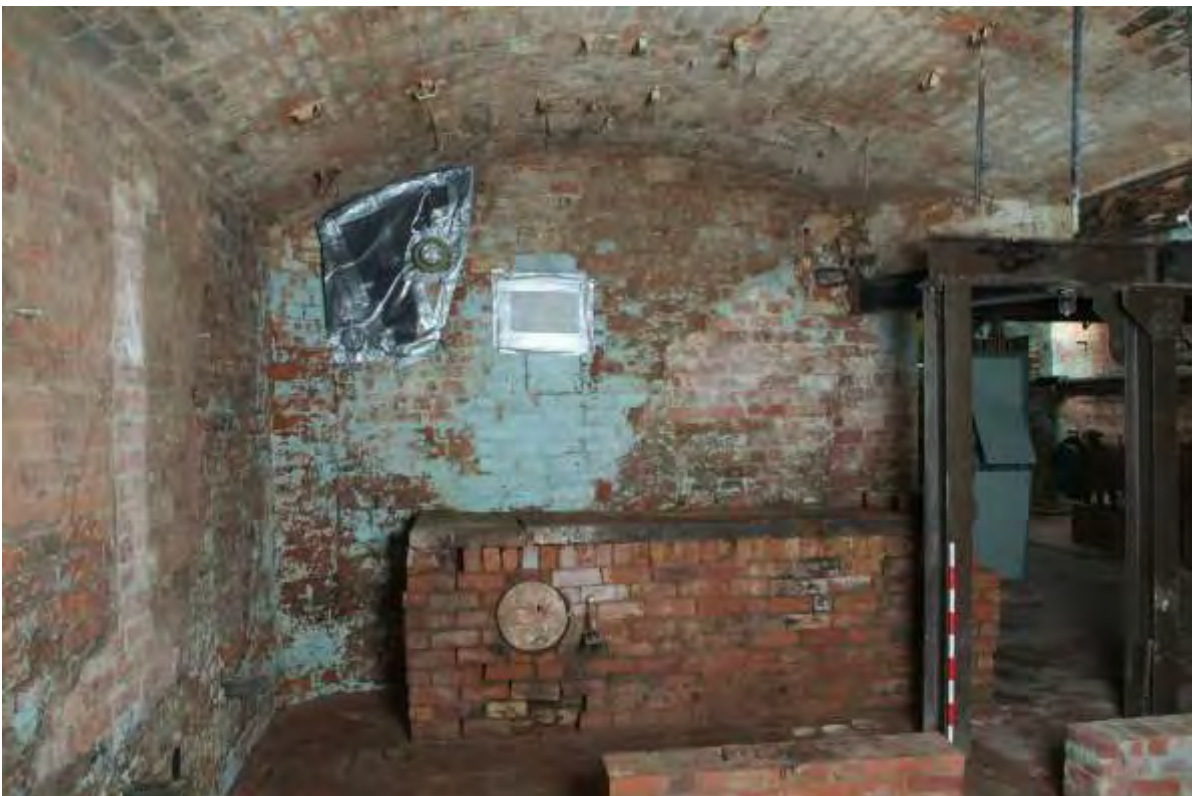
Plate 48.15: Building 48: basement – view of boiler exhaust manifold, view to the west
