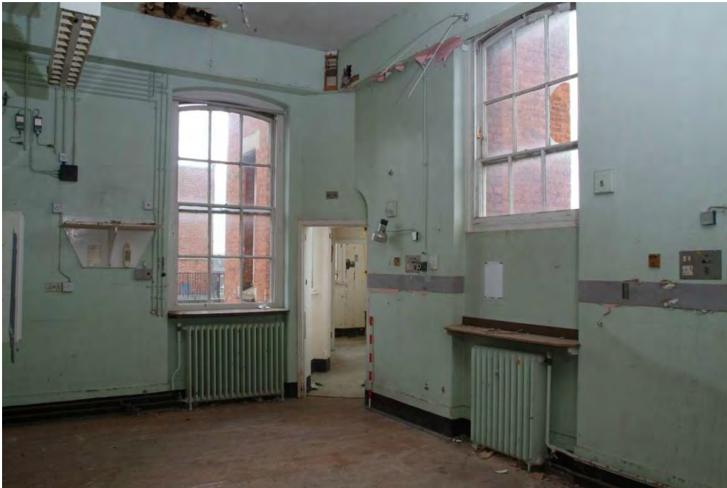
Plate 24.165: Building 24 (FF): west end of Garlick Ward showing short window (right), original window (left) and mis-aligned entrance to tower closet, view to the northwest
