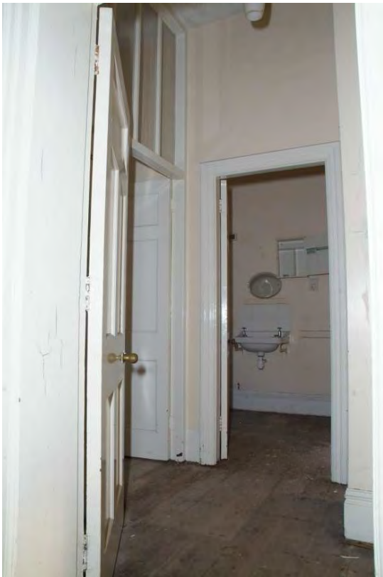
Plate 43.39: Building 43 – ground floor: inserted partitions in eastern room of southern range, view to the southeast
