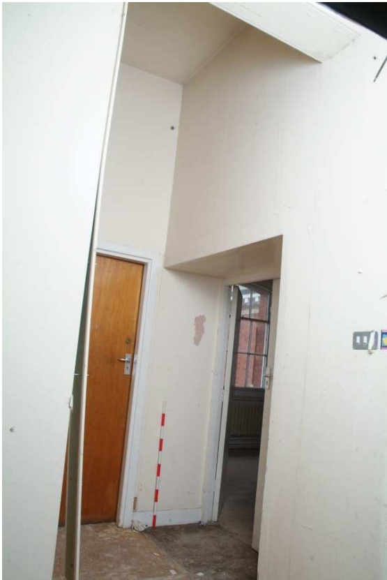
Plate 24.205: Building 24 (SF): inserted opening in the east wall of the central corridor and north wall of Room 3.24, view to the southeast
