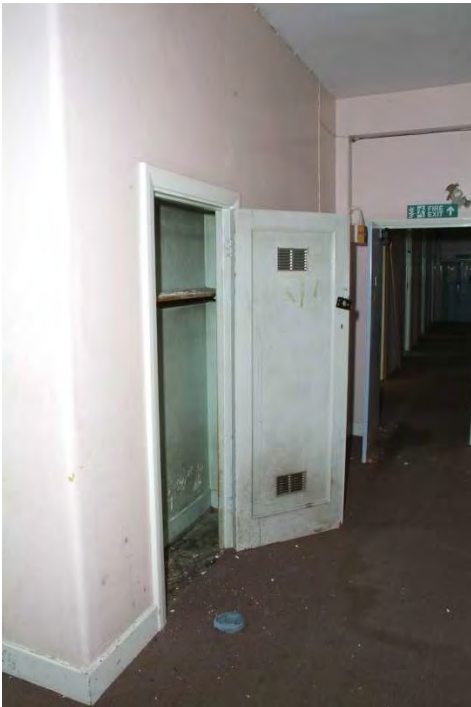
Plate 27.55: Building 27b – ground floor: storage cupboard with original door, view to the southwest
