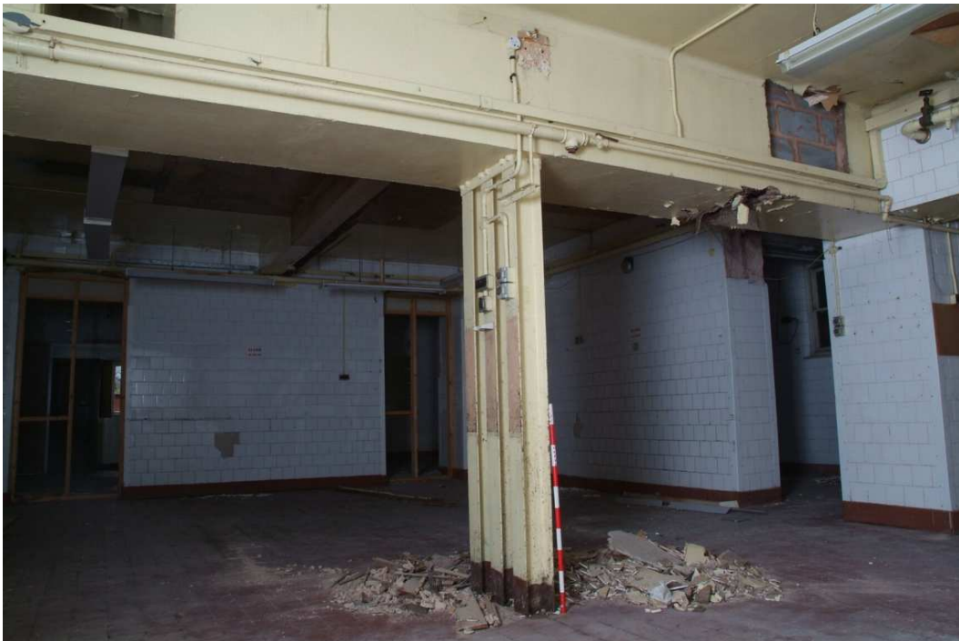
Plate 24.116: Building 24 (LGF): point of western extension to main kitchens, view to the northwest
