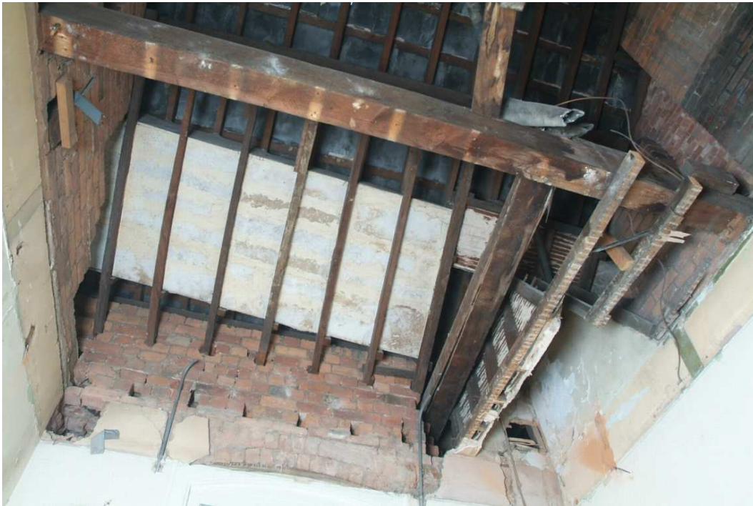
Plate 24.189: Building 24 (SF): historic roof structure following removal of false ceiling over northern stairwell, view to the northwest
