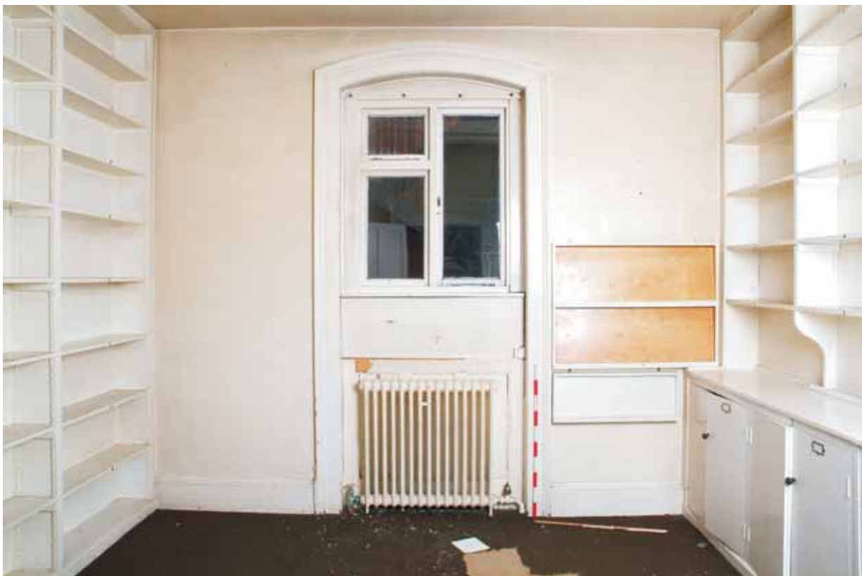
Plate 22.40: Building 22 – connecting range: medical library on upper ground floor, view to the north
