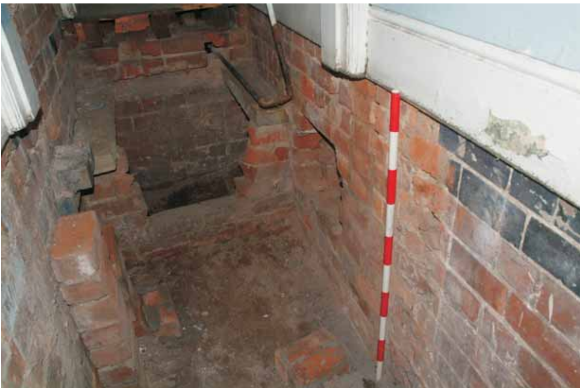
Plate 18.34: Building 18 – ground floor: foundation walls below floor in western closet wing showing truncated stub wall (left) and formerly external 'blue' brick, view to the northeast
