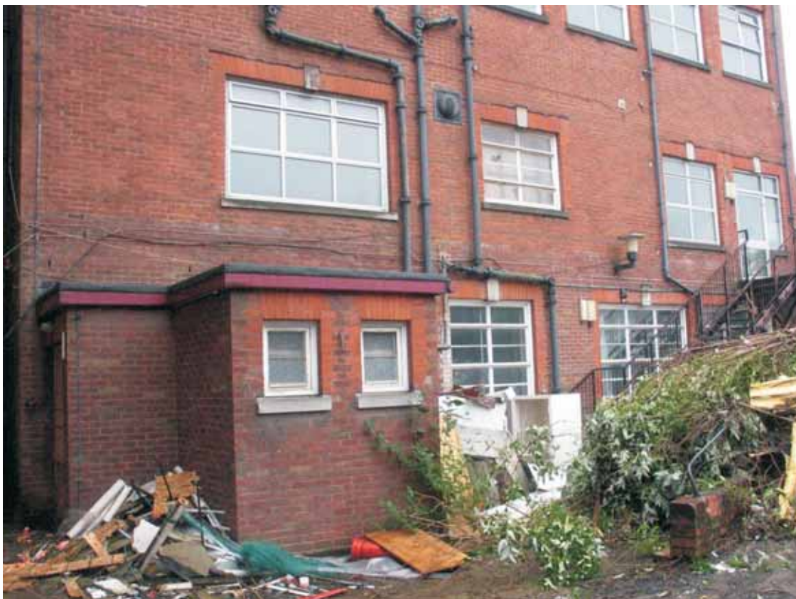
Plate 17.8: Building 17b – visible remnants of the VD Clinic showing northern lavatory wing and change in brickwork above ground floor, view to the southwest
