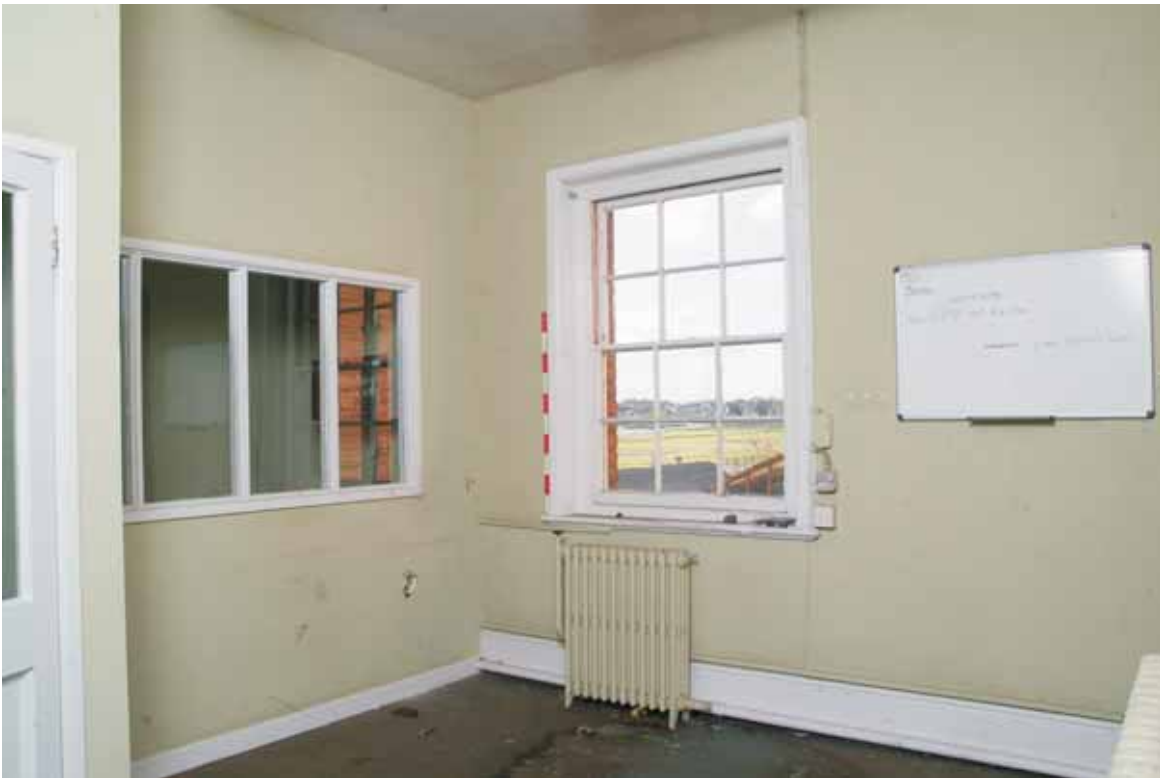
Plate 18.37: Building 18 – first floor: interior of eastern ward showing inserted partition, view to the northwest
