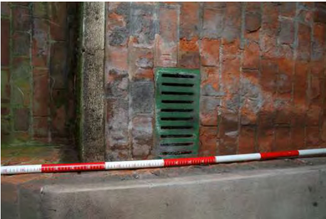
Plate 36.4: Building 36 – detail of original vent in eastern elevation, view to the west
