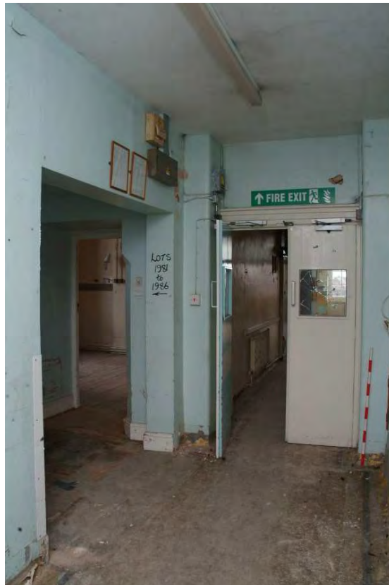
Plate 24.172: Building 24 (FF): southern part of central corridor showing inserted doorway (left) to sluice room [Room 2.24 and 25], view to the southeast
