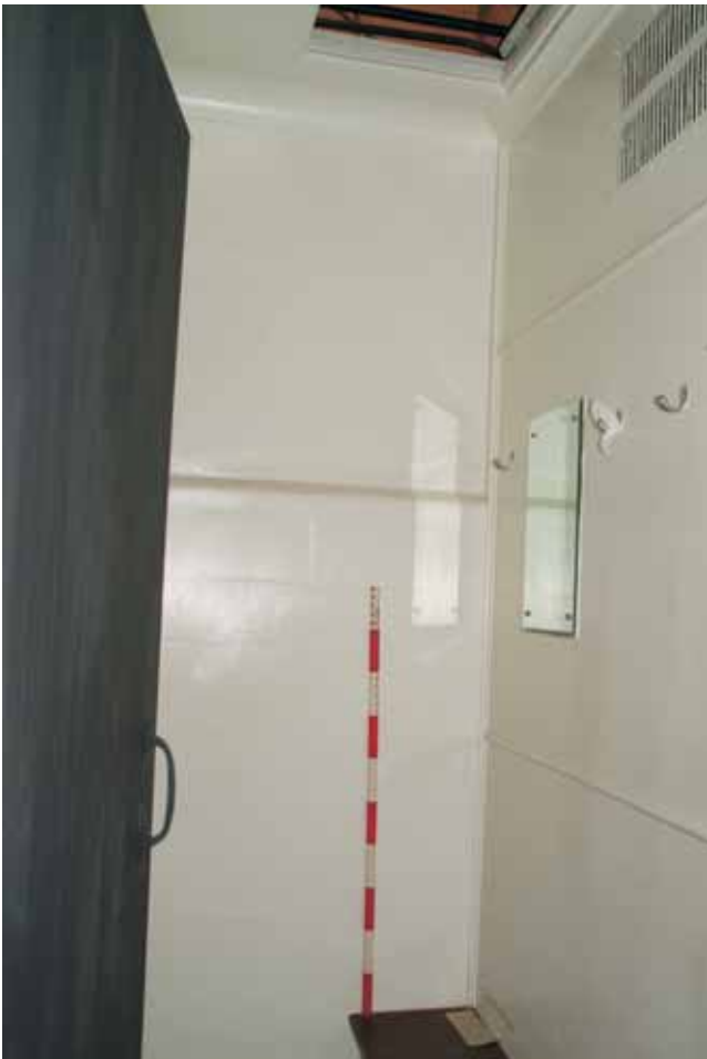
Plate 17.41: Building 17b – ground floor: coved cornice within changing room, view to the north
