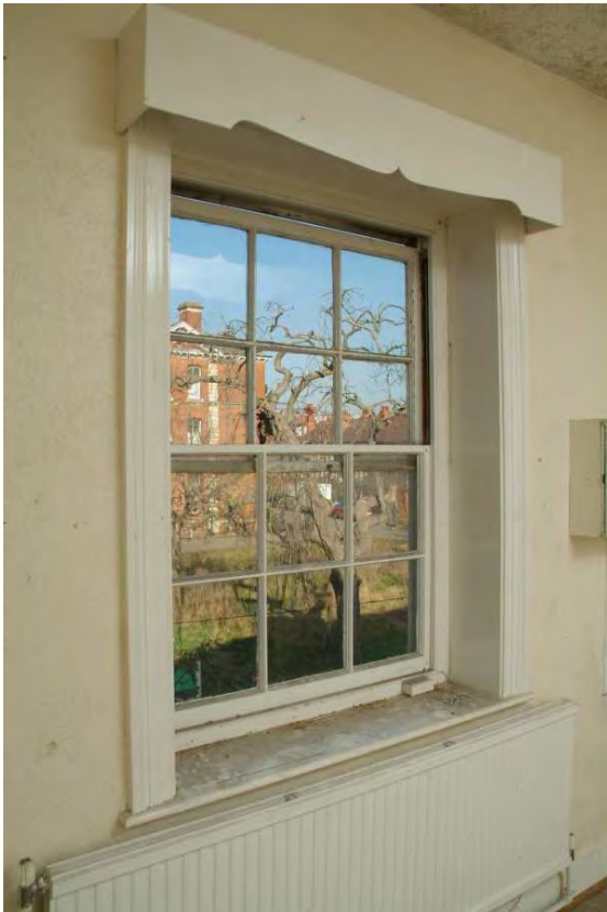
Plate 30.41: Building 30 (FF): northwest principal room showing detail of window and surround, view to the northeast
