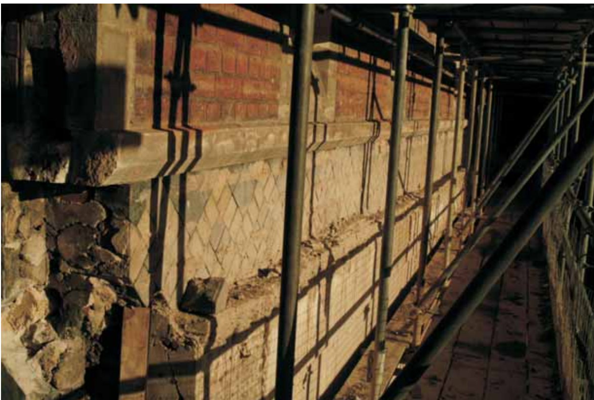
Plate 22.4: Building 22 – detail of southern elevation during removal of brick skin (corridor wall), view to the east
