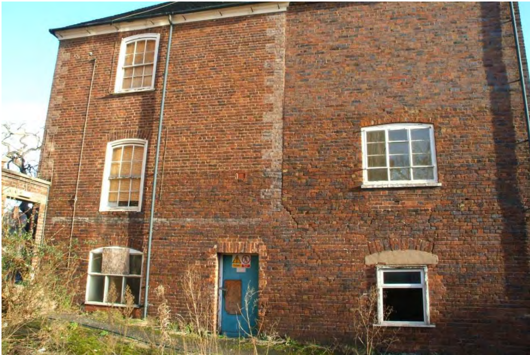
Plate 30.7: Building 30: detail of western elevation showing changes in brickwork, view to northwest
