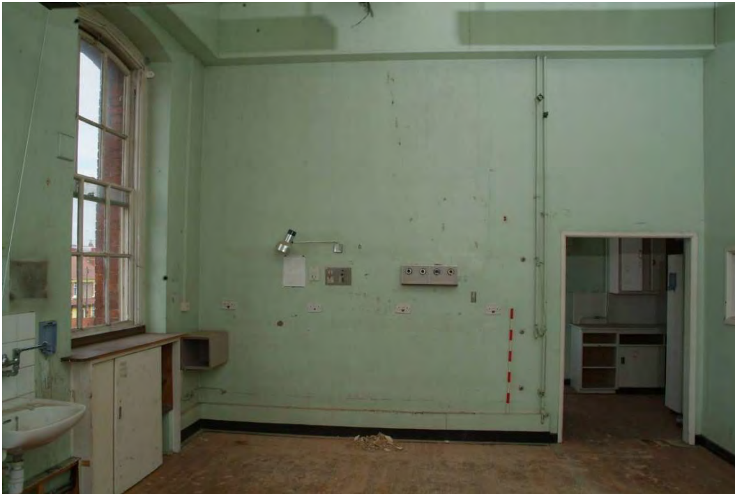
Plate 24.167 Building 24 (FF): east end of Garlick Ward showing inserted entrance to utility store room [Room 2.11], view to the south
