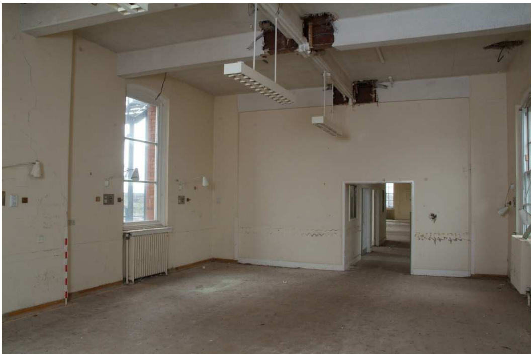
Plate 24.82: Building 24: Wheeley Lea Ward [Room 1.35], showing point of eastern extension, view to the southwest
