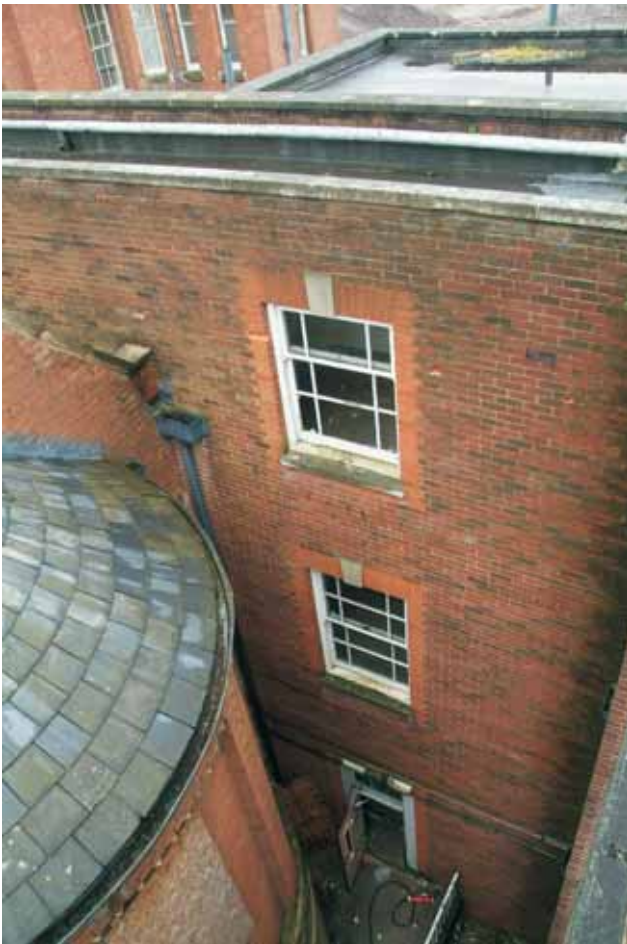
Plate 17.5: Building 17a – exposed north wall of E – W link corridor, view to the southeast
