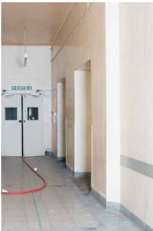
Plate 17.47: Building 17a – second floor: later openings on east side of link corridor accessing 1960s extension (note the change in floor level), view to the northeast
