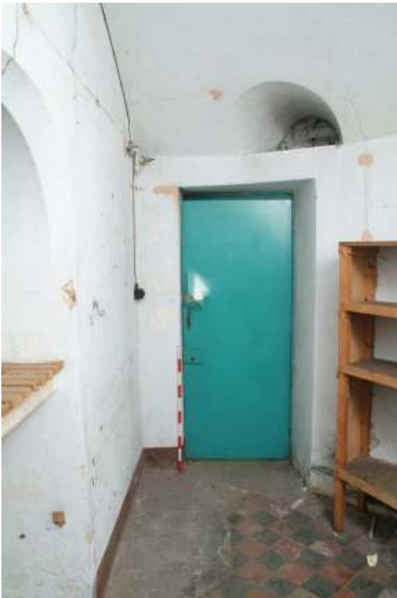
Plate 22.77: Building 22 (LGF): interior of apse showing inserted doorway, view to the south
