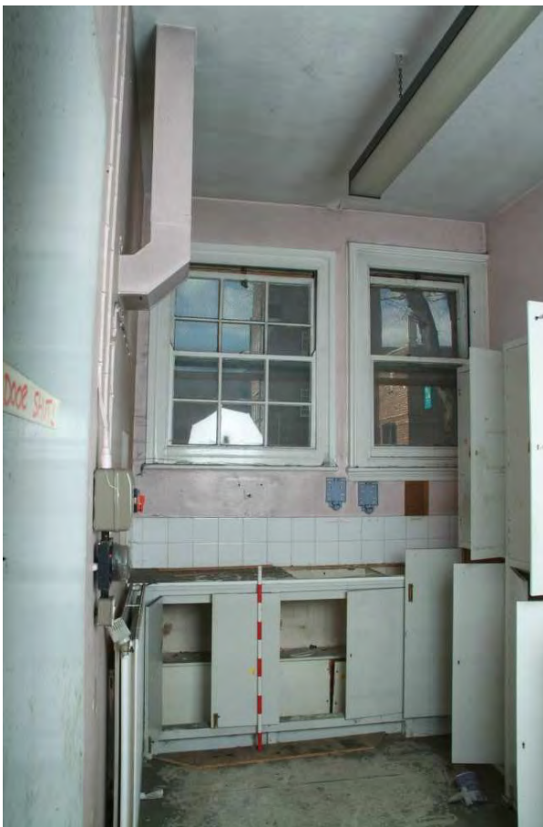
Plate 40.14: Building 40 (LGF): clean utility room [Room 0.39] showing two types of windows, view to the north
