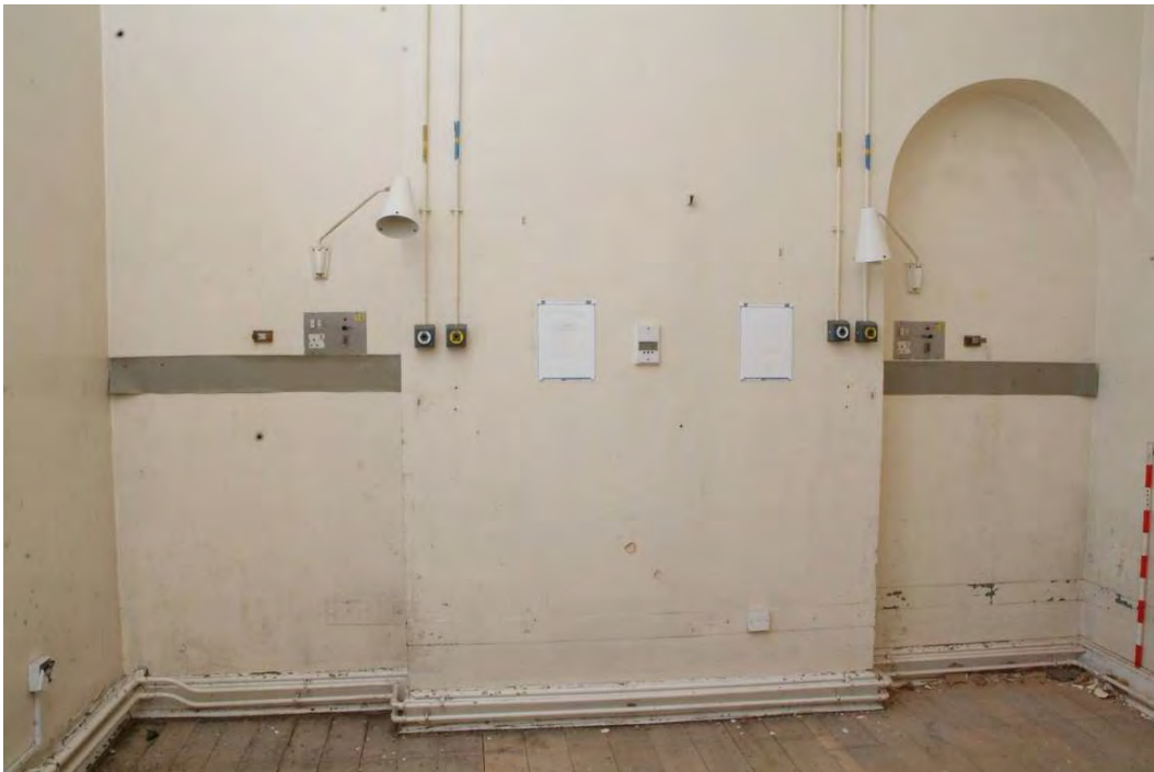
Plate 24.176: Building 24 (FF): interior of ward [Room 2.26] showing blocked fireplace, view to the south
