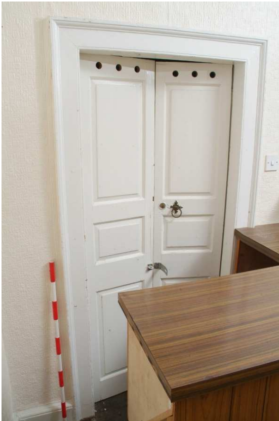
Plate 30.21: Building 30 (GF): northeast principal room showing original doors to wardrobe, view to the southwest
