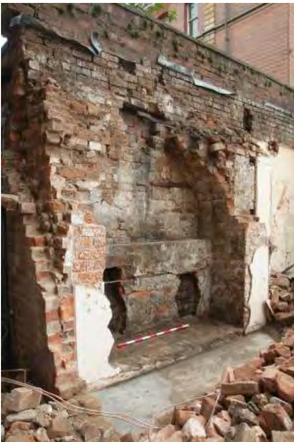
Plate 35.12: Building 35 – view of fireplace following demolition of the building, view to the east
