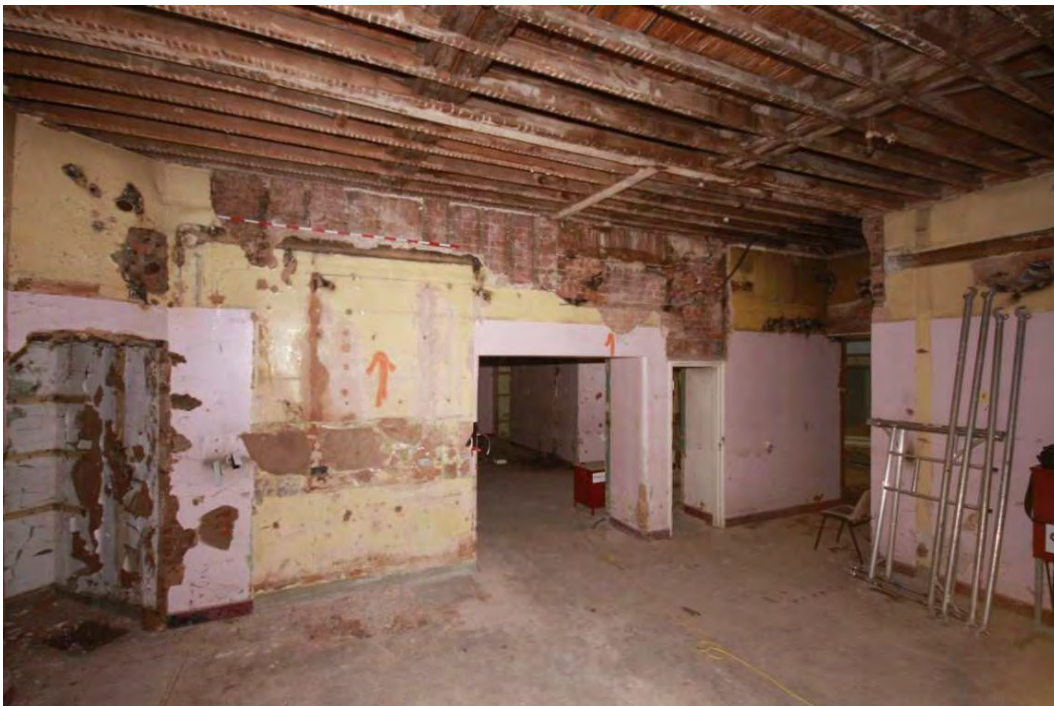
Plate 24.150: Building 24 (LGF): blocked openings in original western elevation of north wing (Building 24a) following soft strip, view to the southeast
