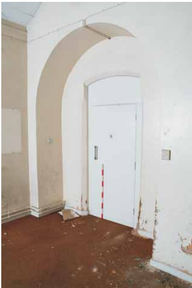
Plate 14.14: Building 14 – detail of original doorway in partition between west wing and central range, view to the northeast
