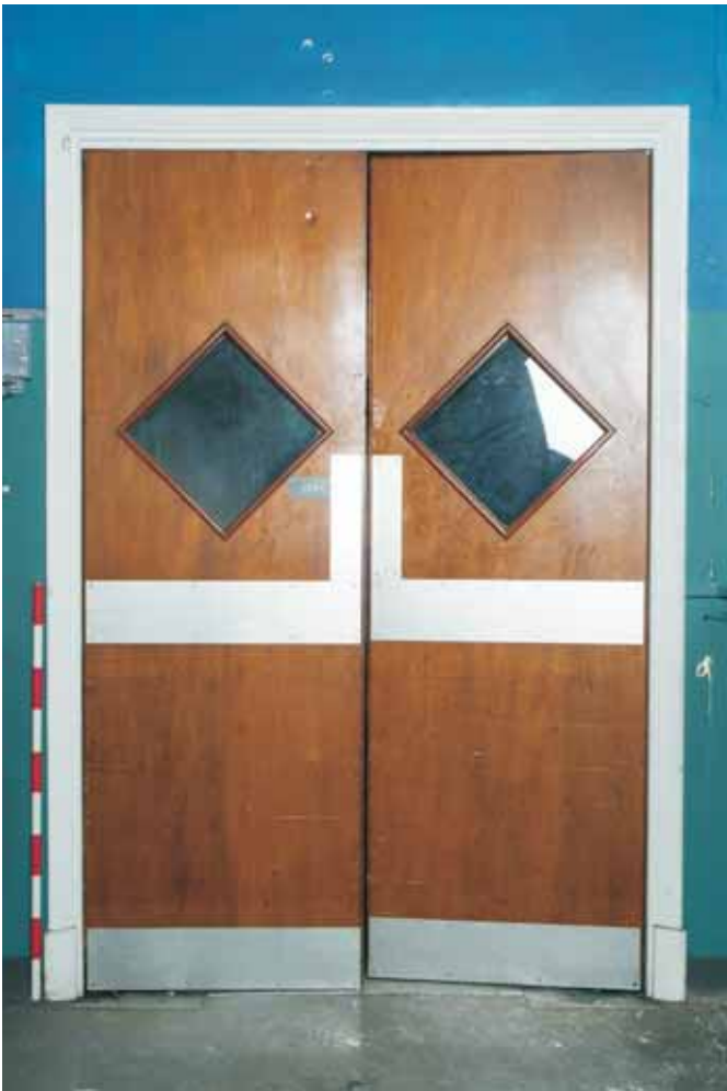
Plate 17.43: Building 17b – first floor: original doors between link corridor and main block, view to the south
