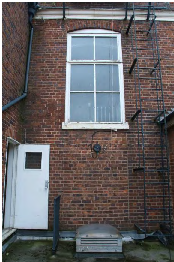
Plate 30.10: Building 30: detail of original southern elevation showing alterations to brickwork below stairlight, view to the north
