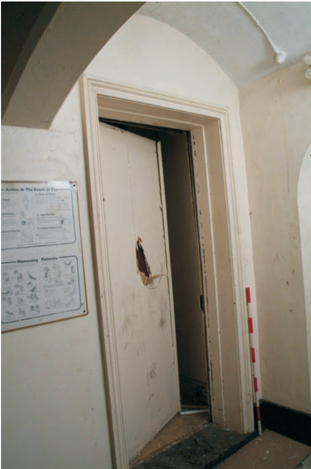
Plate 22.47: Building 22 – connecting range (LGF): door from the central corridor to the 'Contingency Store', view to the southwest
