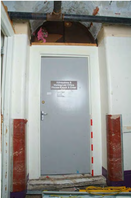
Plate 24.129: Building 24 (LGF): door to central eastern room [Room 102], view to the east
