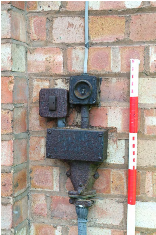
Plate 29.3: Building 29: detail of original switches
