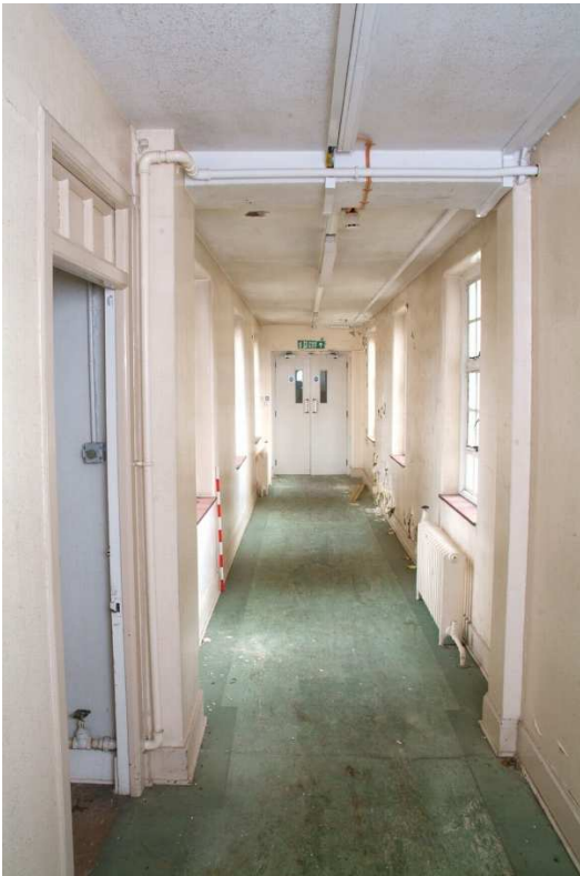
Plate 27.63: Building 27b – first floor: interior of elevated corridor looking from Building 27a, view to the south
