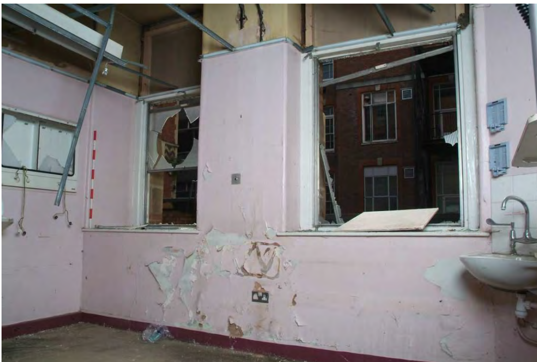
Plate 24.144: Building 24 (LGF): original openings in west elevation of Building 24b [Room 58], view to the southwest
