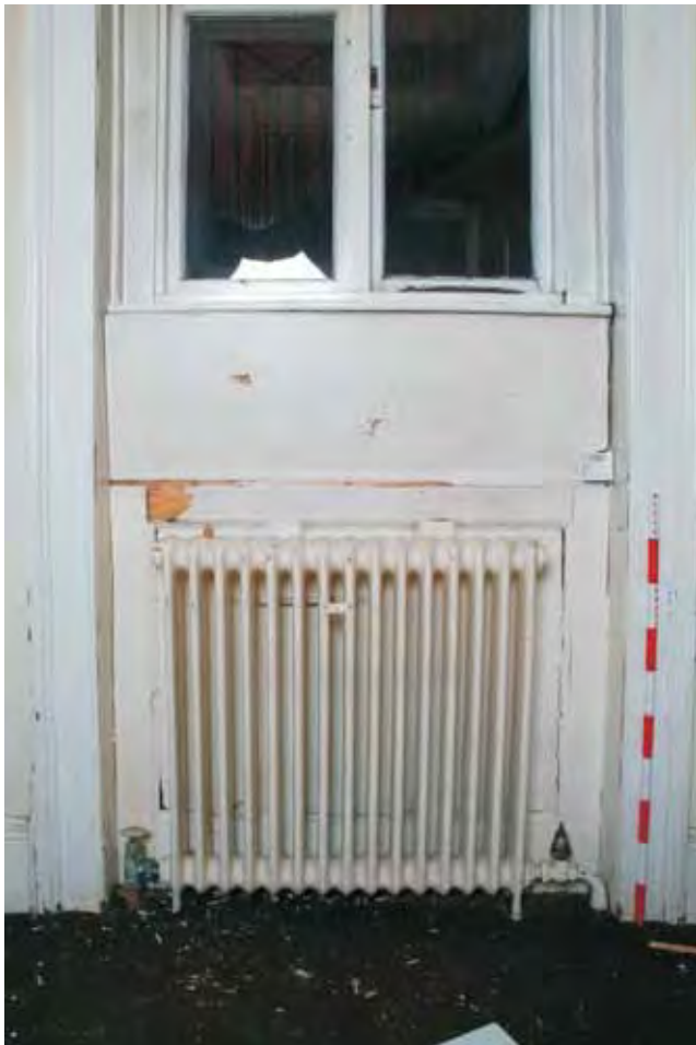
Plate 22.41 : Building 22 – connecting range: medical library on upper ground floor showing detail of original panelling behind radiator, view to the north
