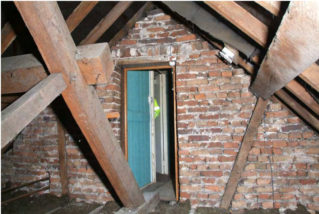
Plate 30.55: Building 30 (attic floor): interior of eastern roof space showing door to northern corridor, view to the west
