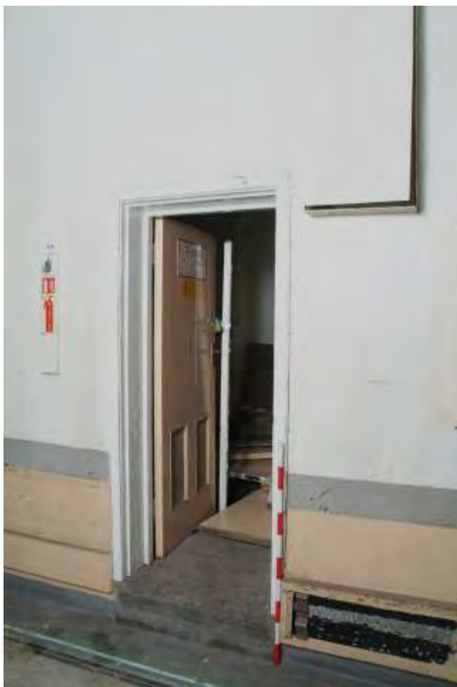
Plate 22.67: Building 22 (LGF): entrance to electricity switch room from the Building 17 link corridor, view to the northwest
