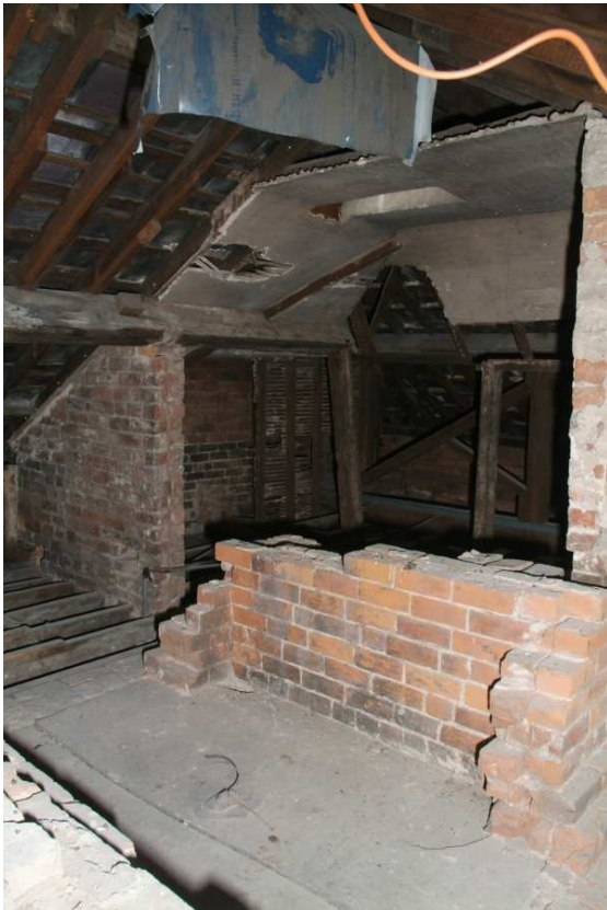
Plate 24.215: Building 24 (Roof Structure): former tank support structure in central part of roof, view to the southwest
