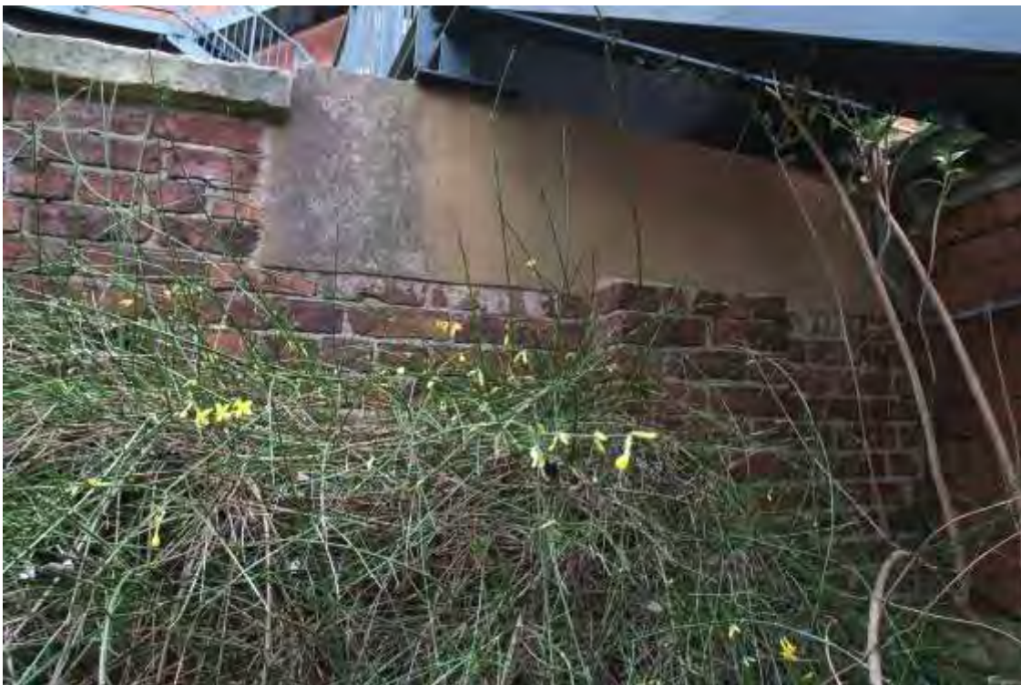
Plate 46.2: Building 46 –southern face to south of Building 36 showing concrete insert for fire escape, view to the northeast
