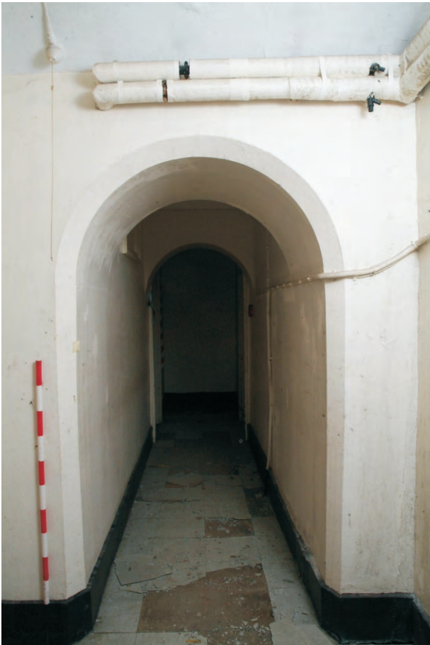
Plate22.45 : Building 22 – connecting range (LGF): opening to the central corridor beneath the nave, view to the west
