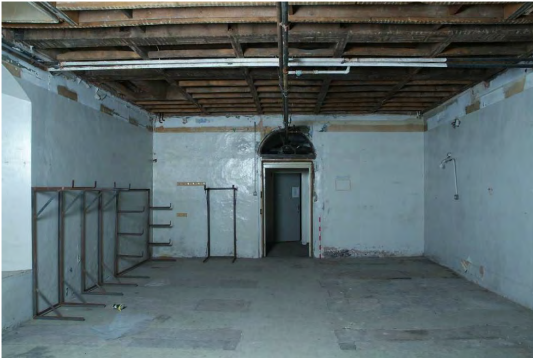
Plate 24.133: Building 24 (LGF): Records Store [Room 91] showing entrance from central corridor, view to the east
