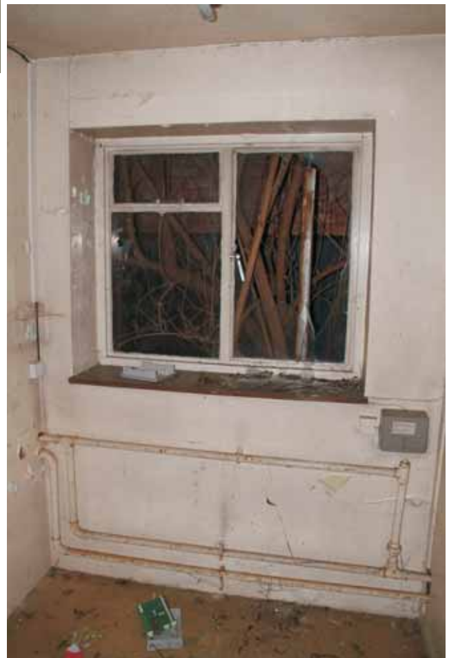
Plate 14.18: Building 14 – detail of metal framed casement in south elevation, view to the southeast
