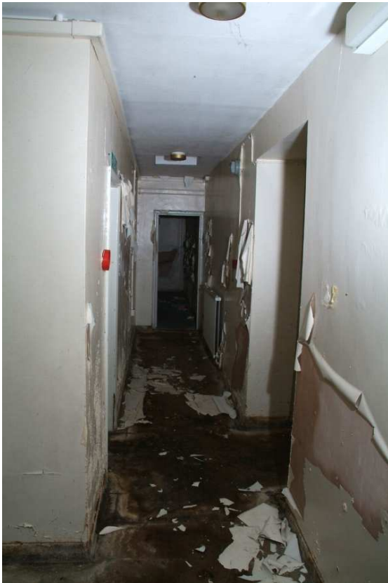
Plate 30.33: Building 30 (LGF): corridor along north of late 20th century extension showing inserted opening through rear wall of original house, view to the west
