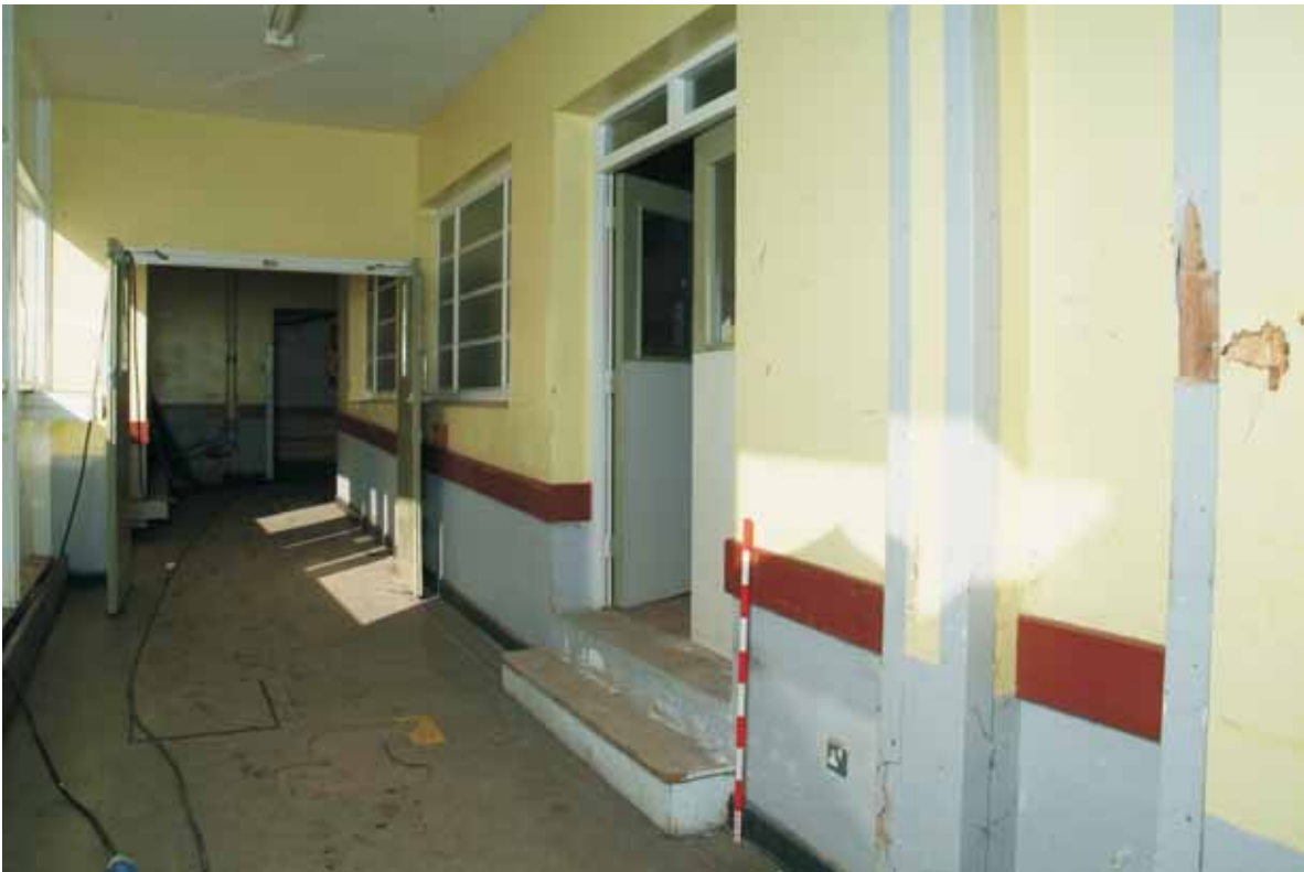
Plate 15.4: Building 15 – interior of north-south section showing doors to kitchens (B.24c), view to the northeast
