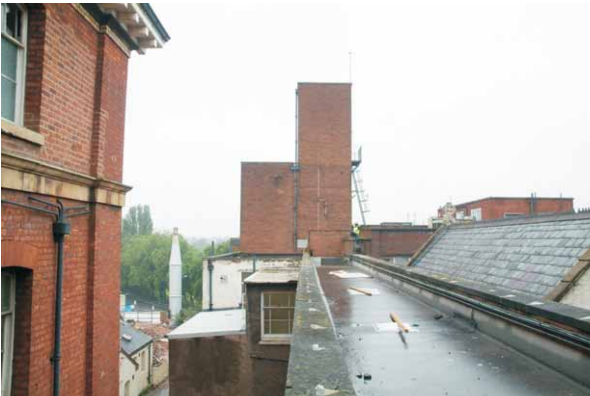
Plate 17.6: Building 17a – flat roof of E – W link corridor with stair/ lift tower in background, view to the west
