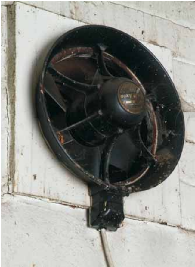
Plate 6.13: Building 6 – detail of 1950 'Vent-Axia' fan, former central workshop
