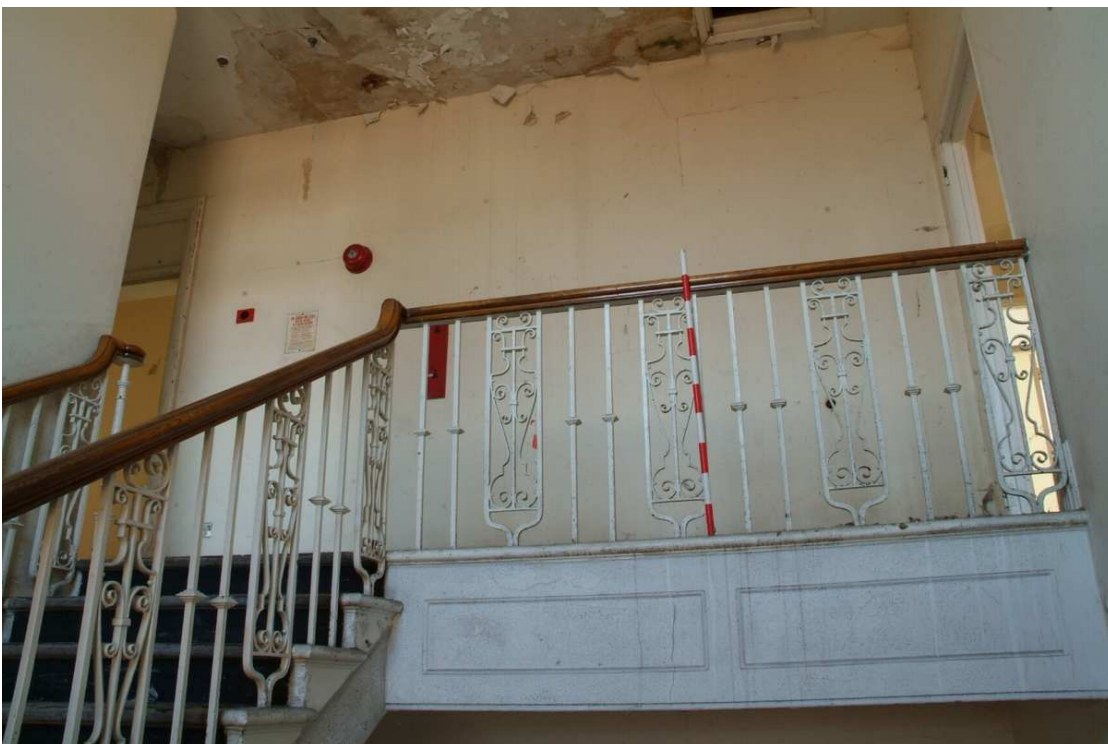
Plate 43.66: Building 43 - first floor: landing showing string and terminal balustrade, view to the west
