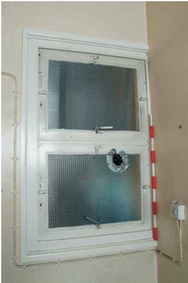
Plate 14.17: Building 14 – detail of metal framed pivoting window in north elevation, view to the north
