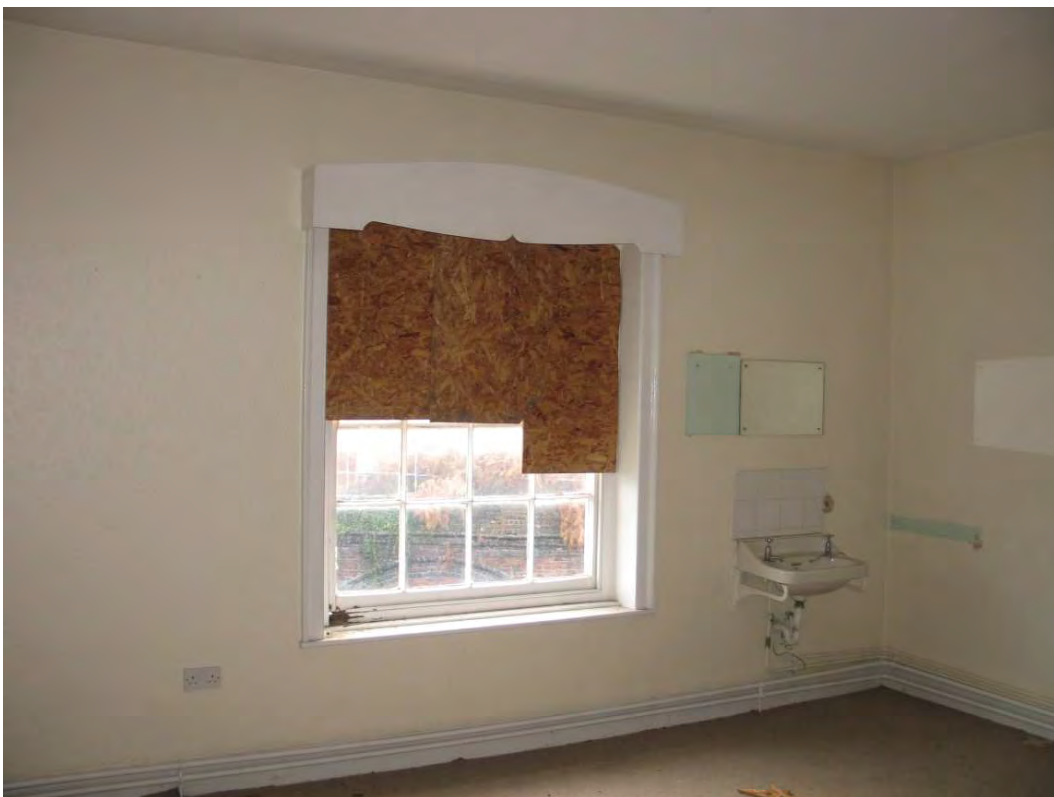
Plate 30.46: Building 30 (FF): bedroom in late 19th century extension to southwest wing, view to the southwest
