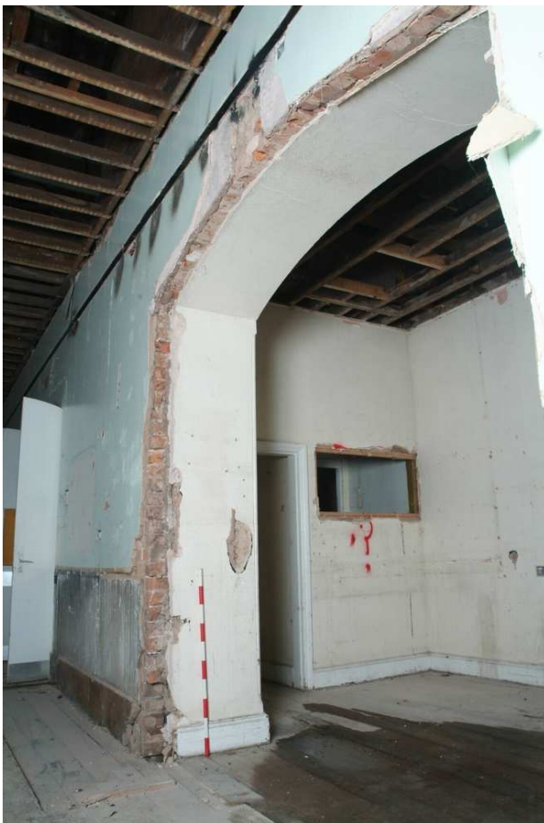
Plate 24.208: Building 24 (SF): inserted opening in the north wall of the Bonaker Ward, view to the northwest
