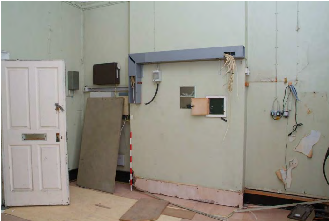
Plate 24.56: Building 24: comms room [Room 1.19], view to the northwest
