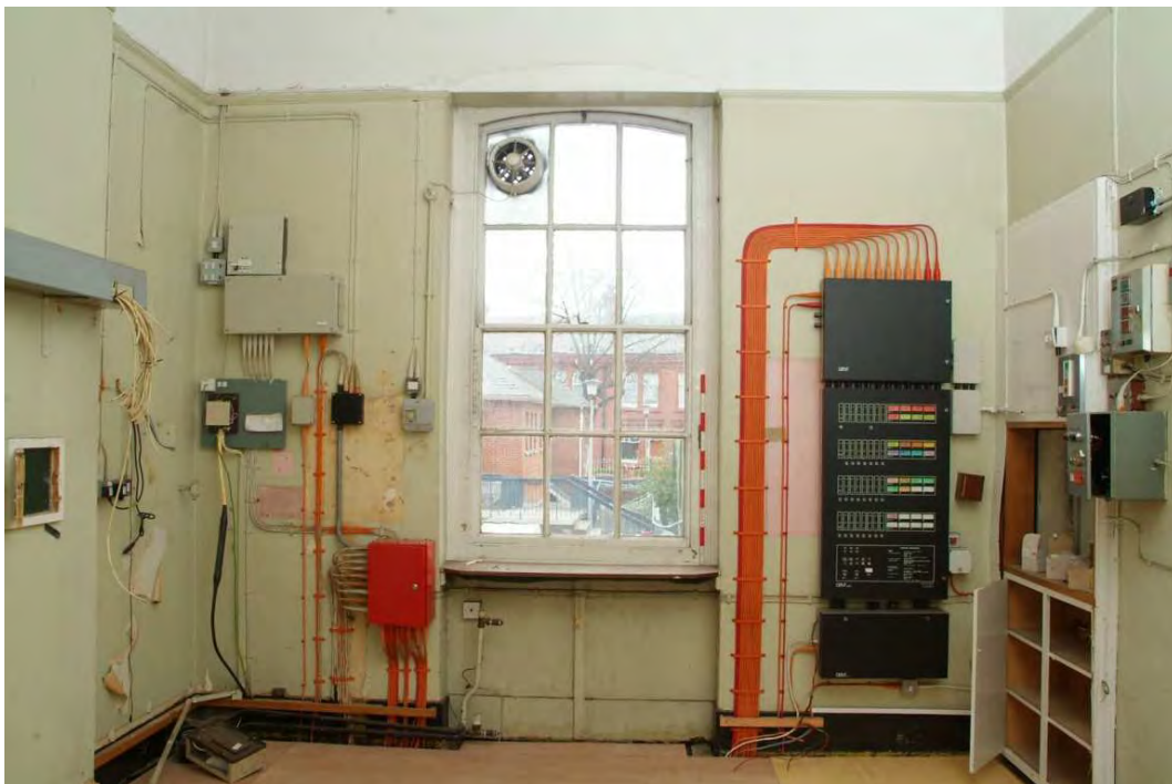
Plate 24.54: Building 24:comms room [Room 1.19], view to the southeast
