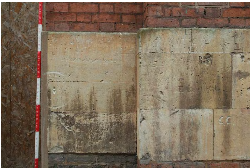
Plate 24.33: Building 24: southern elevation showing detail of graffiti on lower ground floor of original building (Building 24a)
