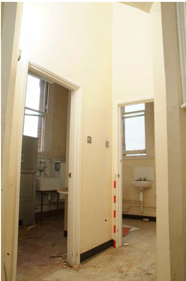
Plate 24.214: Building 24 (SF): interior of southwest corner tower showing lavatory partitions, view to the southwest
