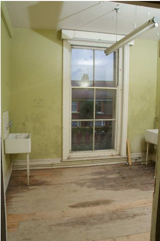
Plate 43.53: Building 43 - first floor: laundry room to the south of the stairwell, view to the southeast
