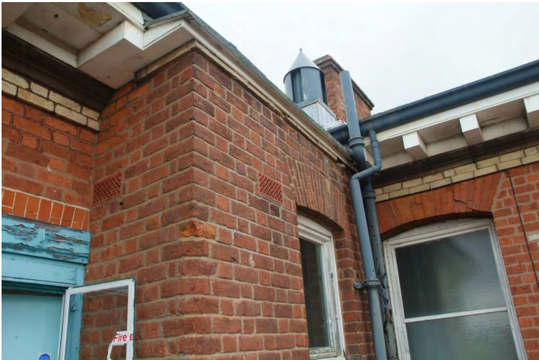
Plate 24.200: Building 24 (SF): cowl on roof above the closet wing, view to the northeast
