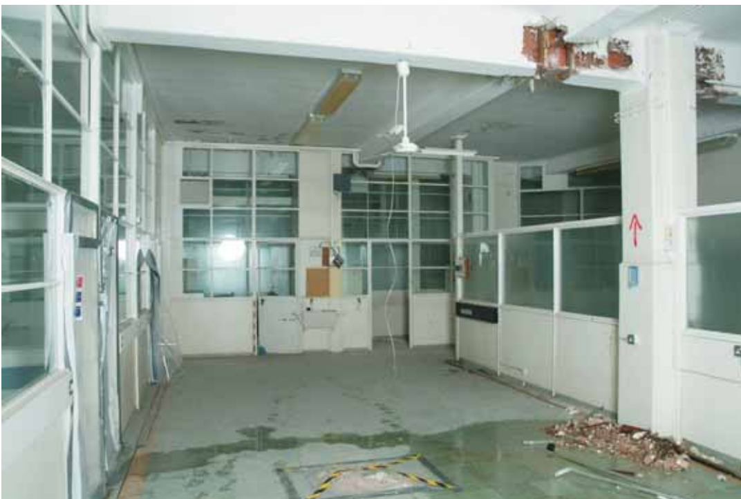
Plate 17.44: Building 17b – second floor: original metal partitions within the children's ward, view to the north
