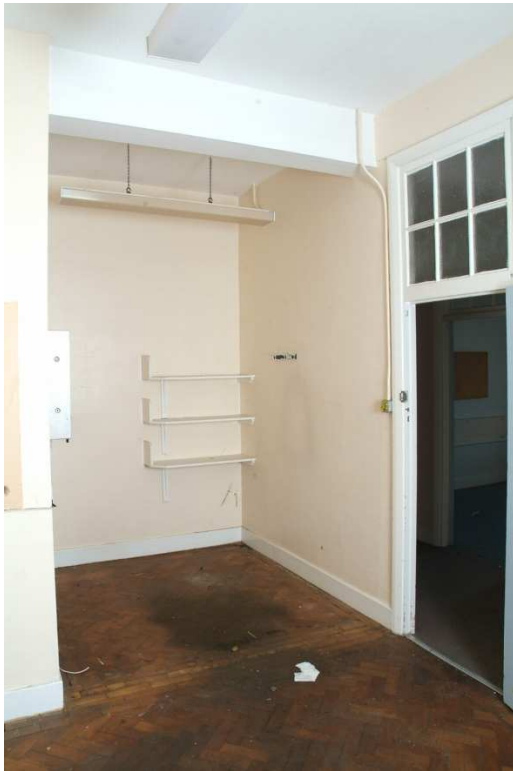
Plate 27.57: Building 27b – ground floor: converted bedroom and store room, view to the south
