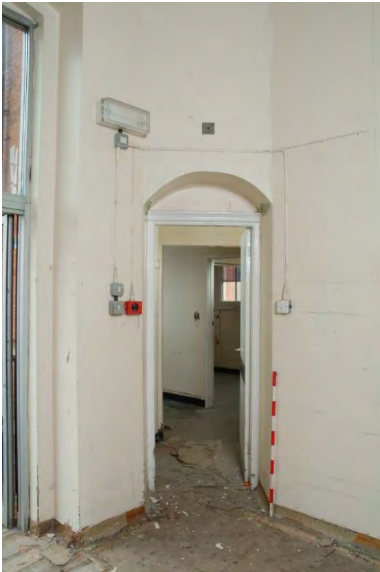
Plate 24.87: Building 24: Wheeley Lea Ward [Room 1.35] showing entrance to corner tower, view to the southeast
