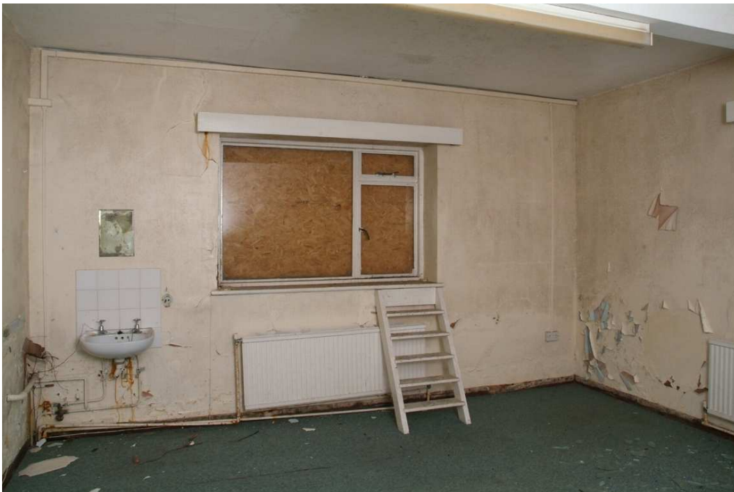
Plate 30.34: Building 30 (LGF): refurbished interior of early 19th century southwest extension, view to the southwest
