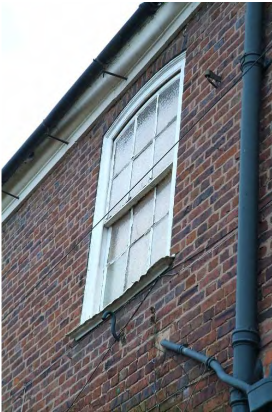
Plate 30.5: Building 30: detail of 1820s first floor window showing eaves cornice, view up and to the southeast
