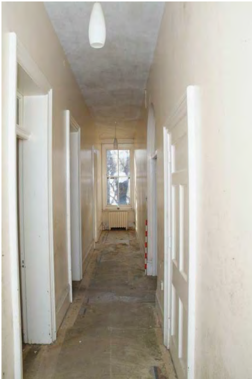
Plate 43.35: Building 43 - ground floor: corridor along north side of southern range, view to the south
