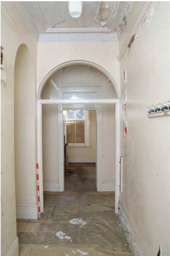
Plate 43.33: Building 43 – ground floor: entrance to southern wing showing wide opening to store room, view to the south
