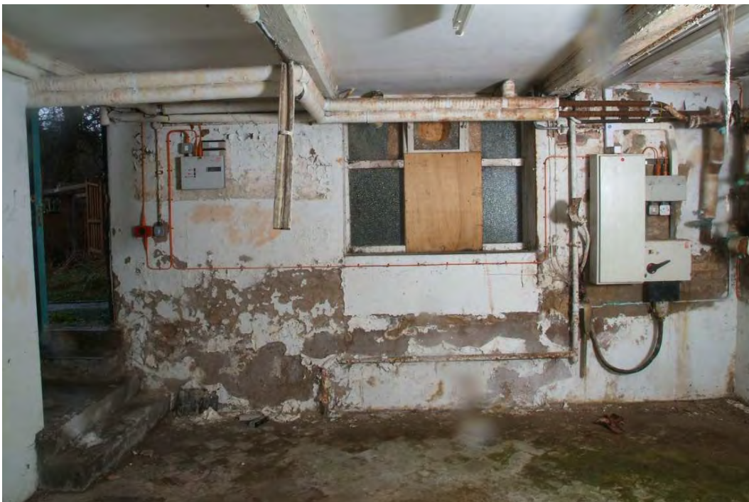
Plate 30.28: Building 30 (LGF): westernmost part of original basement showing part blocked window opening, view to the west
