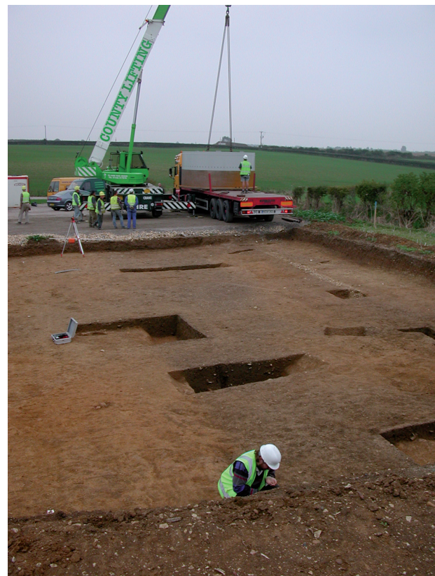
Fig 1 Excavation of trench T7, with unloading of wind turbine base in background
