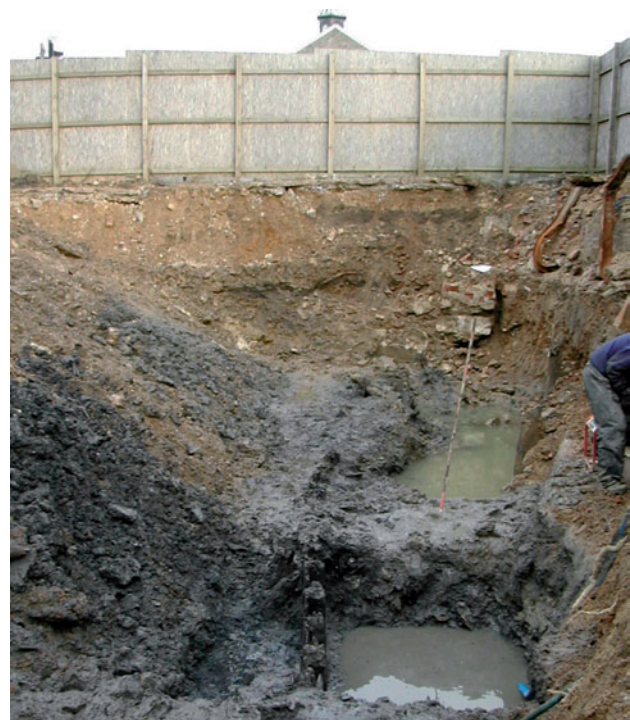
Fig 7 Trench extension, looking east, showing the exposed tops of the posts and the deeper intervention (foreground)
