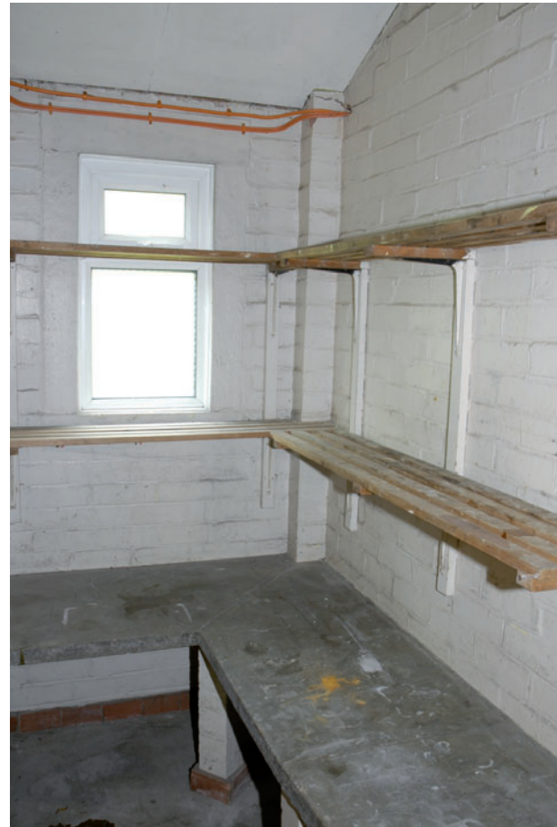
Fig 11 Store room, with stone slab shelf on brick piers, and wooden-slatted shelving
