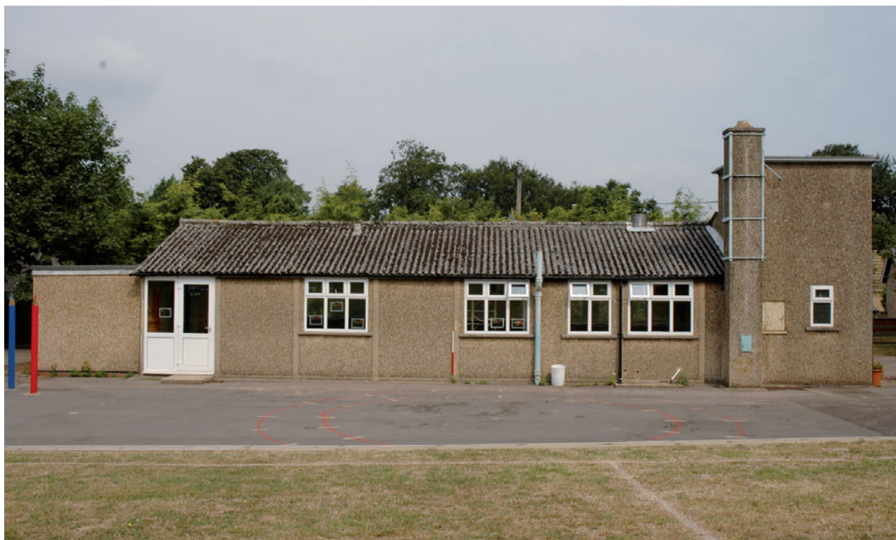
Fig 5 The southern elevation, with the service rooms (right) and the modern extension (left)
