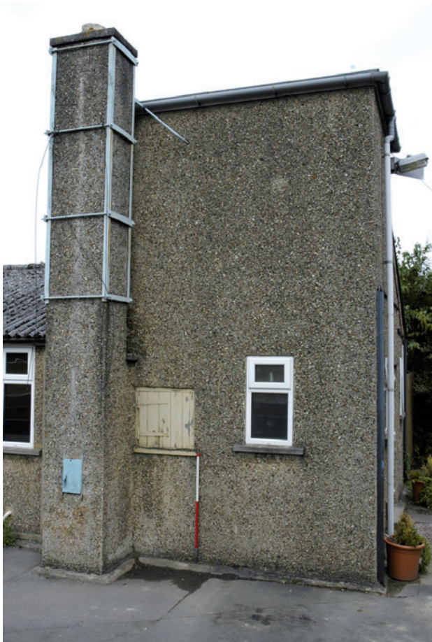
Fig 10 The service rooms, showing the chimney, with supporting metal bands, and hatch opening into the possible coal store
