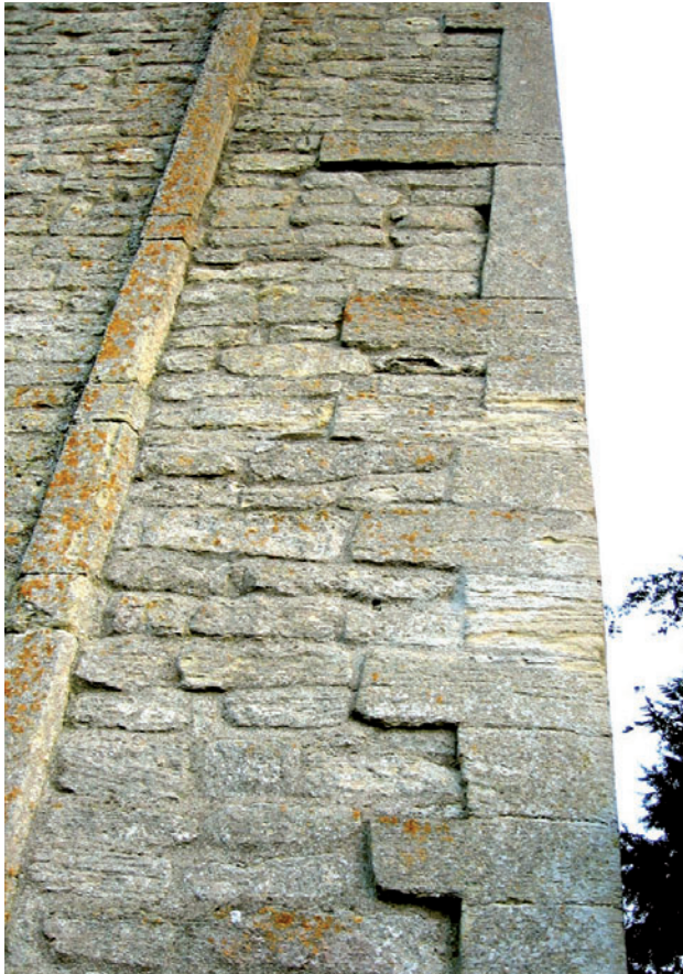
Fig 4 The north-west tower quoin of St John the Baptist, Barnack clearly displays the change in the Barnack Stone bedding orientation in its first stage (The lowest stones (below stone 19, stone 20 BVFL) bedded BH are later replacements)
