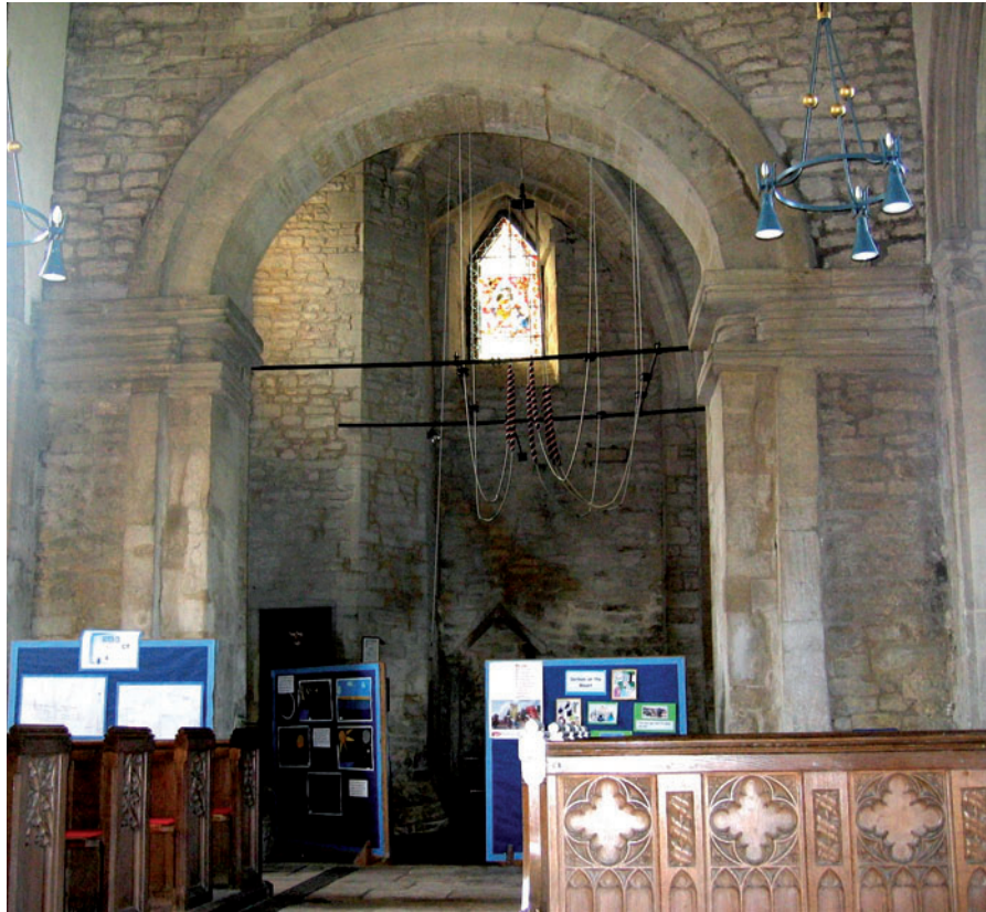
Fig 7 The tower arch of Barnack church is built in Anglo-Saxon style and the lowest readable jamb stones are orientated in the fashion of the period (BVFIA and BH)
