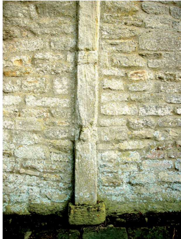
Fig 5 In the north face of the tower at Barnack church the north-east pilaster displays the frequency with which the long stones, in particular, are orientated BVEB
