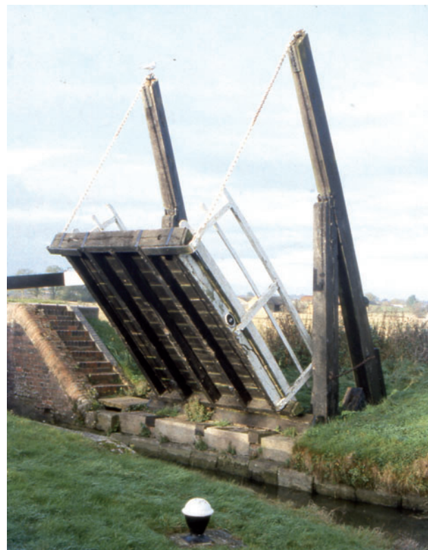
Fig 4 Rothersthorpe Lift Bridge GN5 in the up position, prior to dismantling, looking south-west
