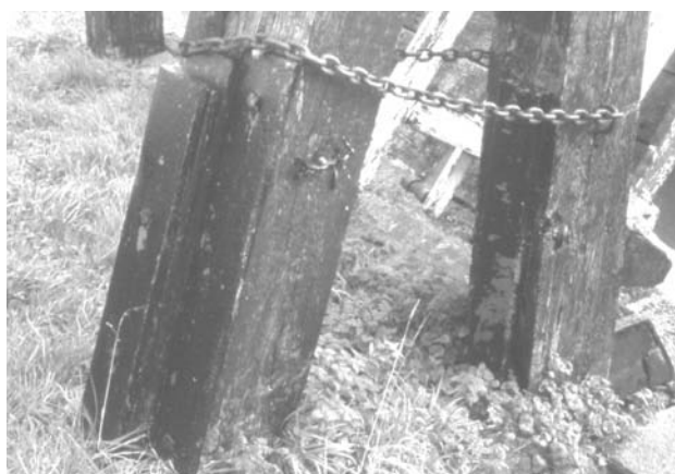
Fig 11 Detail of the iron plates at the base of the counterbalancing beam and upright post
