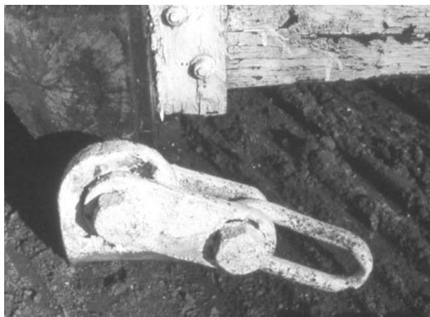
Fig 10 Detail of the replacement chain block fitting from the top of the counterbalancing beam
