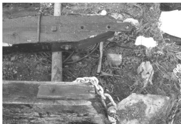
Fig 13 Detail of the original iron straps reused on the upright post and one of the bolt attachments, top, and detail of the 1960s refurbished chain assembly on the top of the counterbalancing beam, below
