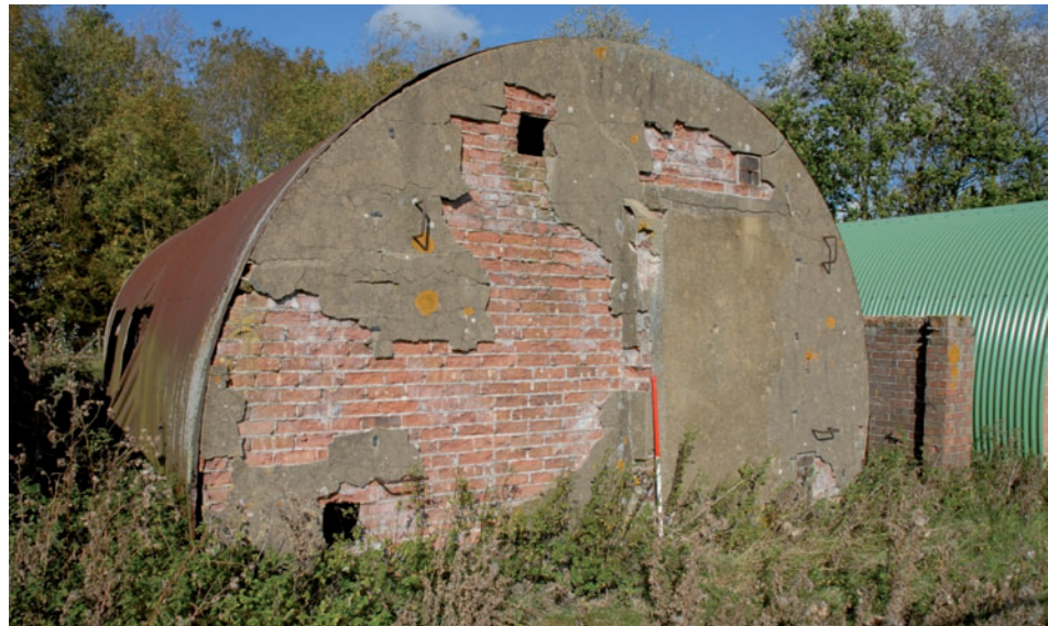
Fig 11 Back wall of Hut 141 showing concrete render over the blocked door, the vents and four iron rungs, looking north
