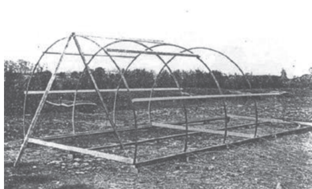
Fig 3 Steel ribs are bolted to the bearers and wooden purlins are fixed to the ribs with hook-bolts
