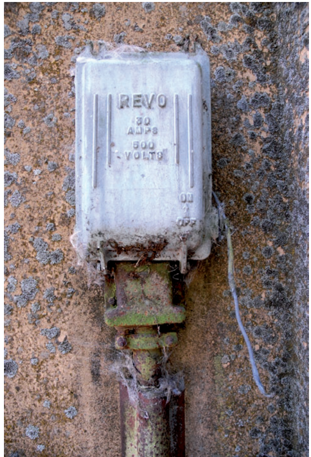
Fig 18 Electric junction box on Hut 141
