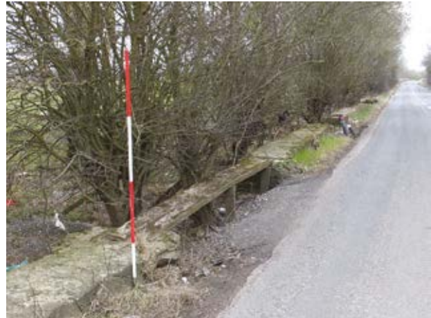
Fig 3 Great Doddington, view south-east along a concrete cylinder-constructed part of the causeway, together with remains of one of the timber boardwalks (Scale 2m)
