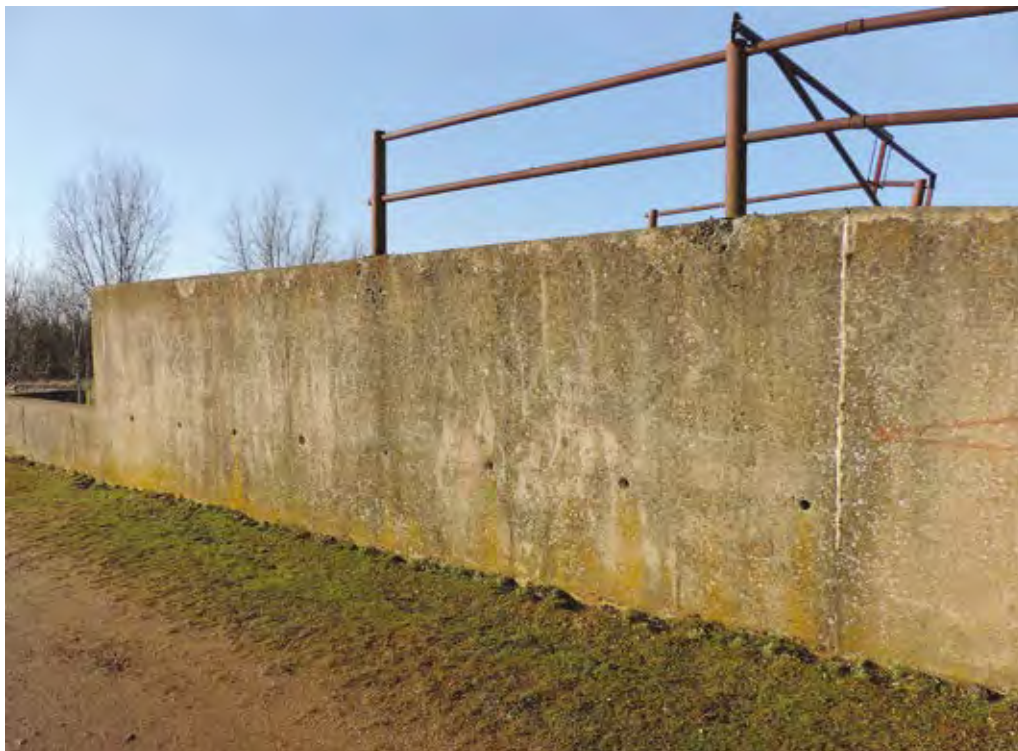
Fig 2 The south wall elevation before the new sand martin holes were installed
