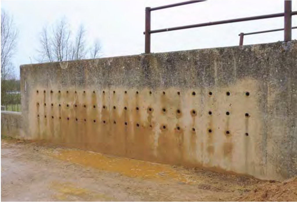
Fig 3 The south elevation wall after the new sand martin holes were installed
