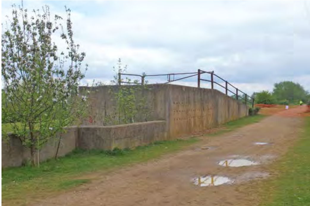
Fig 1 View of the west and south elevations with the three lines of sand martin holes just evident in the latter. The fenced-in ramp beyond and the drop to what would have been the conveyor to the fore, are also evident as is part of the conveyor screen wall extending westward
