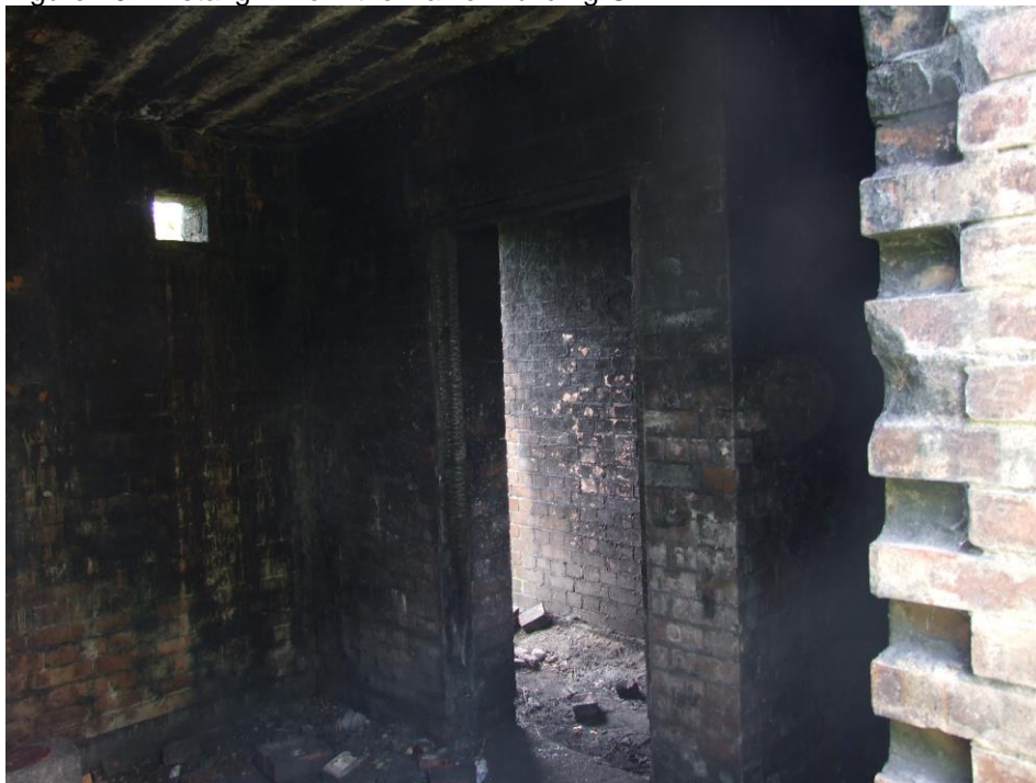
Figure 20 - The interior of Building G (with hole in the wall for the metal grill).
