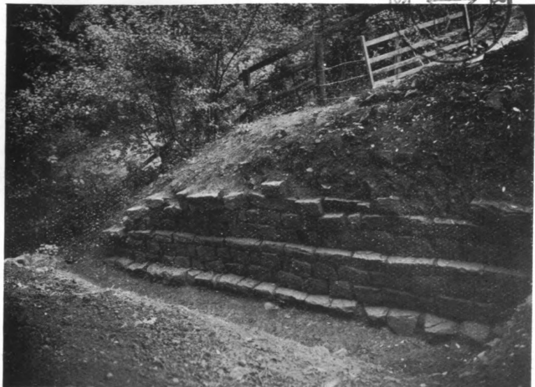
FIG. 1—NORTH FACE OF THE WALL WITH OFFSET THREE COURSES ABOVE FOOTING FLAGS, EAST OF MILECASTLE NO. 48.
