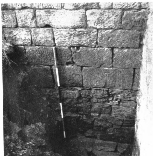
2. The town wall above Close Gate The lower part of the inner face
