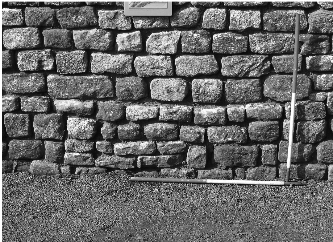
Fig. 21 Discontinuity on the inner face of the west wall of tepidarium E1, viewed from the east, indicating position of blocked flue from auxiliary furnace Q. Photograph, the authors.
