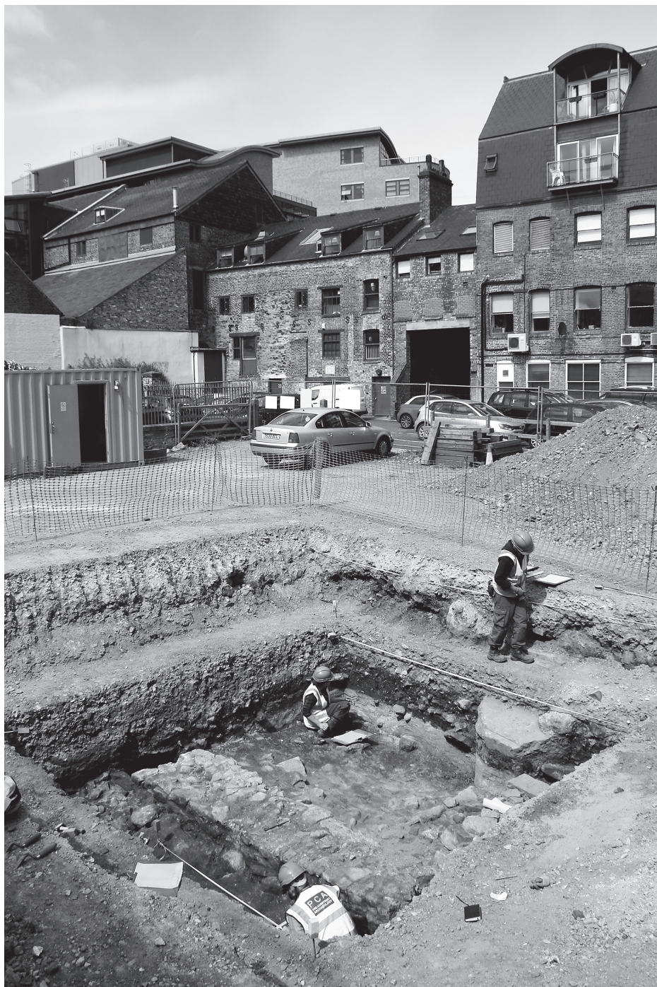
Fig. 3 Trench 1, prior to shoring installation, alleyway access from Broad Chare in centre rearground; looking north-east.
