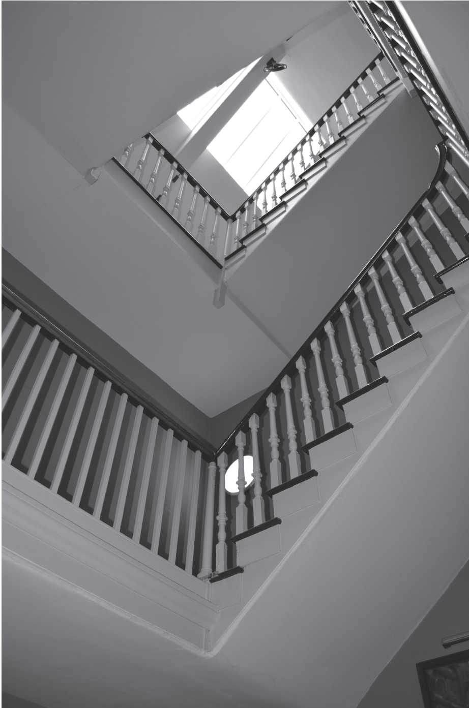
Fig. 9 The alterations to the staircase shown by the change in balustrade. Note the block and tackle on the roof rafter, to hoist items to the attics. (Richard Pears).
