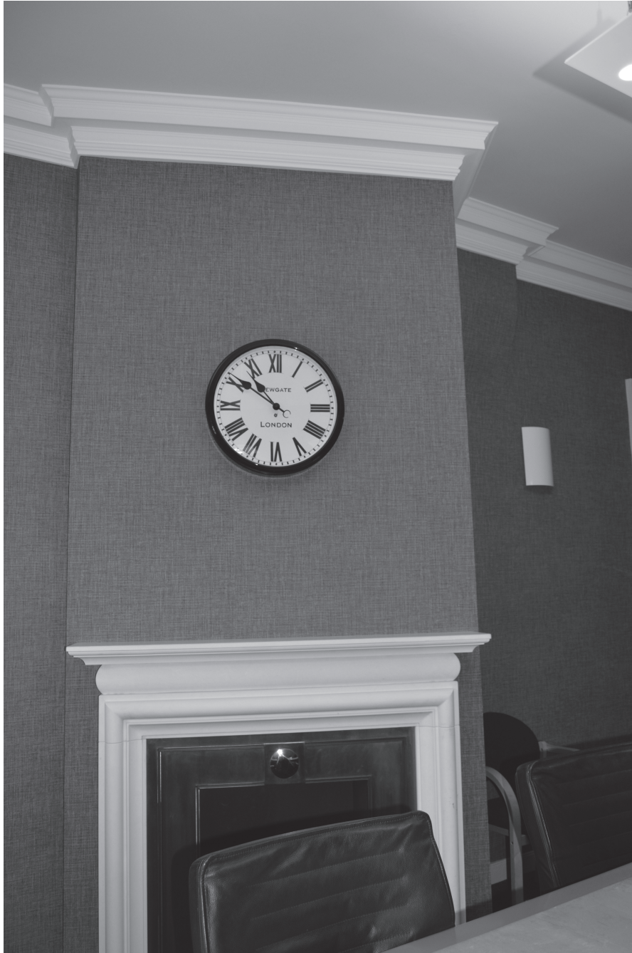
Fig. 8 Custom House: ground floor, south-west room. Inserted fireplace formerly in the corner of the room created by enclosing the ground floor loggia. Original wall of offices later removed leaving fireplace at angle to the larger room; note the protruding stub of wall at cornice level to right of the fireplace.
