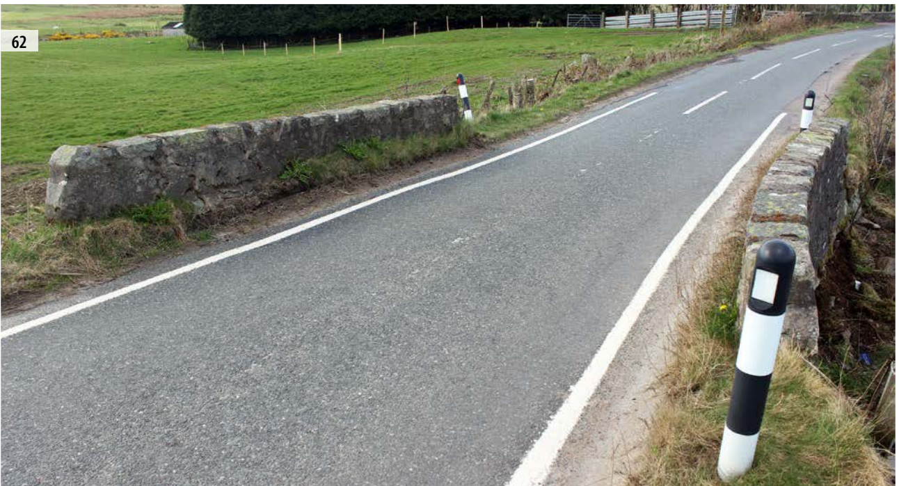
PLATE 59 A view of the bridge in its setting facing S PLATE 60 View of the north facing elevation of the bridge facing SW PLATE 61 View of the south elevation of the bridge PLATE 62 View of the upper side walls of the bridge facing W
