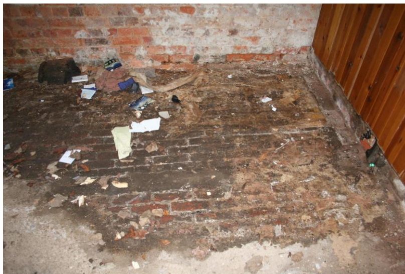
Plate 20: G7, surviving brick flooring in north-east corner
