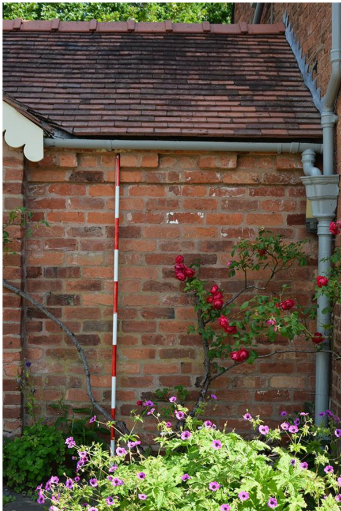
Plate 15: South elevation of bedroom extension of washhouse can be traced in the fabric building.
