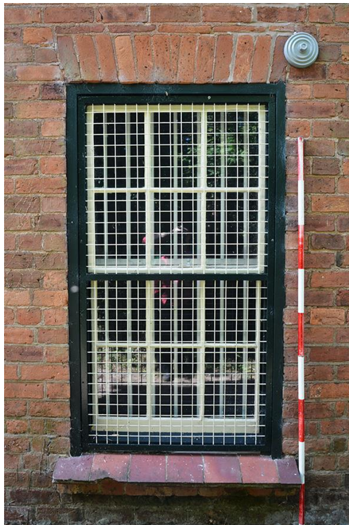
Plate 7: Window on north elevation, original structure of late 18 th century or early 19 th century
