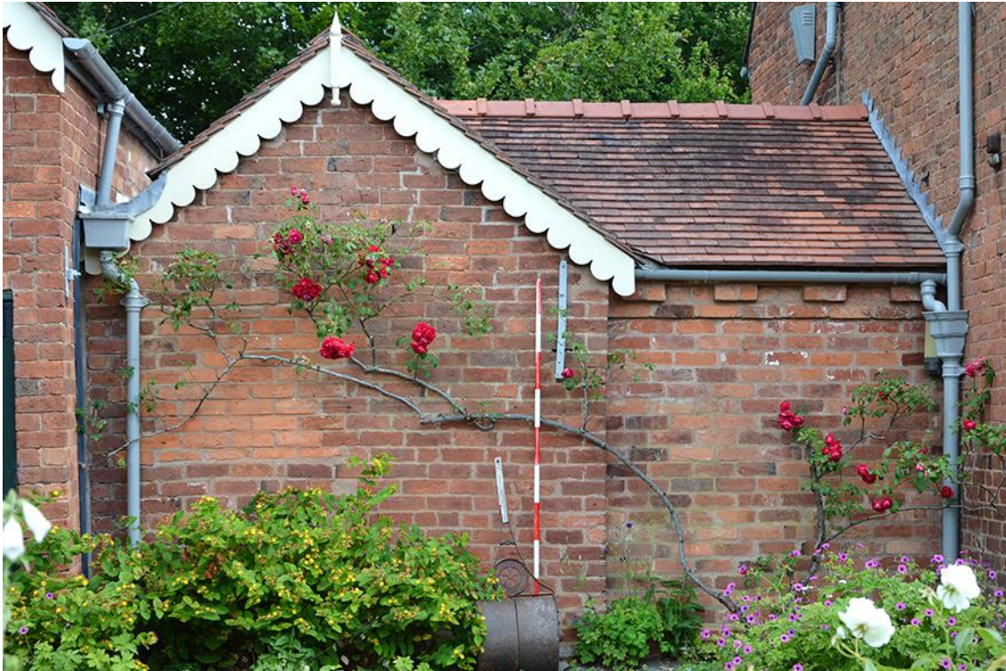
Plate 12: Washhouse west of cottage built c1830, note blocked window (left part only)
