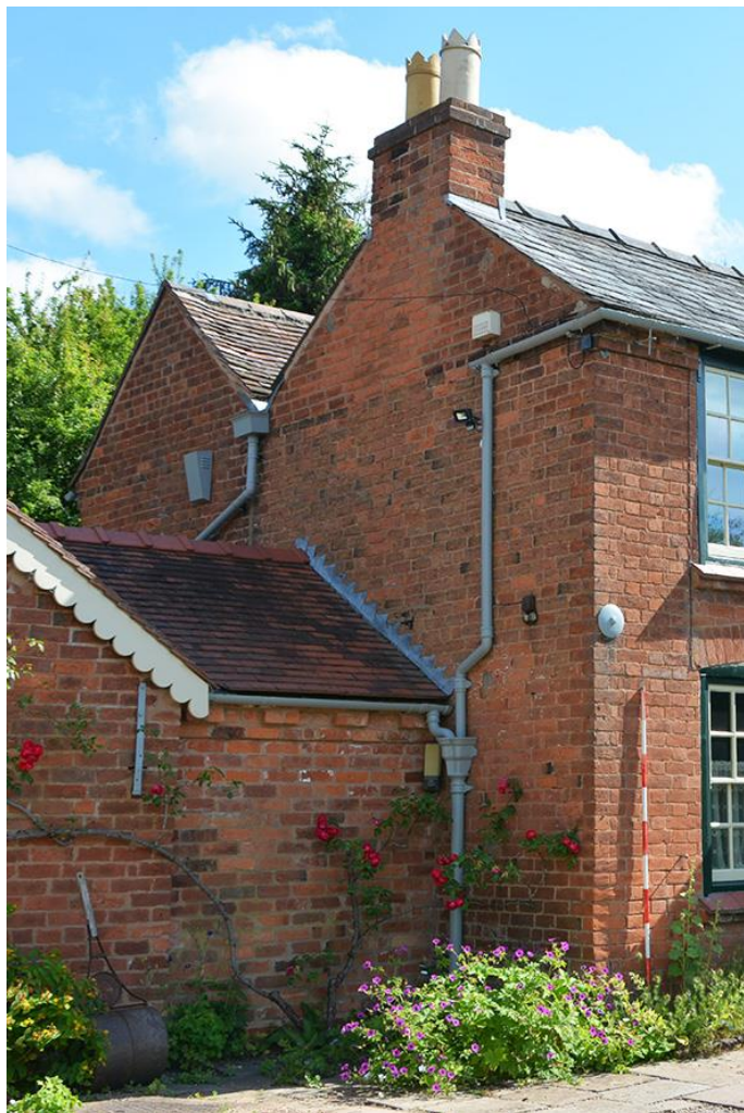
Plate 6: West elevation of the cottage from the south west, showing join between original structure (rear) and later (front)
