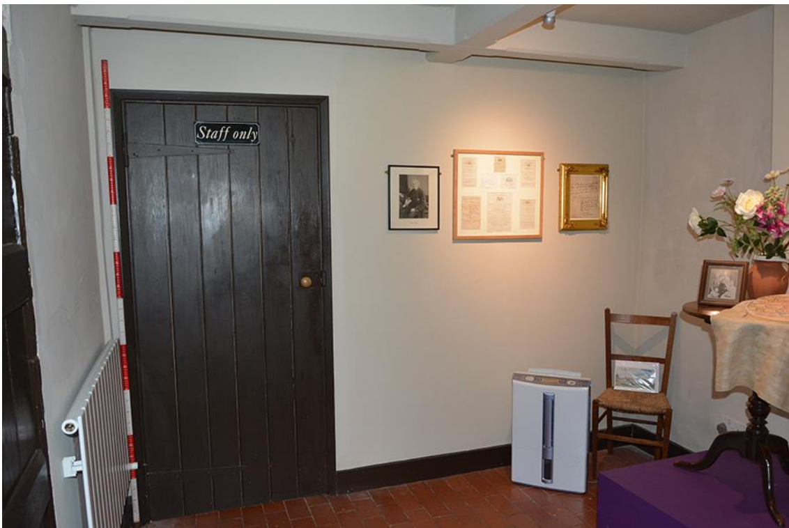
Plate 17: Division added in the scullery, note how ceiling beams continue into wall
