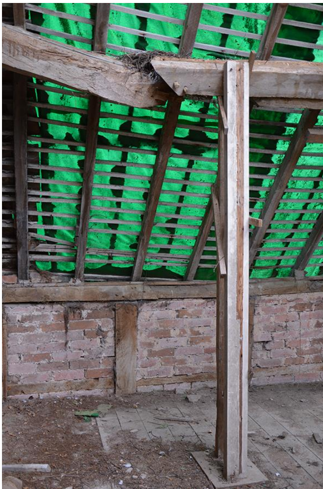
Plate 18 Eastern section, first floor interior showing broken purlin joint
