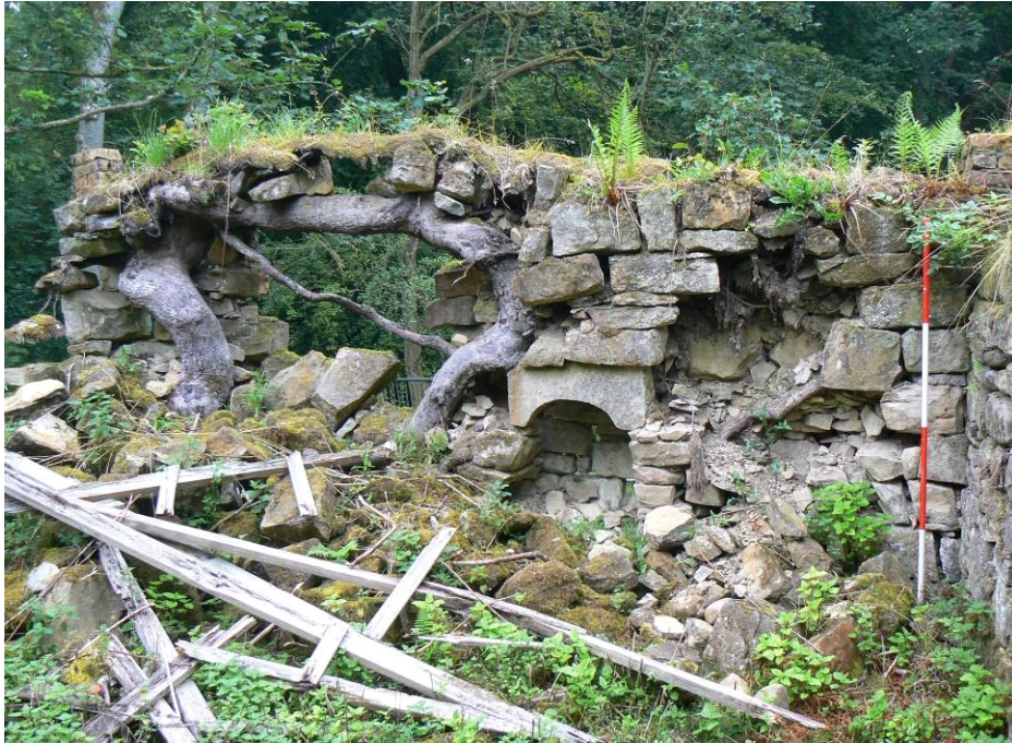
Plate 17: The extensively tumbled (and holed) inner face of the north wall of Building 2 with arched niche [2.2] surviving
