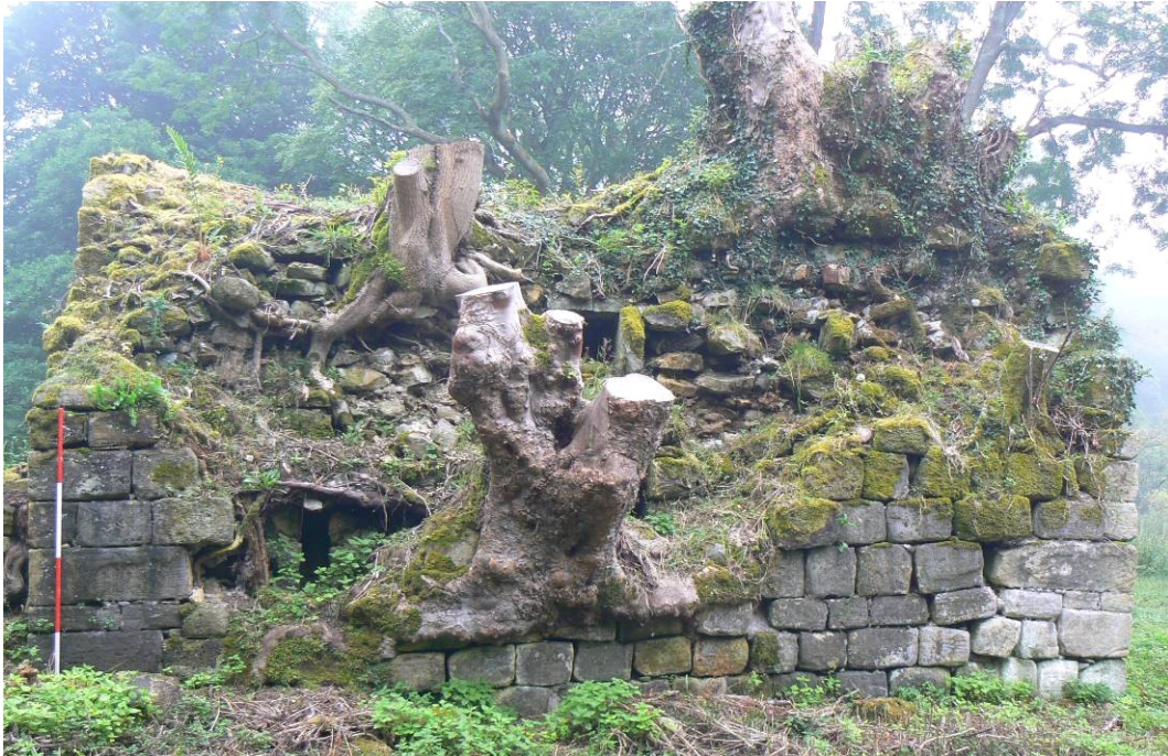
Plate 9: The west face of Overgrass Tower. A large scooped area has gone from the centre exposing the core. The garderobe chute [1.7] can be seen low down, towards the northern block of facing stones and light [1.6] immediately to the right of the central stump.
