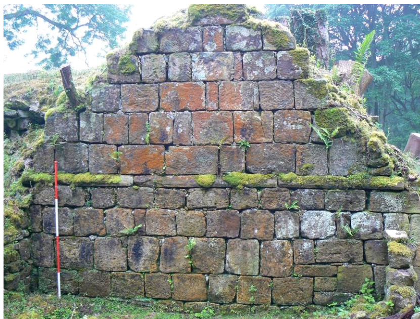
Plate 3: The western part of the north face of Overgrass Tower. To the east of this all facing stones have been robbed away. Red colouration on the stones is lichen. Scale used throughout is 2m long.
