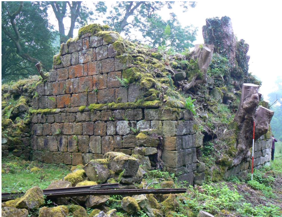
Plate 10: The north-west angle of Overgrass Tower. The remnants of the west wall of building 2 in the foreground.
