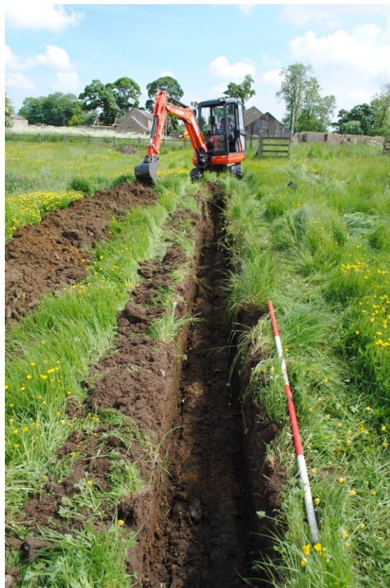
Plate 2: Excavating the outfall drain trench for the sewage treatment plant. Looking east.
