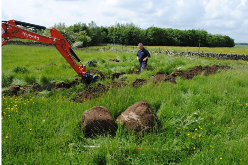
Plate 1: Excavation of the outfall drain trench for the sewage treatment plant beyond the western end of the farm ranges. Looking south-west. The boulders on the grass were removed from the trench.
