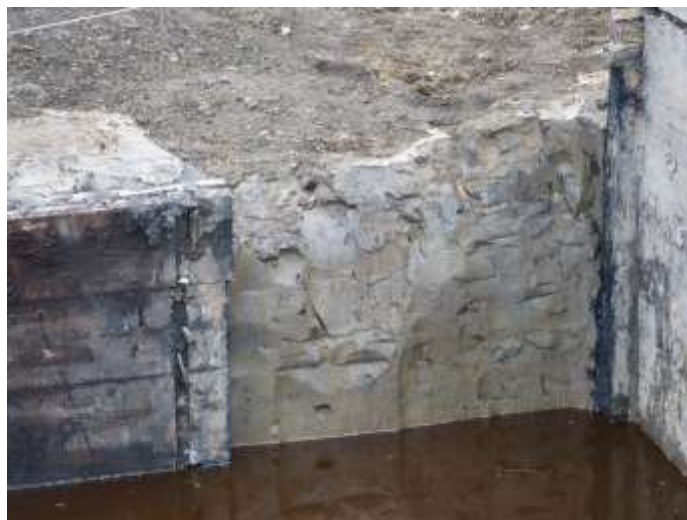
Plate 6: Clay packing exposed in the west face of Pit 2. The channel in the timber lining of the pit for a partition wall can be seen to the left.
