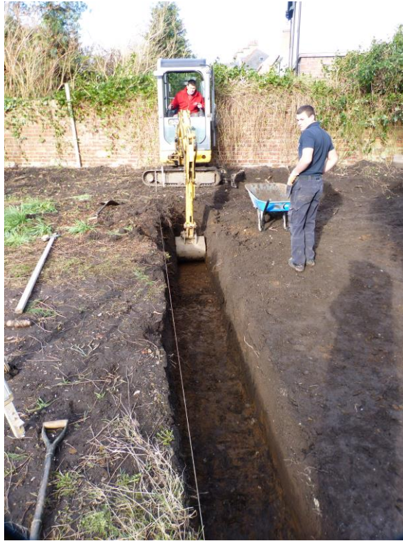
Plate 3: Completing the machine excavation of the south trench of the garage. Looking west.
