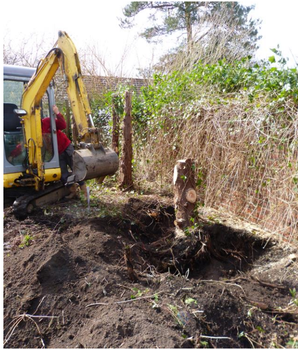
Plate 1: looking south during removal of the leylandii hedge along the western boundary of the site.
