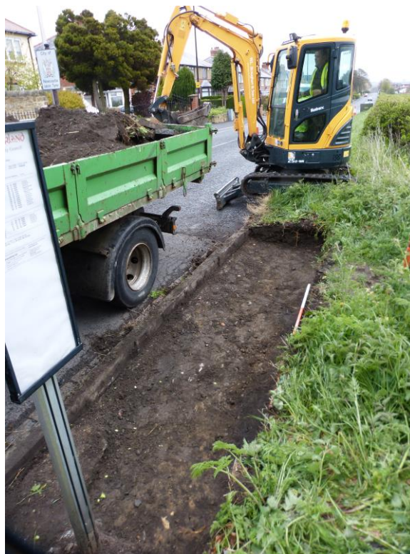
Plate 3: Clearing the site. Excavations extended only marginally deeper than the current road surface
