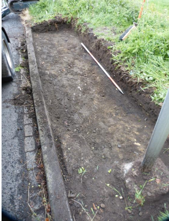
Plate 1: Looking east. Footprint of the new area of hardstanding stripped. Compacted sand and gravel exposed at base with a number of concrete fragments set in this deposit. 2m ranging rod.
