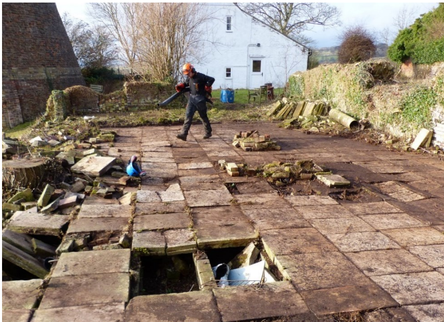
Plates 23 and 24: Pre (top) and post-clearance views of the drying floor (building 7) between the bottle kilns. Looking west.
