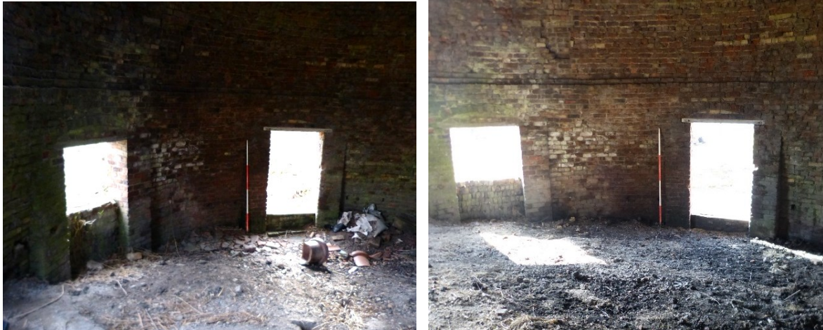
Plates 31 and 32: Pre (left) and post-clearance views of the interior of the eastern bottle kiln. Looking south. 2m scale.
