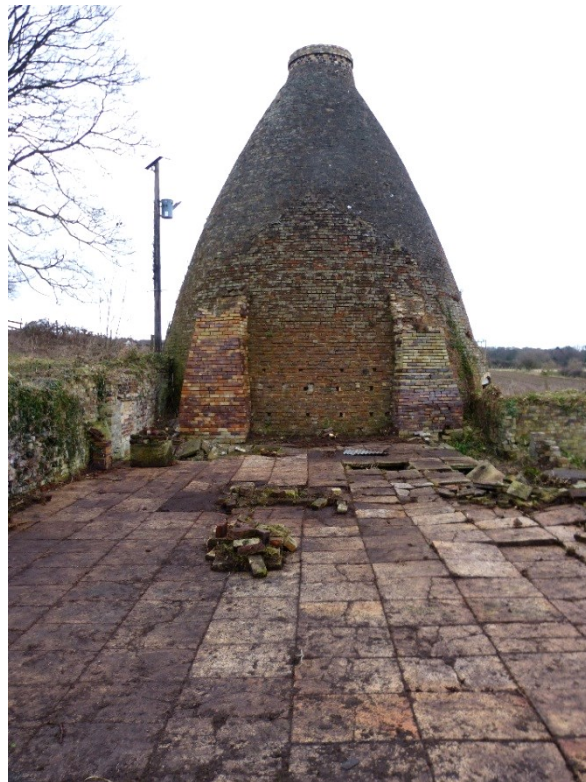
Plate 27: Drying floor (building 7) post clearance. Looking east towards the east bottle kiln.
