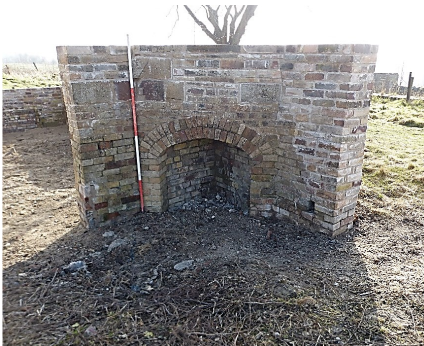
Plates 15 and 16: Fireplace in the south-east corner of the middle room of building 8 to the south of the eastern bottle kiln. Pre (top) and post conservation. 2m scale.
