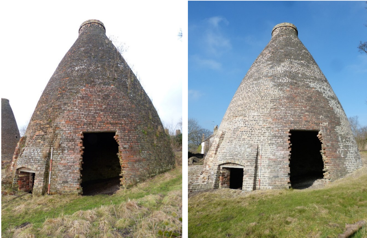
Plates 13 and 14: Eastern bottle kiln from the east. Original south-east entrance at left and late entrance at centre. Pre (left) and post conservation. 2m scale.
