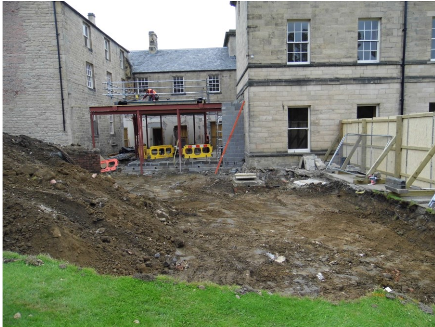
Plate 8: Reduced ground level west of Close House. Looking east.
