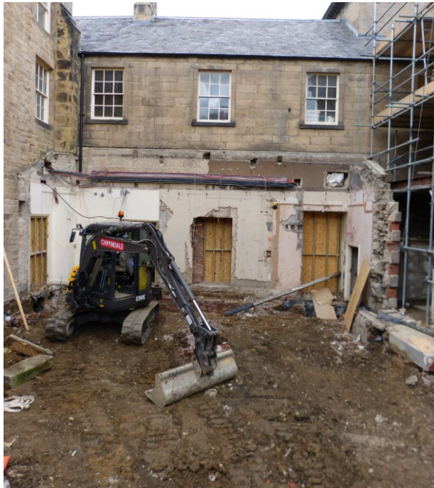
Plate 2: Courtyard post removal of floor slabs and during reduction of ground level. Looking east.
