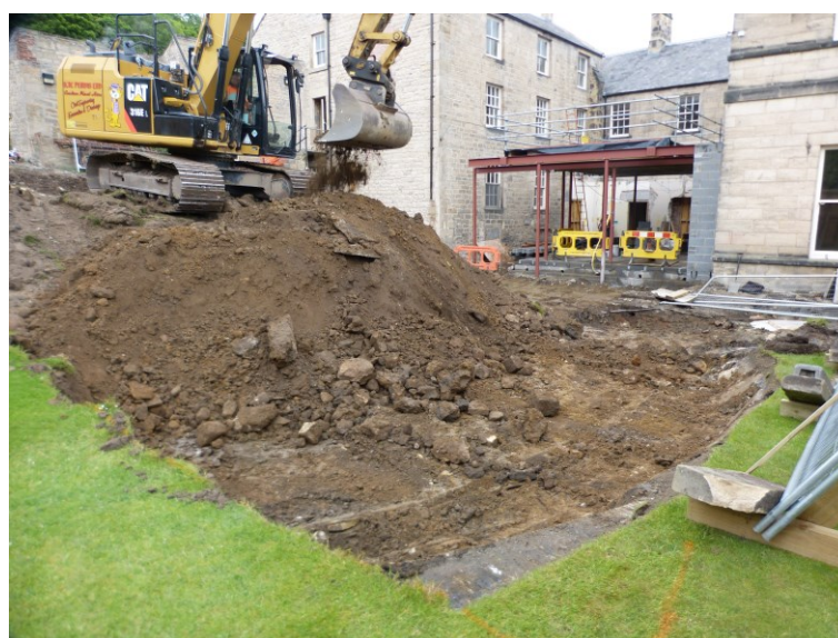
Plate 7: Reducing ground level west of Close House for the garden room. Looking north-east.
