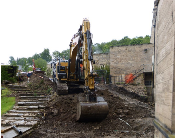
Plate 10: Beginning to cut back the slope north of the Garden Room for the retaining wall. Looking north.
