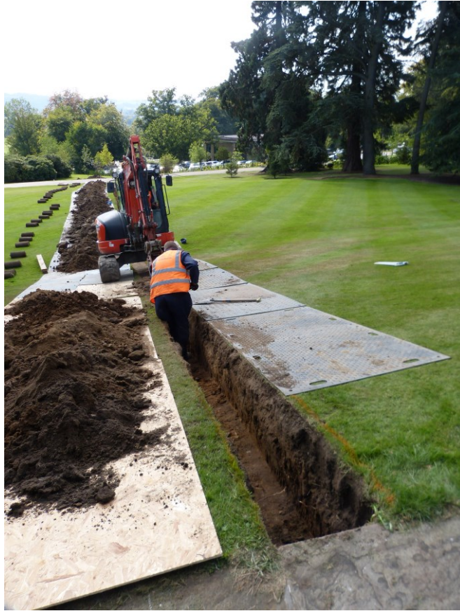
Plate 15: Excavation of the north end of service trench (5) next to the Orangery. Looking south.
