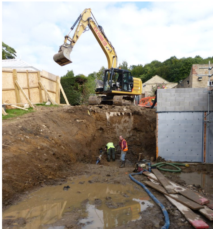
Plate 13: Deep excavation at the north end of the Garden Room with retaining wall to right.
