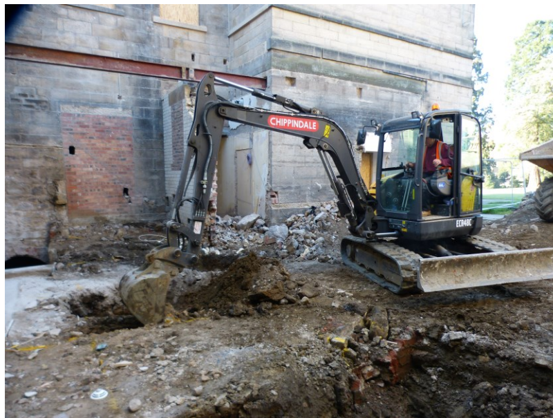
Plate 5: Cutting foundations for the library room structure. Looking south-west across the courtyard.
