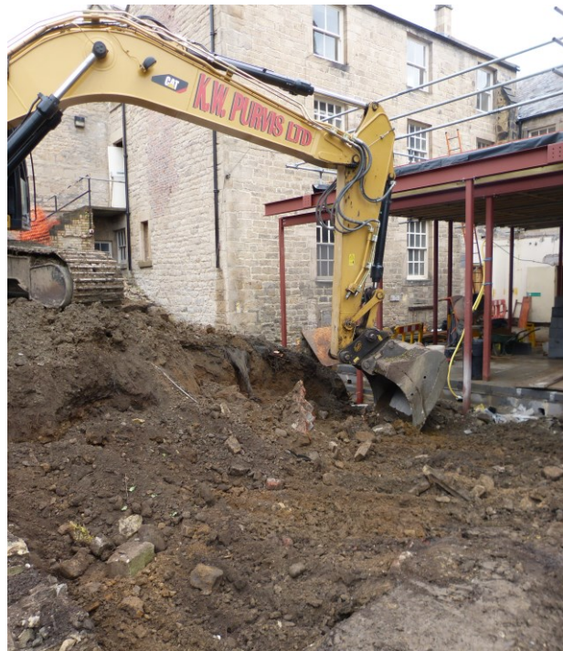
Plate 6: Reducing ground level west of Close House for the garden room. Looking north-east.
