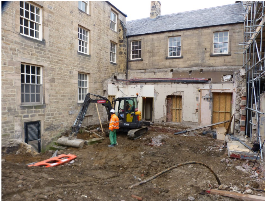
Plate 1: Courtyard post removal of floor slabs and during reduction Of ground level. Looking north-east.
