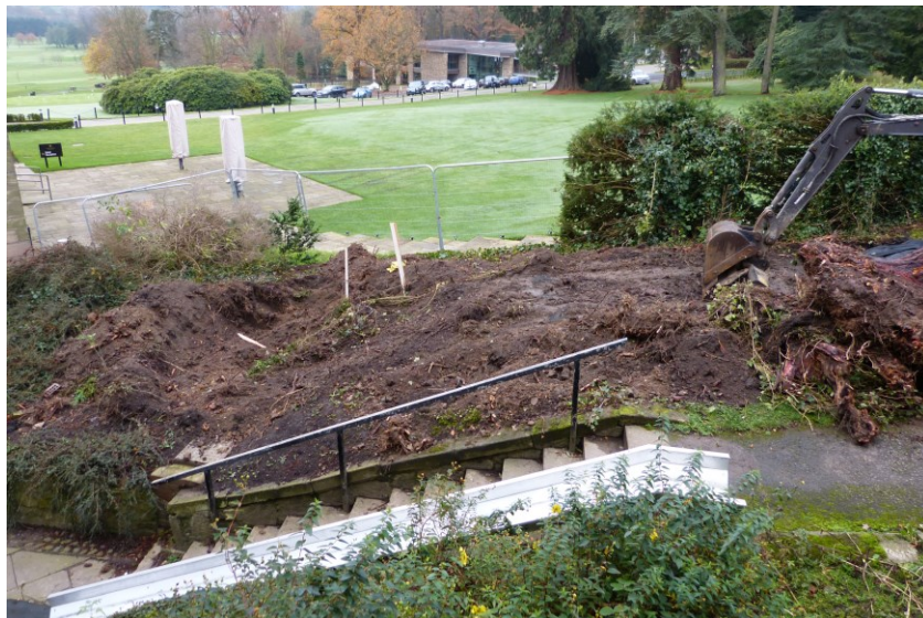
Plate 9: Removing topsoil from the slope next to the Garden Room. Looking south-west.
