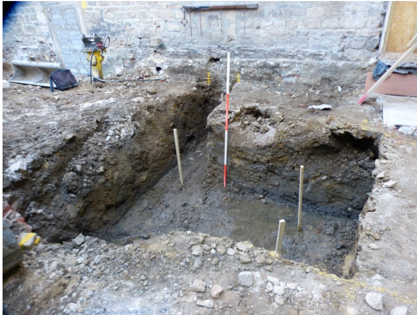
Plate 4: Foundation pit for the library room structure within the courtyard. Looking north.
