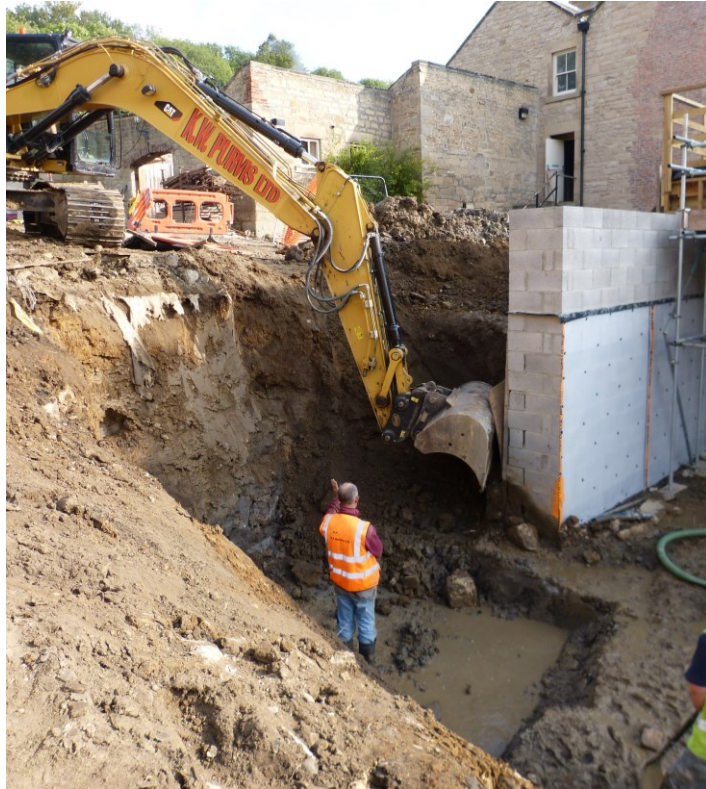
Plate 12: Deep excavation at the north end of the Garden Room with retaining wall to right. Services and other intrusions had previously cut deeply into the area. Looking east.
