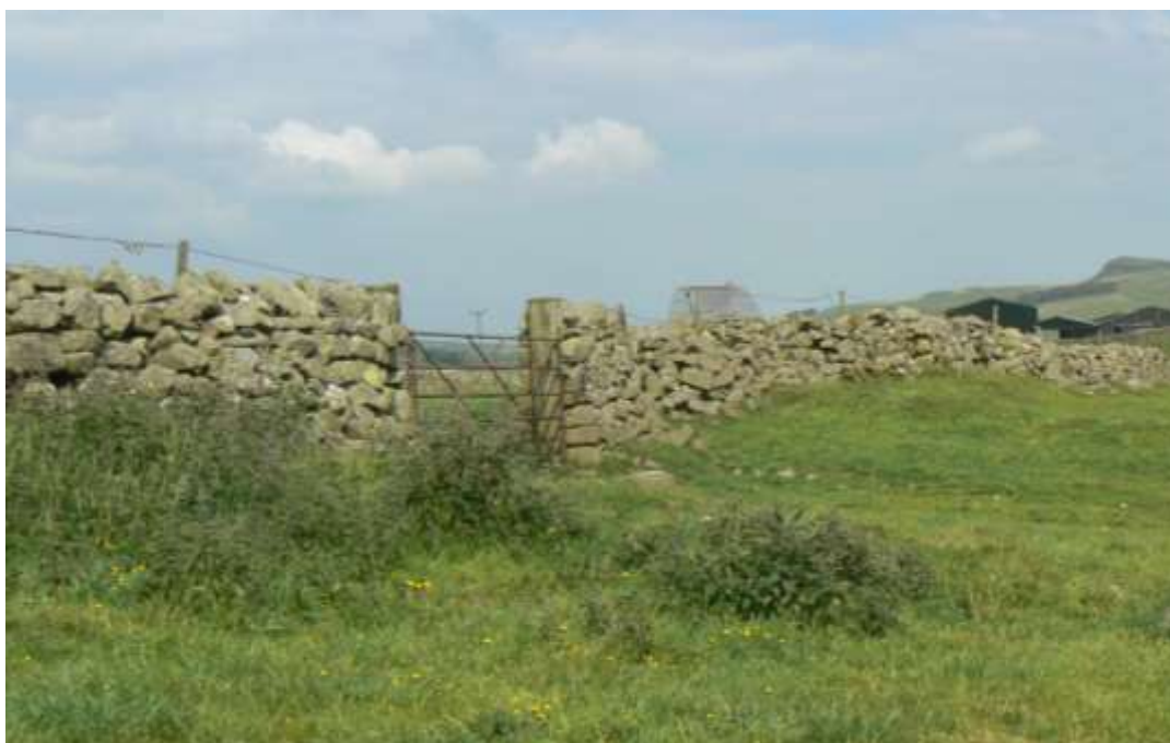
Plate 18: Slumped dry-stone wall west of Great Chesters. Looking east.
