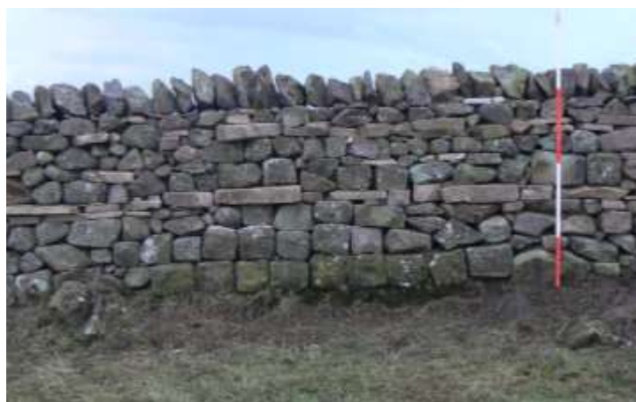
Plate 13: Roman fabric embedded at the base of the north face of the rebuilt dry-stone field wall. West of Great Chesters. 2m scale.
