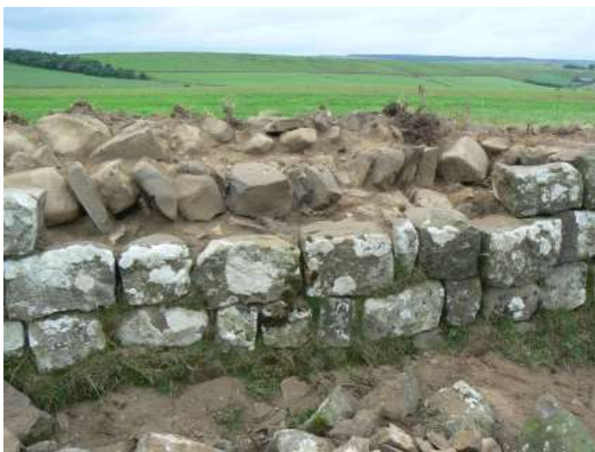
Plate 25: East of Great Chesters. South face of the Wall with core in distinct courses.
