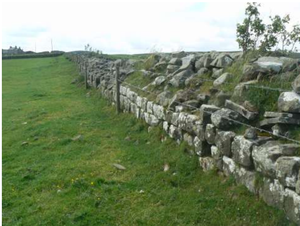
Plate 27: East of Great Chesters. Looking west along the Wall prior to conservation work. Much of the structure is in-situ Roman with a badly decayed overlying dry-stone wall .
