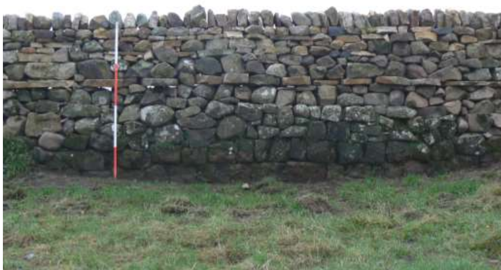
Plate 34: East of Great Chesters. The north face of the rebuilt dry-stone wall with Roman fabric at the base. 2m scale.
