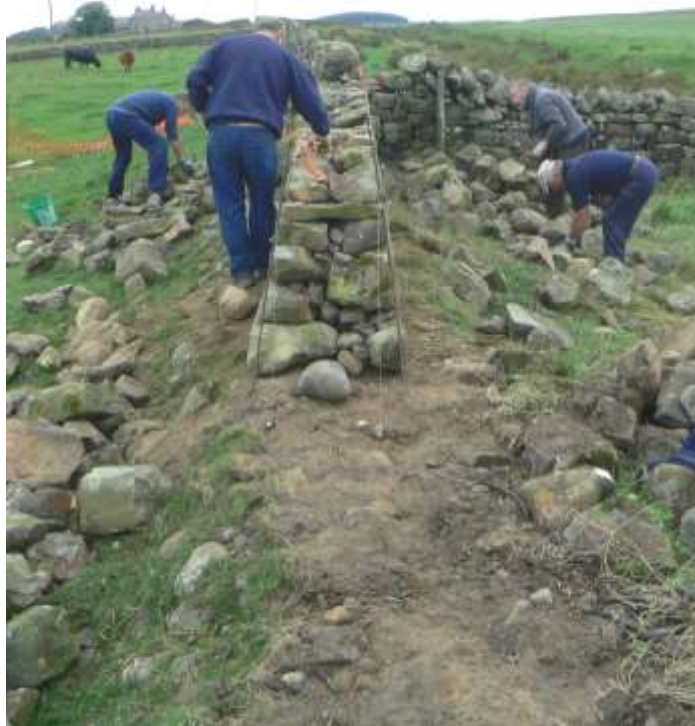
Plate 23: Rebuilding dry-stone wall over the Wall mound. East of Great Chesters, looking west.
