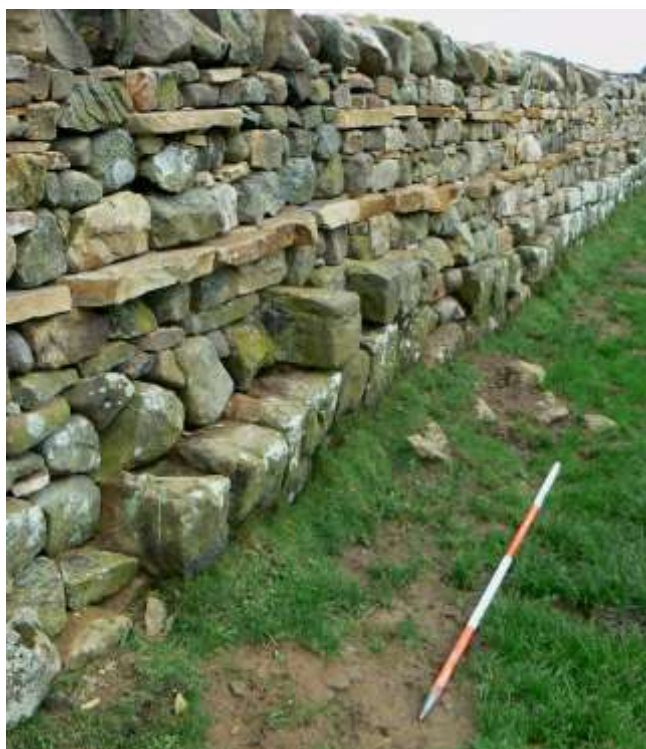
Plate 36: East of Great Chesters. Roman fabric at base of south face of rebuilt dry-stone wall. 2m scale.
