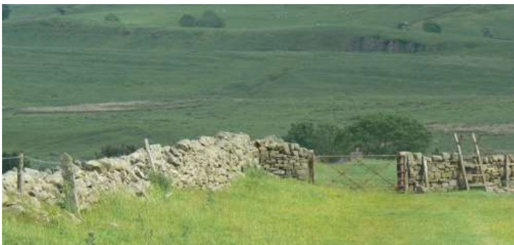
Plate 14: Slumped Dry-stone wall east of Great Chesters looking east towards Burnhead in 2013.
