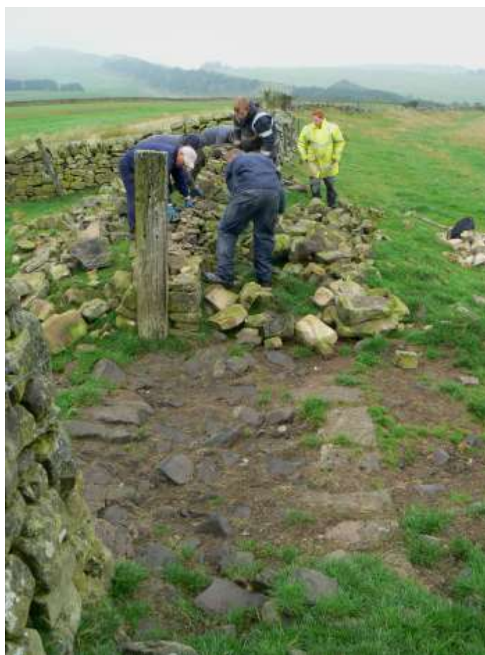
Plate 22: Removing the dry-stone wall east of Great Chesters south face of Hadrian's Wall exposed in the gateway. Looking east.
