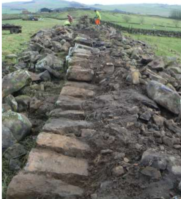
Plate 33: West of Great Chesters looking east. Exposed Roman facing stones (same block as seen in plates 29 and 30) with new dry-stone wall advancing in the background.
