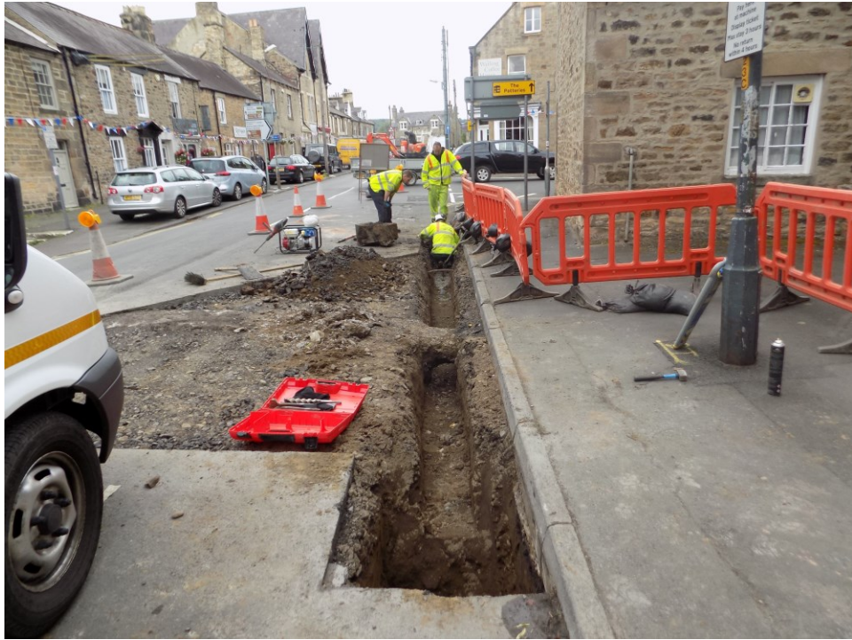
Plate 3: Service trench excavated along the kerbline, gully excavations to either end. Looking north.
