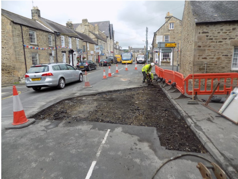
Plate 1: Road surface cut away for the new traffic island. Looking north along Watling Street.
