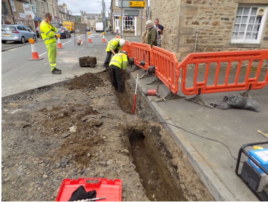
Plate 5: Removing the existing gully at the north end of the works. 1m scale.
