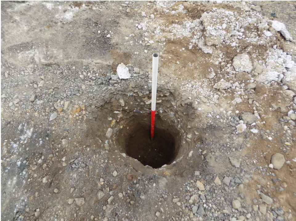
Plate 4: Excavation for new sign post within the area of the traffic island. 1m scale.
