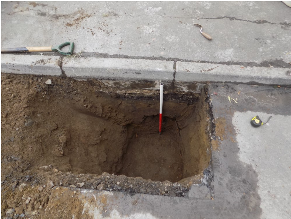
Plate 2: Excavation for new gully at the south end of the works, to a depth of 1.2m showing road construction and sand [04] below. Looking east. 1m scale.
