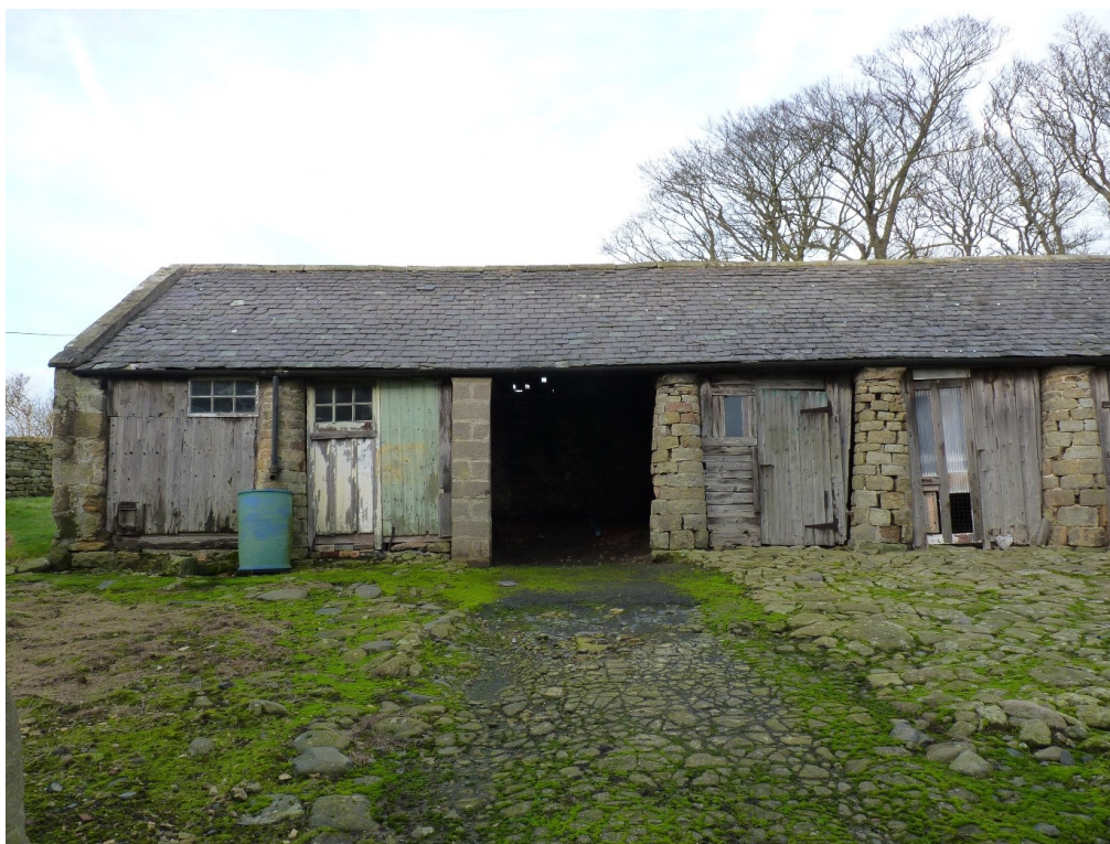
Plate 5: The south face of building (C). Looking north. Bays between columns have been infilled with timber.
