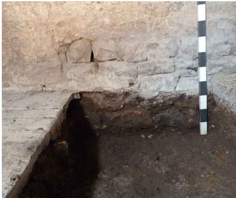
Plate 8: Test Pit 3, against the inner face of the north wall of building C, showing the depth of foundations of the wall and clay subsoil within the pit. 1m scale.
