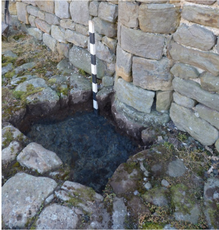
Plate 11: Test Pit 5, against the outer face of the wall of building C fronting the east side of the yard. The cobble surface and pillar base sit directly over grey clay subsoil 1m scale.
