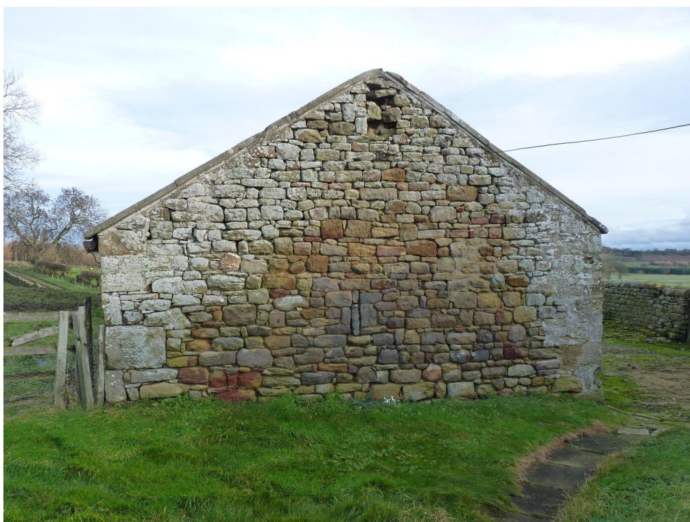
Plate 6: The west gable wall of building (C). Looking east. This would be the location of Trench 1.
