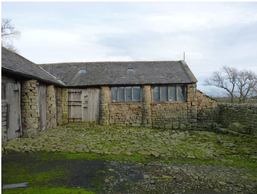
Plate 4: The west face of stone-built agricultural range (C). Looking east across the yard. Originally open between the columns, the bays were at some point infilled with stone.
