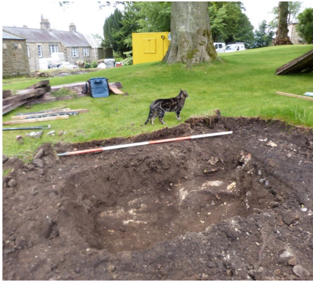
Plate 16: Trench 1 in the area of the new Bio-Mass Building. Looking south. Face of sandstone bedrock exposed in section 0.5m below ground surface.
