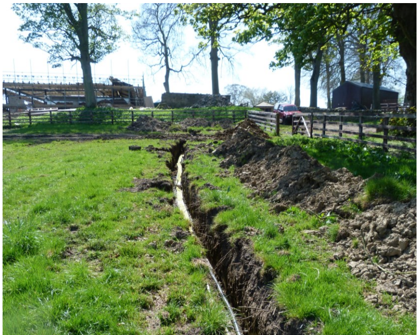
Plate 1: Mains cable running in from the north.
