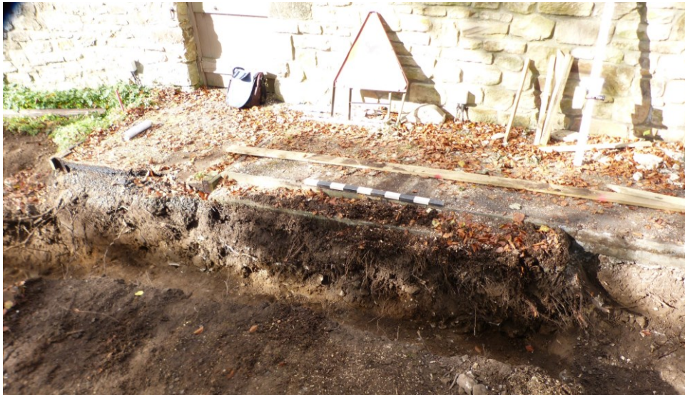
Plate 9: Location of the new eastern gatepost. Looking south-west. On the projected line of the north mound of the Vallum.
