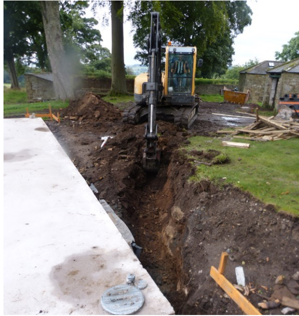
Plate 18: Excavation of trench for service pipes to Outbuilding 1 from the new Bio-Mass Building. Looking east.
