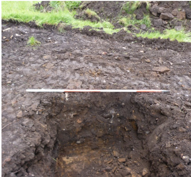
Plate 17: Trench 2 in the area of the new Bio-Mass Building. Looking north. Sandstone bedrock exposed at the base of the pit at c.1m deep.
