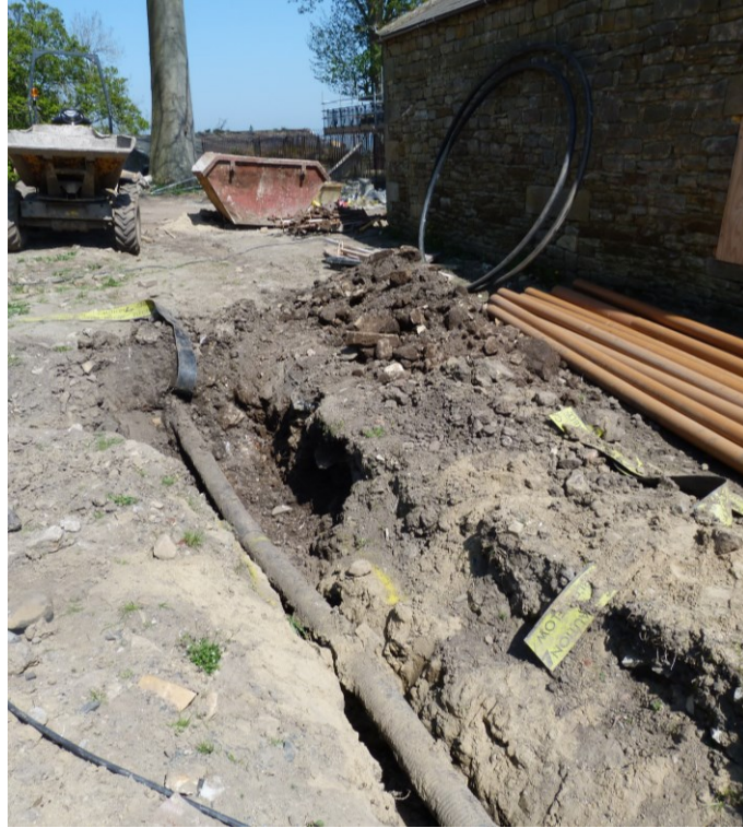
Plate 2: mains cable exposed between outbuildings. Looking north.
