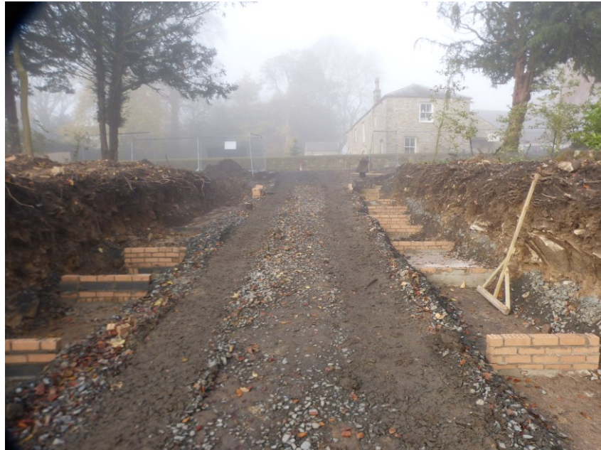
Plate 14: The ramp under construction, looking west towards Walwick Lodge. Bedrock is exposed along the flanks.
