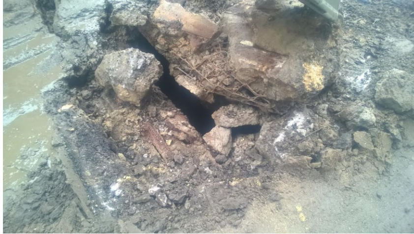
Plate 1: the well as first exposed. The concrete reinforced cap had slumped.
