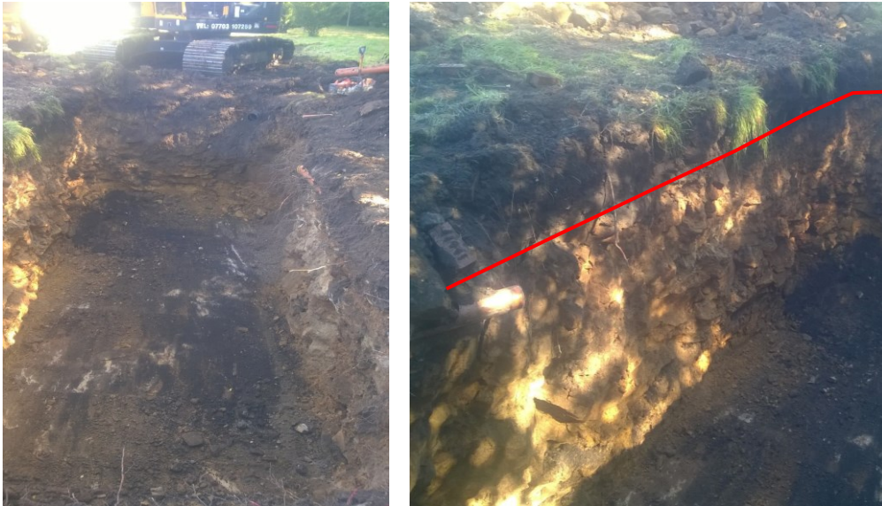
Plates 5 and 6: Excavation of the slightly enlarged pit for replacement of the package treatment plant. Red line in plate 6 indicates level of sandstone bedrock exposed across the pit.
