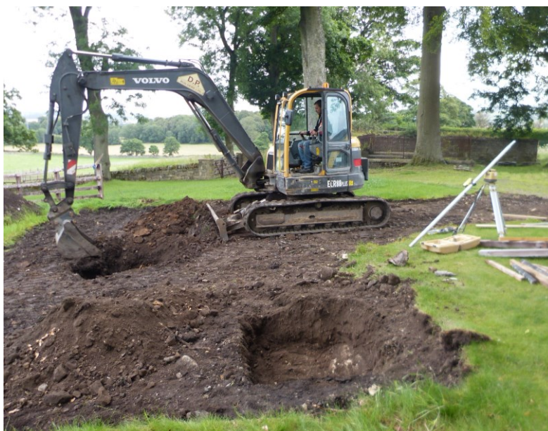
Plate 15: Machine excavator digging test pit 2 in the stripped footprint of the new Bio-Mass Building. Looking east.
