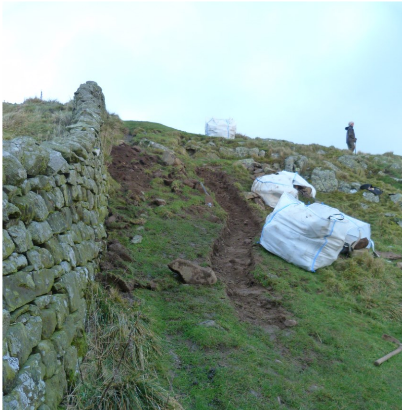
Plate 13: The same area as shown on plate 12, during excavation of the foundation slot or 'tray' for the pitched stone steps. Looking east.
