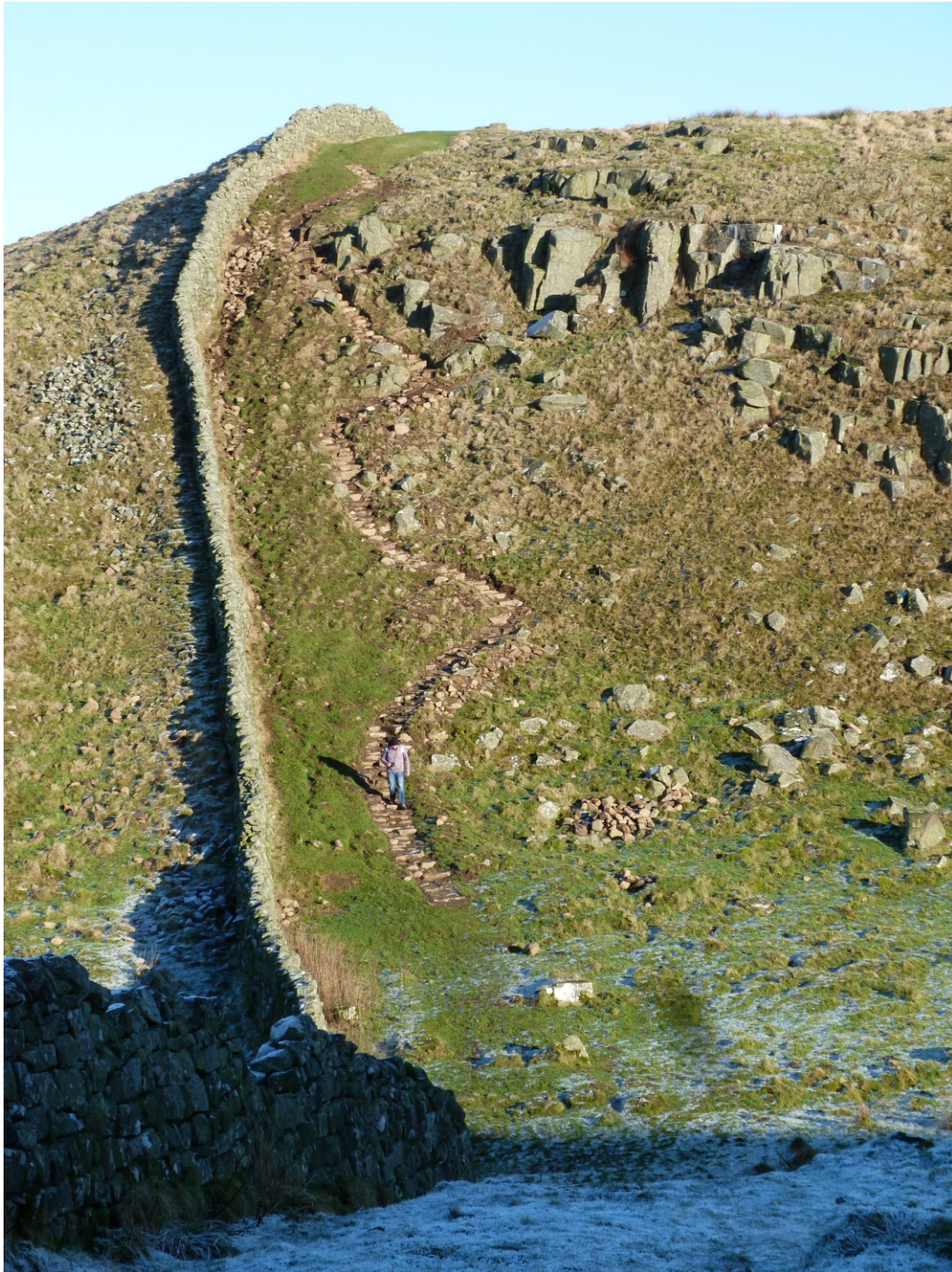
Plate 3: Area A. Looking east, following completion of the pitching. The developed path utilised natural contour to create an easier route.
