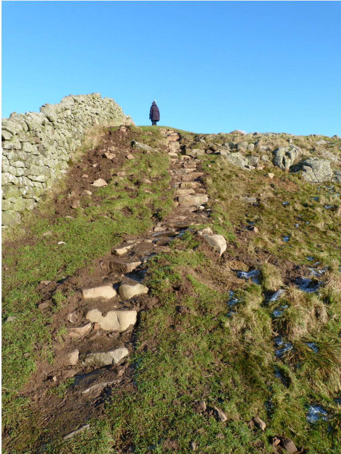
Plate 14: The same area as shown on plate 12 following completion of the pitching works. Looking east.
