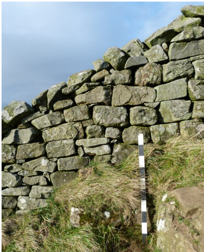
Plate 5: Area of deep erosion with exposed bedrock. Area A looking north. Dry stone wall overlies the Roman Wall. Possibly insitu facing stones exposed at base of 1m scale.
