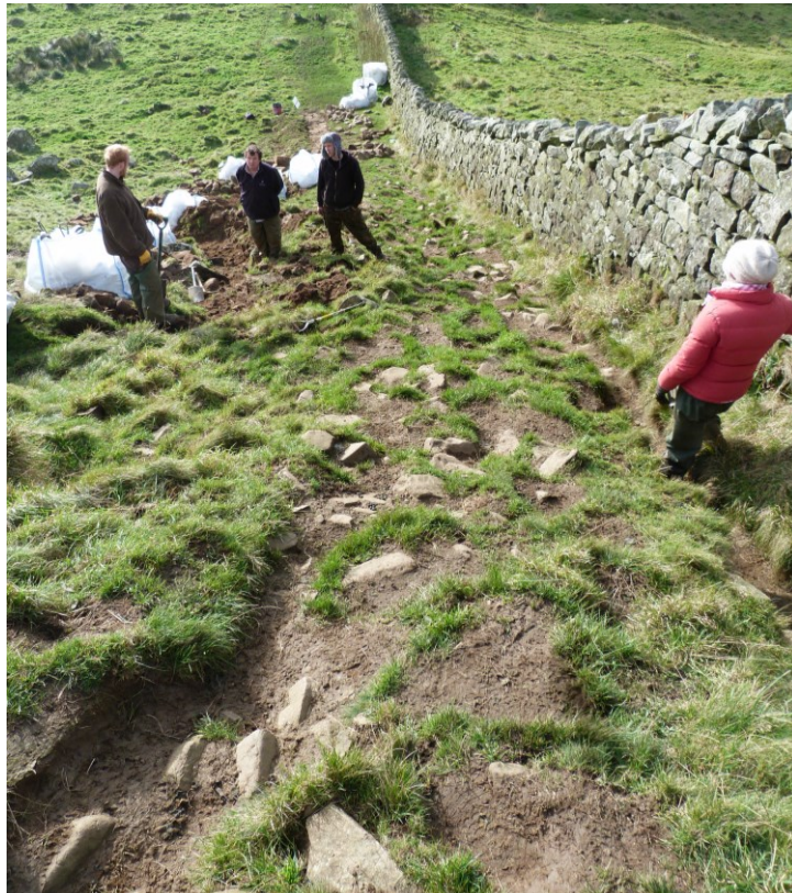
Plate 7: Looking west. Area A. Manual excavation for the 'tray' or slot. Working upslope.
