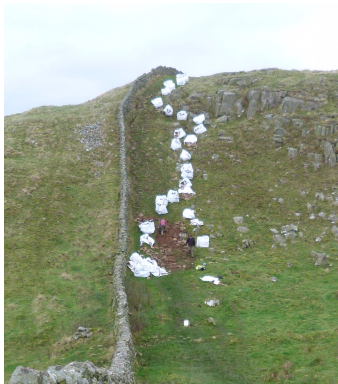
Plate 2: The same area as works commenced. The white sacks hold the air-lifted pitching stone.
