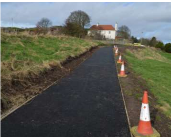
Plates 5, 6 and 7: Looking north at work progressing to the south of Fields House. Upper: East kerb fixed with groundworks progressing on the west flank; Middle: Compacting sub-base; Lower: The new path completed. Soil removed from the west flank was spread to the east.
