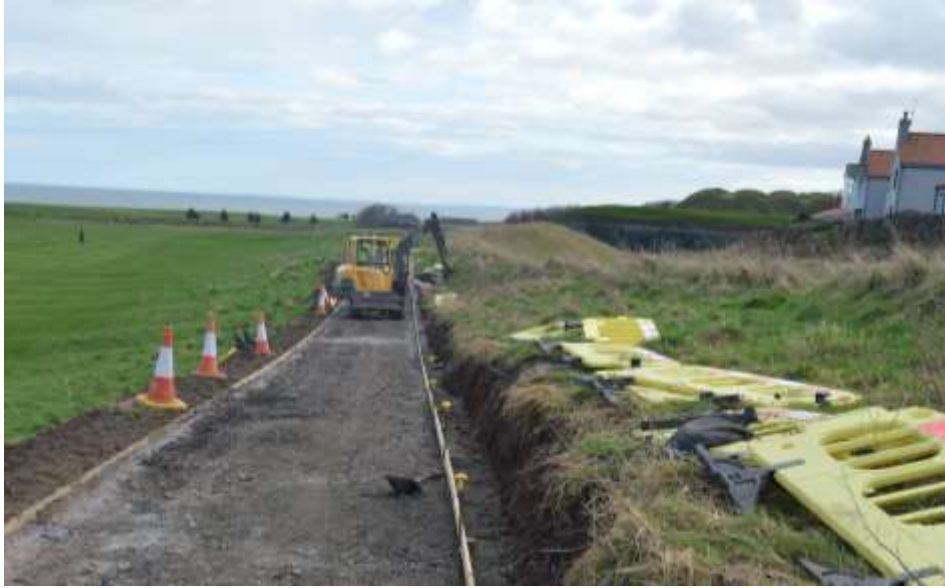
Plate 11: The maximum encroachment into deposits west of the path. Looking south c.120m from Fields House.
