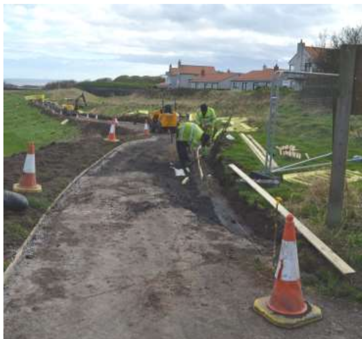
Plate 3: The new line defined with kerbing on both edges. Looking south just past Fields House, the Edwardian defences to the right
