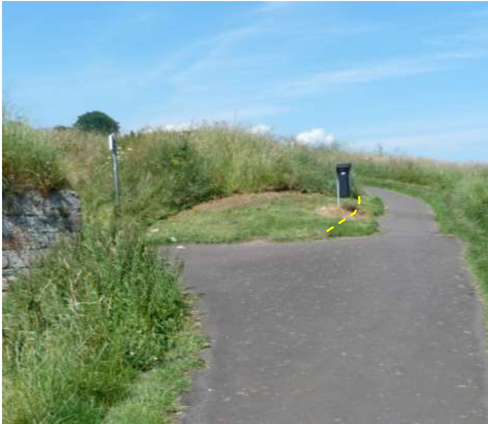
Plate 29: Before works. Located on figure 6. Looking north, Batardeau to left. Hatched yellow line shows intended widening.
