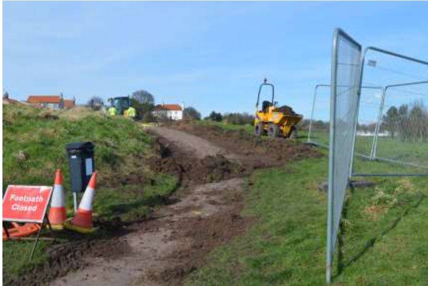
Plate 13: Just north of the batardeau, showing excavation along the east side of the path, avoiding the medieval earthwork to the west.
