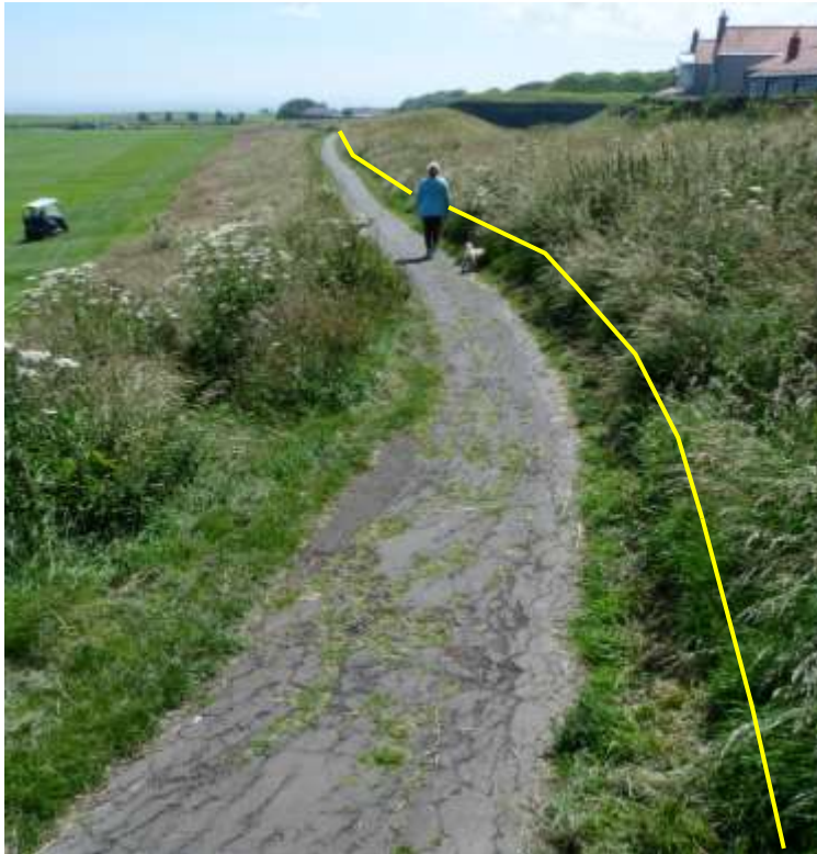
Plate 21: Before works. Looking south alongside Edwardian ditch (to right). Extent of counterscarp can be seen in distance. Yellow line shows intended widening.
