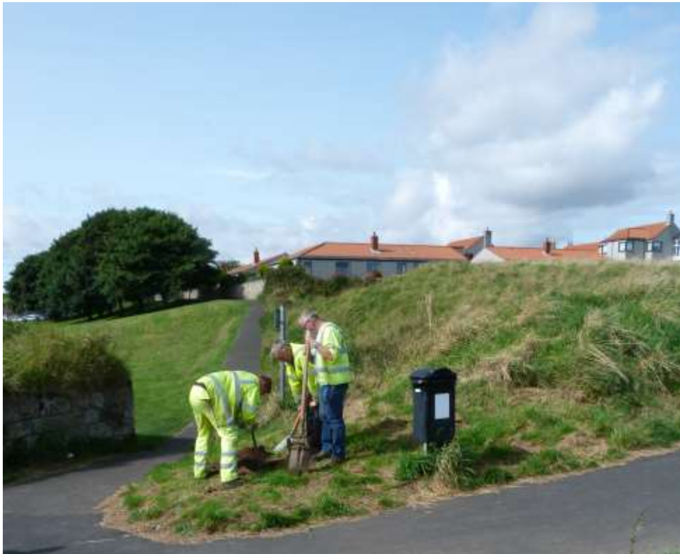
Frontispiece: Excavating a post hole for the new way-markers north of the Batardeau.
