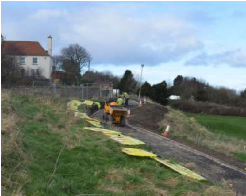
Plate 4: The surface of the old path stripped away and soil from trimming back the west flank of the path spread on the eastern slope.
