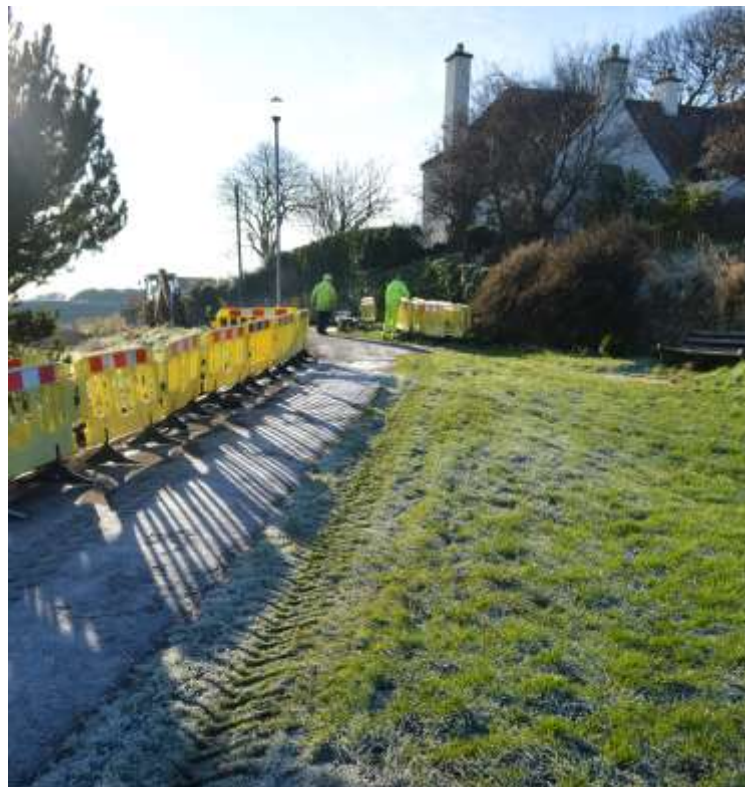
Plate 1: Working south towards Fields House at the north end of the footpath.
