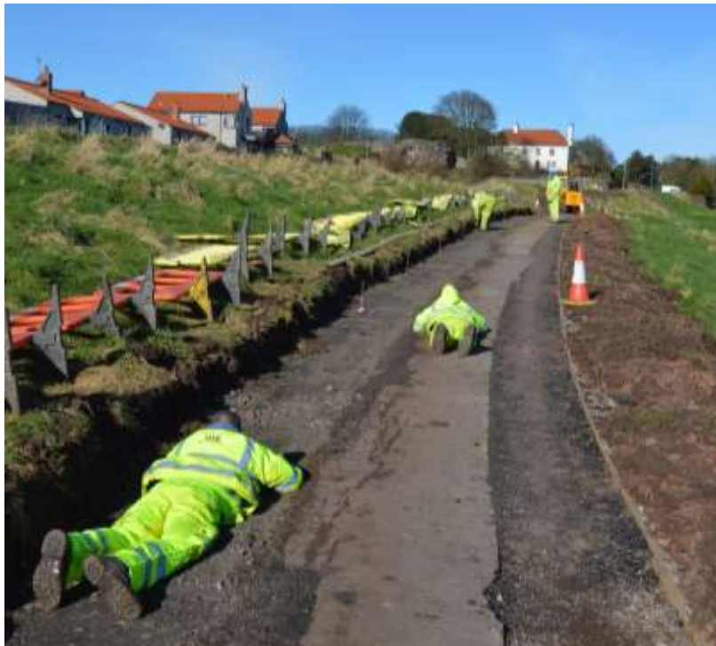
Plate 10: Checking the slope profile of the new path following completion of ground works.
