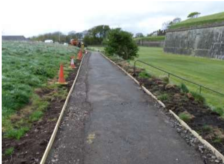
Plate 8: Wooden kerbing set out on the path alongside Brass Bastion. Looking south. In this area the path has been widened to the east.
