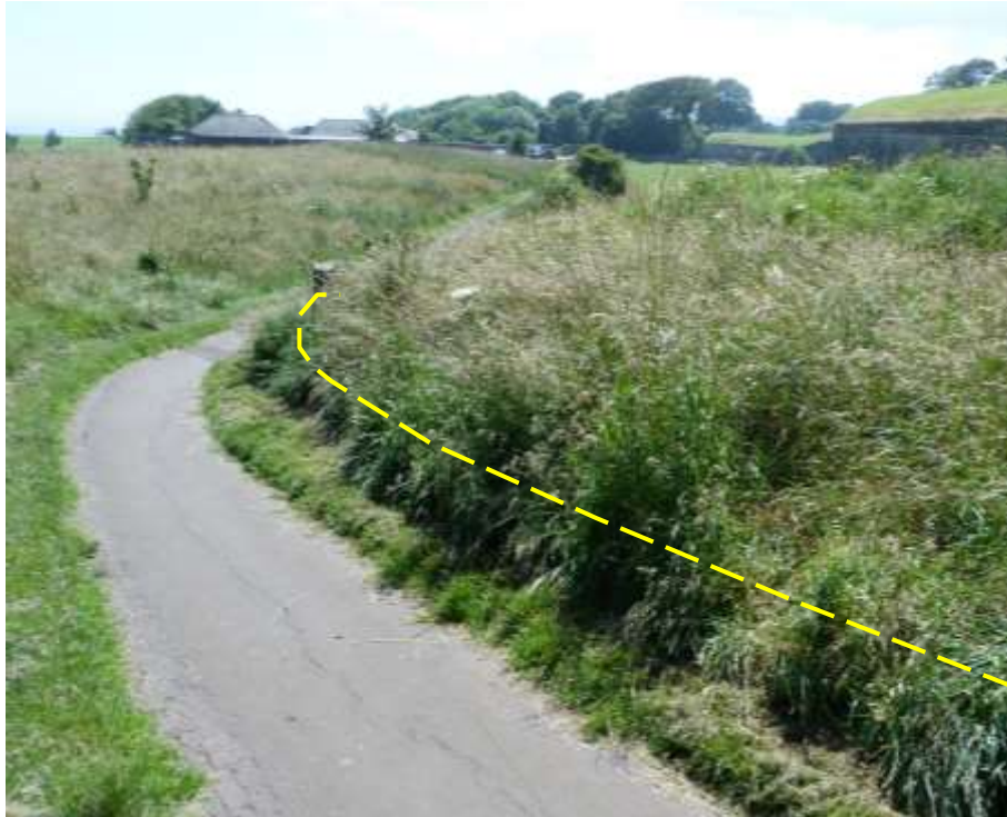
Plate 25: Before works. Located on figure 6. Looking south. Earthworks of north-east angle of Brass Bastion Counterscarp to right. Hatched yellow line shows intended widening.
