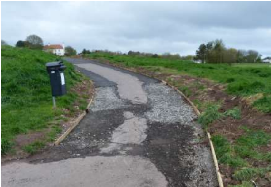
Plate 14: Same view as plate 13 with earthworks completed and kerbing laid for the wider path.
