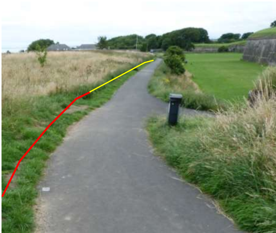
Plate 28: After works. Same as plate 27. Red line shows widening as carried out and continuation in yellow.
