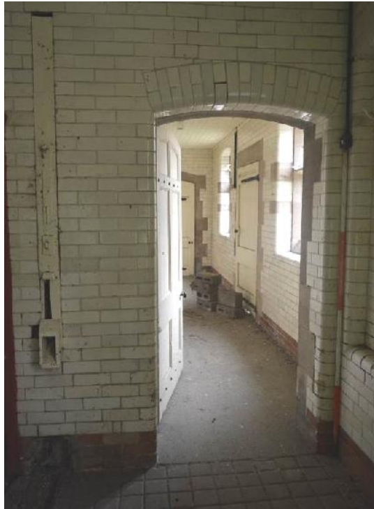
Plate 49: Passage way in front of the hay store from the west stalls. Looking east. Feed chute to left.
