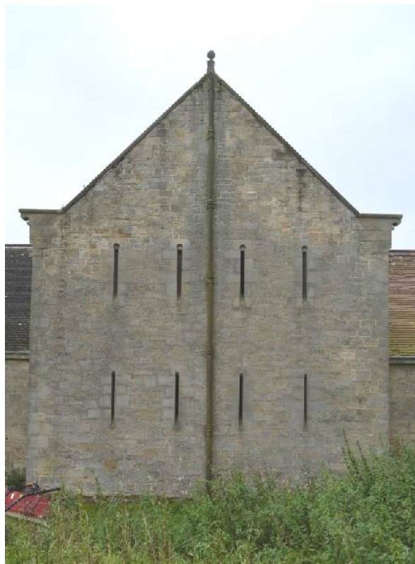
Plate 8: Projecting block in the north face of the north range. Looking south.
