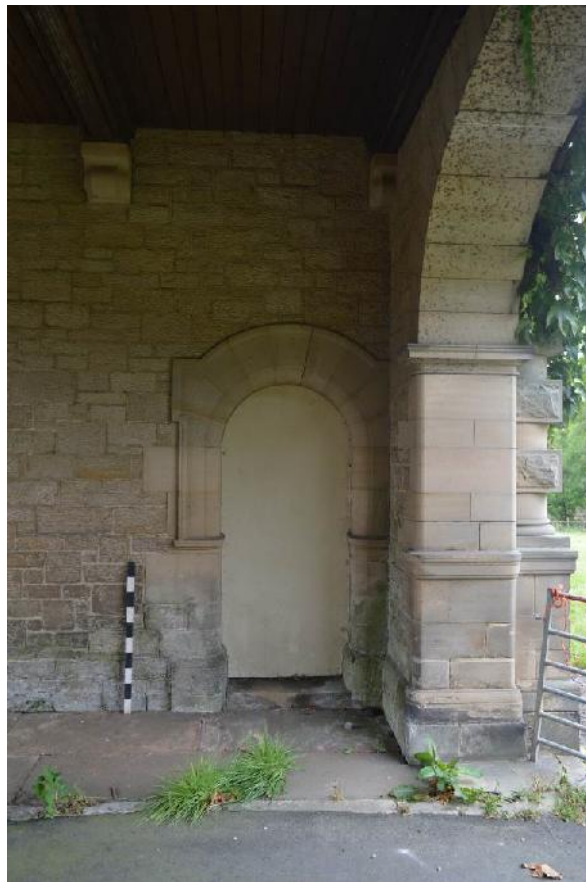
Plate 25: Boarded-up door on the east side of the entrance arch.
