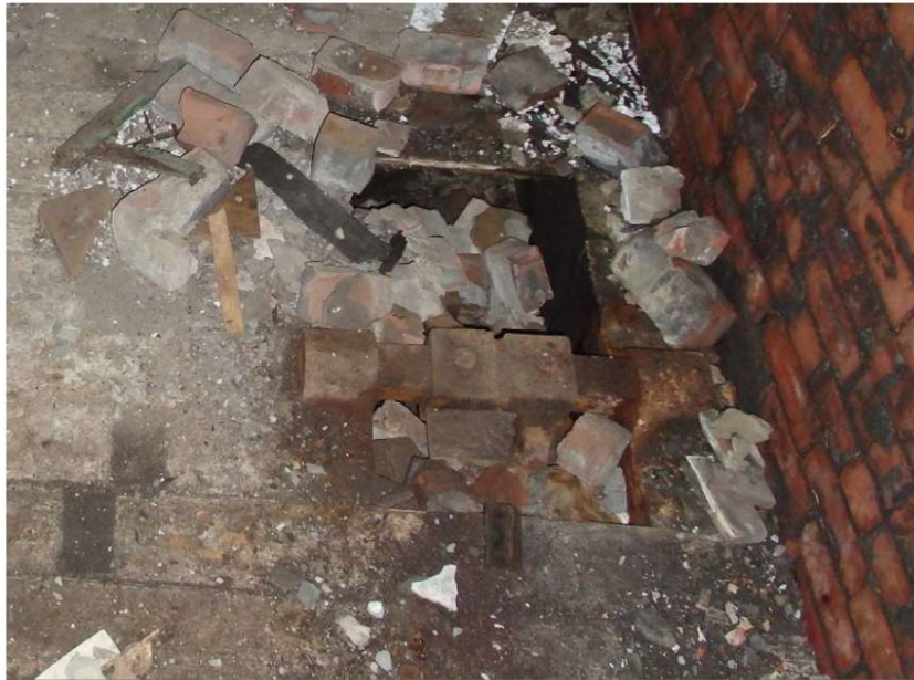
Plate 11: Ground-floor, looking north. Brake transmission lever in floor obscured by rubbish and building debris prior to clearance.
