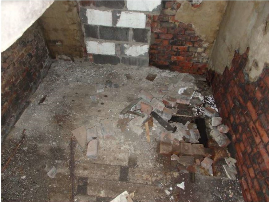
Plate 9: Ground-floor. Looking north. Blocked door in north wall of ground floor with obscured brake lever to the right.
