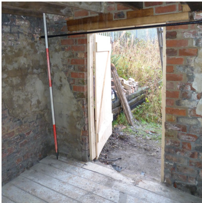
Plate 10: North-east wall after removal of door blocking and fitting of new door leaf.
