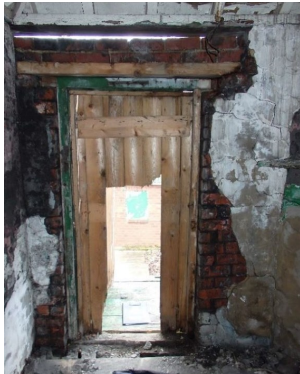
Plate 3: Looking south. First floor. Door in south-west wall before conservation.
