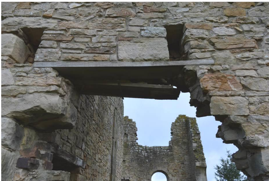
Plate 26: Defective lintel in the south wall of the Engine House in 2017.
