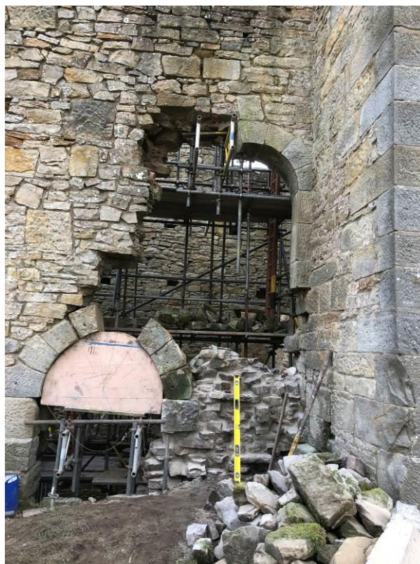
Plate 13: West face of the Engine House. Working on the arch and adjacent rebuilt masonry.
