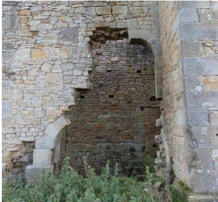
Plate 5: West wall of the Engine House in 2017. Looking east showing the two tumbled arches.
