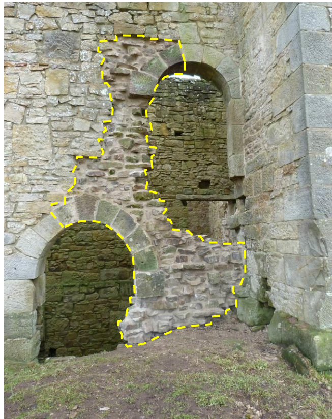
Plate 15: West face of the Engine House, both arches completed. Yellow broken line indicates rebuilt fabric.
