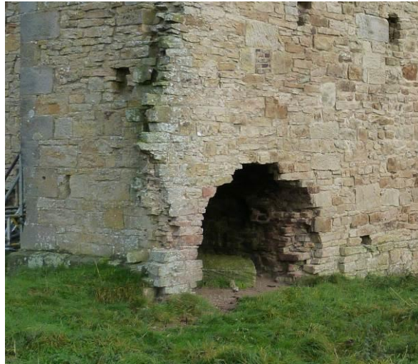
Plate 22: Opening in south face of the chimney flue prior to conservation works.
