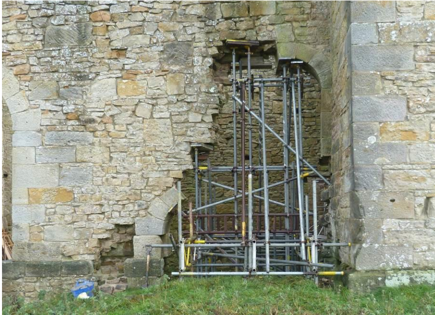
Plate 6: The west wall of the Engine House in 2019. Looking east. Scaffolding has been added to support the surviving parts of the arches.
