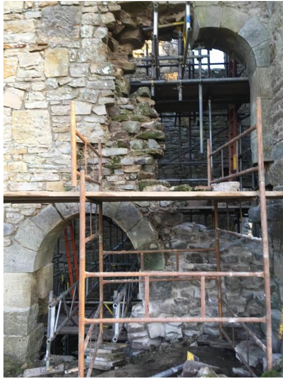
Plate 14: West face of the Engine House. Lower Arch completed. Work on upper arch underway.
