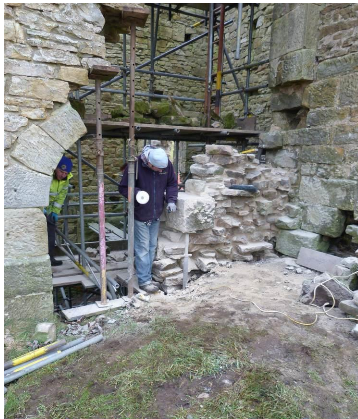
Plate 9: West wall of the Engine House looking south-east. Working on masonry built up to the south of one of the arches.
