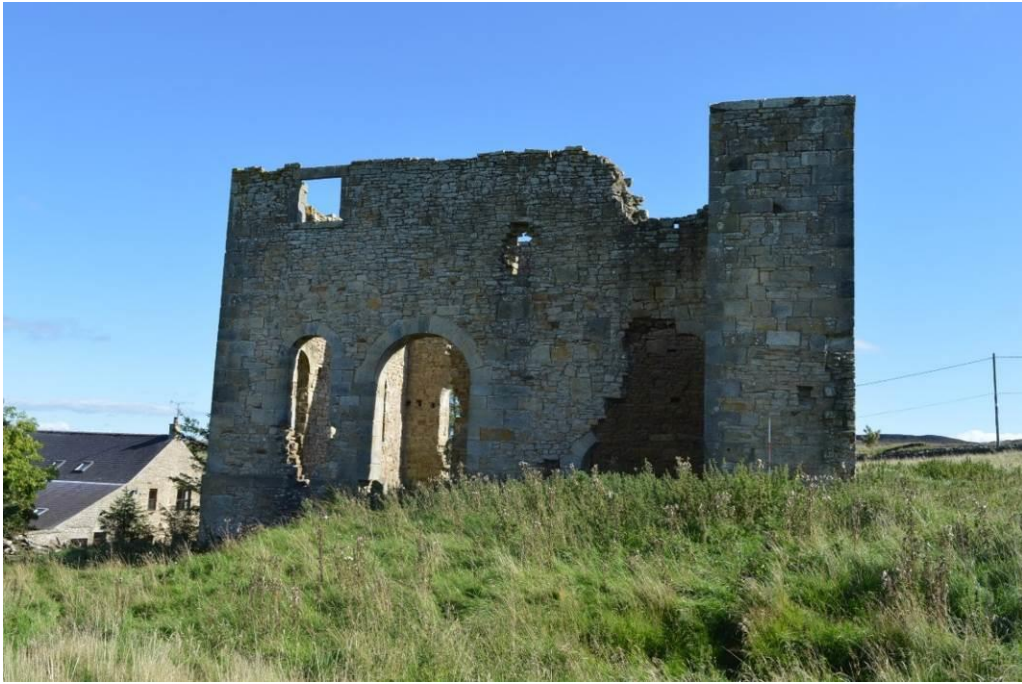
Plate 3: The engine house from the west, a square chimney forming the south-west corner.
