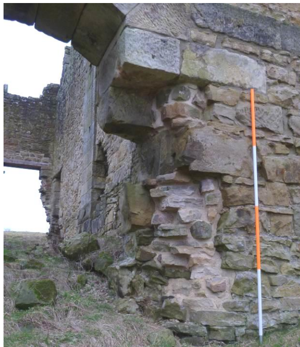
Plate 34: West jamb of east opening in the north wall of the engine house in 2019. Corework pieced in to support existing fabric.
