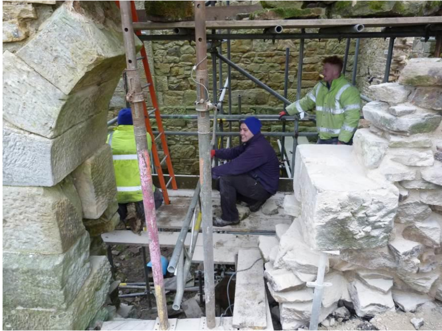
Plate 10: West wall of the Engine House, looking east. Rebuilt masonry to right.
