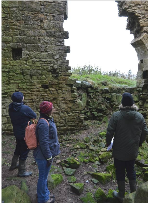
Plate 16: Inside the Engine House in 2017. Looking at tumbled arches in the west wall.
