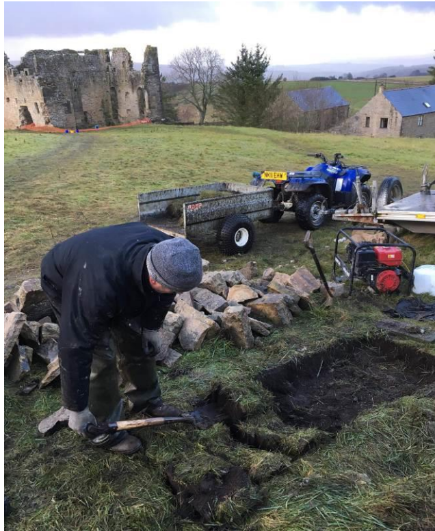
Plate 37: Beginning de-turfing for the foundation Slot of the new wall. Looking north-west.
