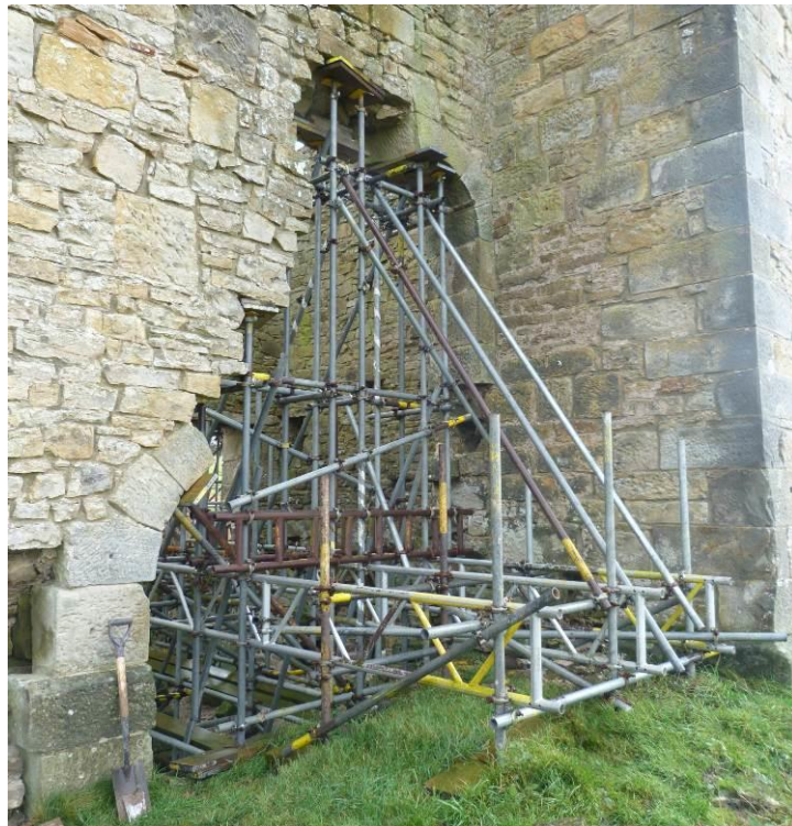
Plate 7: West wall of the Engine House looking south-east at scaffolding supporting the tumbled arches.
