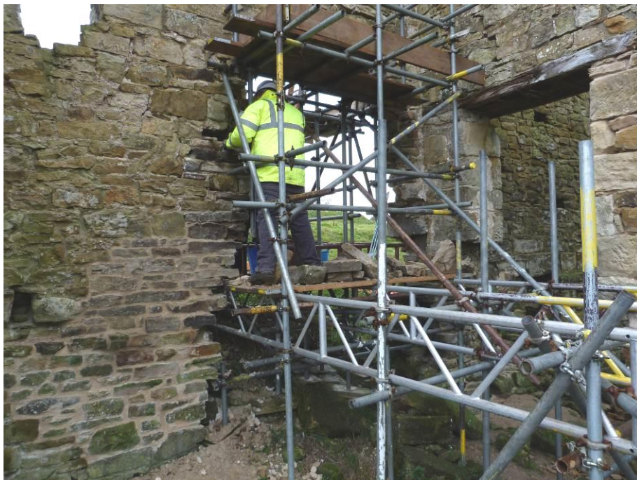
Plate 28: The opening in the south wall of the Engine House. Looking South-west during conservation works.
