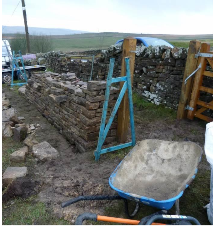
Plate 39: The new wall under construction; gate posts and gate in place. Looking north.
