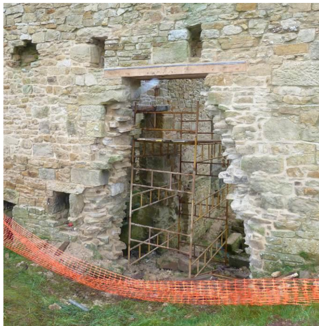
Plate 30: The opening in the south wall of the Engine House. Work completed in late 2018 with a new substantial timber lintel. Looking north-west.
