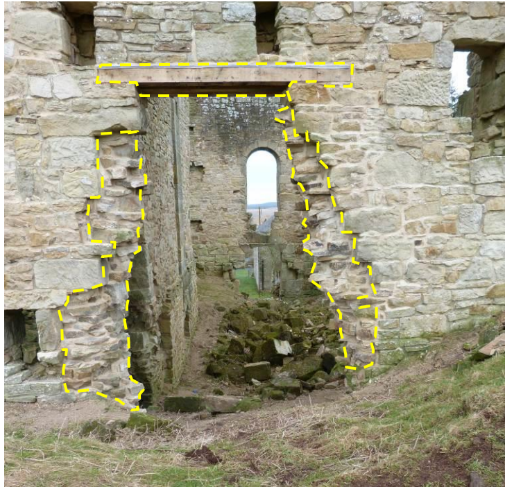
Plate 31: Opening in the south wall of the Engine House in 2019. Looking north. Inserted work in broken yellow line.
