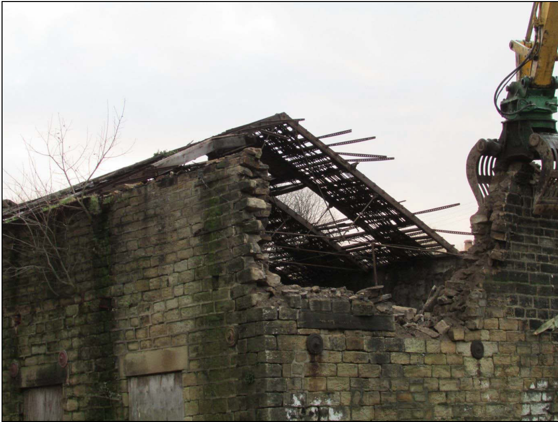
Plate 89 The west shed during demolition. The roof was constructed entirely from iron
