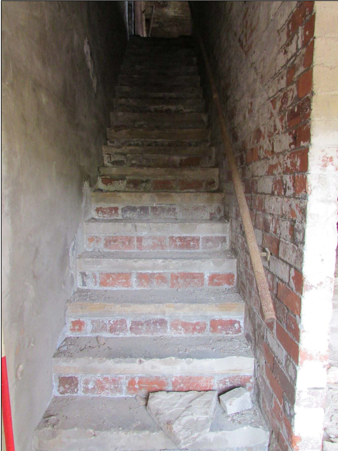
Plate 53 Later steps leading from the second to the third-floor of the engine house
