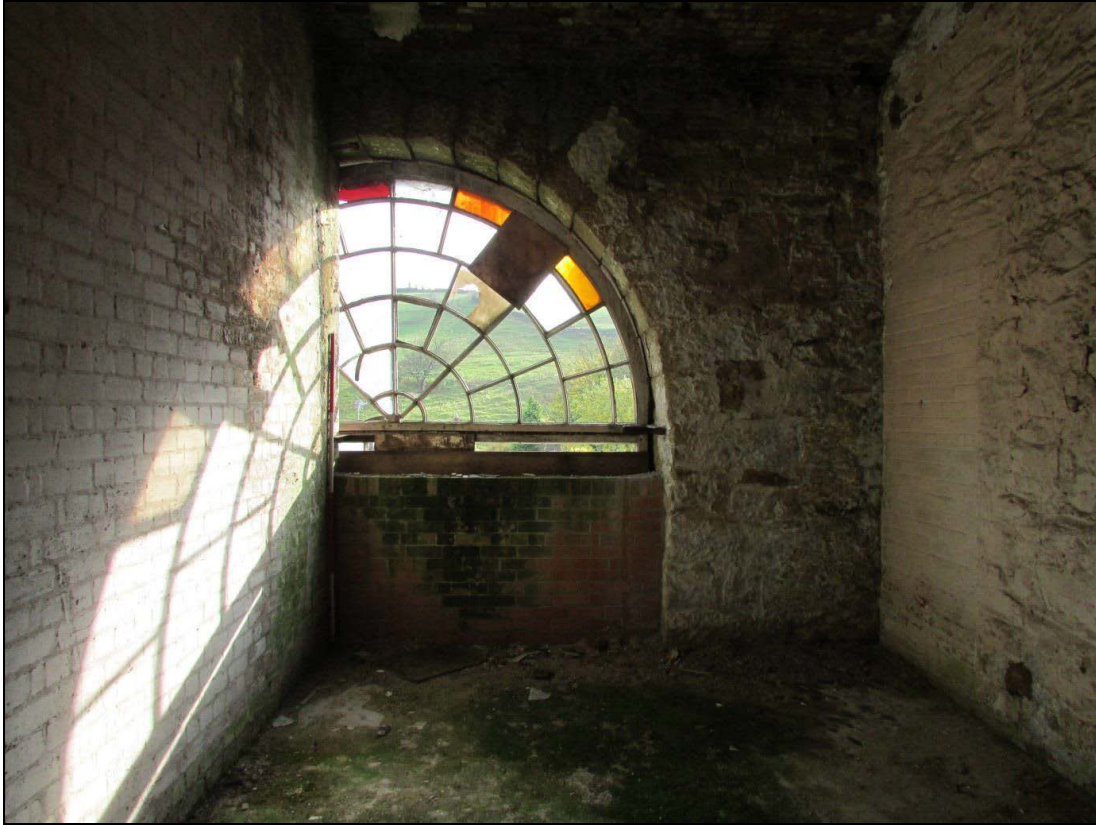
Plate 55 The original fanlight of the engine house was blocked by the lift shaft (to the left) and a c.1.00m high brick partition
