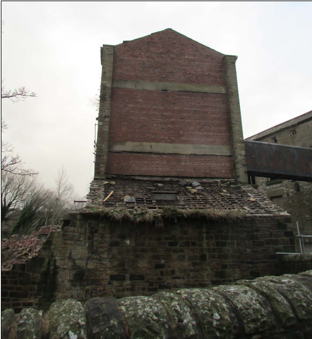
Plate 66 South elevation of the office block, which appears to have been rebuilt along with the stone lean-to on the ground-floor level
