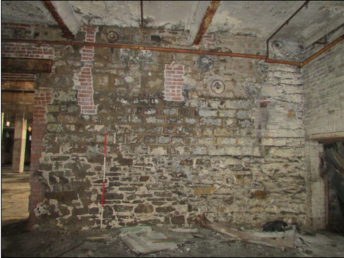
Plate 40 Examples of later brick repairs within the gearing wall, possibly after removal of the engine
