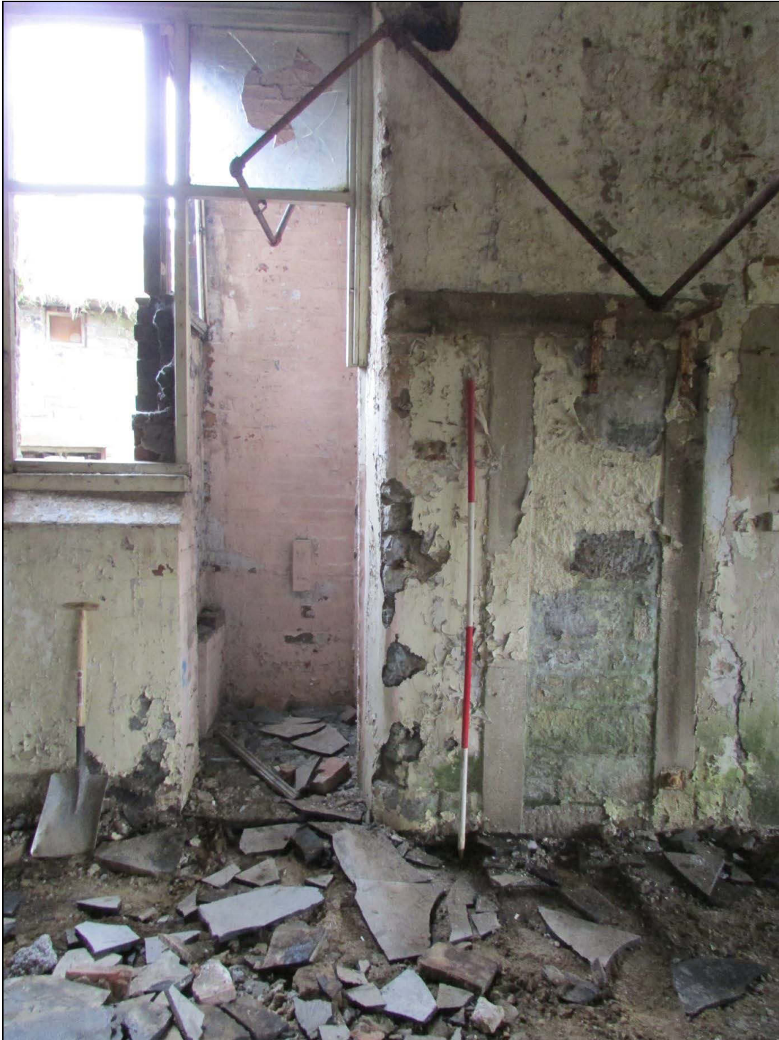
Plate 21 The entrance on the left leads into the privy tower extension and the blocked entrance led originally into the privy tower
