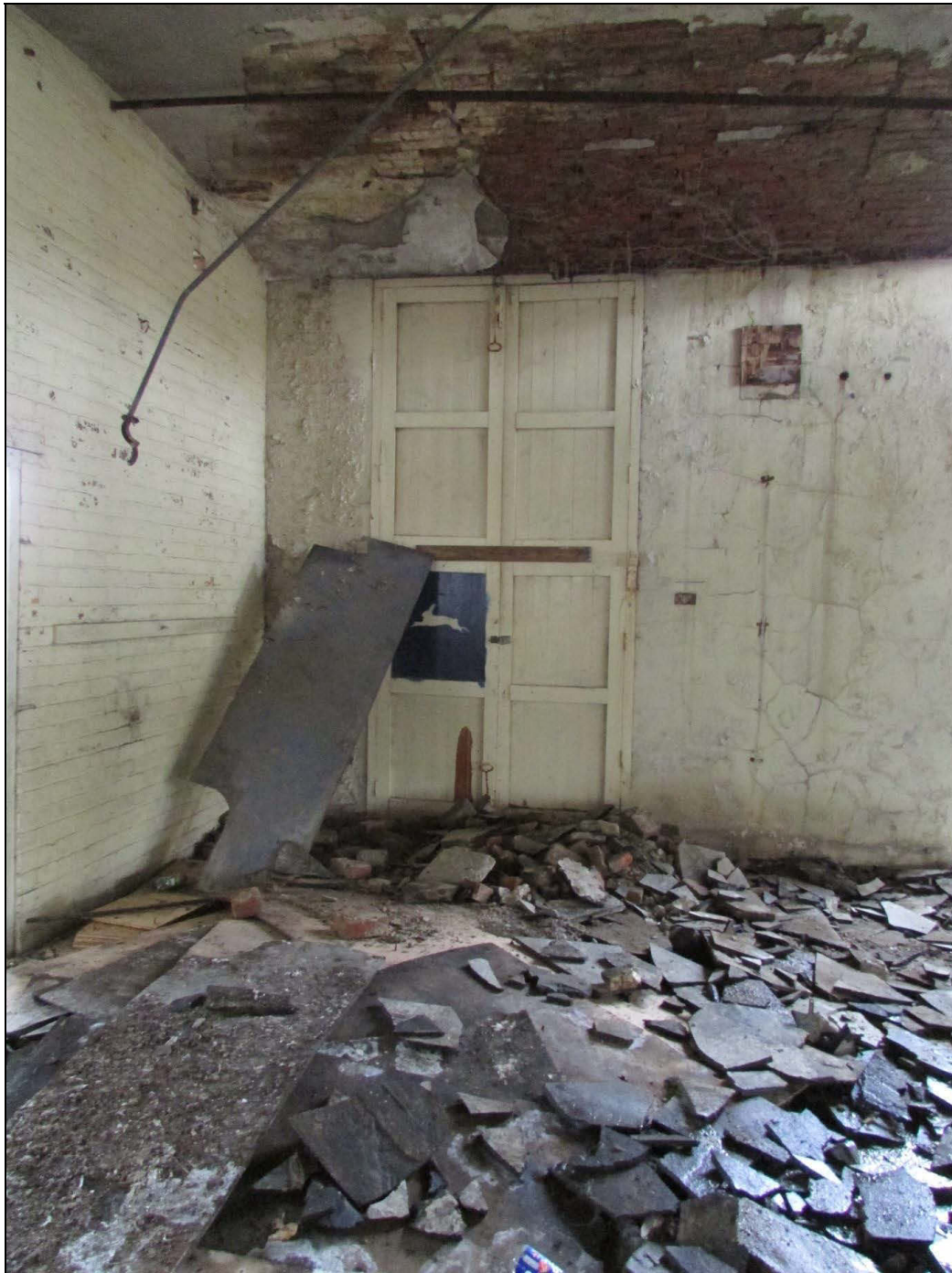
Plate 20 Wooden taking-in door visible immediately to the south of the later toilet block
