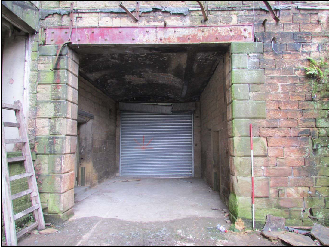
Plate 69 Entrance to covered walkway between the spinning mill and the office block, also showing a later RSJ and fixtures for a possible canopy above
