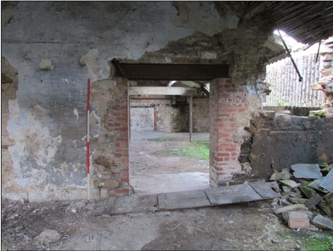
Plate 30 An inserted entrance into the engine house and position of robbed out top steady bracket (to the right)
