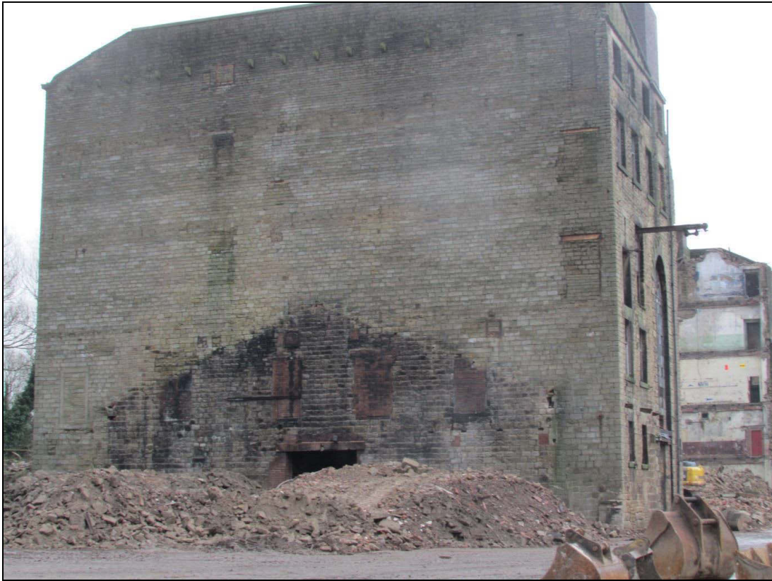
Plate 32 General view of the Engine House western elevation, after removal of the 20th century warehouse (its former position still visible)
