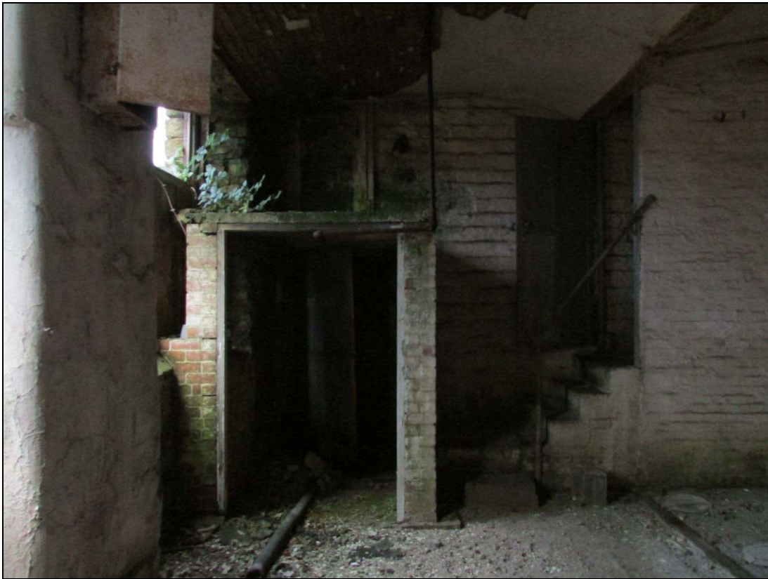
Plate 47 Later machine made brick divisions (including the stairs to the right) within the first-floor of the engine house
