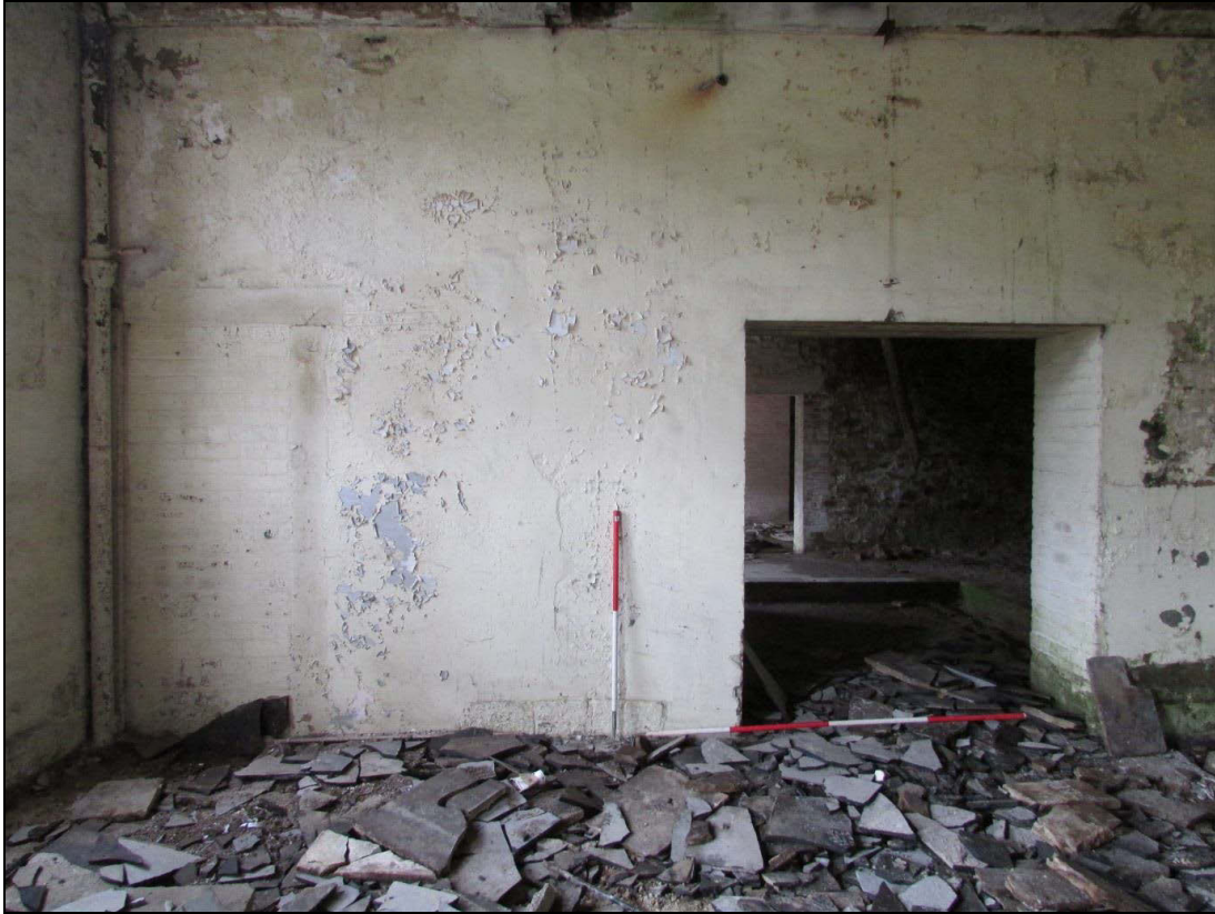
Plate 23 On the second-floor, the entrance on the right has been inserted at a later date, whilst the entrance to the left has been blocked
