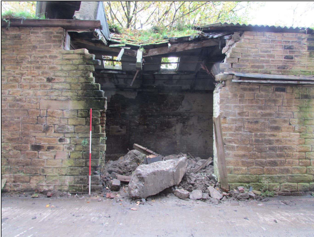
Plate 78 There appears to have been an entrance located here into the east shed, however roof collapse has damaged this area
