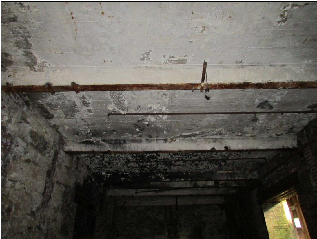
Plate 41 The flat ceiling of the engine house ground-floor, which is probably later in date
