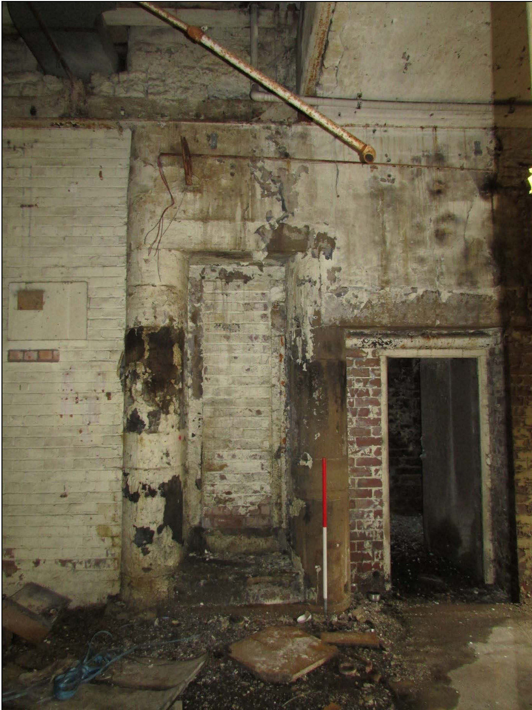
Plate 10 Blocked entrance into the former privy tower, with the later entrance to the lift shaft on the right, subsequently made smaller
