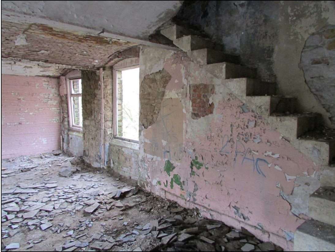
Plate 74 Later steps leading to the third-floor within the office block. Also visible beneath the plaster is the brickwork blocking one of the windows
