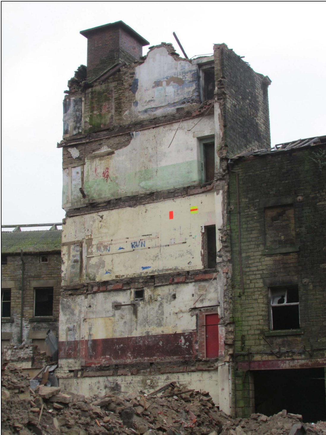
Plate 91 The demolition of the central part of the mill revealed the phasing of the lift shaft
