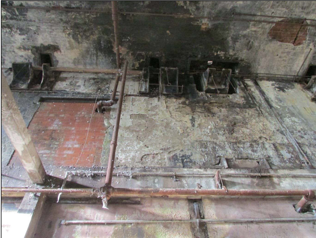
Plate 16 The bracket and aperture for the driveshaft is located to the right; a blocked entrance and two more brackets are shown to the left
