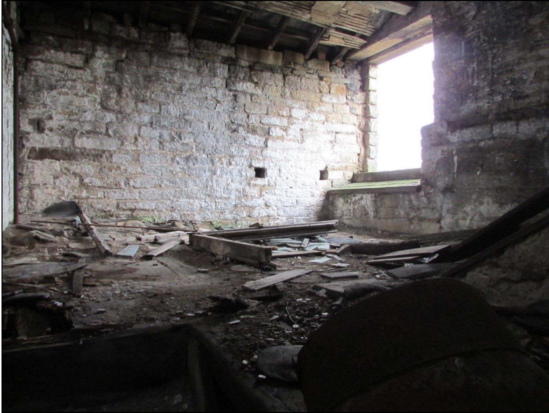
Plate 31 A small attic space located in the stair tower and accessed from the fourth-floor
