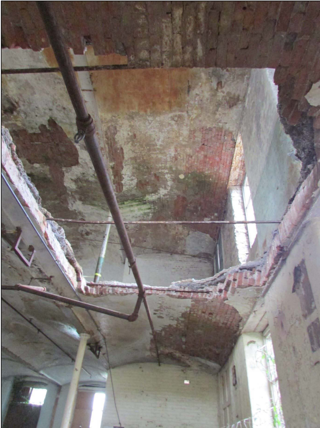
Plate 17 A small part of the second-floor ceiling had collapsed within the eastern part of the mill, exposing the metal tie-beams integral to the fireproof arches' structure
