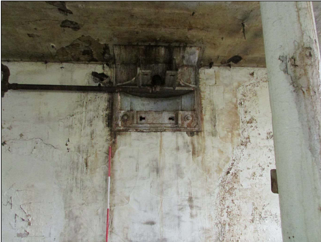
Plate 22 Metal bracket on the second-floor gearing wall to support the upright shaft
