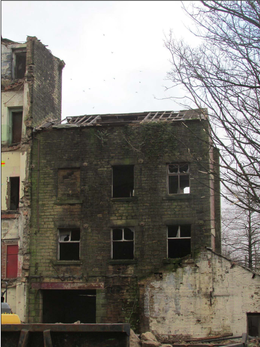
Plate 67 Western elevation of the office block, after the demolition of the sheds
