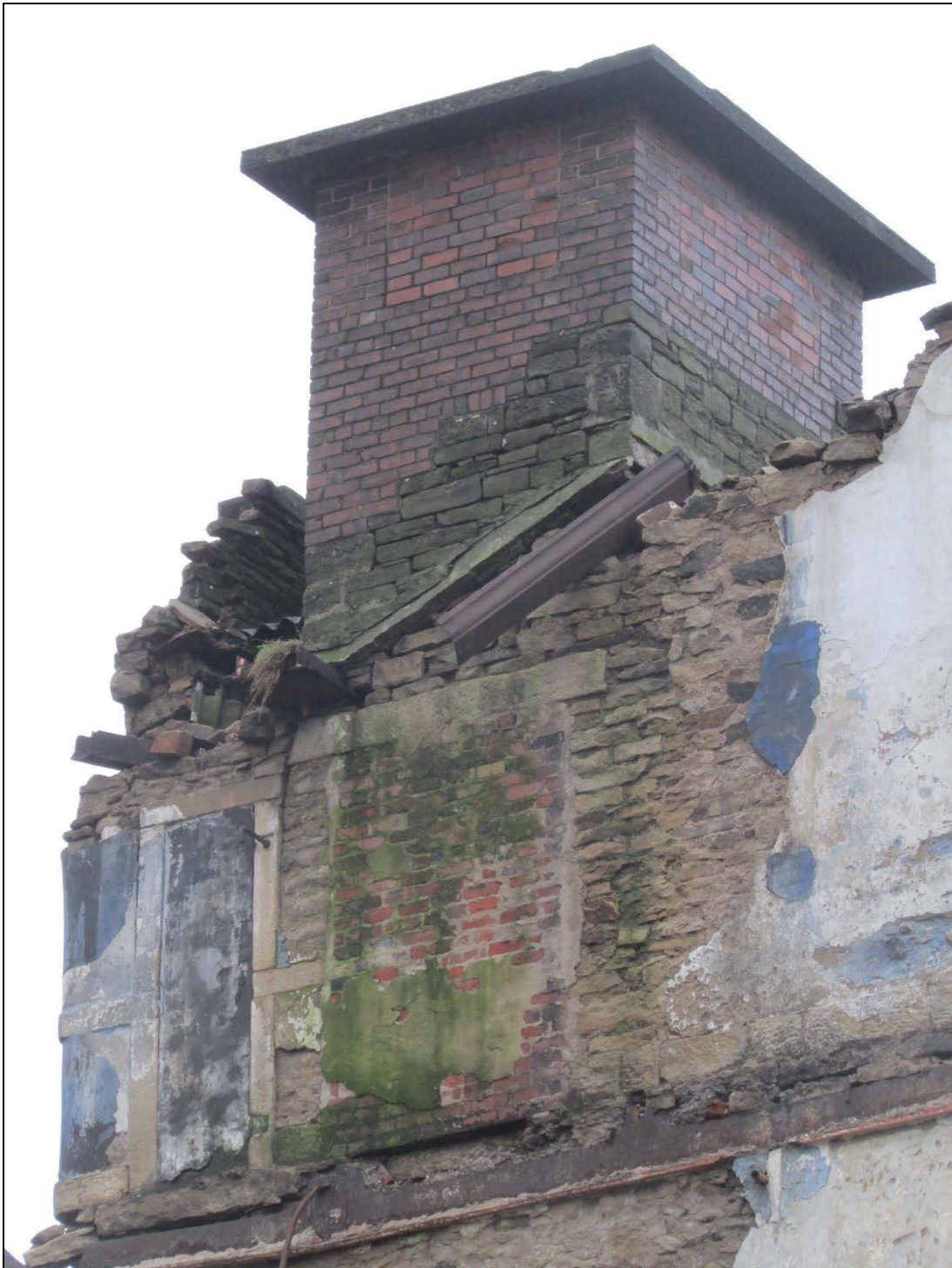
Plate 6 Close-up of the eastern lift shaft headgear shows the partial reconstruction in brick, as well as subsequent blocking of apertures
