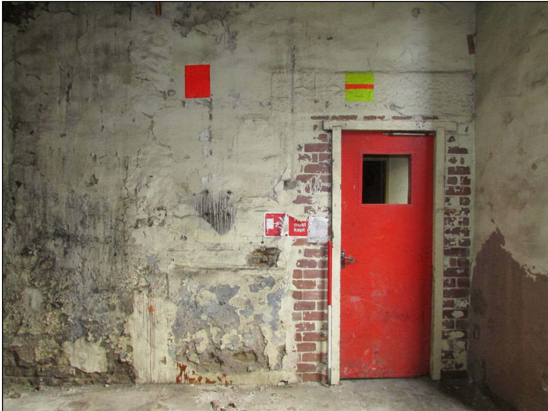
Plate 92 The entrance into the spinning mill from the stair tower, modified and made smaller
