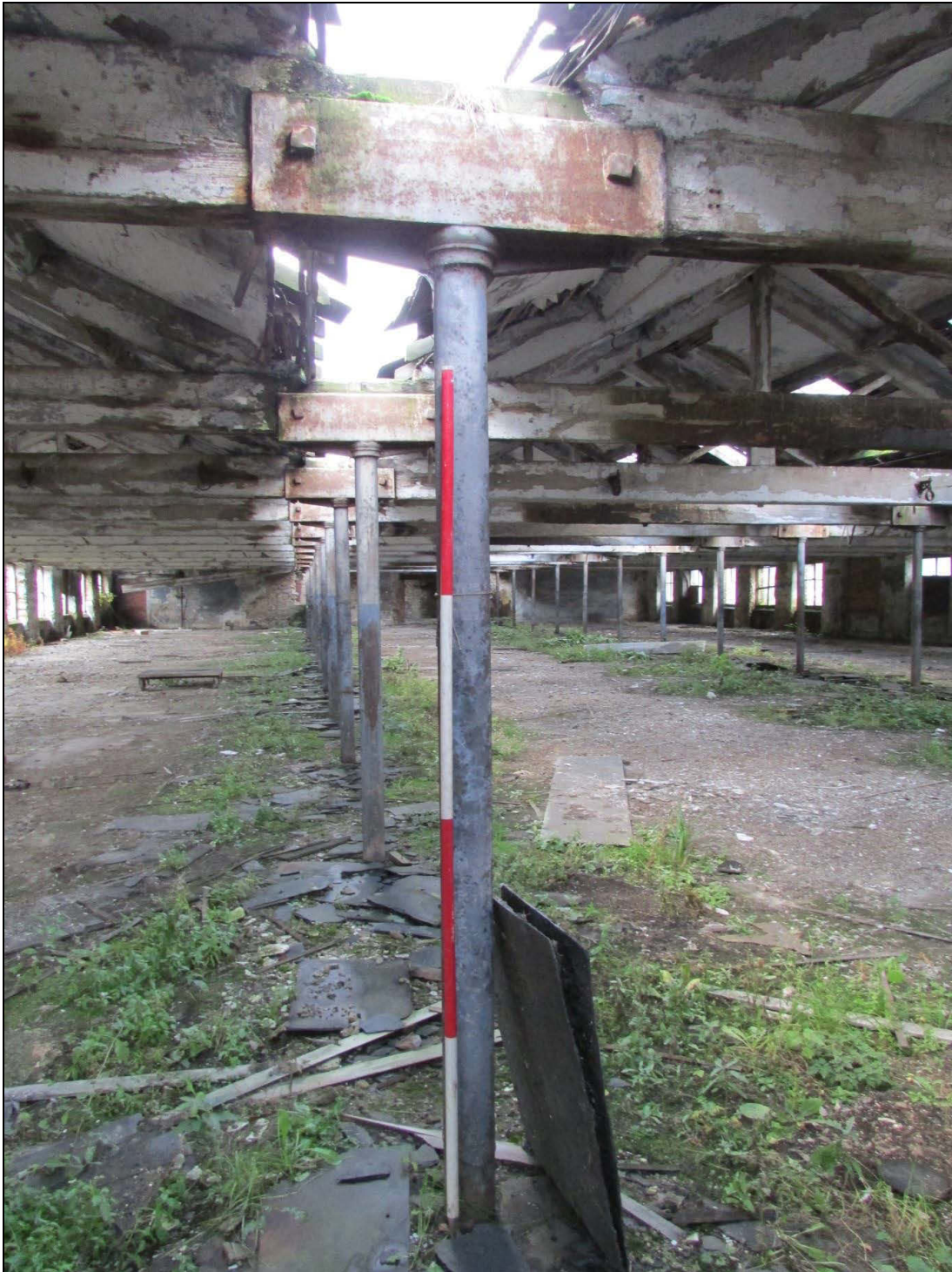
Plate 28 Detailed shot showing how the roof was supported using the cast iron columns
