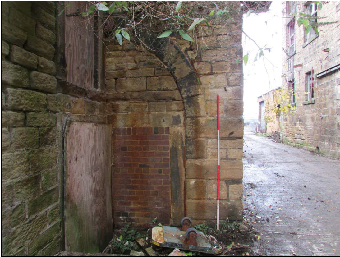
Plate 88 The eastern elevation of the west shed, with a former arched entrance with two phases of blocking evident
