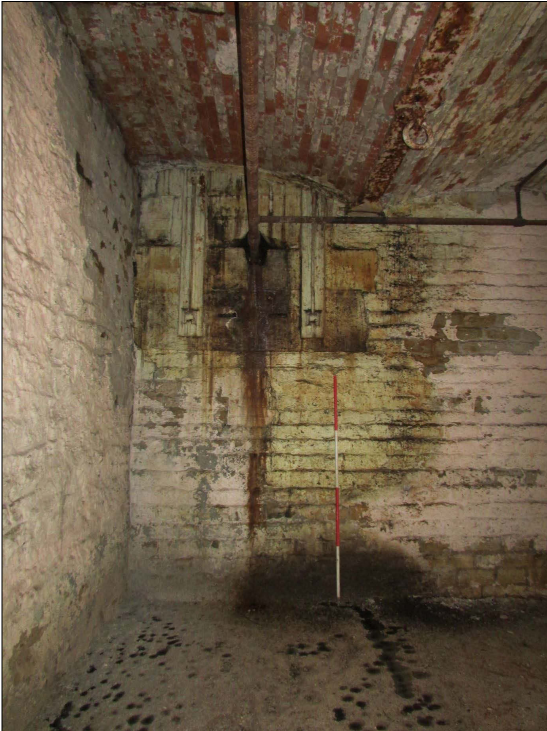
Plate 57 Original metal brackets supporting the power transmission system, later adapted for a sprinkler system.
