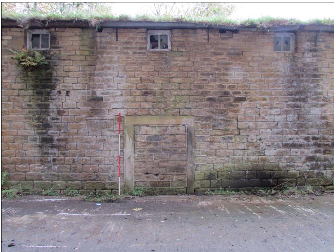
Plate 79 Blocked entrance in East Shed
