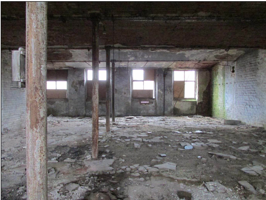
Plate 60 Instead of a dividing wall, the third-floor of the engine house had a run of axial columns supporting a fireproof ceiling
