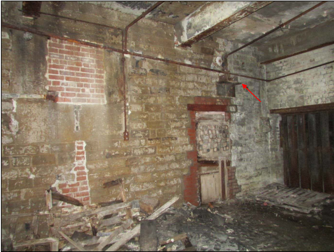
Plate 49 Another inserted doorway had been blocked subsequently with a mixture of unknown materials. An original engine fitting is visible above (arrowed)
