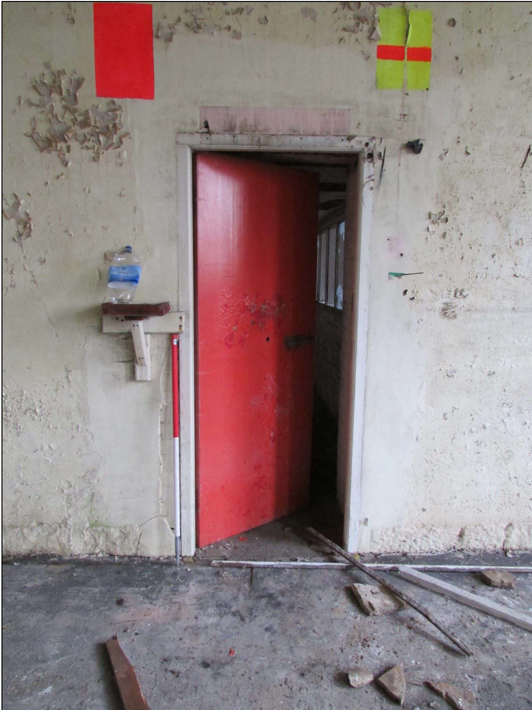
Plate 24 Later inserted entrance into the northern part of the engine house on the second-floor
