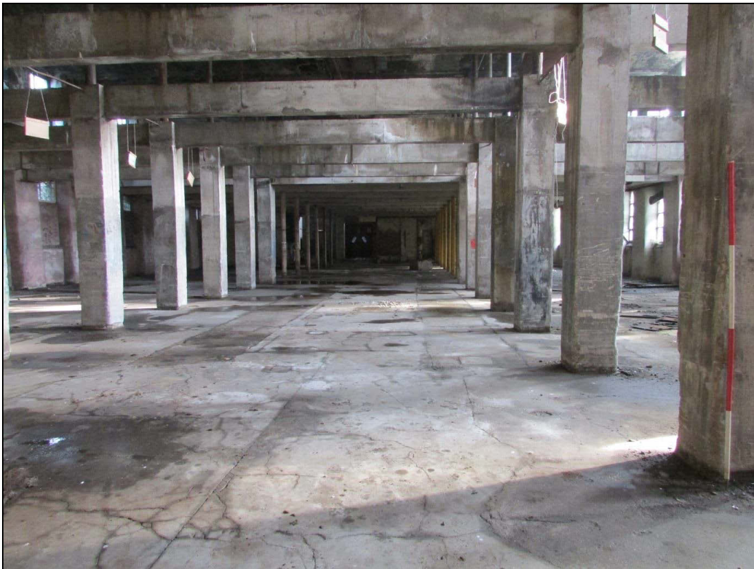
Plate 7 The iron columns at the western end of the mill were encased in concrete
