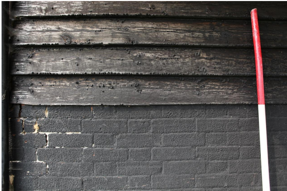
Illus. 8. A detail of the granary's heavily tarred eastern external brickwork and weatherboarding protected by the later implement shelter. There is some evidence of earlier red-ochre pigment beneath the tar.
