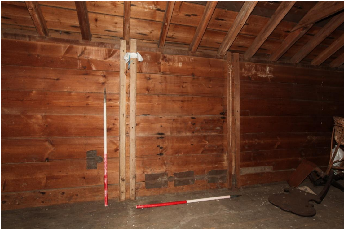
Illus. 14. A detail of the eastern loft interior showing the nailed patches of sheet tin to the deal boarding. The circular patch on the left appears to be the base of a tin can. A series of chalk tally marks are visible on the top board (see detail in illus. A2. 16).
