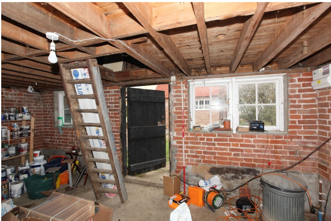
Illus. 10. The interior of the western ground-floor facade showing cement repairs to the cut brickwork on the right of the door. The windows also appear to cut the brickwork on the left and may have replaced smaller originals.
