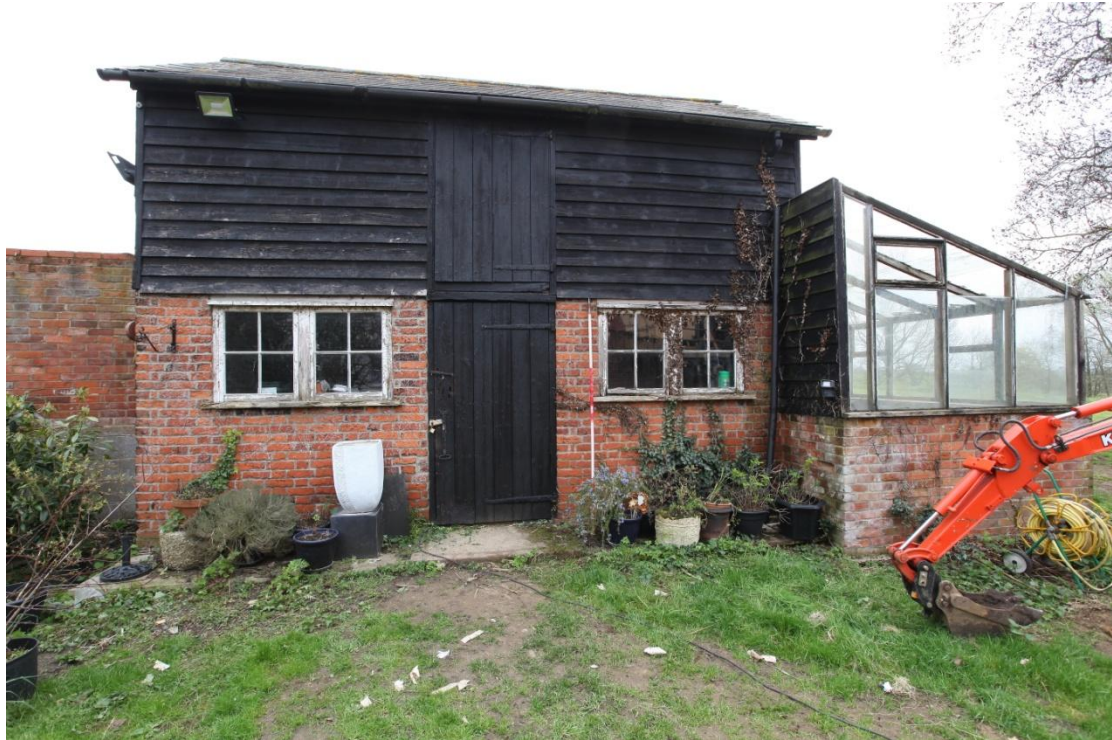
Illus. 5. The granary's western facade showing its red-brick lower storey and the central loading door of the weatherboarded loft. The ground-floor doorway is respected by closers (quarter bricks) to the right but its left-hand jamb cuts the brickwork suggesting it has been widened. The present windows date from the 20 th century and also interrupt the brickwork.
