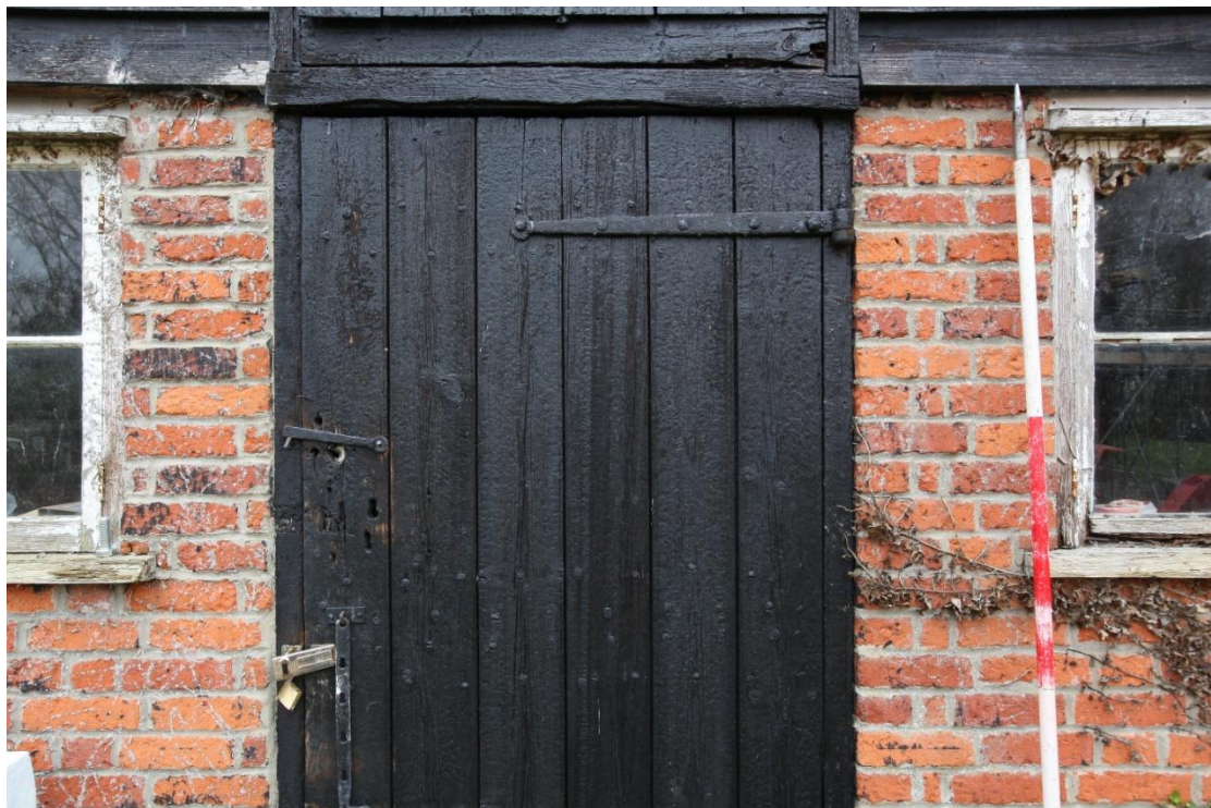
Illus. 6. A detail of the heavily tarred western entrance door with closers to the right and cut bricks to the left.
