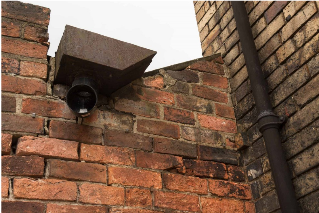
Figure 21. Part of the north end wall of the Drying Shed, showing iron rainwater goods, and cement-bonded brickwork in the gable abutting the wall of the Moulding Shop on the right.
