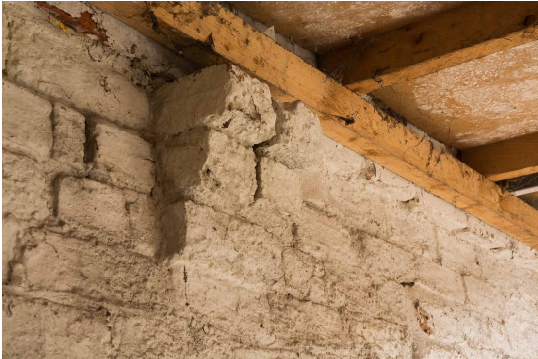
Figure 18. Corbel in the south wall of the Drying Shed that formerly carried a truss of the Saggar House roof.
