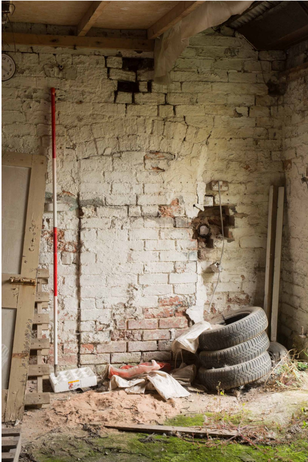
Figure 12. Blocked original doorway in the north gable end of the Drying Shed.
