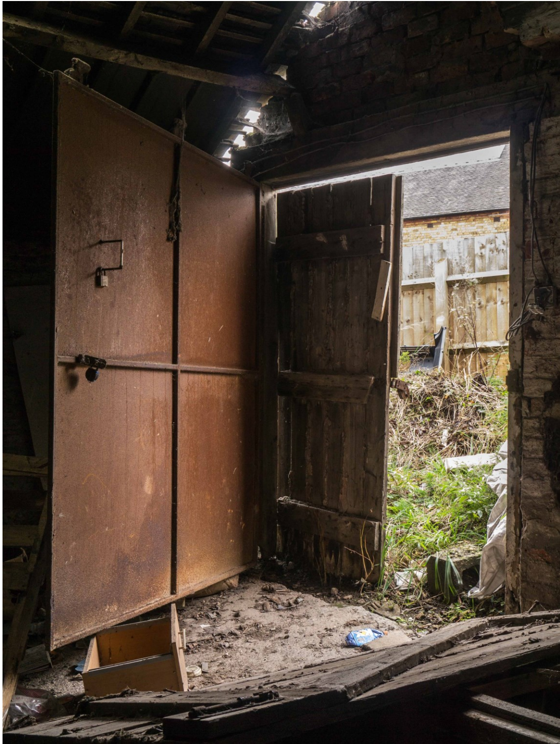
Figure 20. Steel door added to the Saggar House entrance. Hinges along the top show that it was salvaged from another site.
