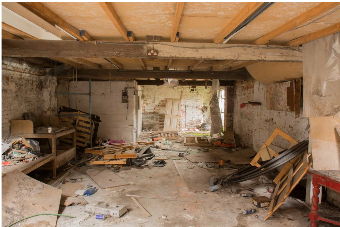
Figure 16. The interior of the Drying Shed, looking north. The blockwork partition is at the back on the left.
